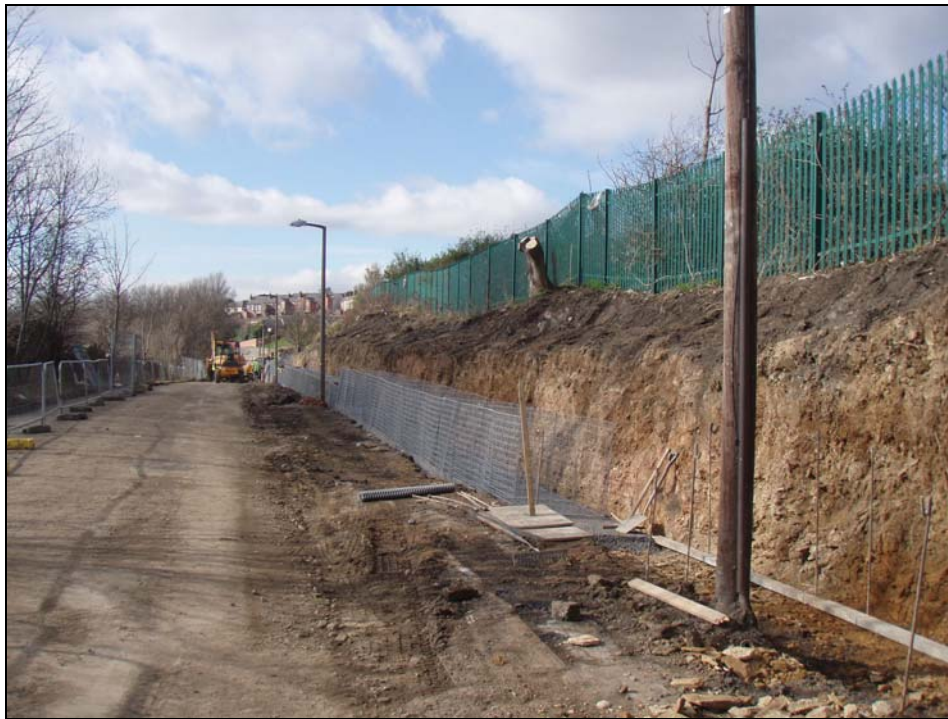
Fig. 8 View of work in progress. (The streetlights show the original width of the bank before it was excavated to accommodate the gabions).
