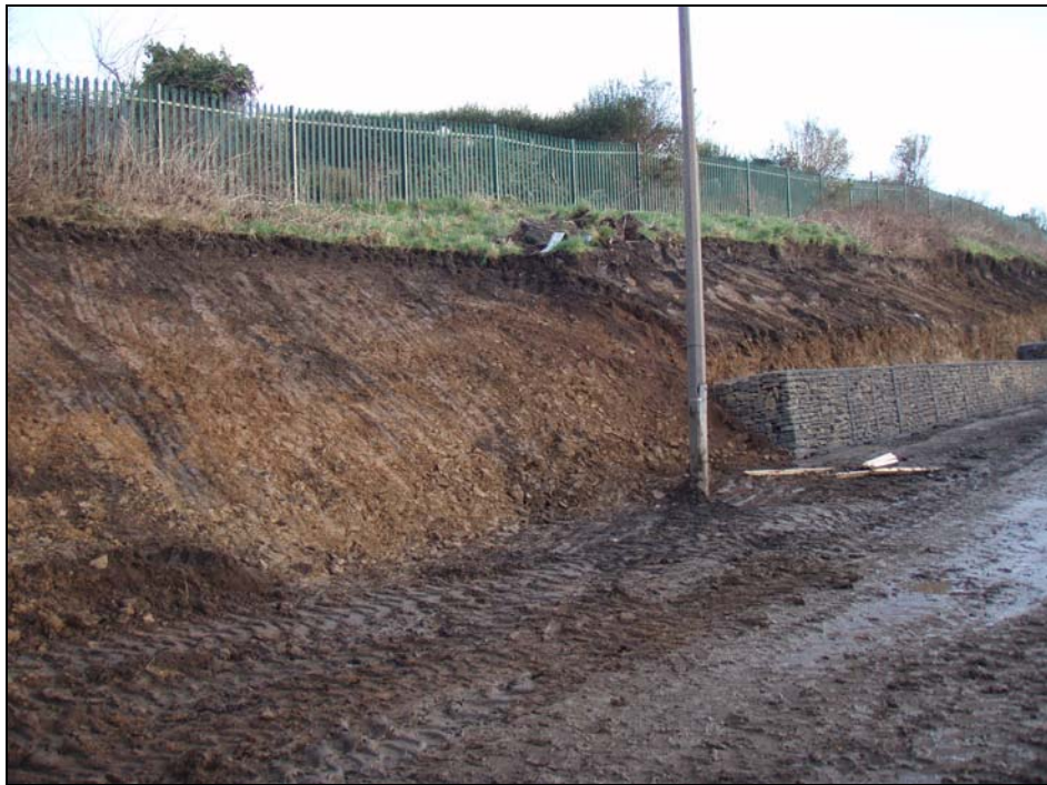
Fig. 9 View of the bank showing the end of the gabions and the start of the battered slope.
