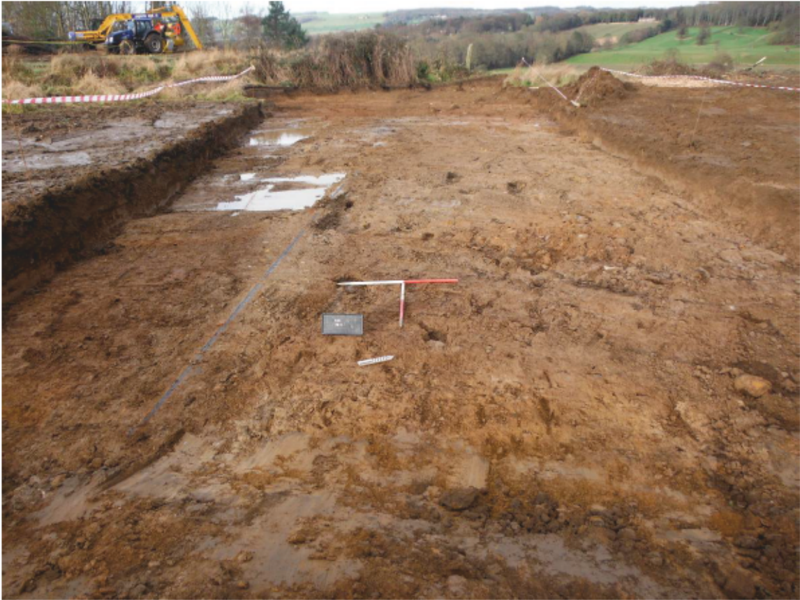
Figure 3. View looking north east of ramp access trench including foul pip trench F004 (scale= 2 x 1m).
