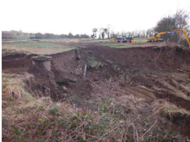
South-east facing view of landslip at the northern extent of the site.
