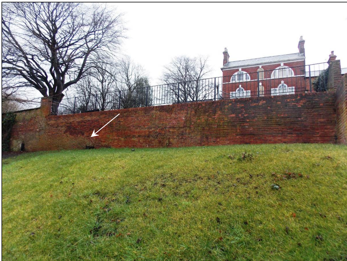
Figure 9: Retaining wall of the Apple Store with evidence of rebuilt brickwork (arrow).
