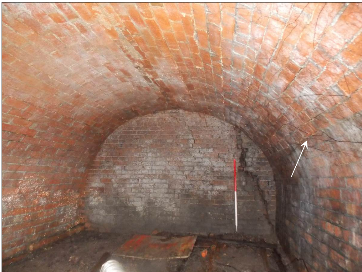
Figure 19: Construction joint/break (arrow) within the north-eastern wall (scale 1m).
