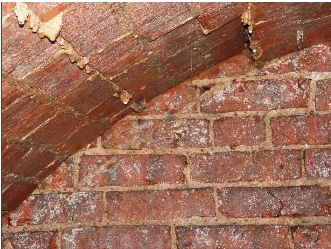
Figure 21: Detail of dislodged arched section.
