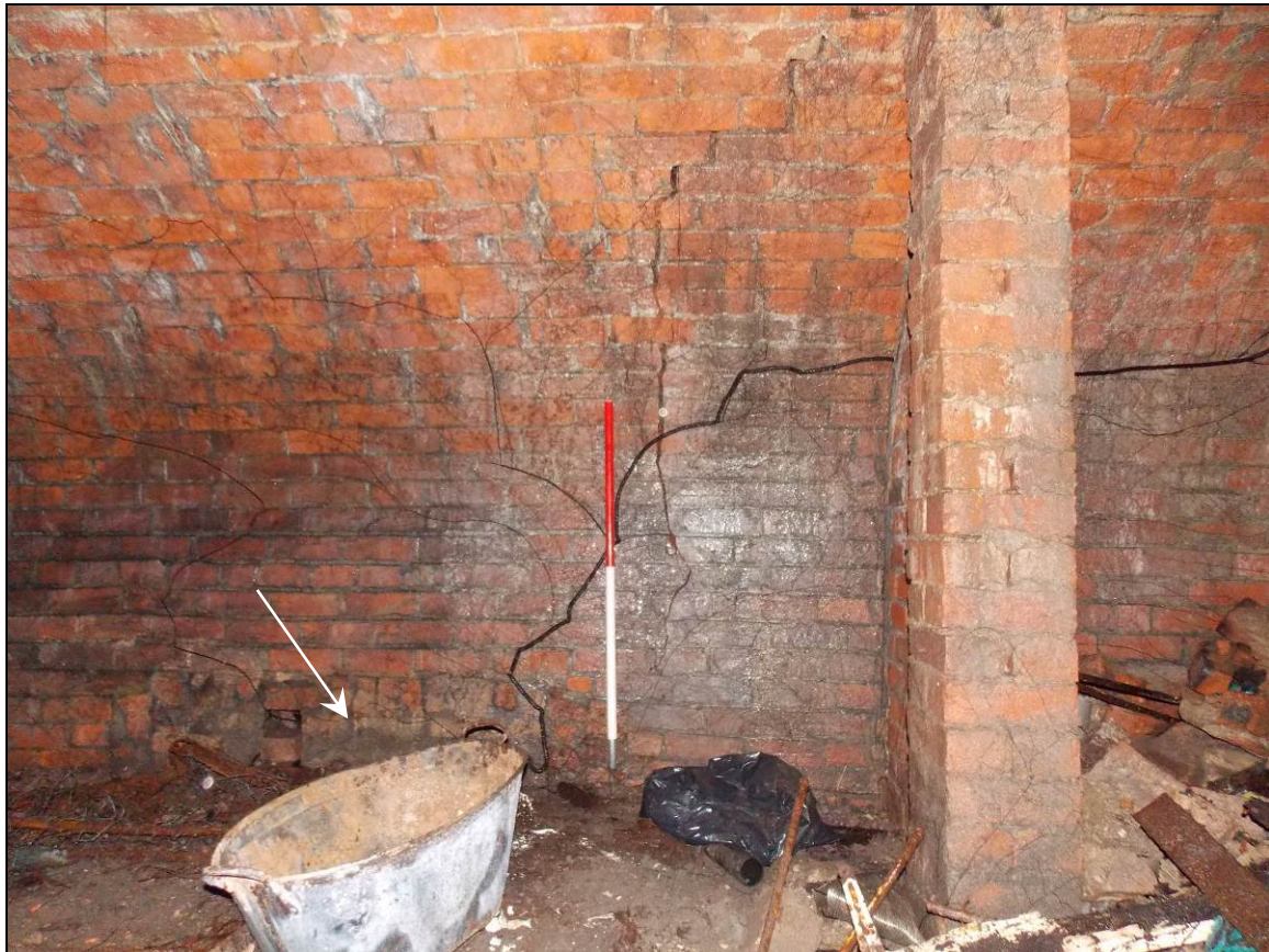
Figure 18: Bricked-up former opening (arrow) within the lower section of the north-eastern wall (scale 1m).
