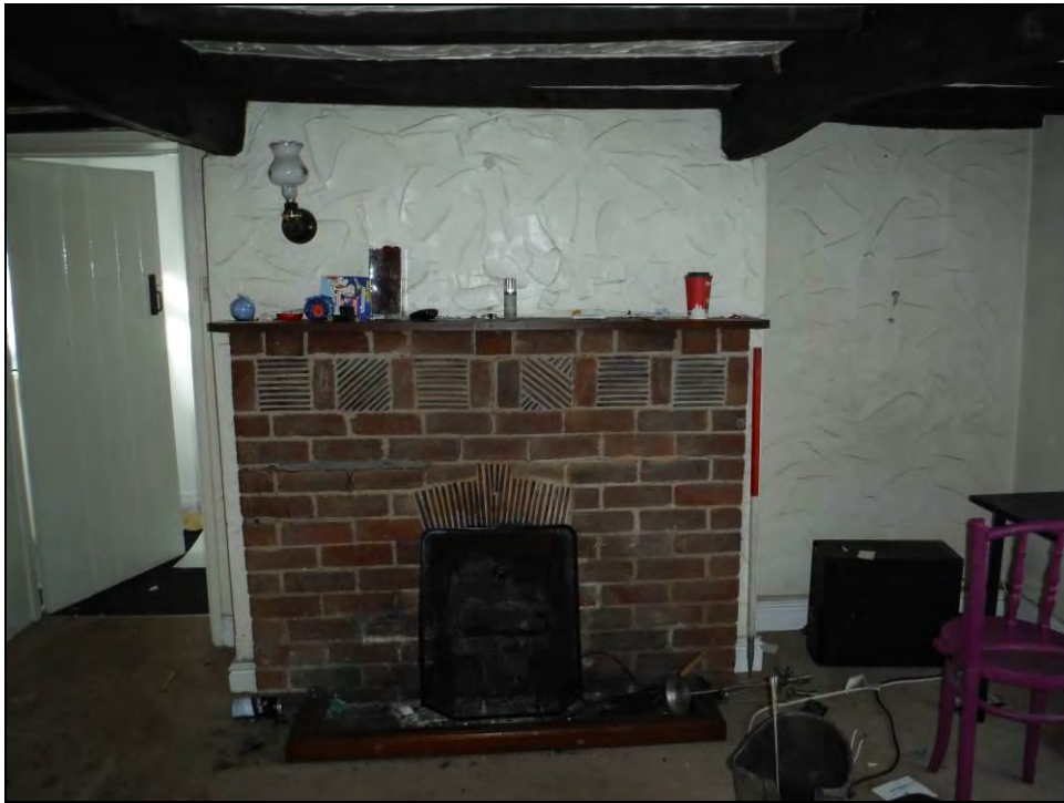
Figure 37. North-west wall of Room G5 showing doorway communicating with Room G7 and the brick-built fireplace (scale = 1 x 1m).
