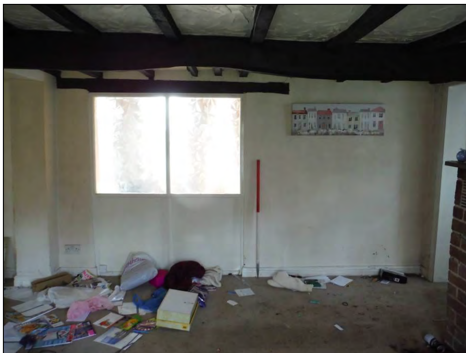
Figure 35. South-west wall of Room G5. Note the timber lintel above the part-glazed partition, demarcating a pre-existing door opening (scale = 1 x 1m).
