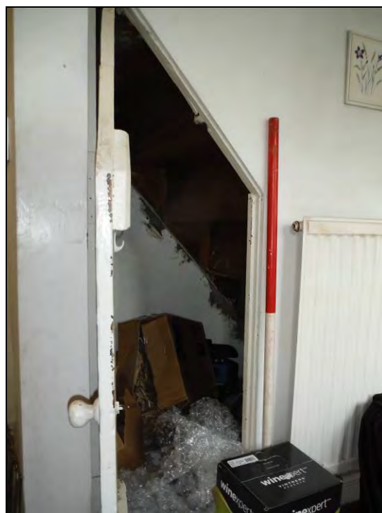
Figure 25. Understairs cupboard at the northern extent of Room G3 (scale = 1 x 1m).
