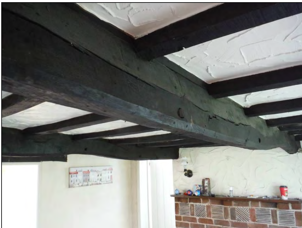
Figure 38. Detail of the binder beams and floor joists projecting from the ceiling of Room G5.
