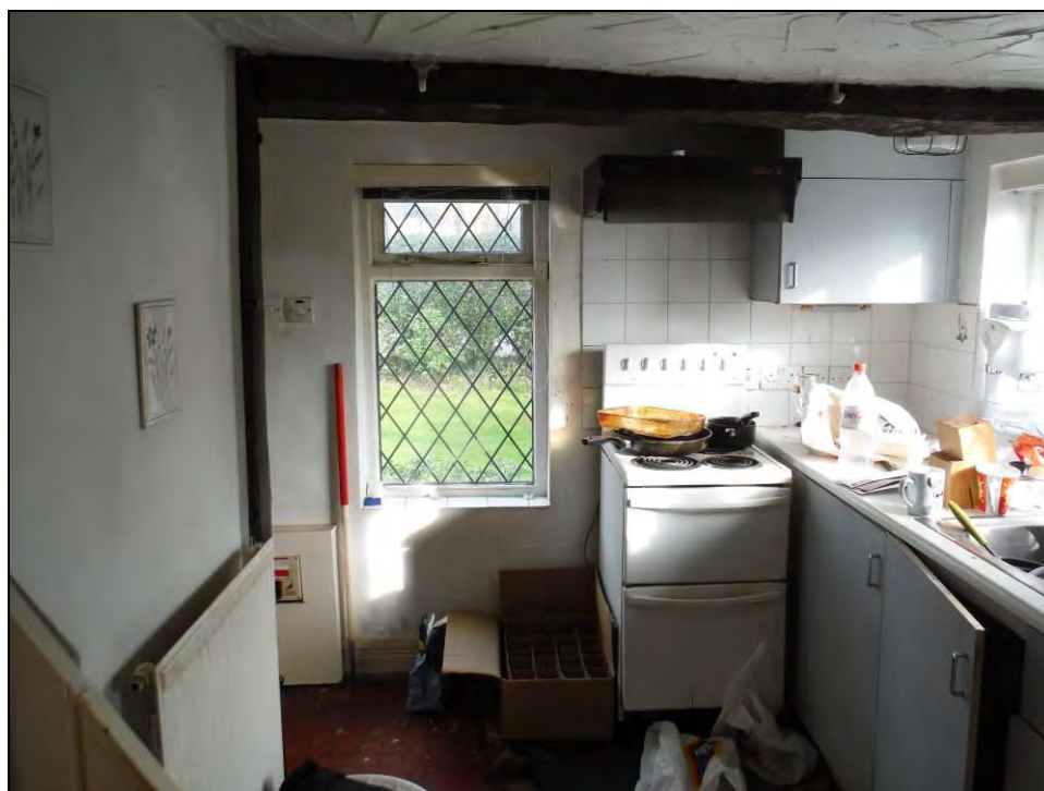
Figure 26. North-east facing view of Room G3. Note the hooks on the south-west side of the binder beam in the ceiling (scale = 1 x 1m).
