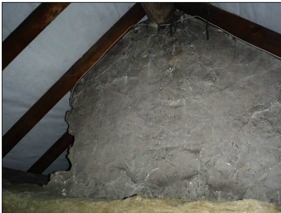
Figure 59. North-west face of the brick-built partition wall rising through the attic space from Rooms F1 and F3. Note the position of the ridge-purlin seated against the wall.
