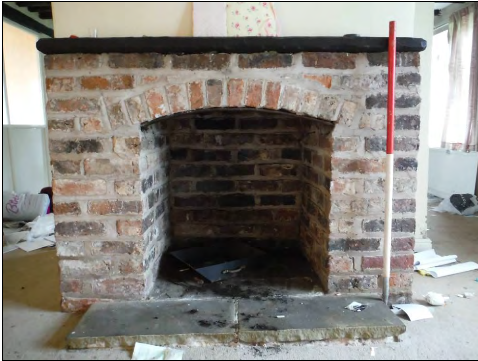
Figure 29. Fireplace and chimney breast projecting from the north-west wall of Room G4 (scale = 1 x 1m).
