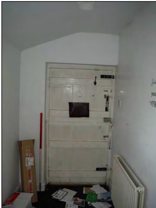
Figure 41. North-east wall of Room G7 with front entrance doorway (scale = 1 x 1m).
