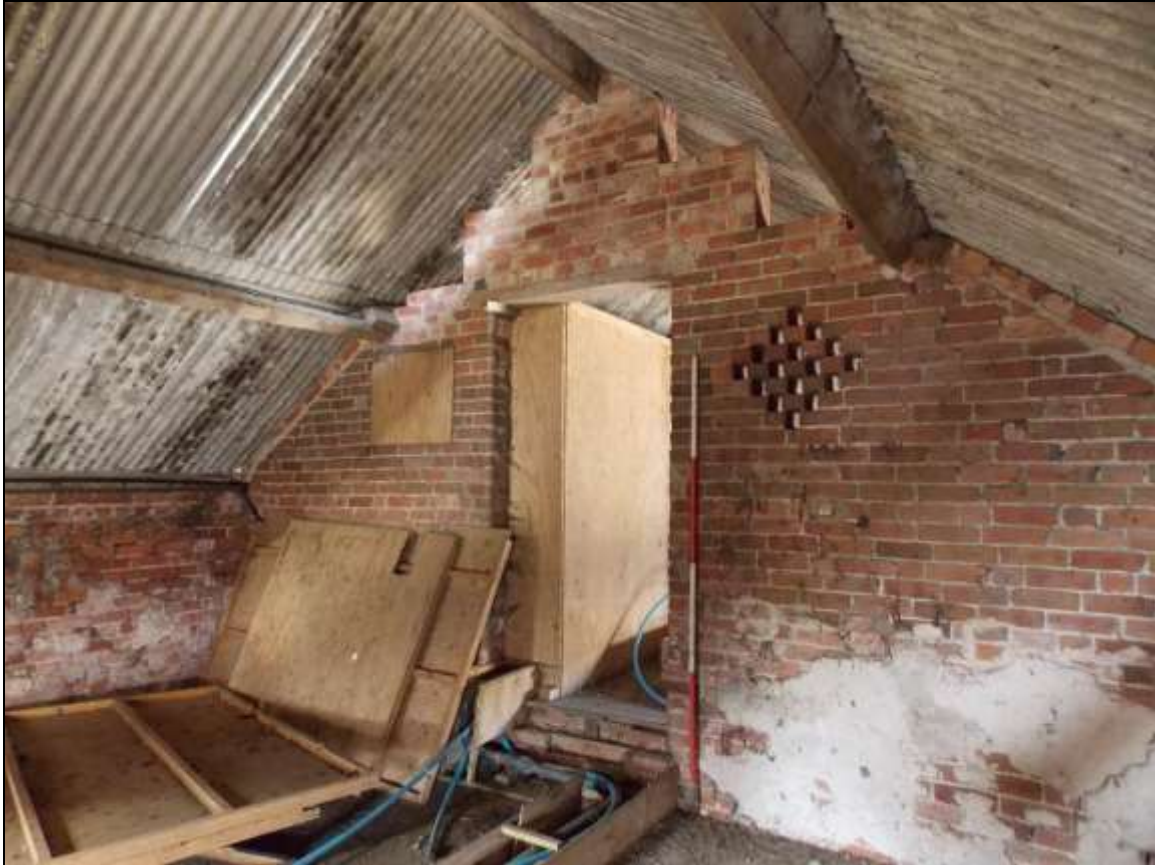
Plate 37: Outer face of gable wall viewed from the adjacent Building C, looking north-west (scale 2m).
