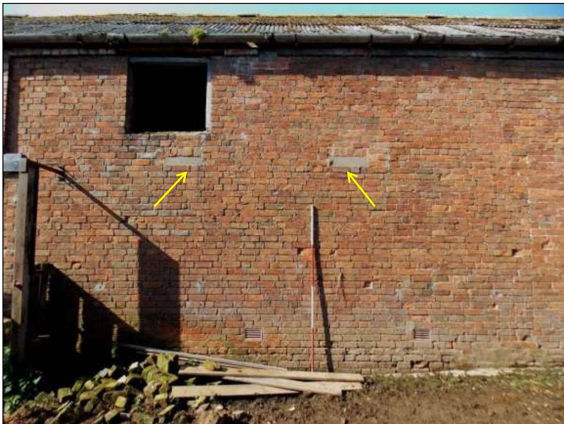
Plate 27: Detail of north-eastern wall with inserted concrete pads (arrows) for internal RSJ (scale 2m).
