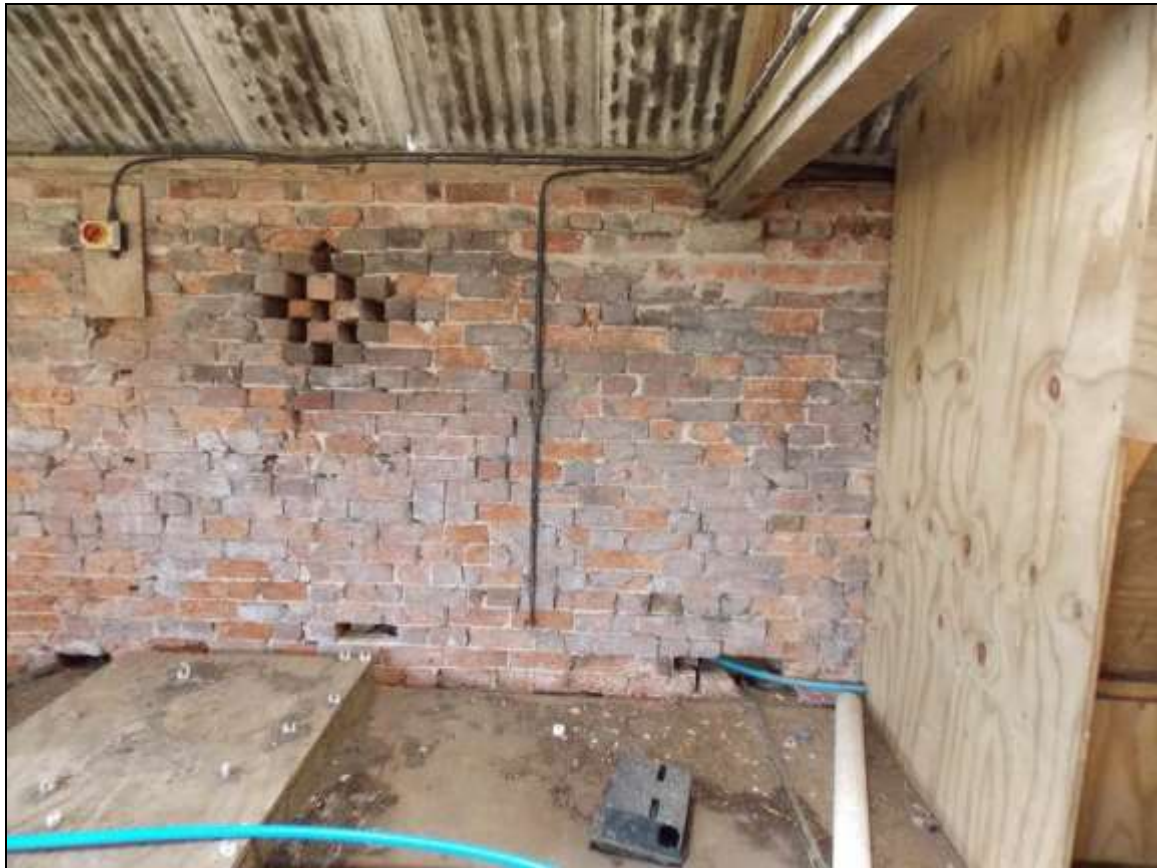
Plate 55: Detail of primary brickwork with vent and later bricks supporting the roof structure.
