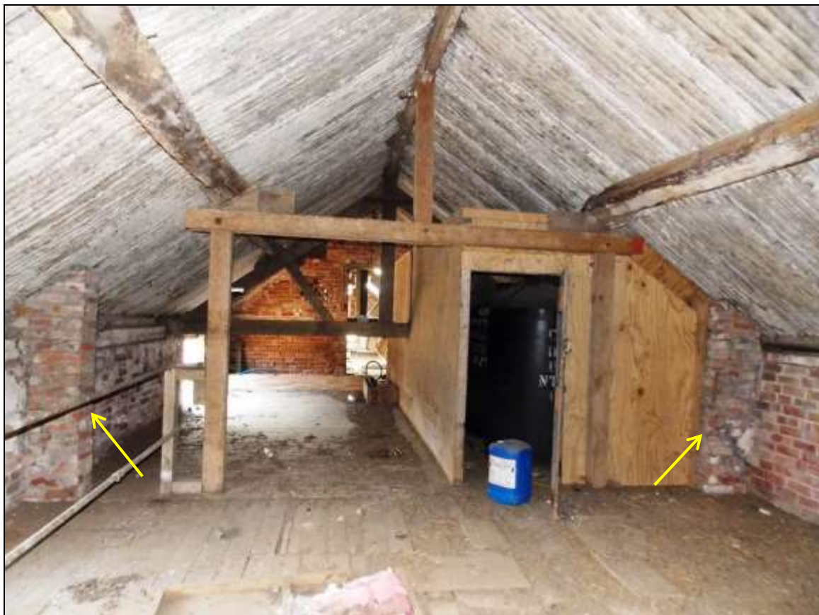
Plate 24: Loft storey with remnants of former gable wall of the adjacent Building C (arrows).
