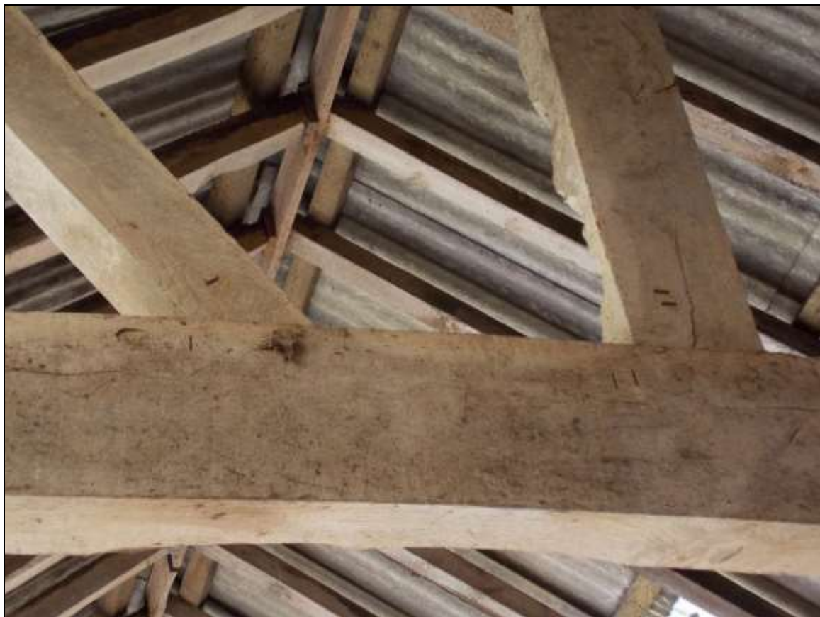
Plate 79: Upper face of truss with peg's heads and associated carpenter's assembly marks.
