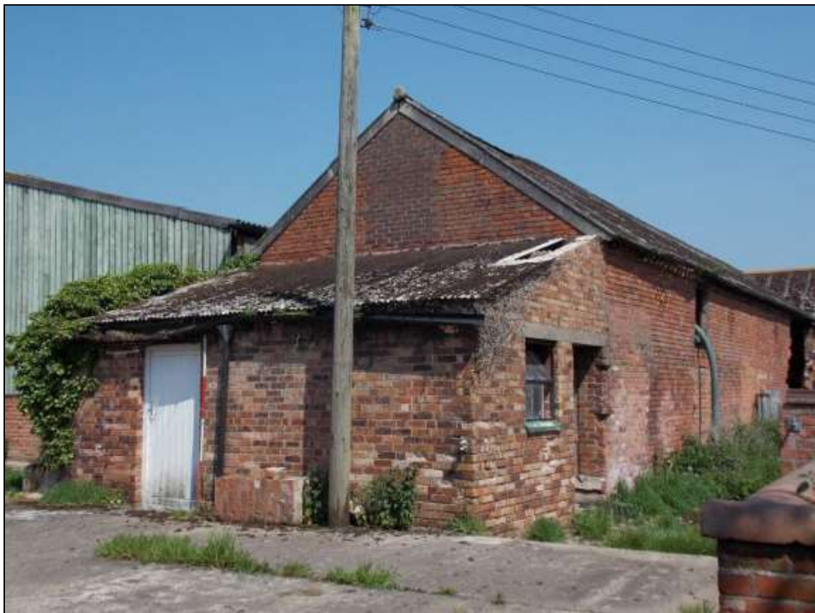
Plate 62: Gable wall of Building F and later lean-to extension Building I, looking north-east (scale 2m).
