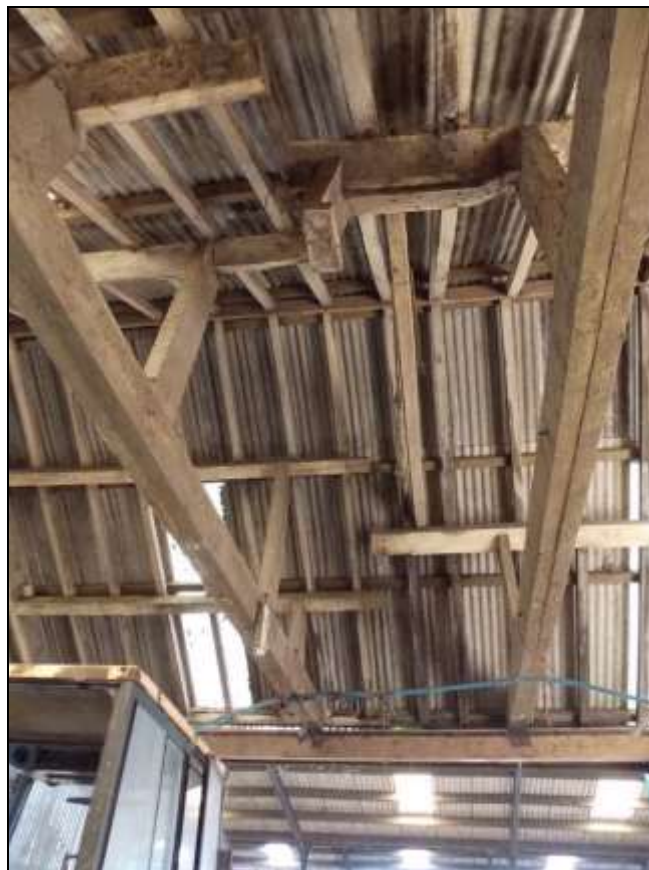
Plate 77: Detail of improvised trusses supporting the edges of side purlins of Buildings F and G.
