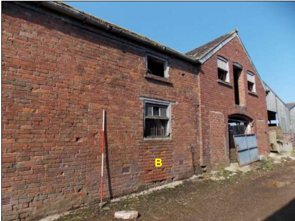
Plate 16: North-eastern wall of Building B along the central lane of the farm (scale 2m).
