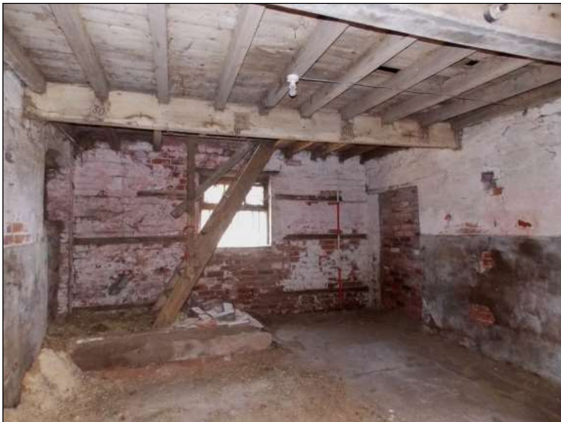
Plate 20: Ground floor with fixed timber ladder for the upper storey, looking north-east (scale 2m).
