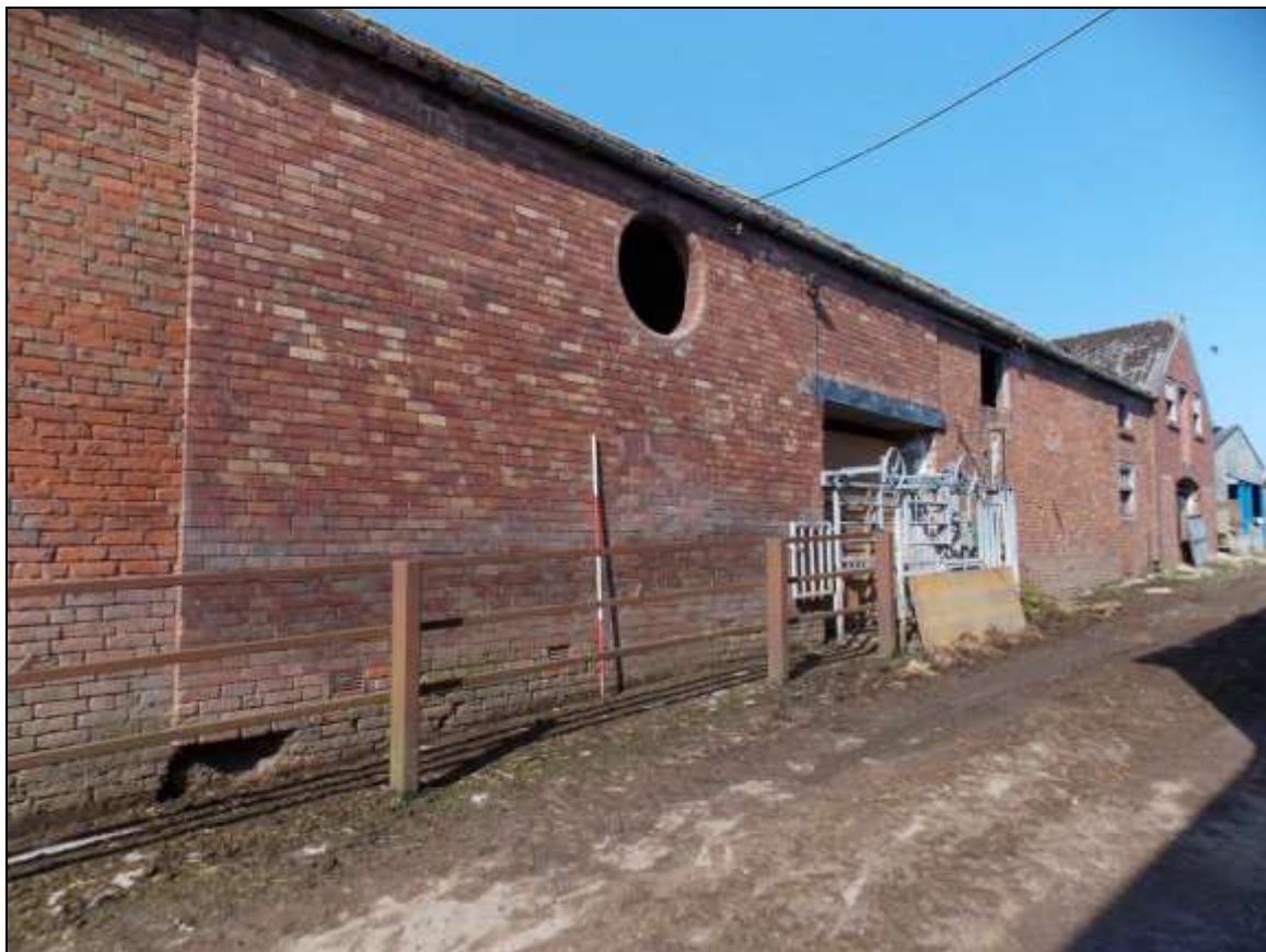
Plate 43: Refaced brickwork within the north-west side of the north-eastern elevation (scale 2m).
