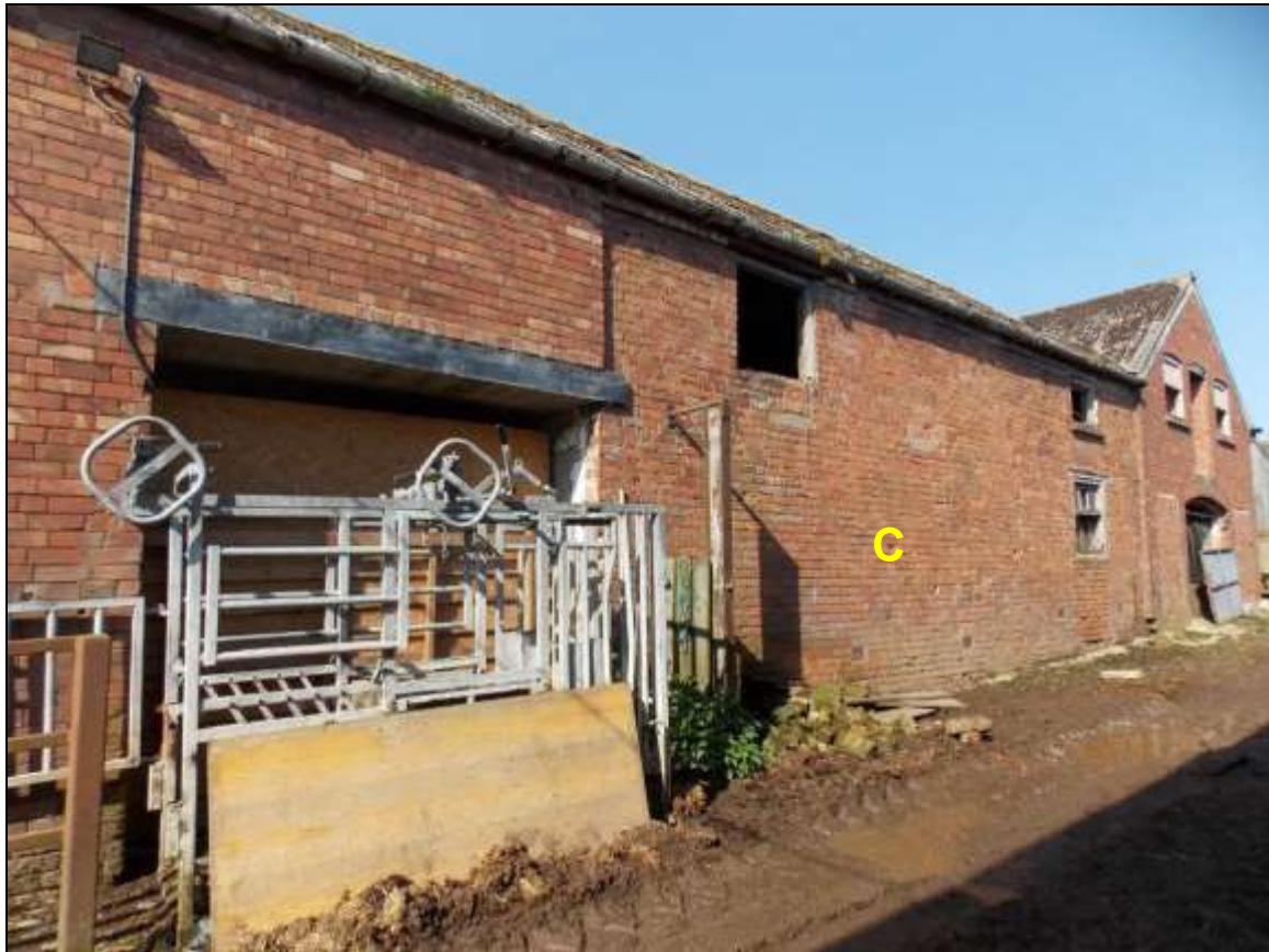
Plate 26: North-eastern wall of Building C along the central lane of the farm (scale 2m).
