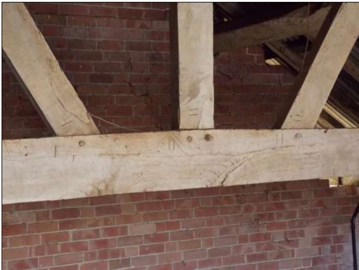
Plate 15: Upper face of truss with peg's heads and associated carpenter's assembly marks.
