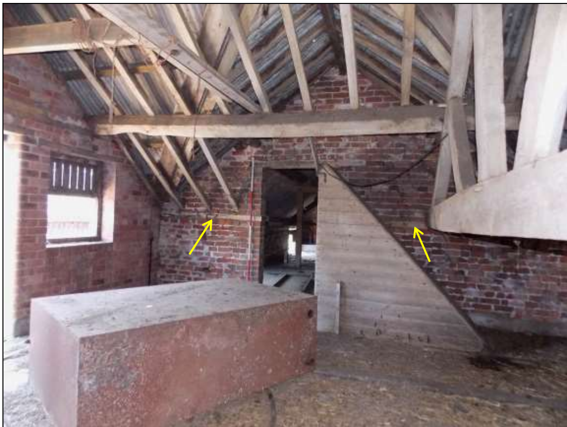
Plate 13: Primary wall plate (arrows) within the gable wall dividing Buildings A and G (scale 2m).
