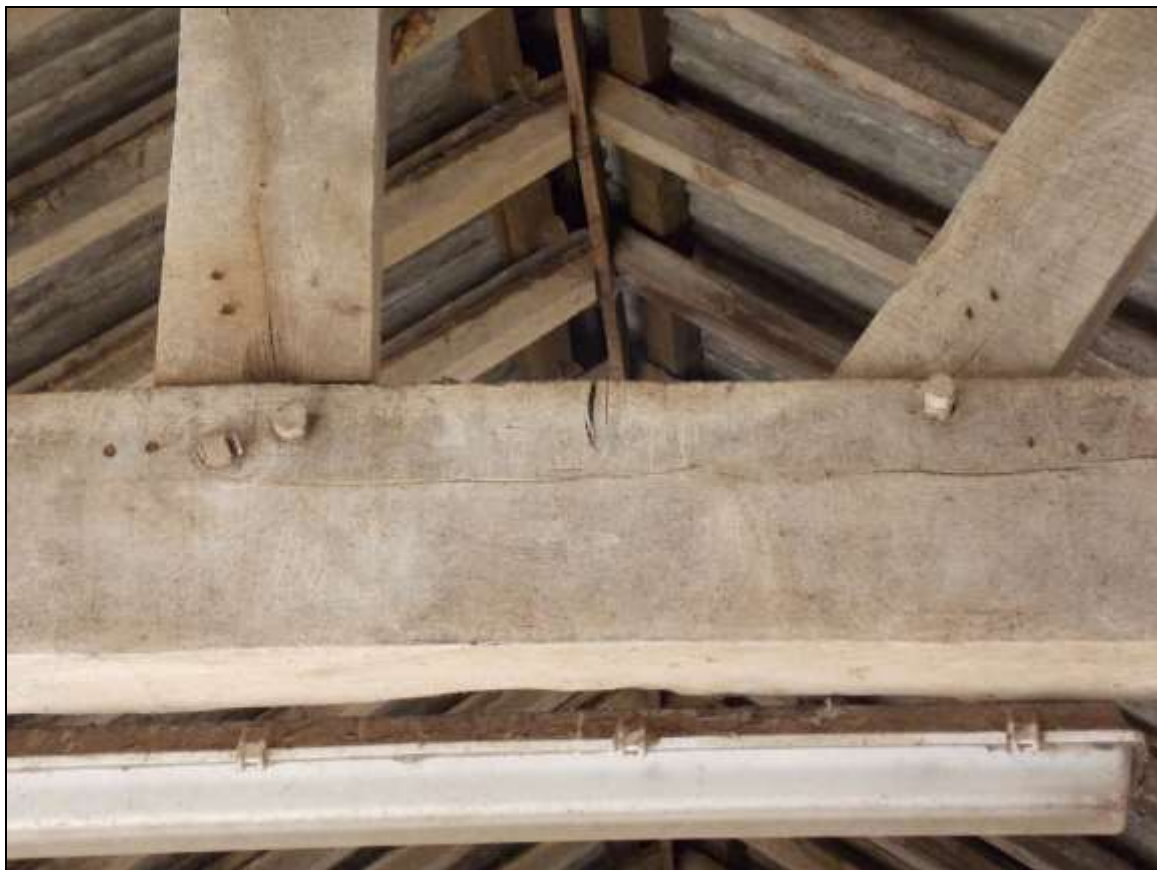
Plate 81: Upper face of truss with peg's heads and associated carpenter's assembly marks.
