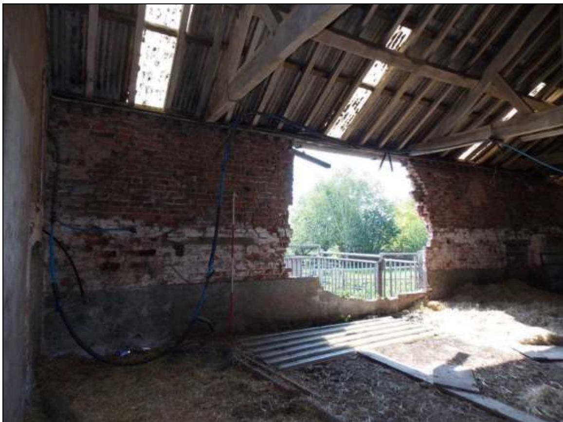
Plate 75: Internal view of Building G with partially demolished wall, looking south-east (scale 2m).
