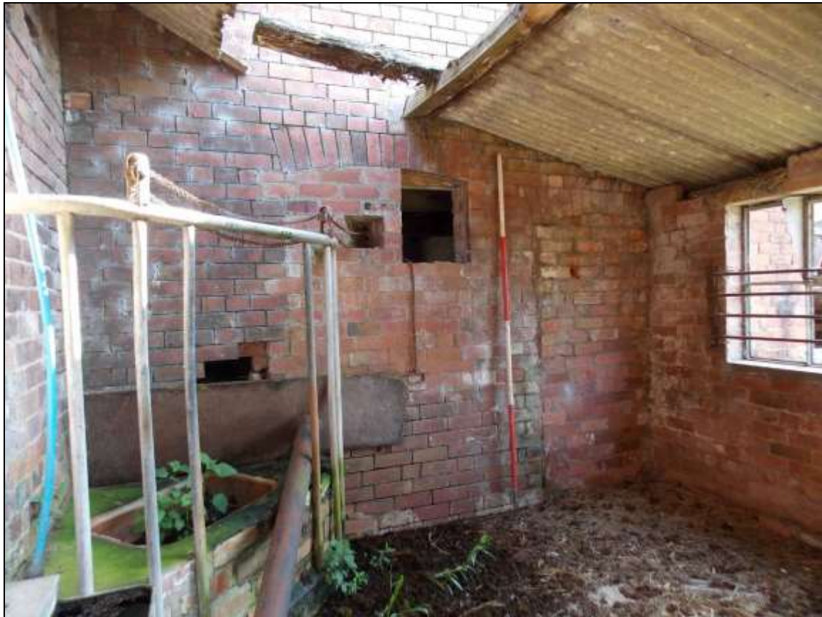
Plate 18: South-western wall of Building B, viewed from inside Building H (scale 2m).
