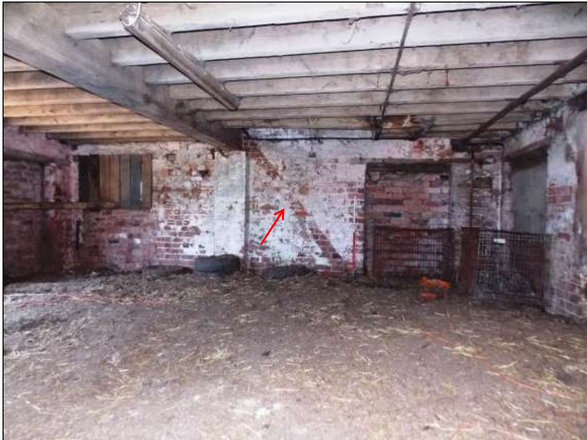
Plate 10: Scar of former staircase (arrow) against the south-eastern wall, looking north-east (scale 1m).
