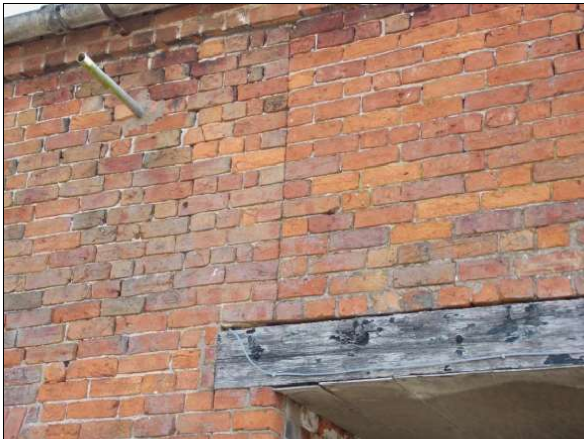
Plate 31: Detail of vertical construction joint between Buildings C and D, looking north-east.
