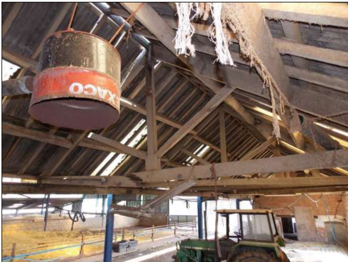
Plate 67: South-western truss with cracked tie-beam, looking north-east.
