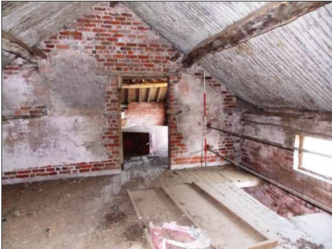
Plate 25: Loft storey with inserted doorway to Building A, looking north-west (scale 2m).
