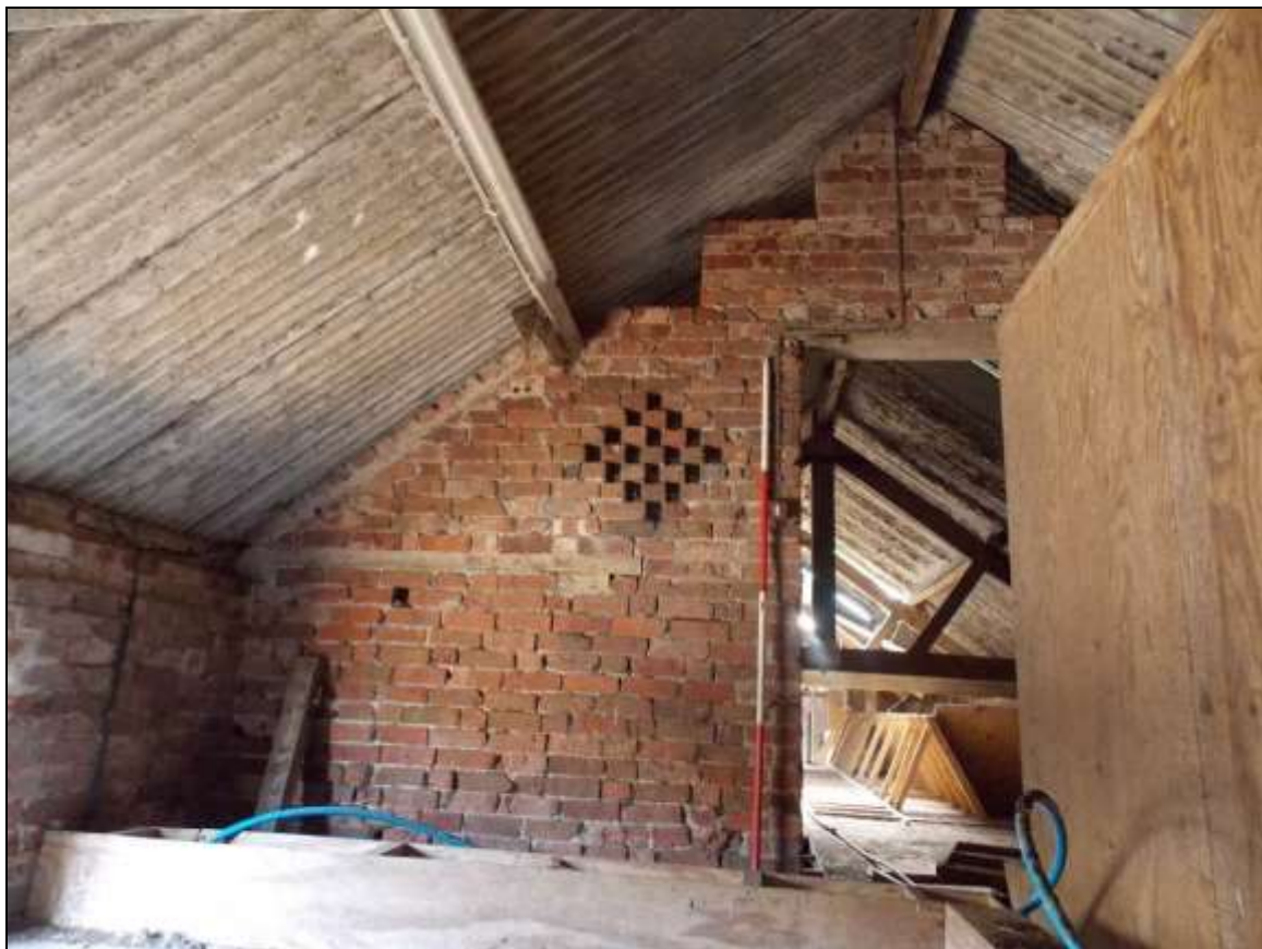
Plate 36: Loft storey looking towards the gable wall of the adjacent Building D (scale 2m).
