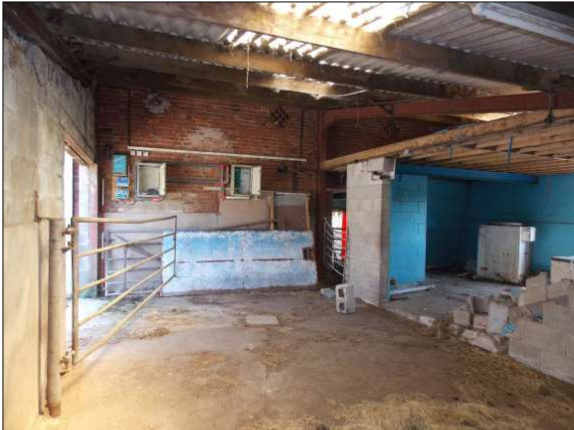
Plate 46: South-western elevation with diamond-shaped vents viewed from inside Building E (scale 2m).
