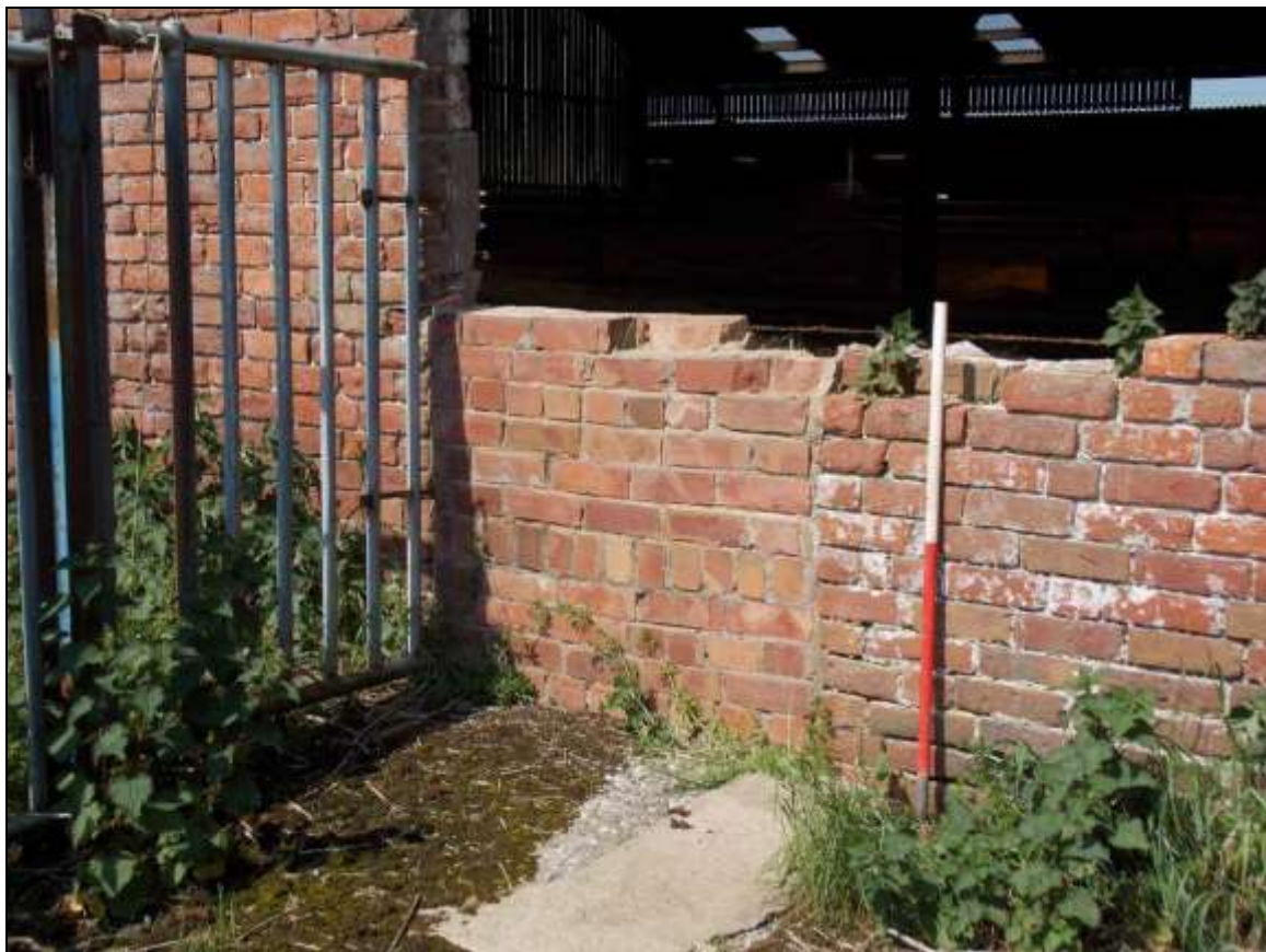
Plate 72: Detail of the remains of a blocked-up doorway, looking north-west (scale 1m).
