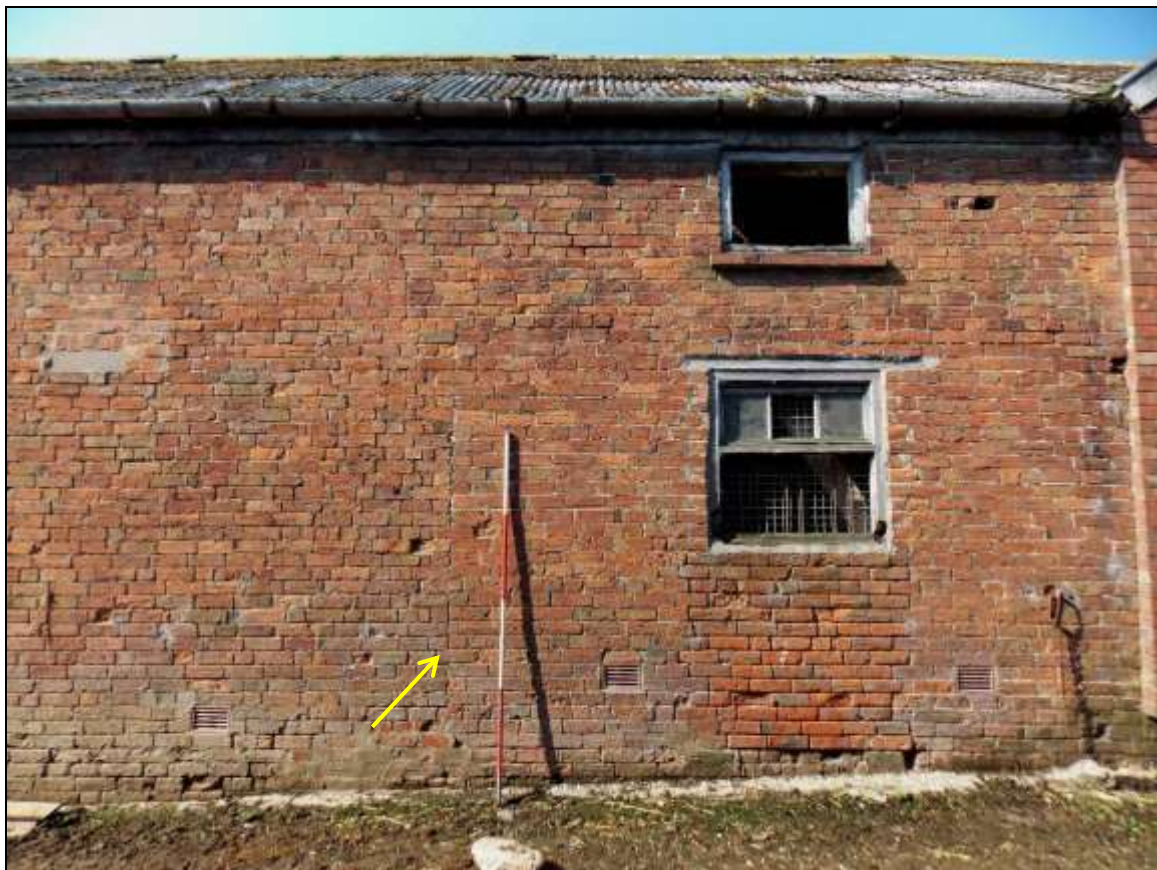
Plate 17: Vertical construction joint (arrow) between Buildings B and C, looking south-west (scale 2m).
