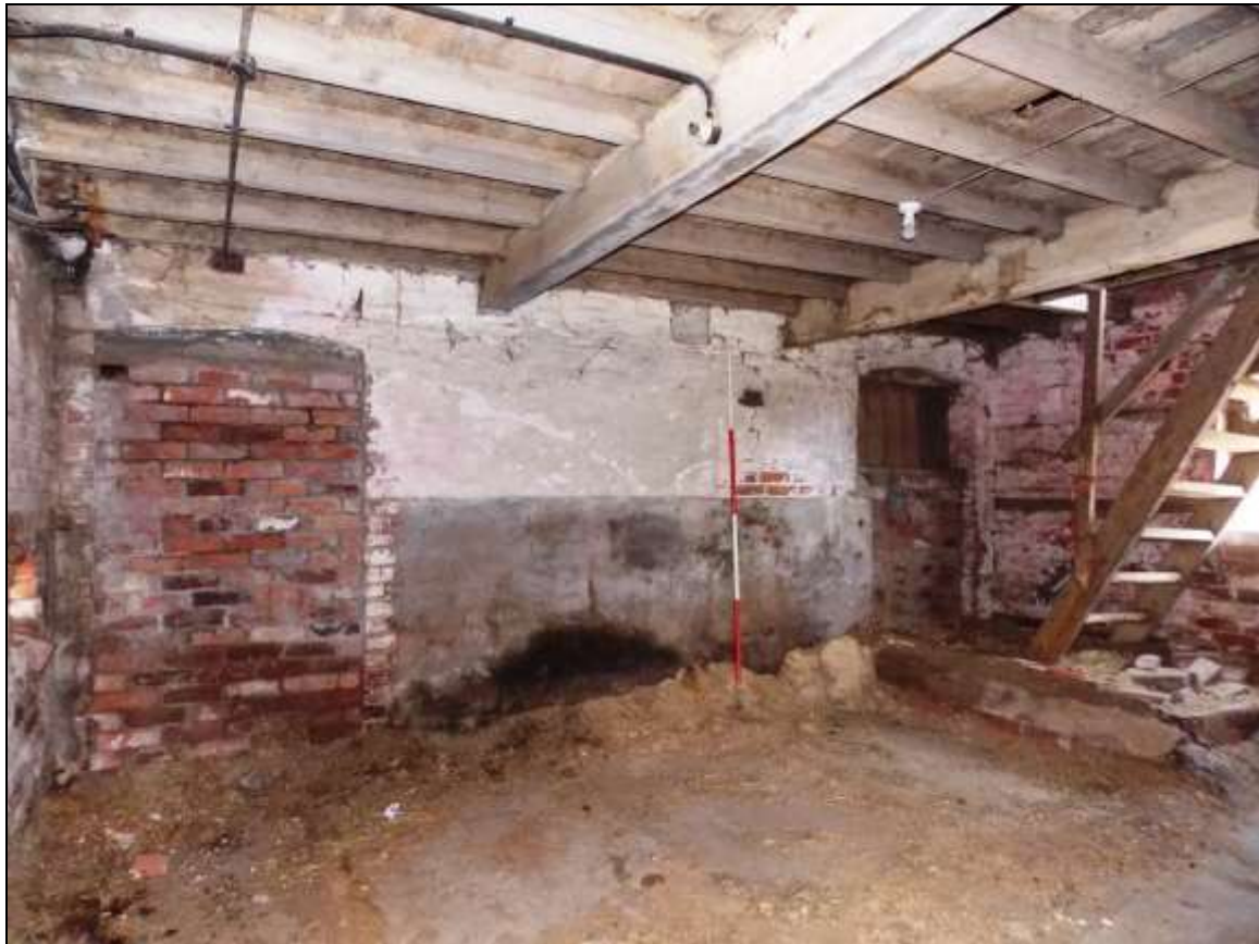
Plate 19: Ground floor of Building B with blocked-up doorways within the north-western wall (scale 2m).
