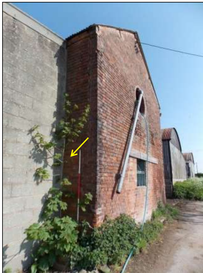
Plate 45: Gable wall and blocked-up opening (arrow) within the south-western elevation (scale 2m).
