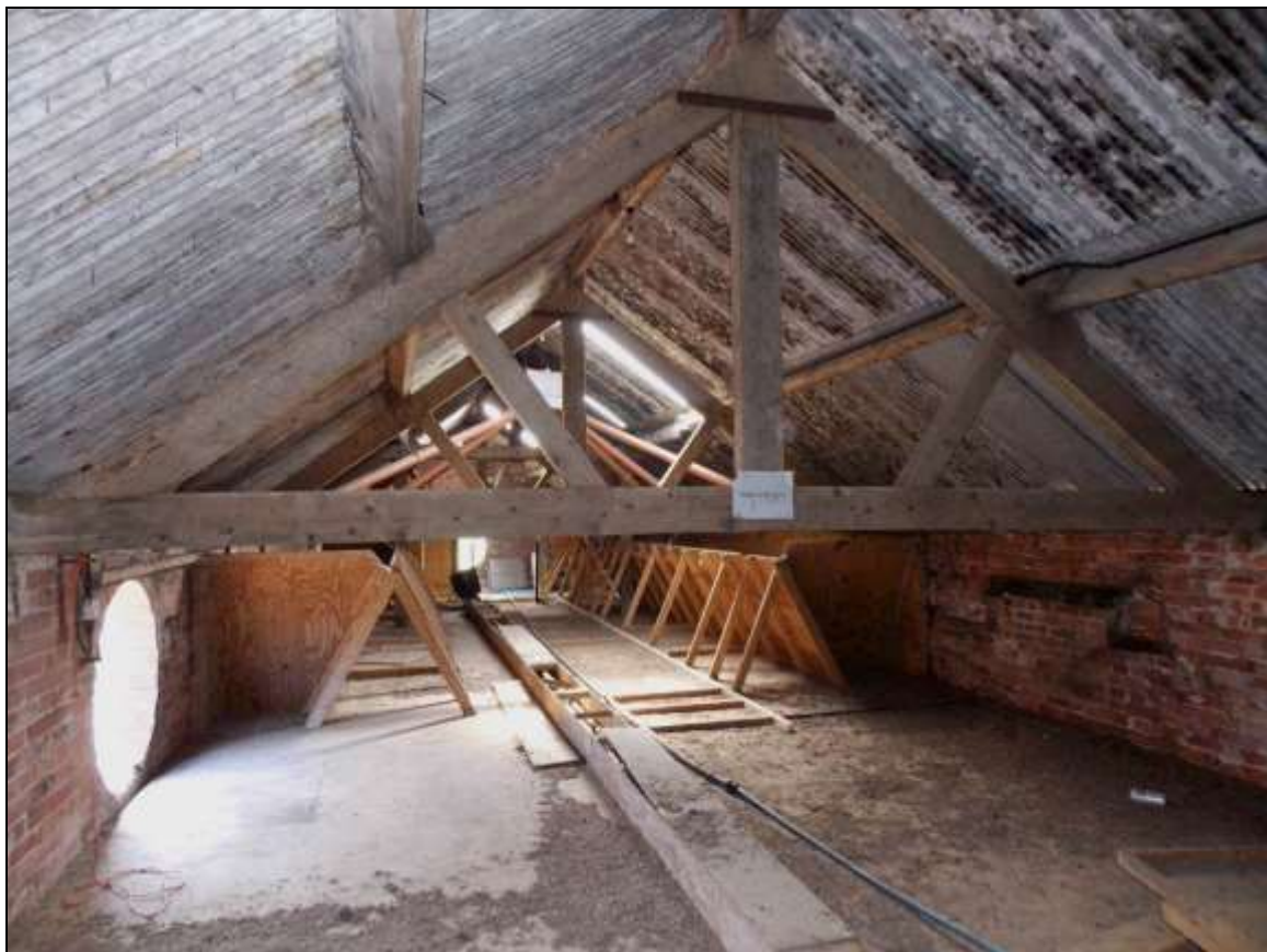
Plate 52: King-post trusses equivalent to the one within the adjacent Building C, looking south-west.
