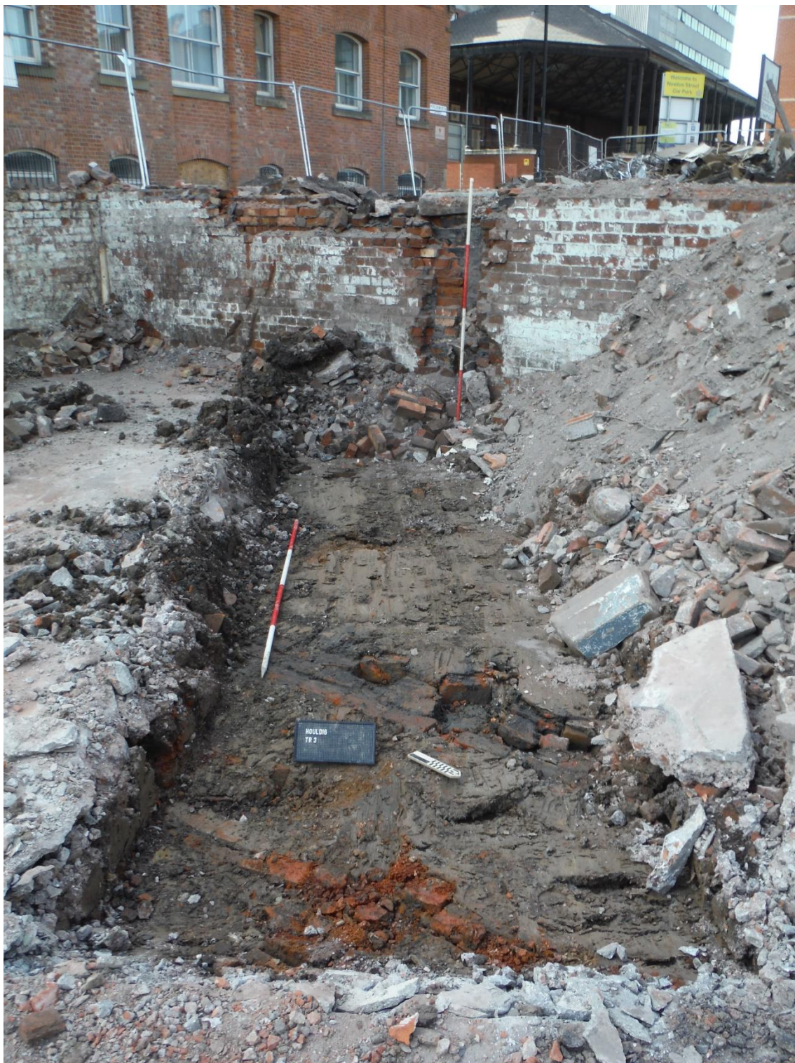
Figure 19. Overview of eastern end of Trench 3, with wall of 47 Houldsworth Street still standing in background, looking east (scale 2 x 2m)
