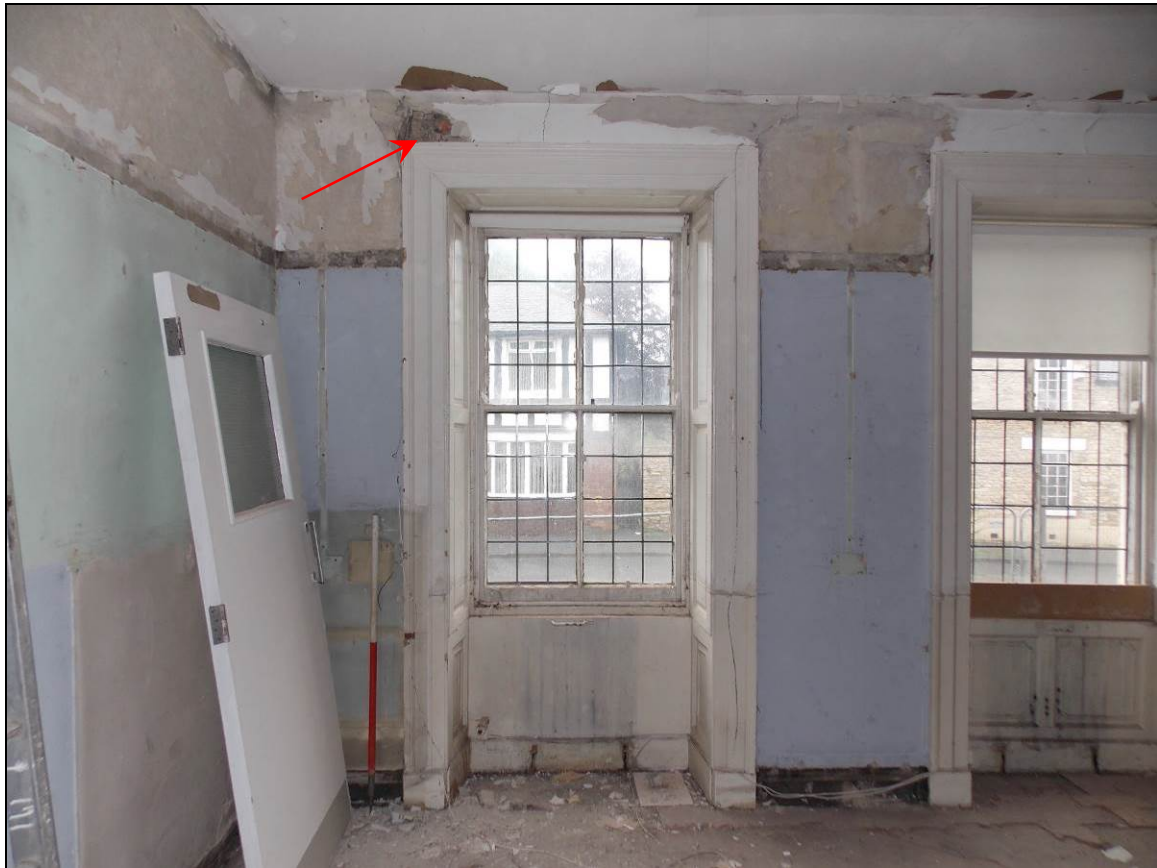
Figure 9: Window opening within the adjacent room G2 with comparable brickwork above the lintel (arrow).
