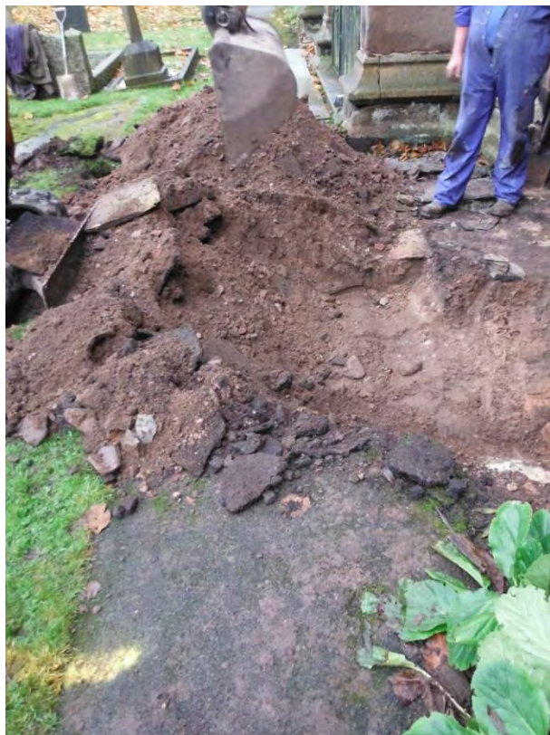
Figure 4. Working shot looking east showing removal of sand (105) beneath tarmac path (104) and slabs (F101).
