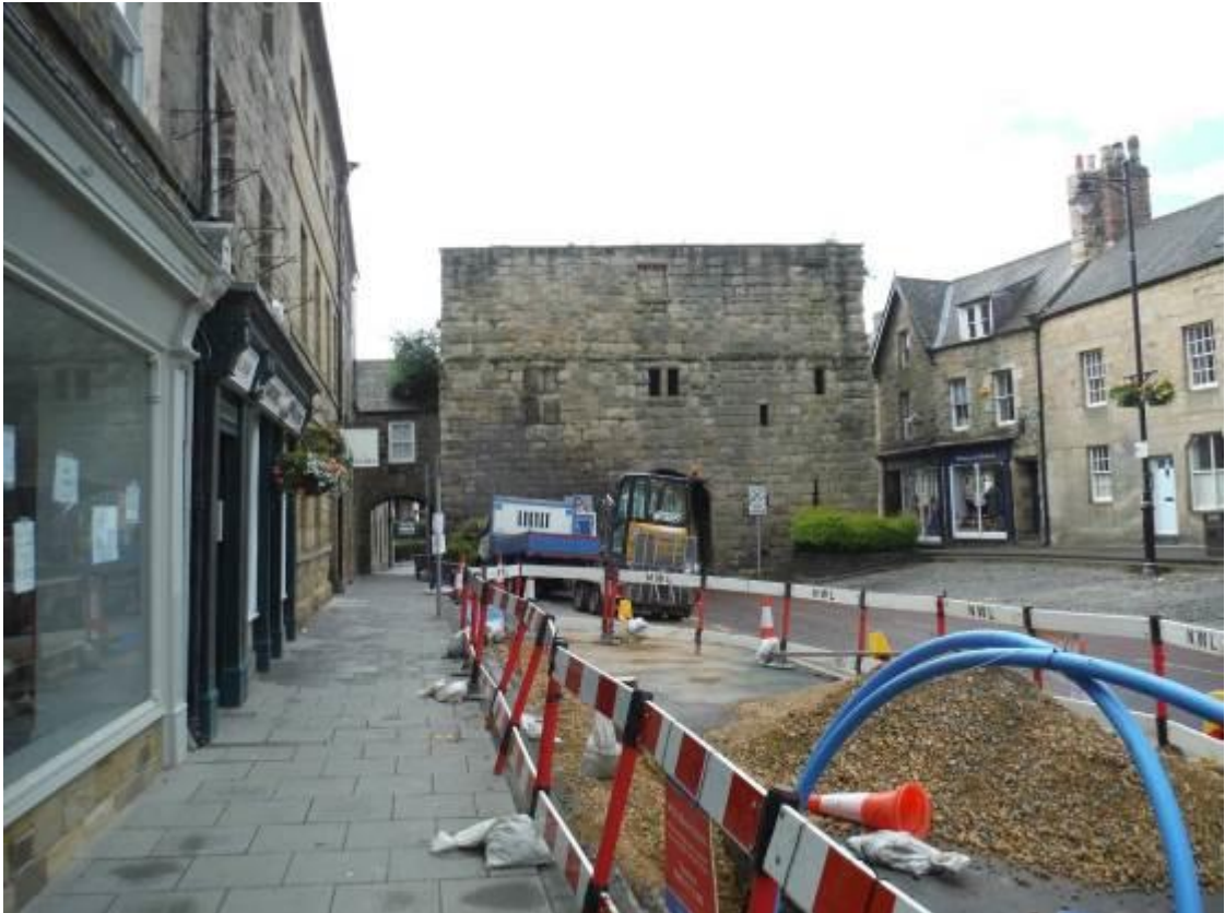
Figure 10: View of the trench looking south east. Note Bondgate tower in the background (scale = 1 x 1m)
