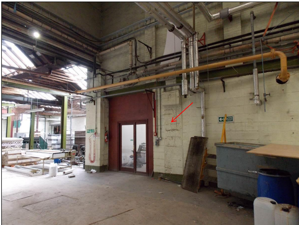
Plate 31: Stone pilaster with corbel (arrow) within the partition wall to the adjacent Building 4.
