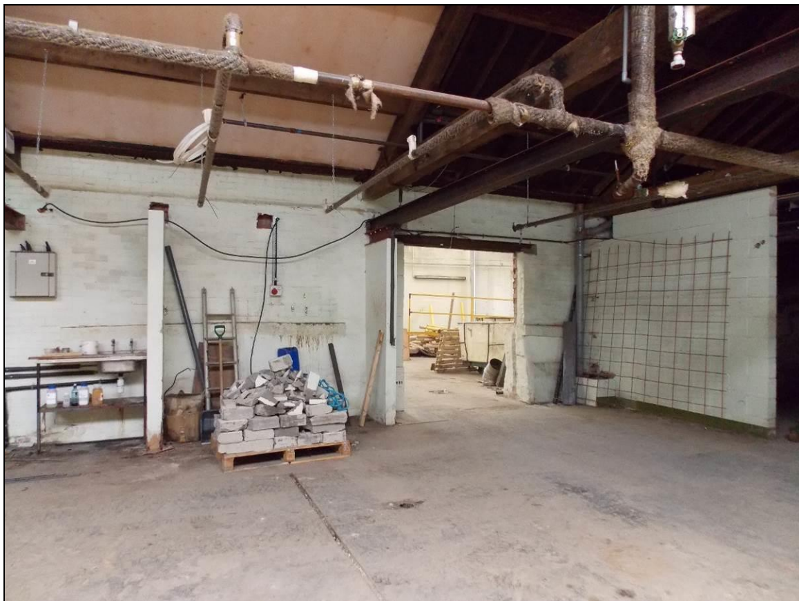
Plate 26: Internal view of Building 4A with blocked-up windows of adjacent Building 5, looking north-west.
