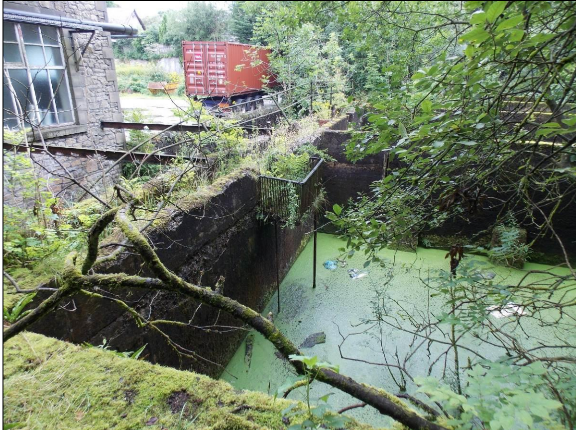
Plate 63: General view of the tanks, looking north-east.
