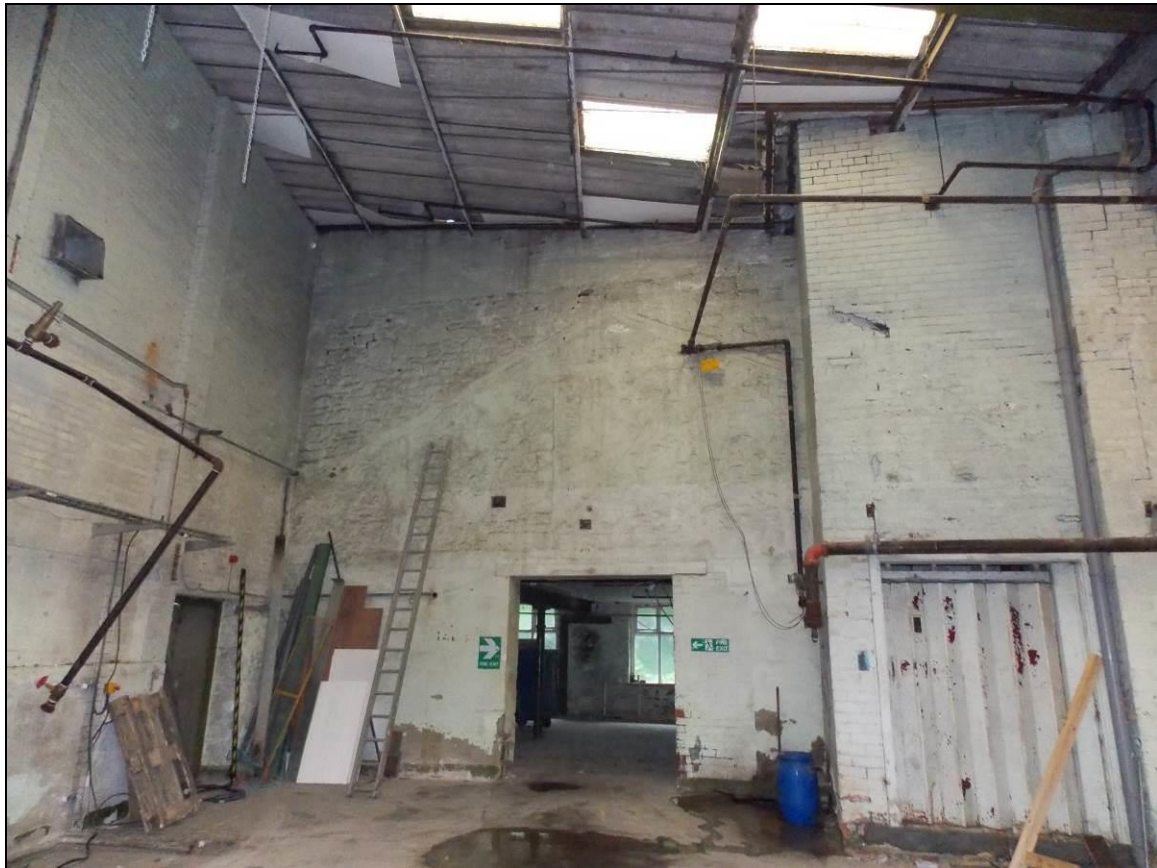
Plate 30: South-eastern end of Building 5 with a lower gable wall and an adjacent lift shaft.
