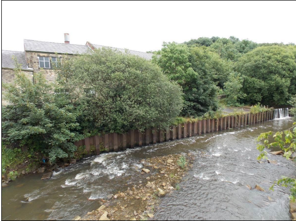
Plate 70: Croft End Mill along the River Irwell viewed from Stubbins Bridge, looking north-east.
