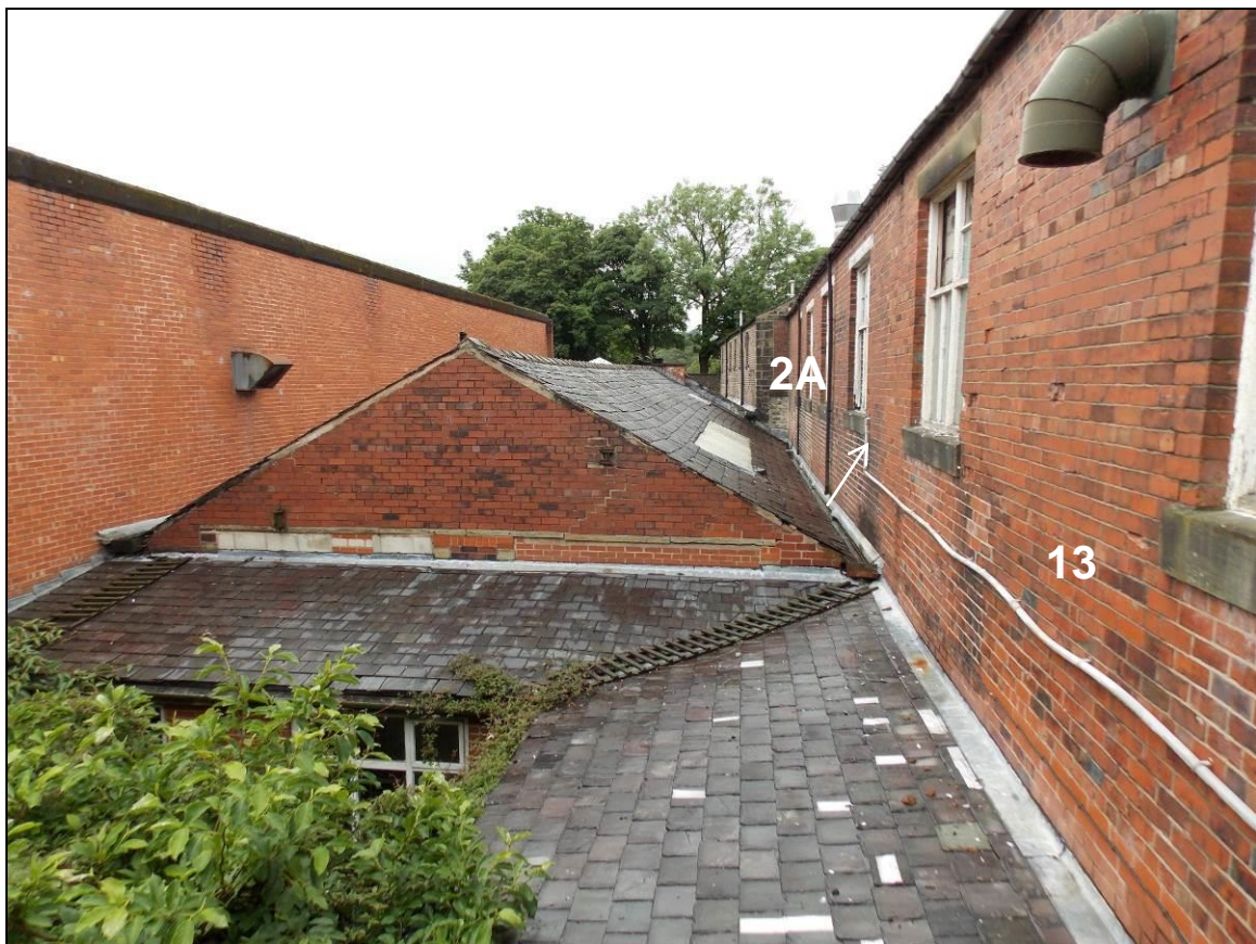
Plate 14: South-west elevation of Buildings 2A and 13 with construction joint (arrow), looking north-west.
