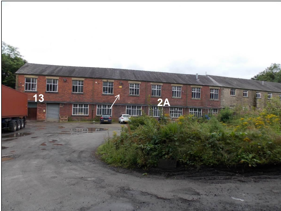
Plate 13: North-east elevation of Buildings 2A and 13 with construction joint (arrow), looking south-east.
