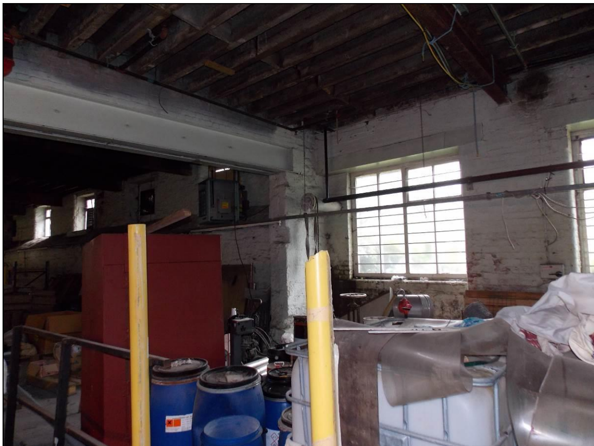
Plate 16: North-western end opened up to the adjacent Building 2 with an RSJ girder, looking north.
