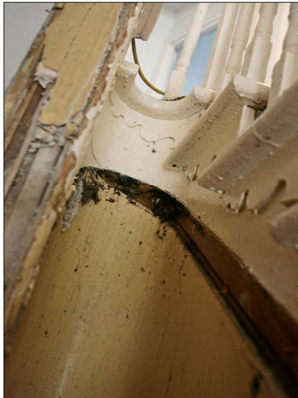
Fig. 23 Doubled back wall in staircase, ground floor
