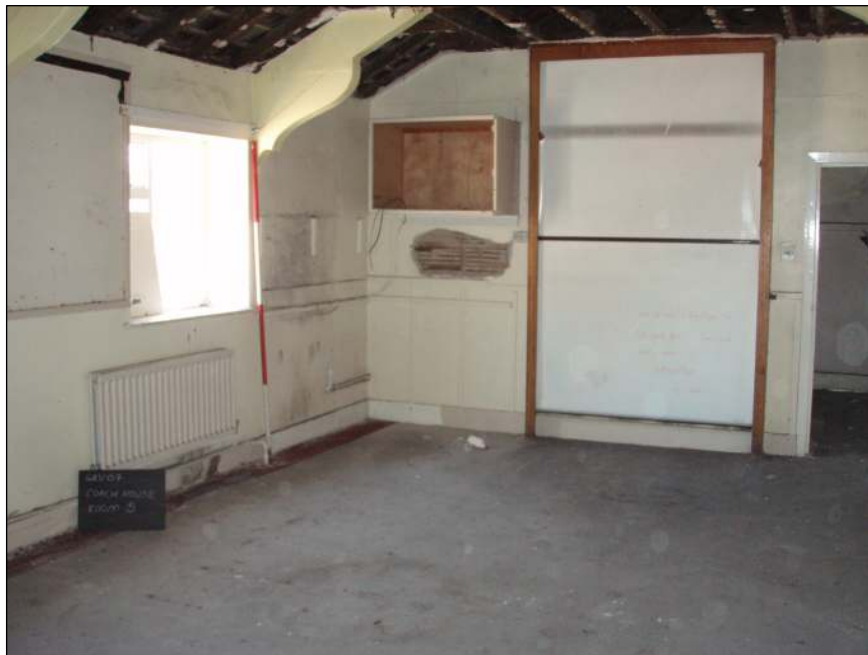
Fig. 67 Room Five showing decorative fittings attached to original roof beams, scale 2m
