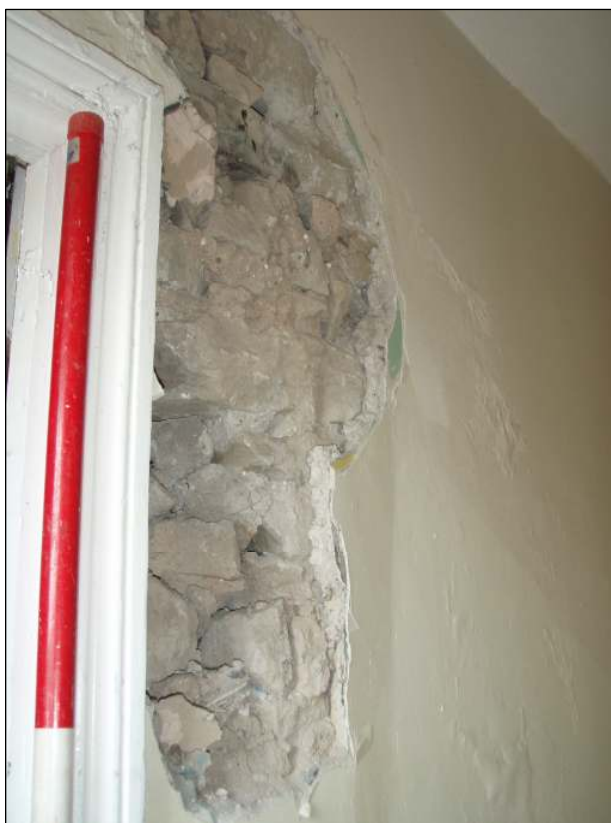
Fig. 65 Damage to wall on first floor landing of Coach House (red section of scale bar measures 0.50m)
