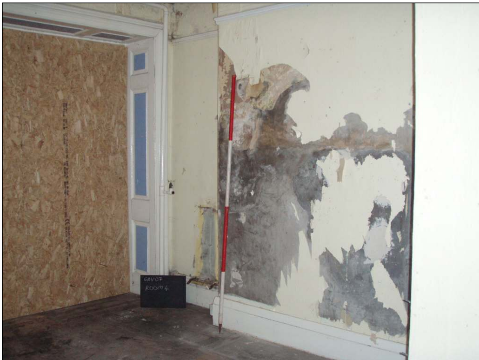
Fig. 33 Blocked access in Room Four. The heating pipe can be seen in the far corner, scale 2m
