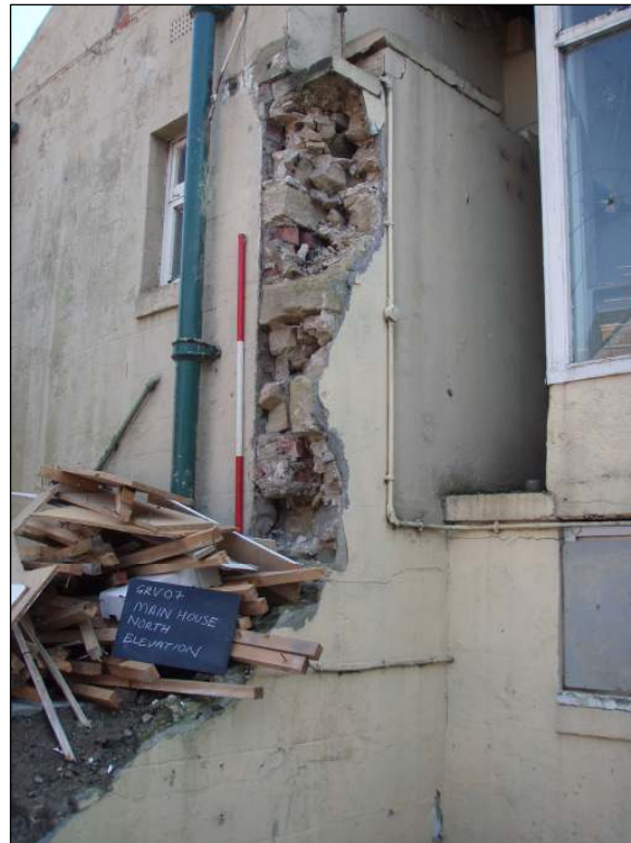
Fig. 15 Damage to wall in north elevation, scale 2m
