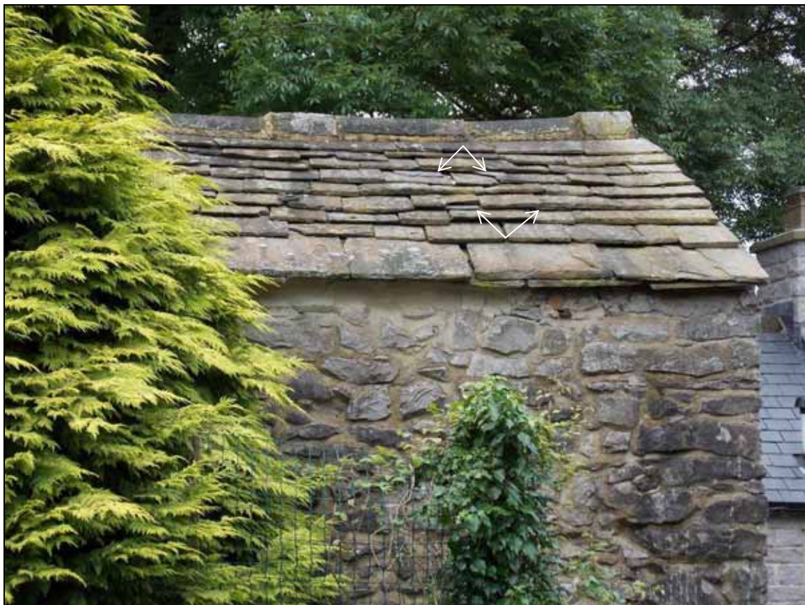
Plate 8: Southern pitched stone roof with slate repair (arrows), looking north.
