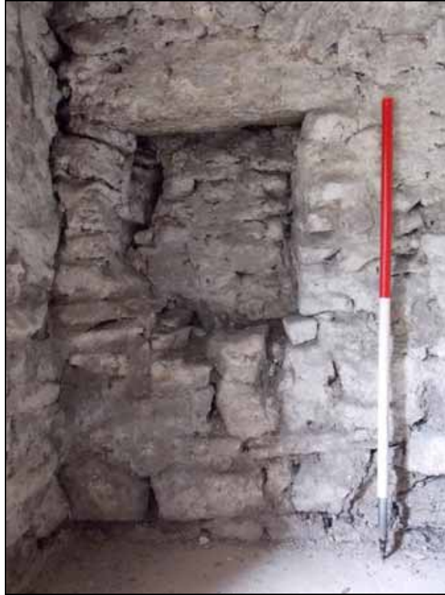
Plate 36: Detail of niche within the east wall on the ground floor (scale 1m).
