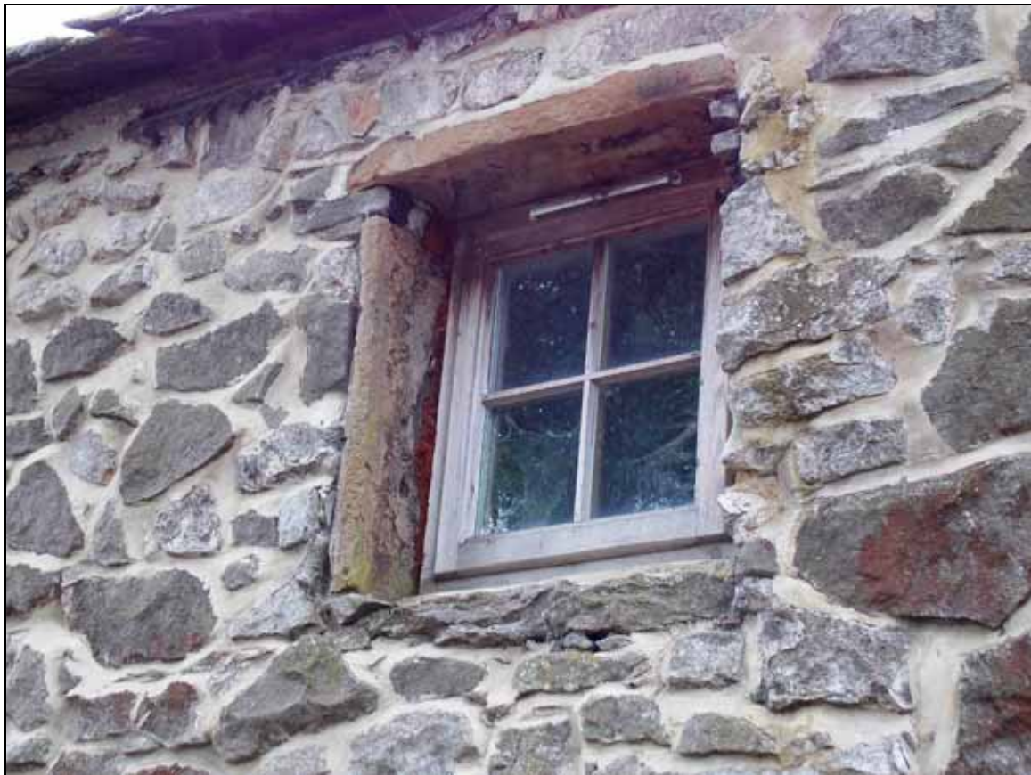
Plate 6: Detail of window opening on the first floor of the south elevation, looking south-east.
