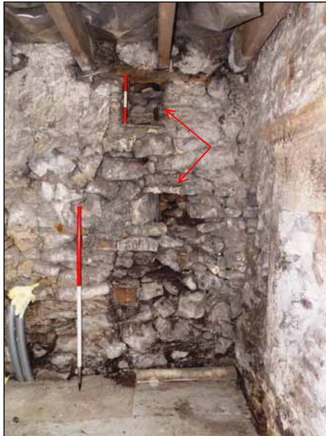
Plate 30: Small niches (arrows) within the western end of the south wall (scale 1m and 300mm).
