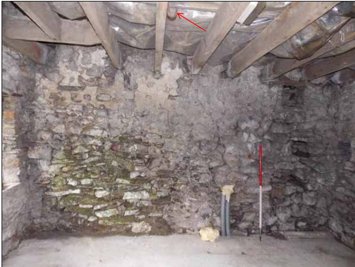
Plate 28: South wall and iron hook (arrow) attached to ceiling joist (scale 1m).
