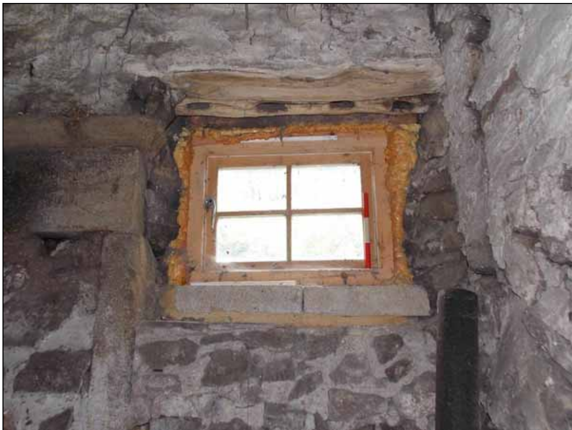
Plate 27: Detail of inserted window opening with reused lintel, looking west (scale 300mm).
