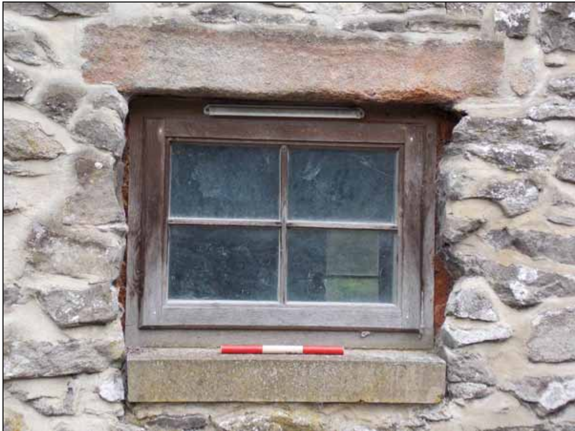
Plate 21: Detail of inserted window within the west elevation, looking east (scale 300mm).
