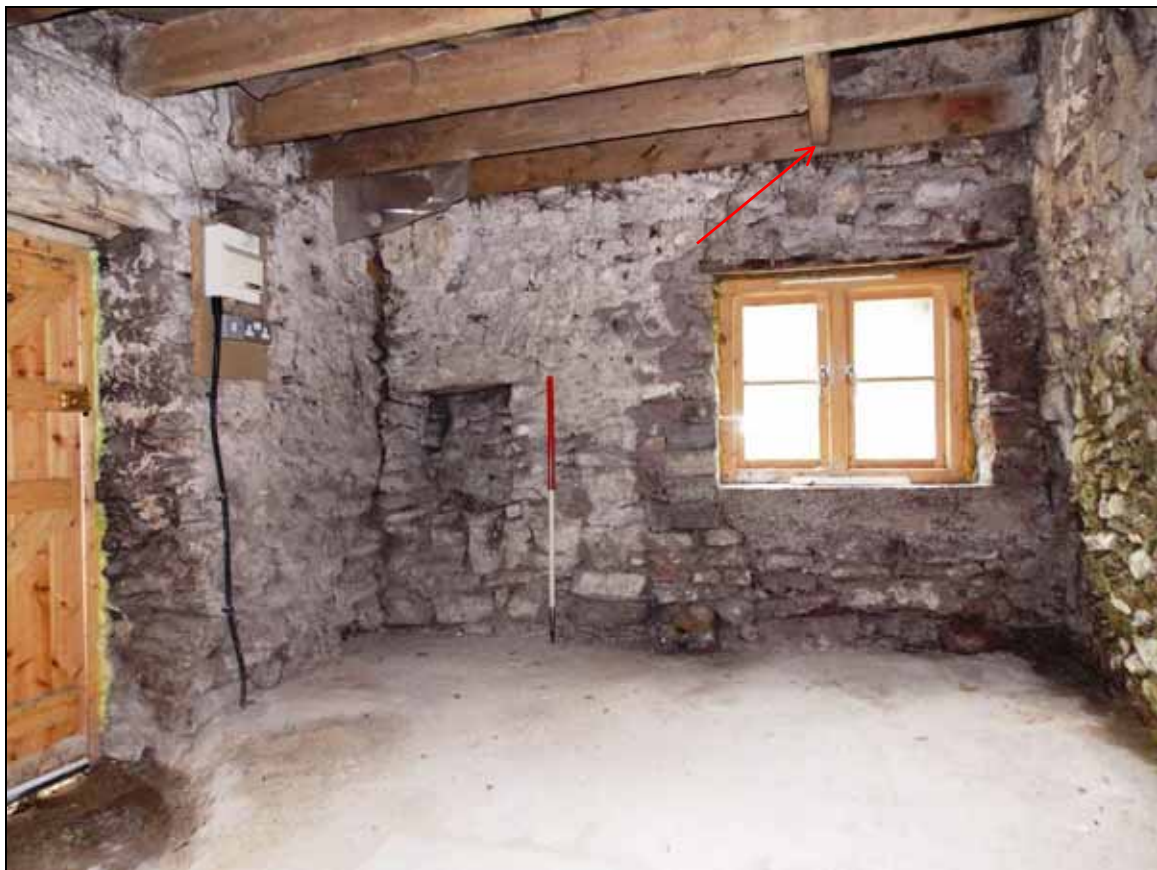
Plate 35: East wall and trimmer joists (arrow) for access to the upper loft storey (scale 1m).
