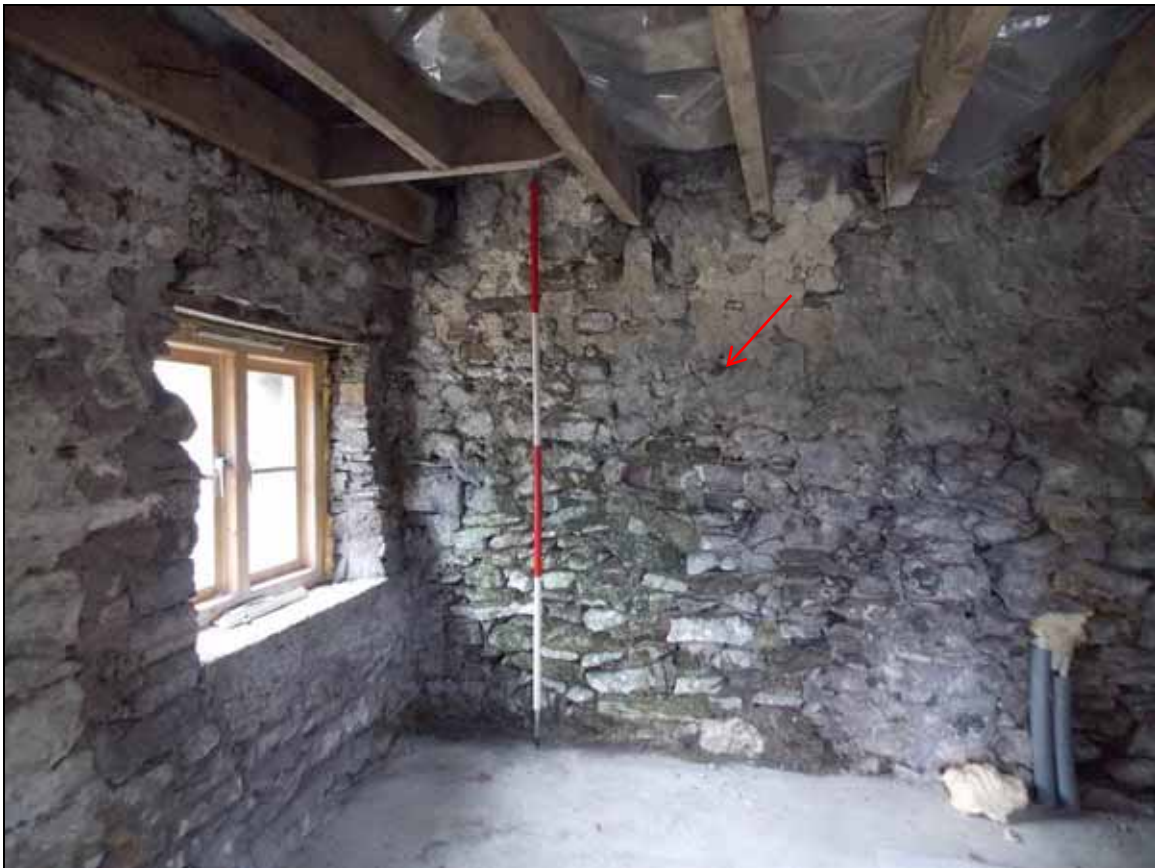
Plate 33: Embedded borer (arrow) within the eastern side of the south wall (scale 2m).
