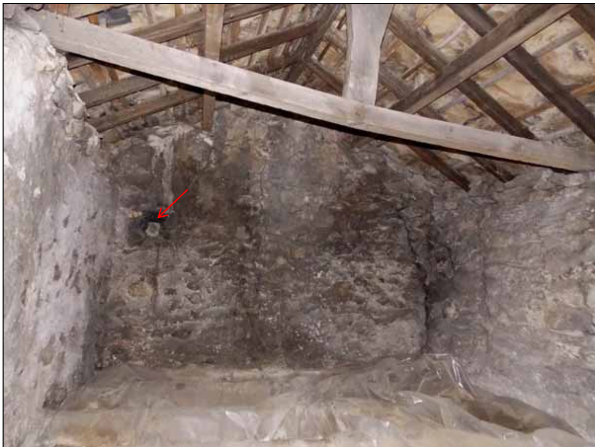
Plate 39: West wall of the loft with deep slot (arrow).
