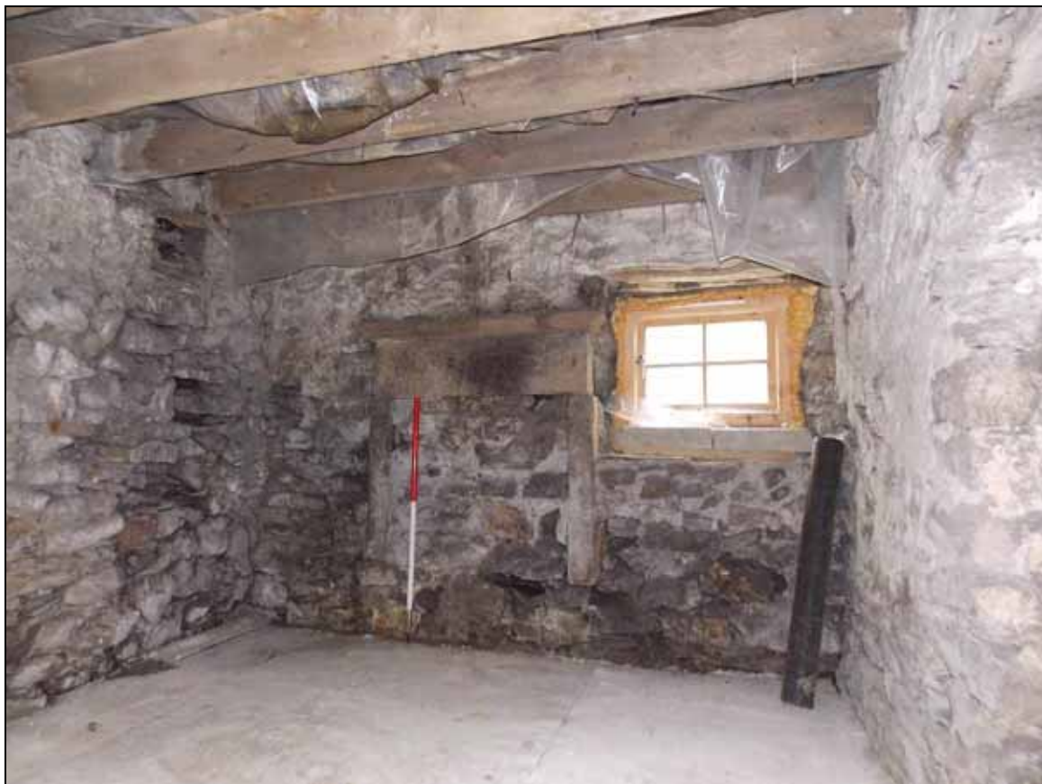
Plate 25: West wall with blocked-up fire place and inserted window opening (scale 1m).
