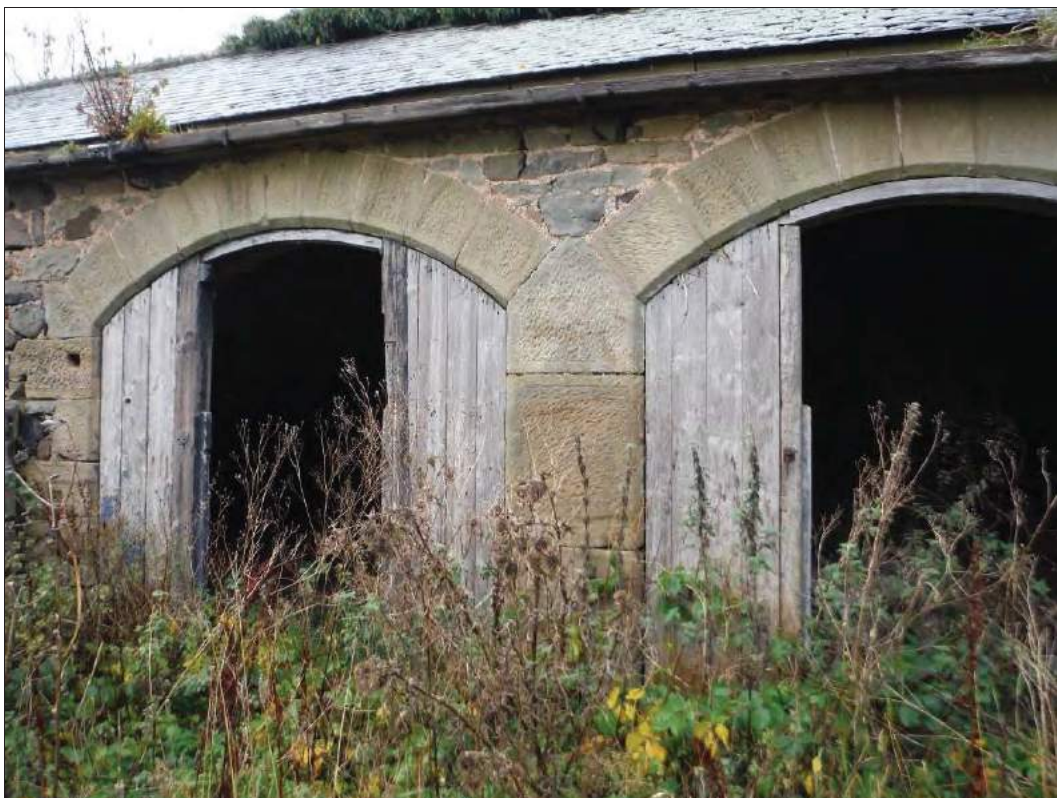
Figure 26: The northern two archways on the east elevation of the shelter shed with later inserted timber doors.
