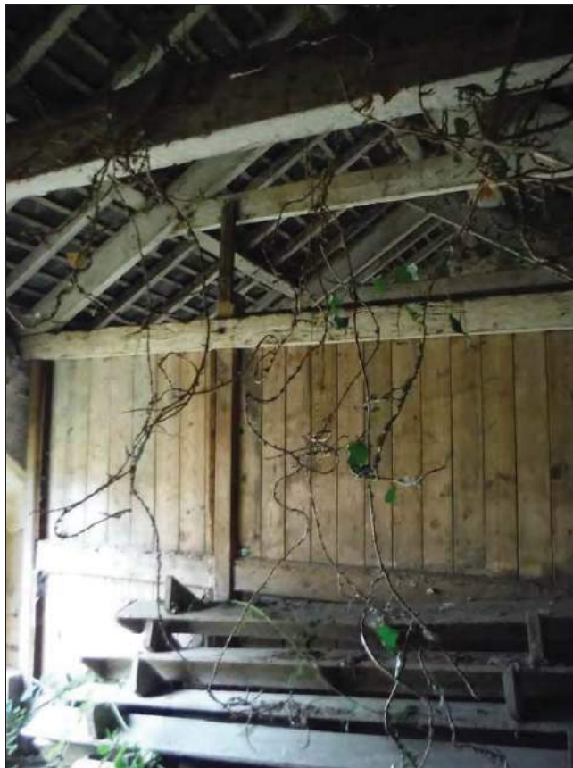
Figure 28: Inserted timber partition between the northern two arches of the shelter shed, looking south.
