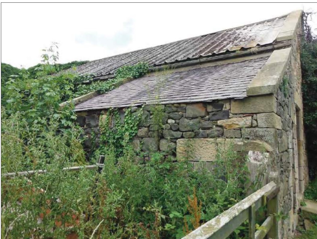
Figure 20: South elevation of the possible turnip store on the east end of south elevation of the cowhouse, looking north.
