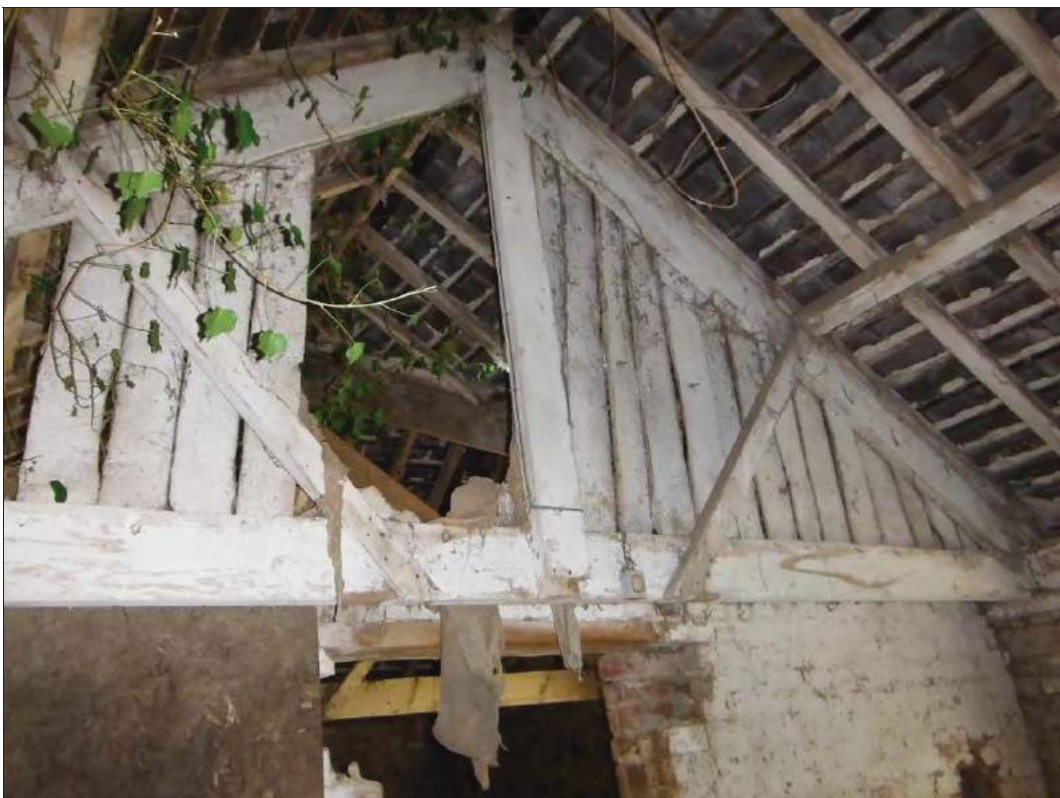
Figure 22: Timber boarded roof truss towards the western end of the cowhouse with a brick partition wall beyond.
