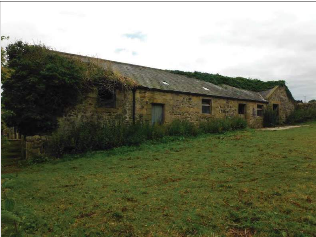
Figure 16: North elevation of the cowhouse forming the northern wing of the farm buildings range, looking south-west.
