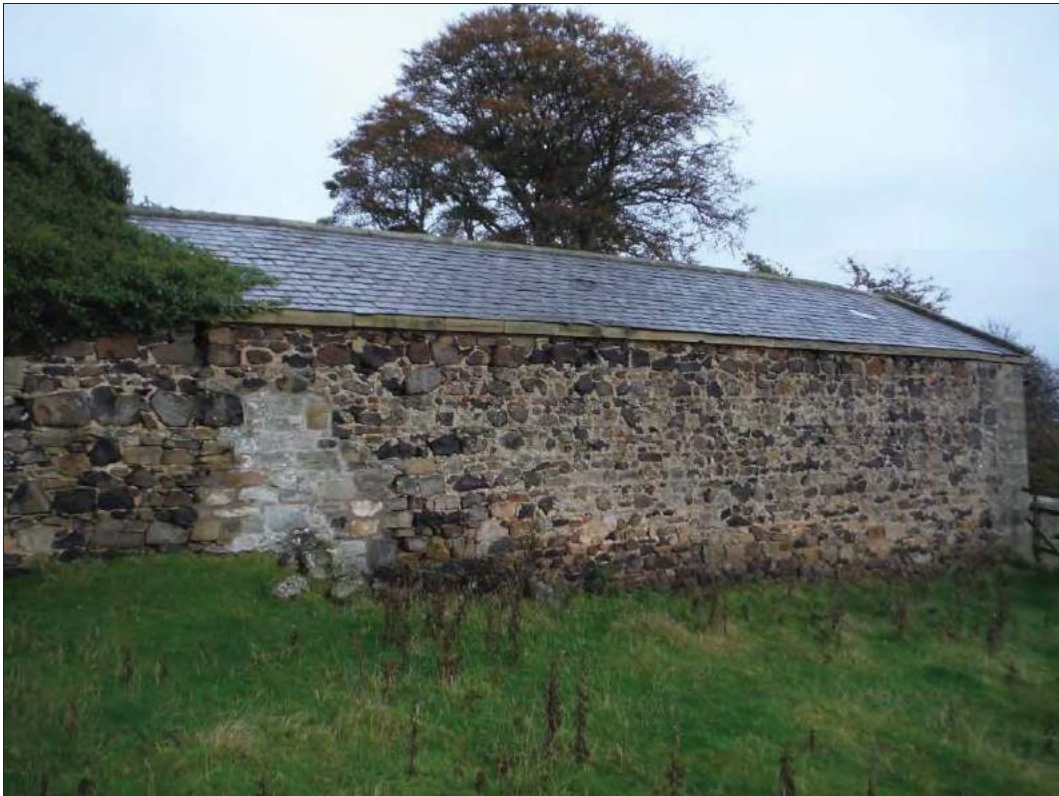
Figure 36: South elevation of the cart shed showing the small ventilation slit towards the west end of the wall and the patched masonry to its east side.
