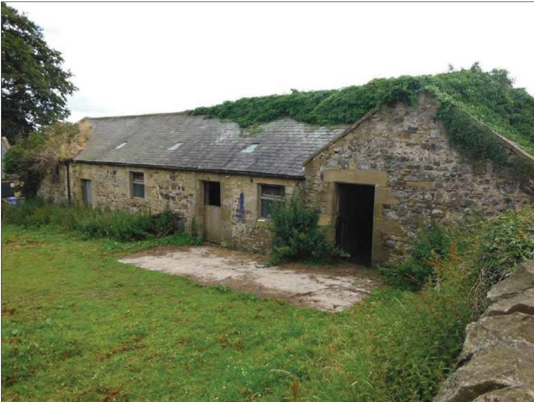
Figure 17: North elevation of the cowhouse forming the northern wing of the farm buildings range, looking south-east.
