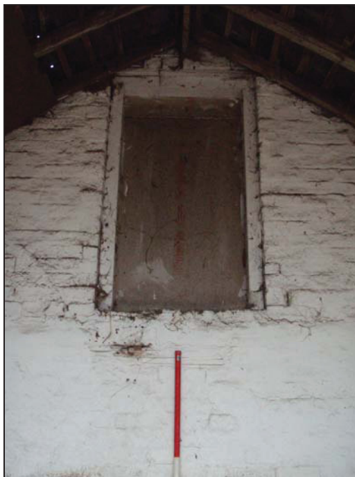
Figure 24. Boarded hay loft door in north-east wall of southern room (facing north-east) (scale = 2m).
