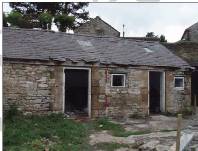
Figure 5. The single storey building and roof at The Croft, Bakewell (facing north) (scale = 2m).
