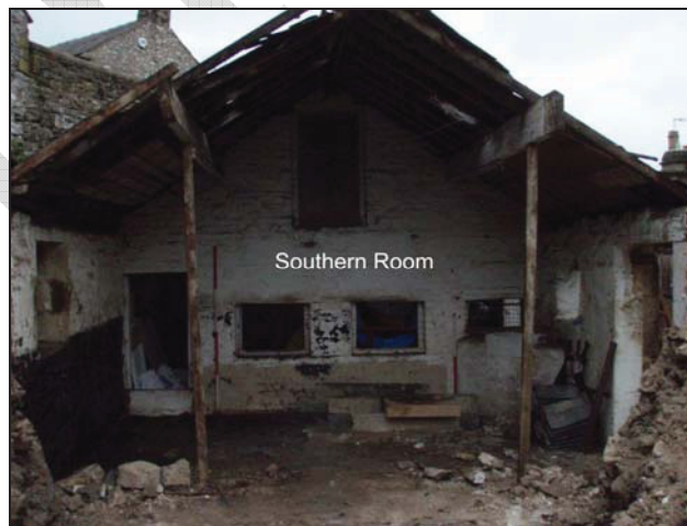
Figure 17. Interior of southern room after demolition of south-west wall and entranceway (facing north-east) (scale = 2m).
