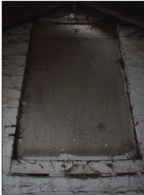
Figure 36. Blocked hay loft door in south-west wall of northern room (facing south-west).
