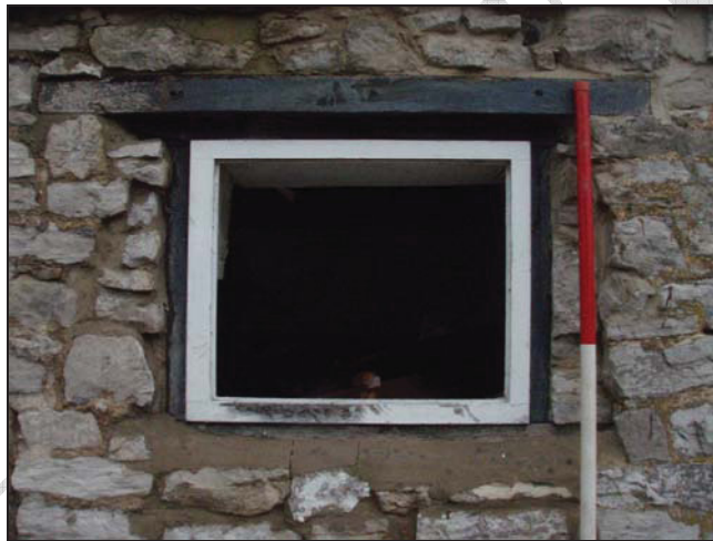
Figure 11. Window from the mid-section of the south-east wall of The Croft (facing north-west) (scale = 2m).
