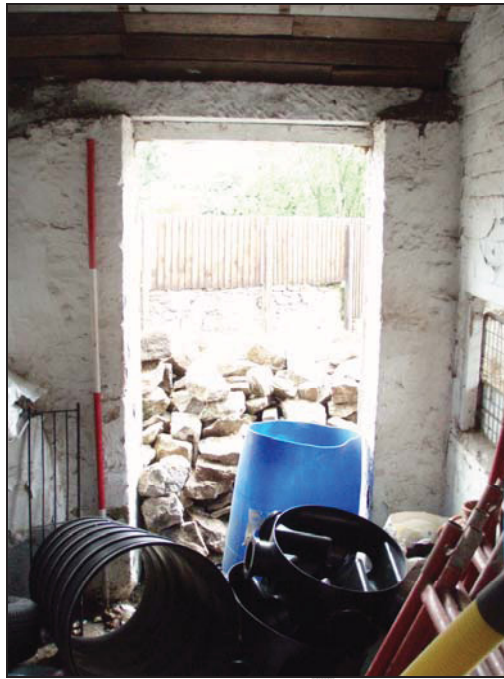
Figure 34. Door in the south-east room of northern room (facing north-east) (scale = 2m).
