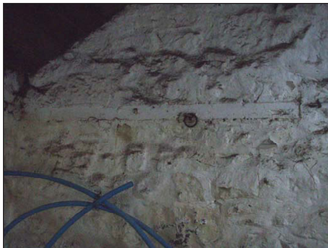
Figure 38. Metal hoop inserted into the north-east wall of the northern room (facing north-east).
