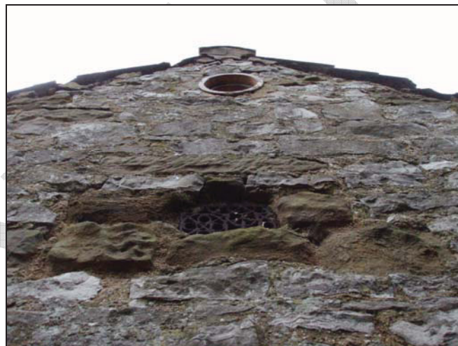
Figure 9. Air vent and pipe in the north-east wall of the building (facing south-west).
