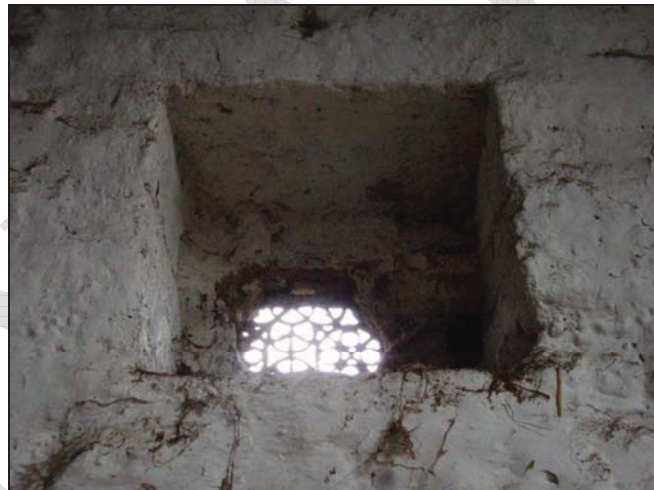
Figure 37. Air vent in the north-east wall of the northern room (facing north-east).
