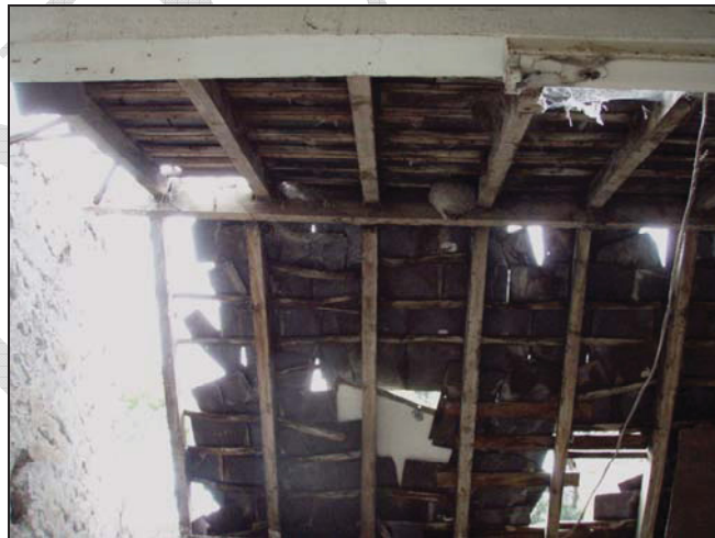
Figure 29. Roof of the southern room showing the windows and holes which have been boarded over (facing north).
