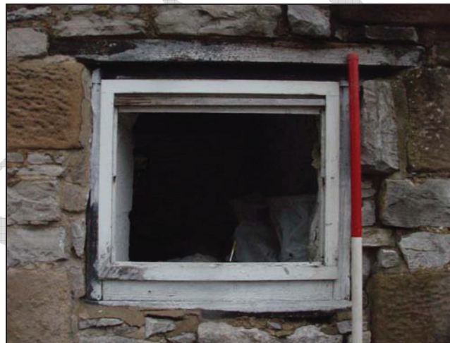
Figure 13. Window from the north end of the south-east wall of The Croft (facing north-west) (scale = 2m).
