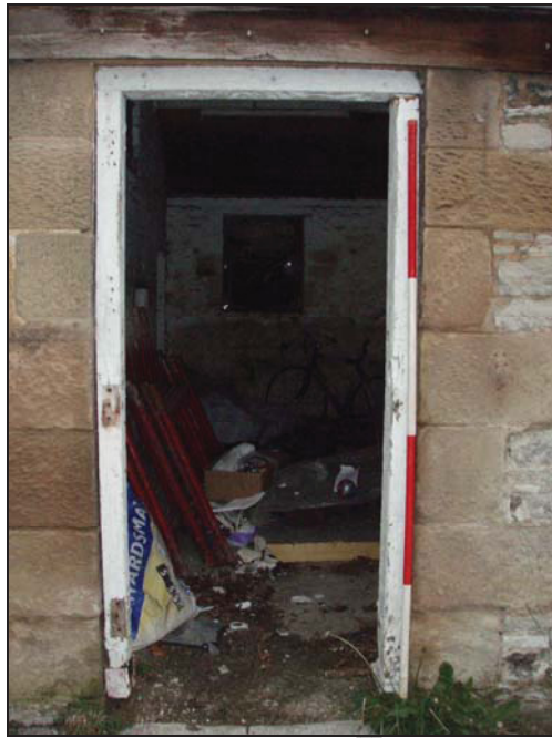
Figure 14. Doorway from the north end of the south-east wall of The Croft (facing north-west) (scale = 2m).
