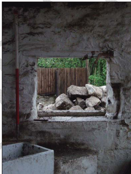
Figure 21. Window in south-east wall of the southern room (facing south-east) (scale = 1m).
