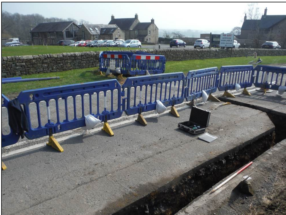
Figure 9. View facing south-east across Trench 19 towards Shawwell Farm. Surface (031) was identified at the base of the trench excavated through the grass verge east of the road (centre background) (Scale = 1 x 1m).
