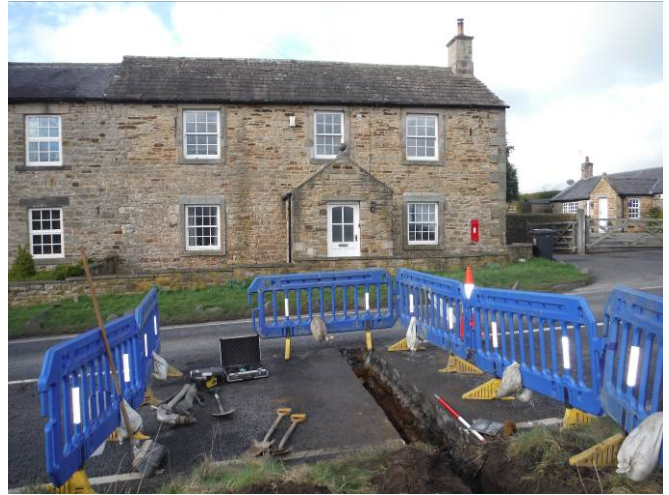
View facing west of Trench 6 looking towards The Counting House, Stagshaw Bank
