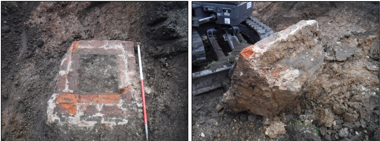
Figures 4 and 5. Post-excitation of structure [003] looking southwest and post-removal of structure [003] looking west
