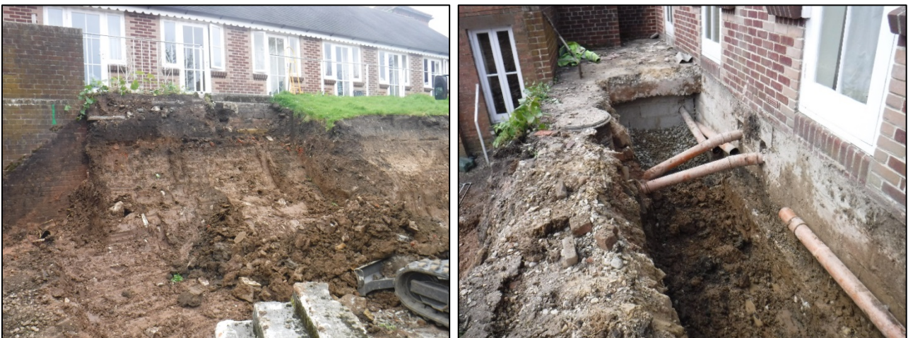
Figures 9 and 10. Post-excitation of staircase [011] looking northwest and general shot of trench looking southwest
