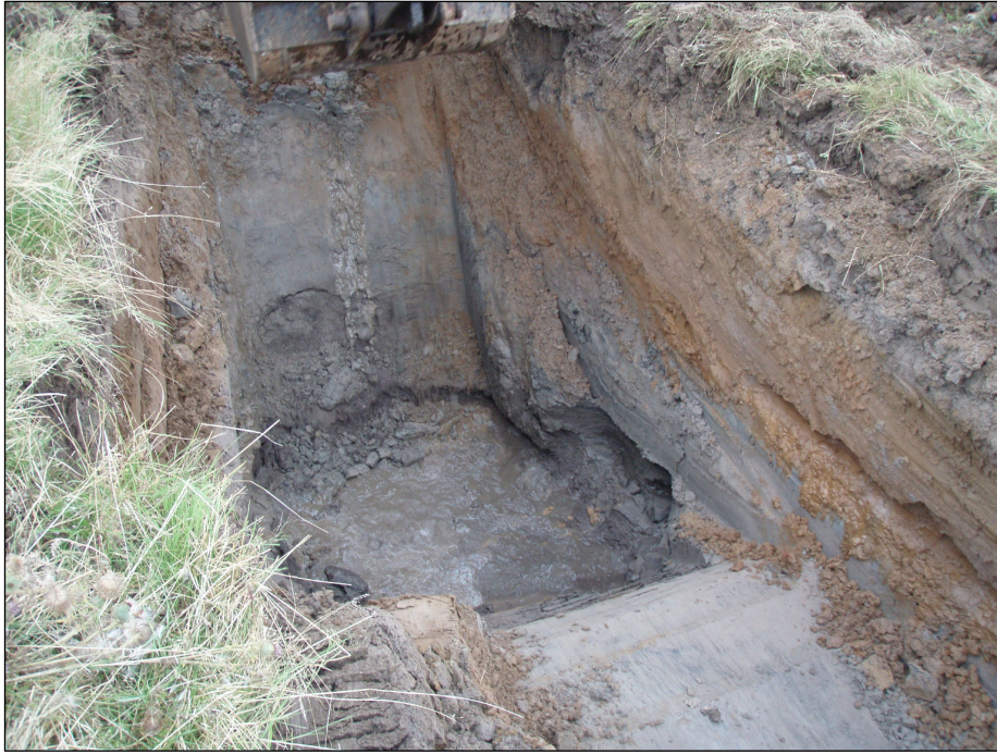
Fig. 4 Sondage excavated in western end of Trench 1 showing silts and clays (brown and orange) and coarse sands and gravels (greys). The photograph also shows the rapidly inflowing water causing collapse to the sides of the trench.
