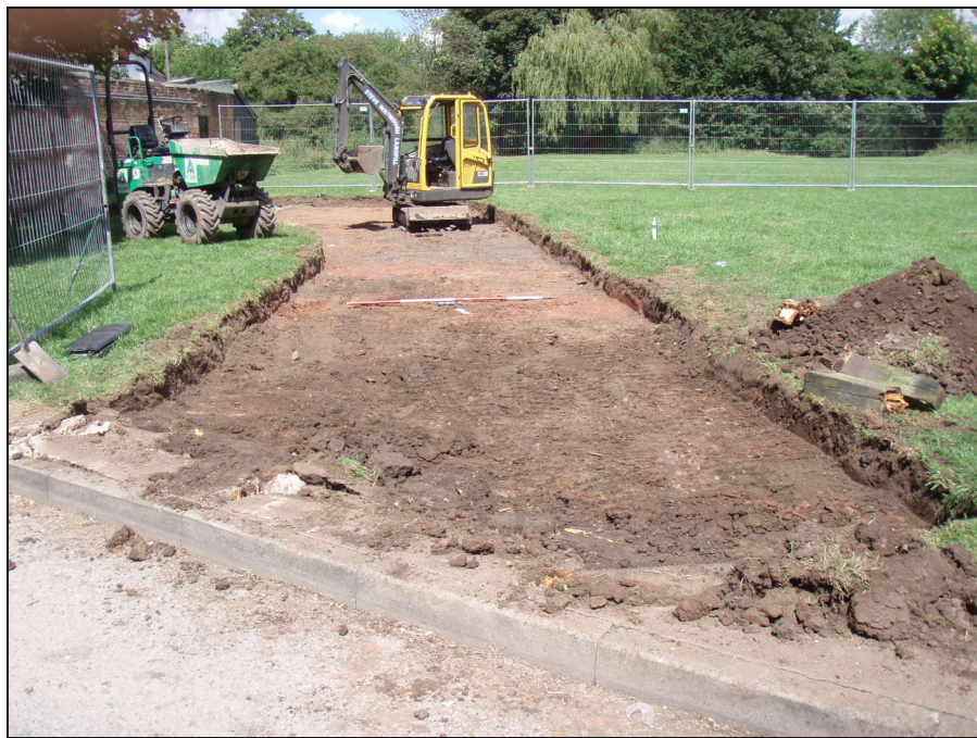
Fig. 5 View of the access track abutting kerbstones of road leading to the car park, looking south. Scale: 2m
