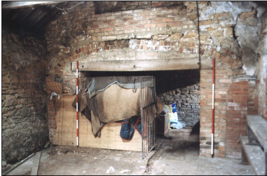
Figure 35: L-Plan barn, Room 2, looking east, showing brick arch knocked through to communicate with outshot, Room 3
