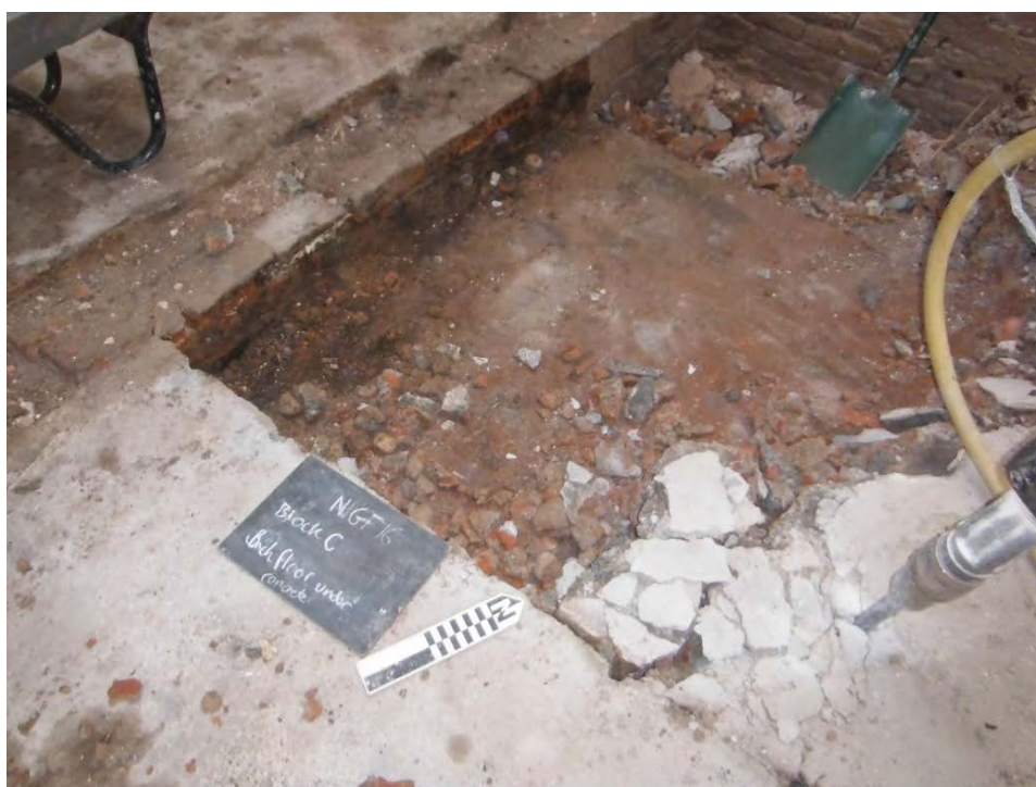
Figure 22. Exposing blue engineering brick surface (1019) after removal of concrete (1017) and brickcrete (1018) surfaces in room G3 of Block C, looking north-west. Visible wall is the remnant footing of the dividing wall between rooms G2 and G3. Scale: 0.25m.
