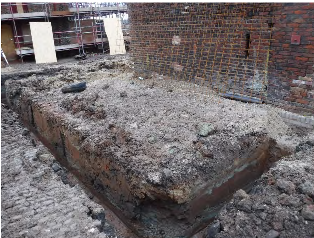
Figure 14. Newly excavated footings through natural clay (1002) after removal of former lean-to footing by the Block B south-west gable end. Two vertical black lines through the clay represent the timber slots for posts associated with the former lean-to. No scale.
