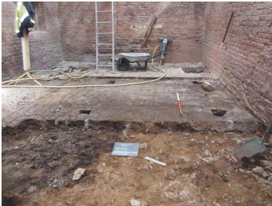
Figure 20. Granite-setts (1021) with sand bedding material (1025) after removal of concrete (1020) in room G1 of Block C, looking south-west. Note remnant of concrete surface beneath wheelbarrow and post-holes through the cobbled floor. Scale: 1m.
