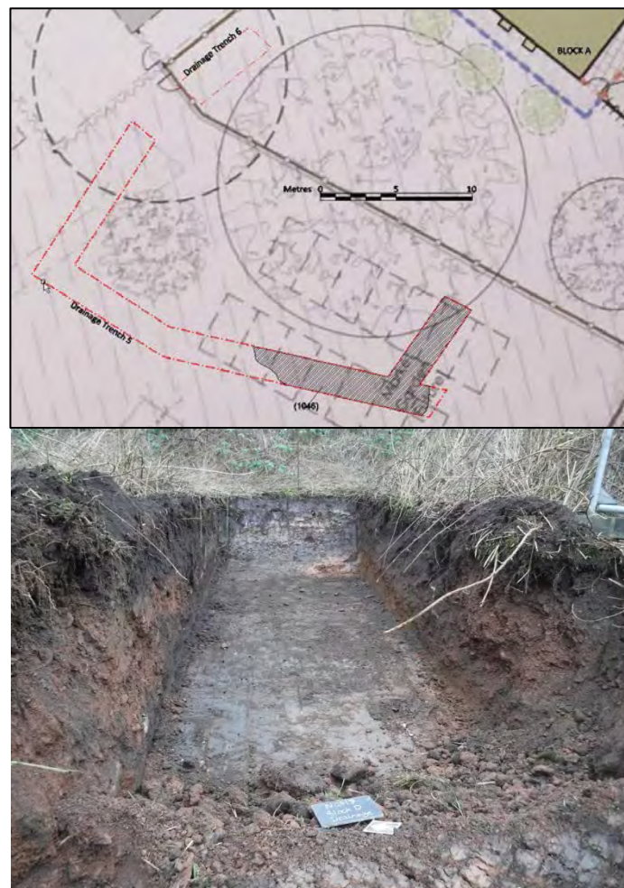
Figure 35. (Upper) Plan showing location of Drainage Trenches 5 and 6. Scale: as shown. (Lower) Rubble spread (1046) within Drainage Trench 5.
