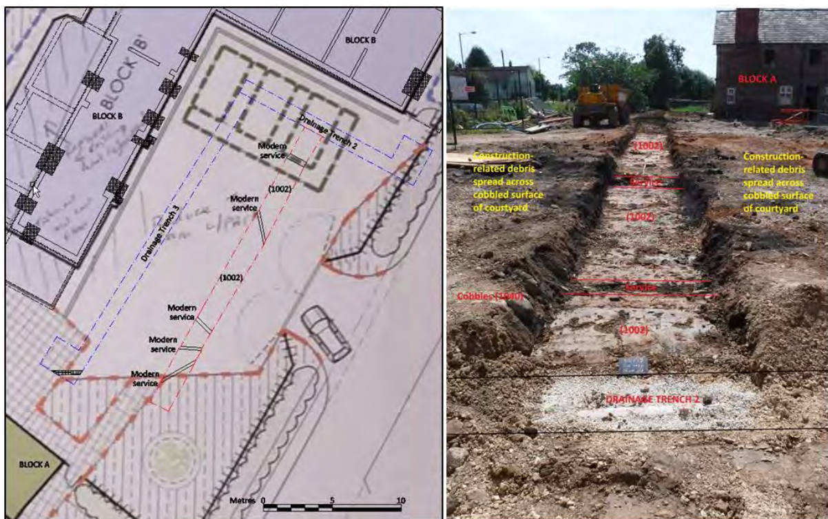
Figure 38. (Left) Plan showing location of investigation trench through the courtyard/carpark area. Scale: as shown. (Right) Annotated photo showing courtyard/carpark trench, looking south-west. Scale: 2m.
