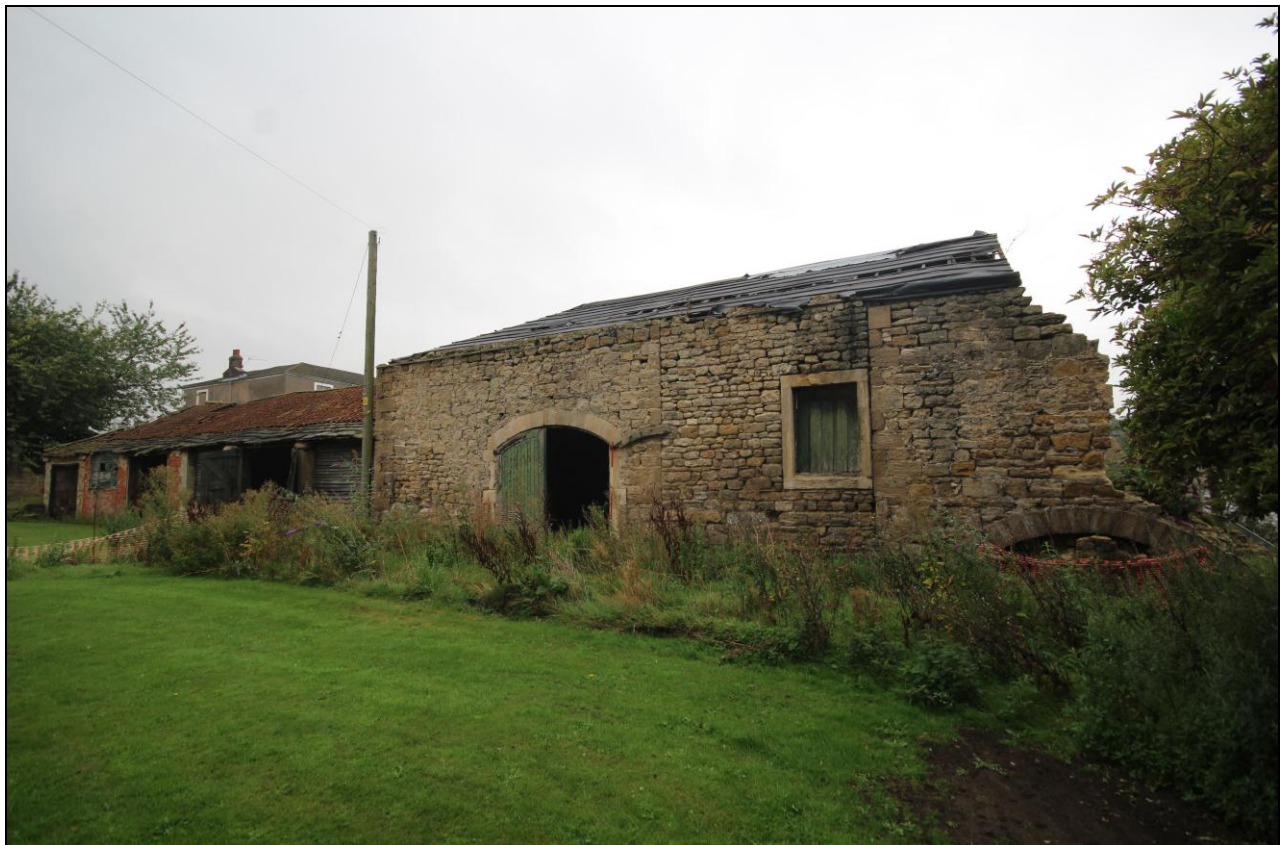
Figure 25: View of the partially collapsed building E, facing south west.
