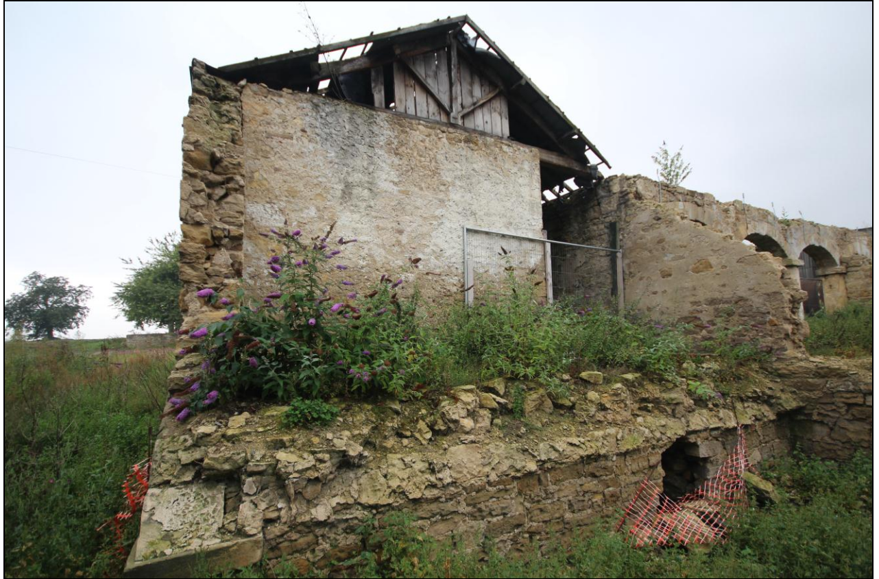
Figure 26: View of the collapsed northern section of building E.
