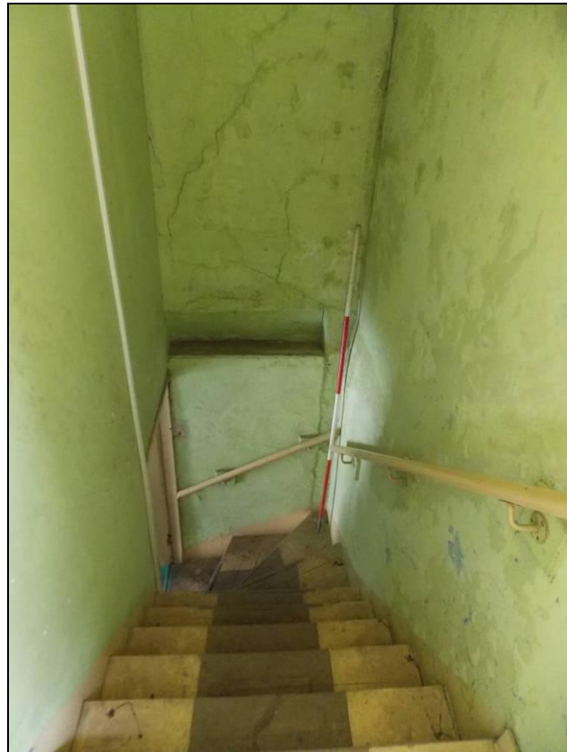
Figure 8: Staircase to the first floor with former opening blocked up, looking east, 2m scale.
