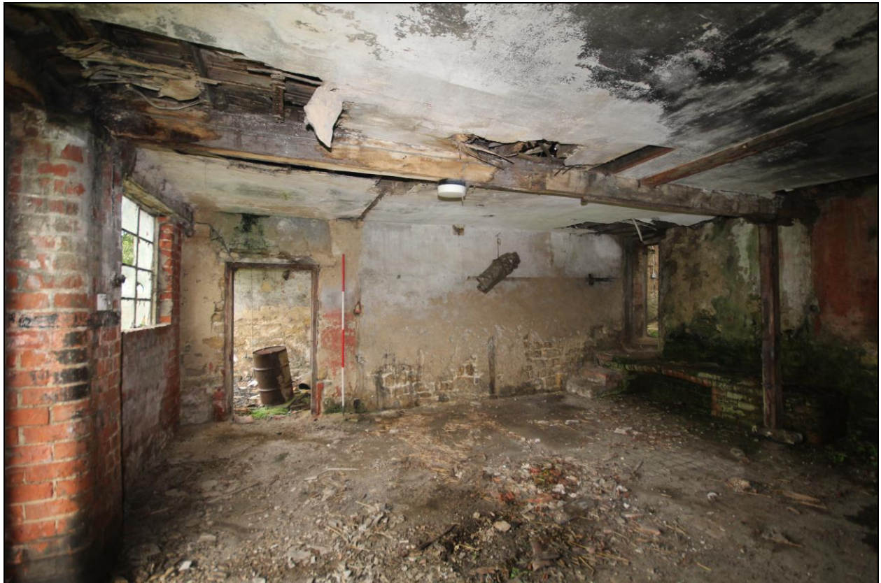
Figure 20: View of the interior of building D, facing south west, 2m scale.
