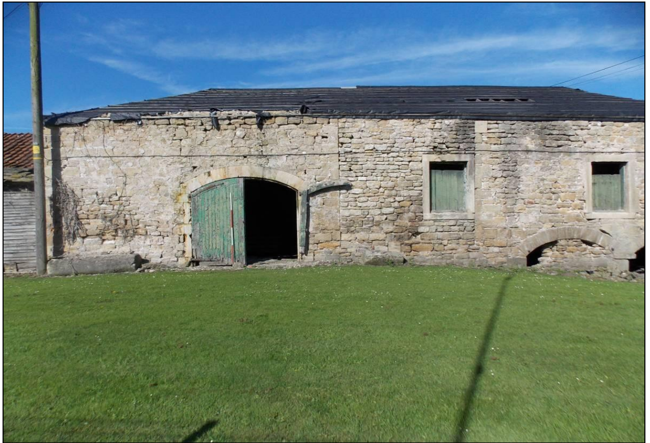
Figure 22: East elevation showing central opening blocked up and open-fronted basement in 2012, 2m scale.
