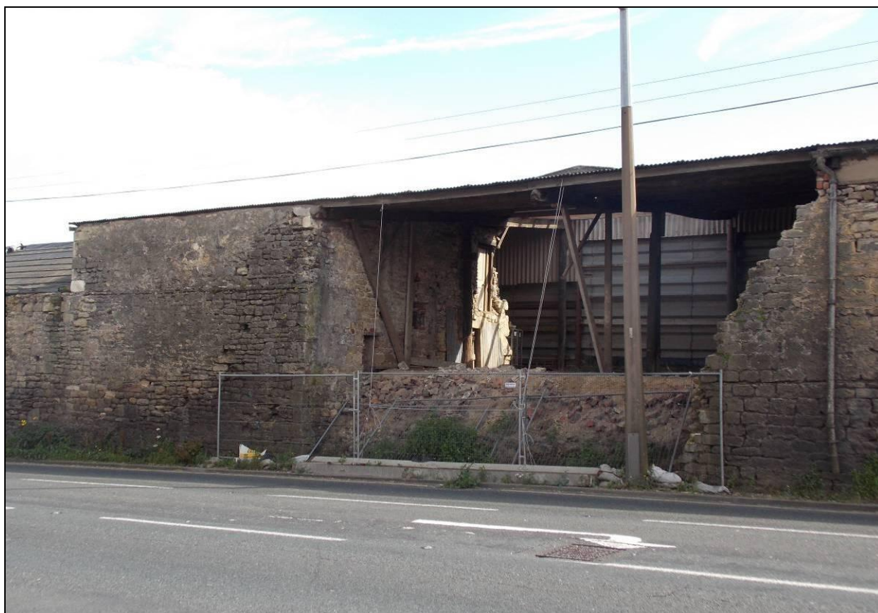
Figure 35: North elevation of Building G and collapsed wall of Building H in 2012, looking south-east.
