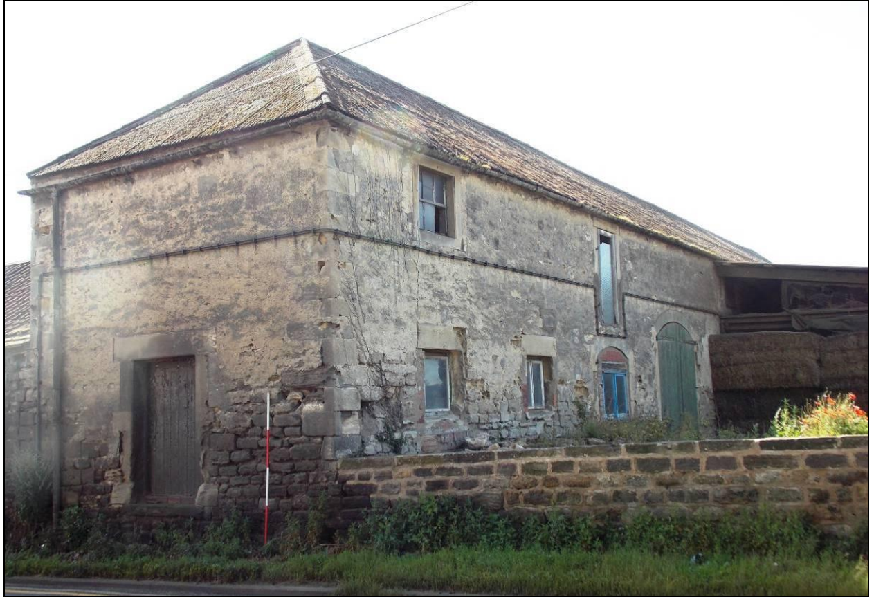
Figure 54: North and west elevations of Building L, looking south-east in 2012, scale 2m.
