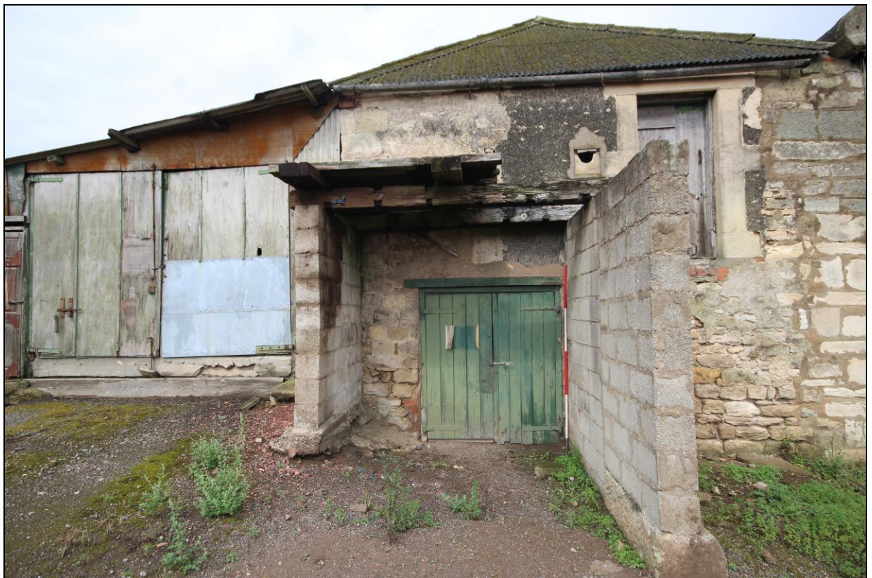
Figure 53: View of the one of the entrances to building L along the south elevation, 2m scale.
