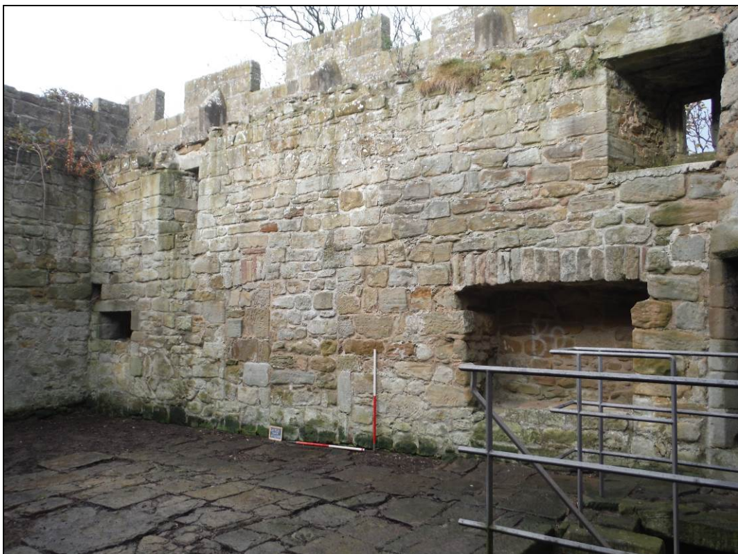
Figure 21. The southern extent of the north-western elevation of the pele tower's first floor. Scales = 2 x 1m.
