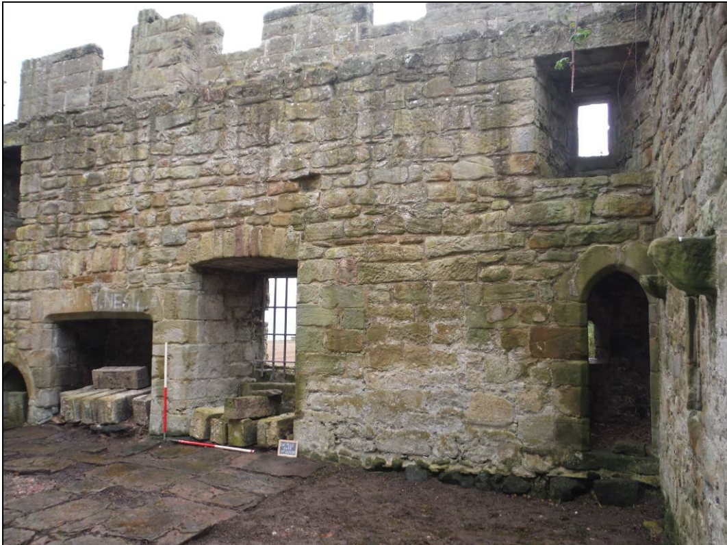
Figure 18. The southern extent of the south-eastern elevation of the pele tower's first floor. Scales = 2 x 1m.
