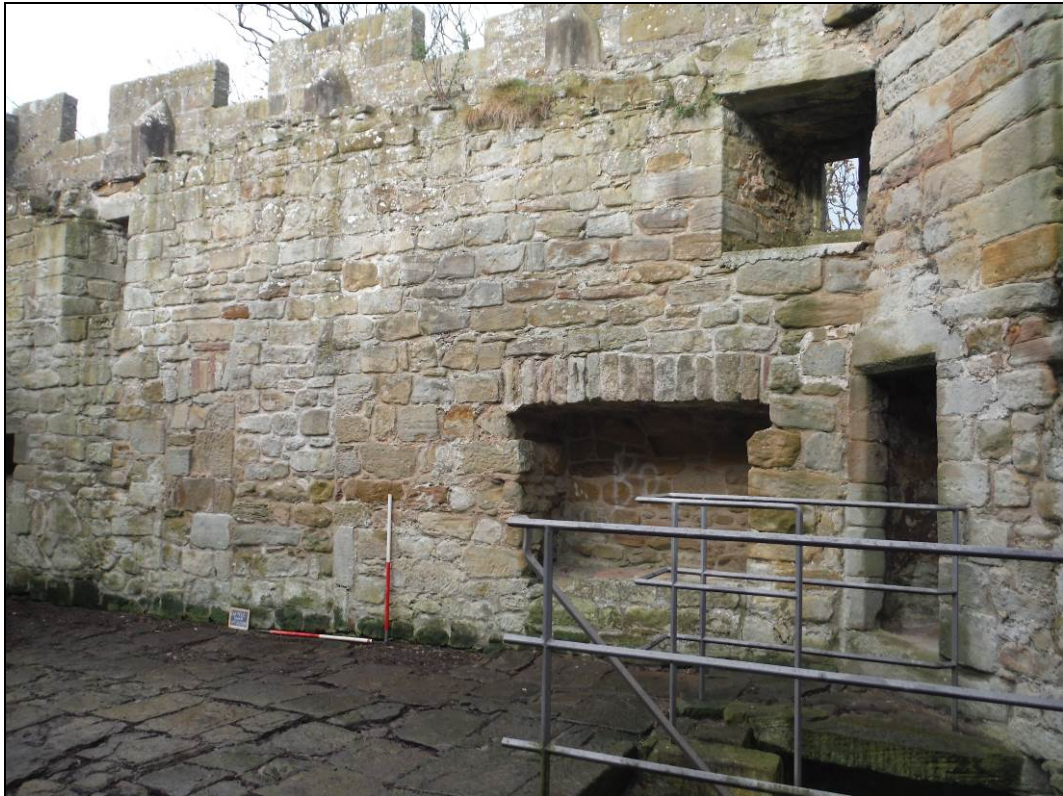
Figure 20. The northern extent of the north-western elevation of the pele tower's first floor. Scales = 2 x 1m.
