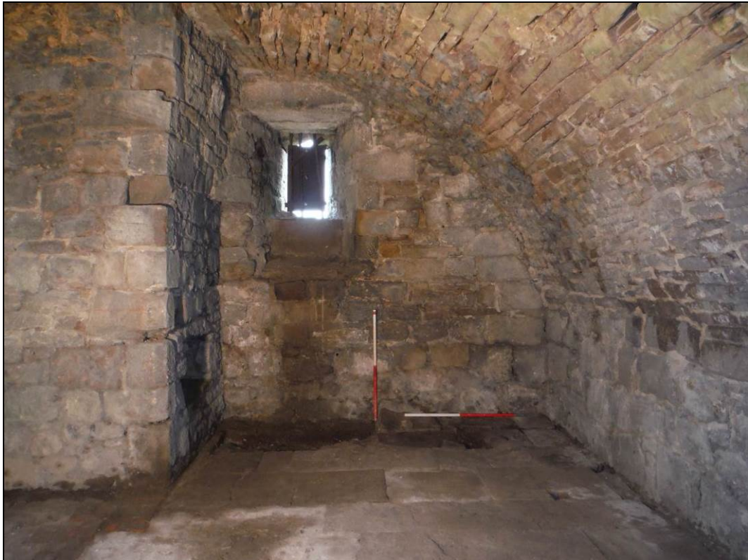
Figure 6. The recess behind the staircase within the ground floor of the pele tower. Scales = 2 x 1m.
