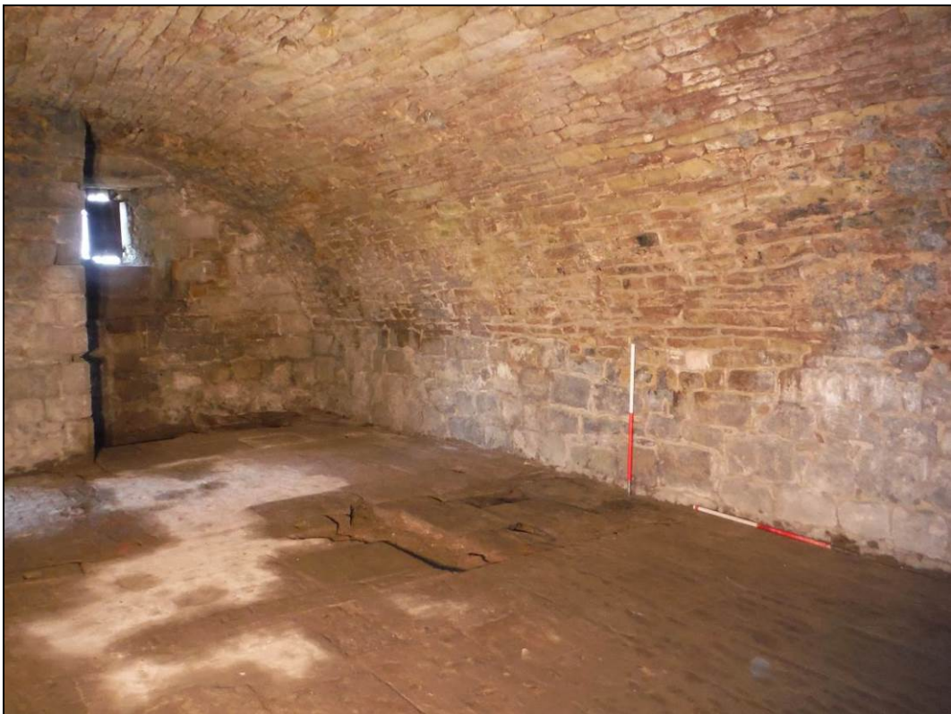
Figure 9. The south-eastern elevation of the pele tower's ground floor. Scales = 2 x 1m.
