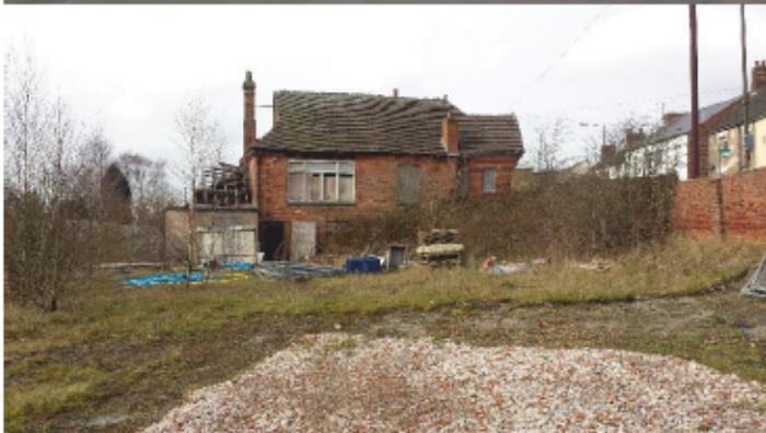
Photograph shows the Existing condition of the Grade II Listed building which sits adjacent to the site
