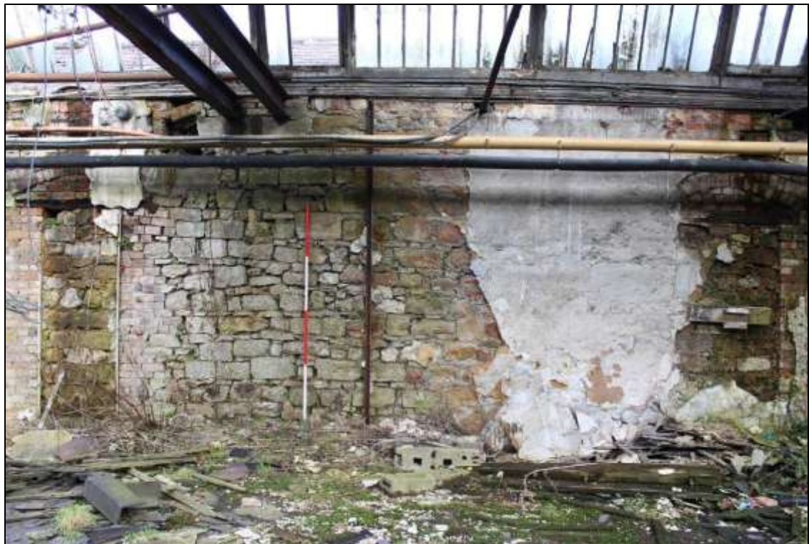
Figure 69: View of the northern wall of the western section of the northern wall of the former mule spinning shed.
