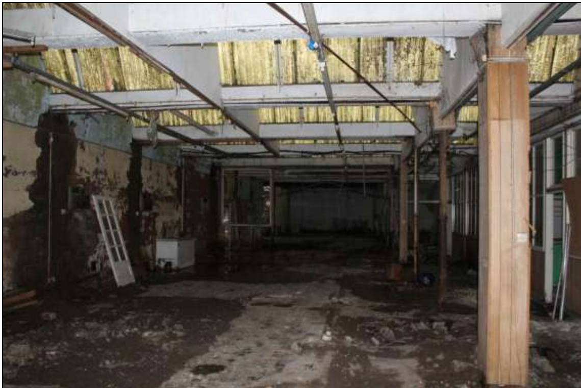
Figure 61: View of the eastern section of the former mule spinning shed, facing north.
