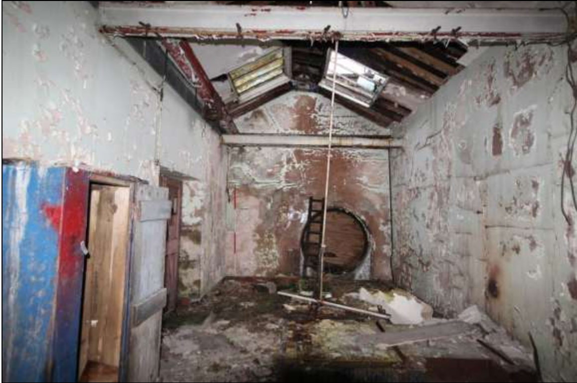
Figure 84: View of the circular hole in the eastern wall of the former plant room which would have held a turbine, 2m scale.
