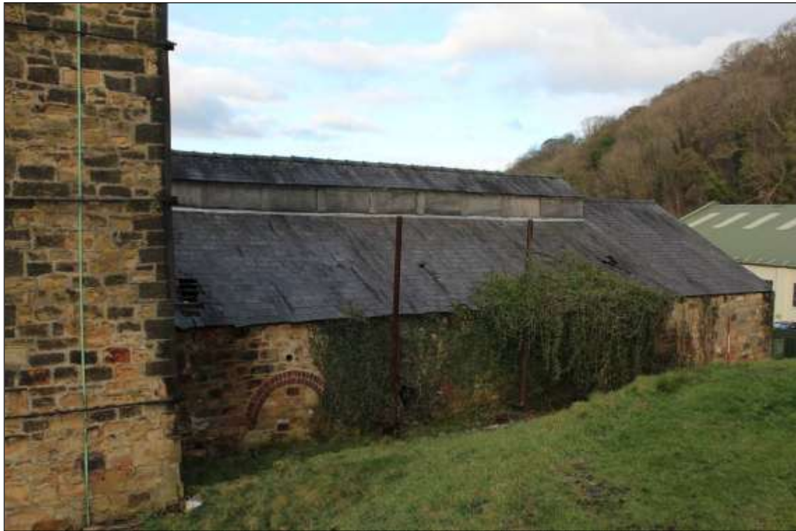
Figure 88: General view of the eastern elevation of the retort house, facing north west, 2m scale.
