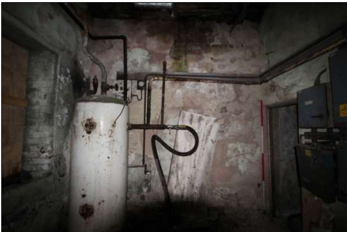
Figure 51: View of a utilities room to the north of the main mule spinning shed, 2m scale.
