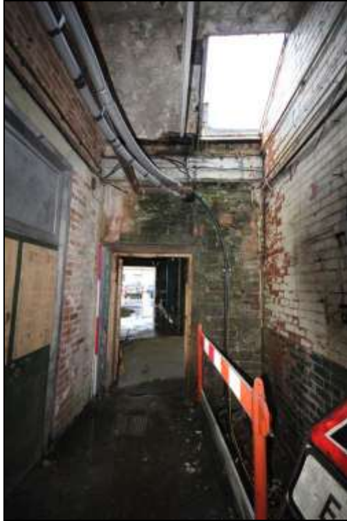
Figure 54: View of the later inserted passageway connecting the former mule spinning shed to the adjacent northern building, 2m scale.
