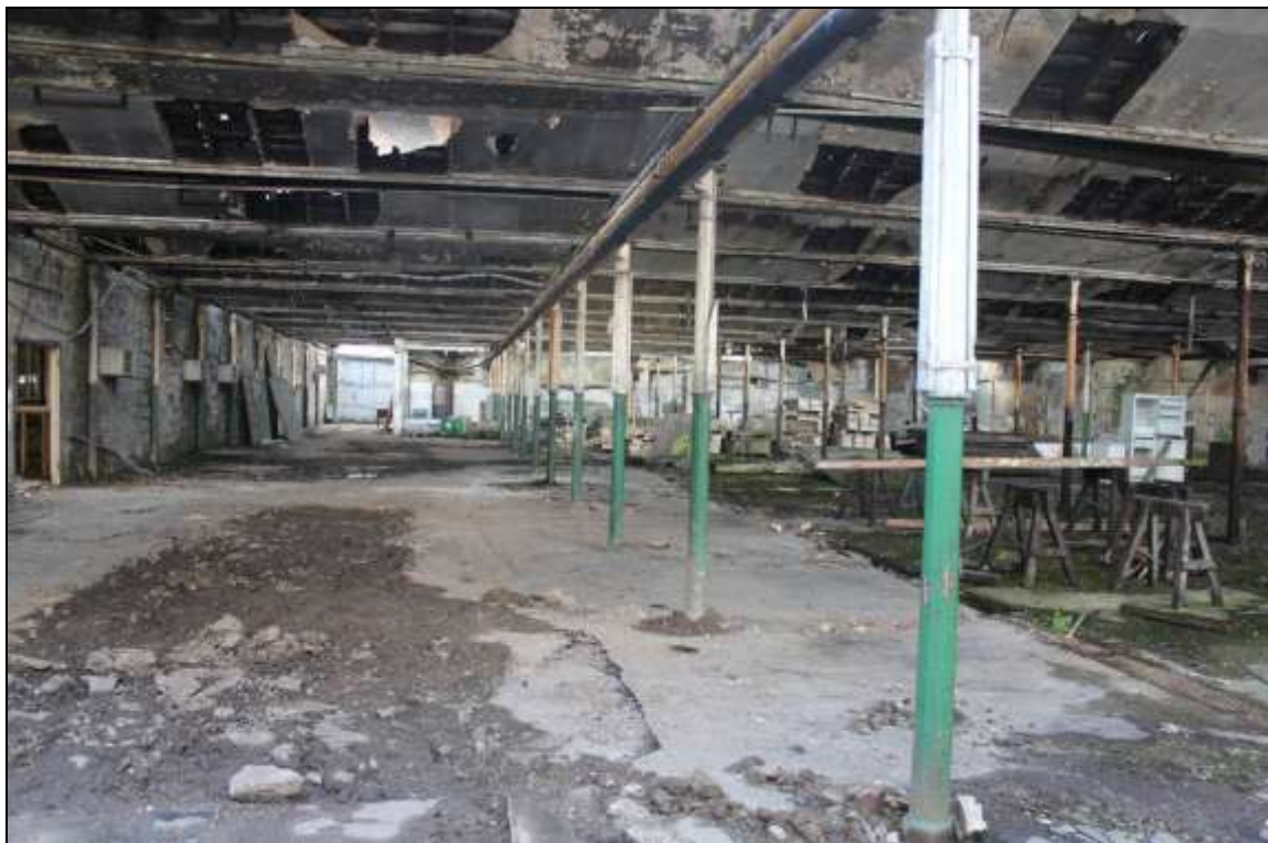
Figure 33: General view of the interior of the western section of the former mule spinning shed, facing south west.
