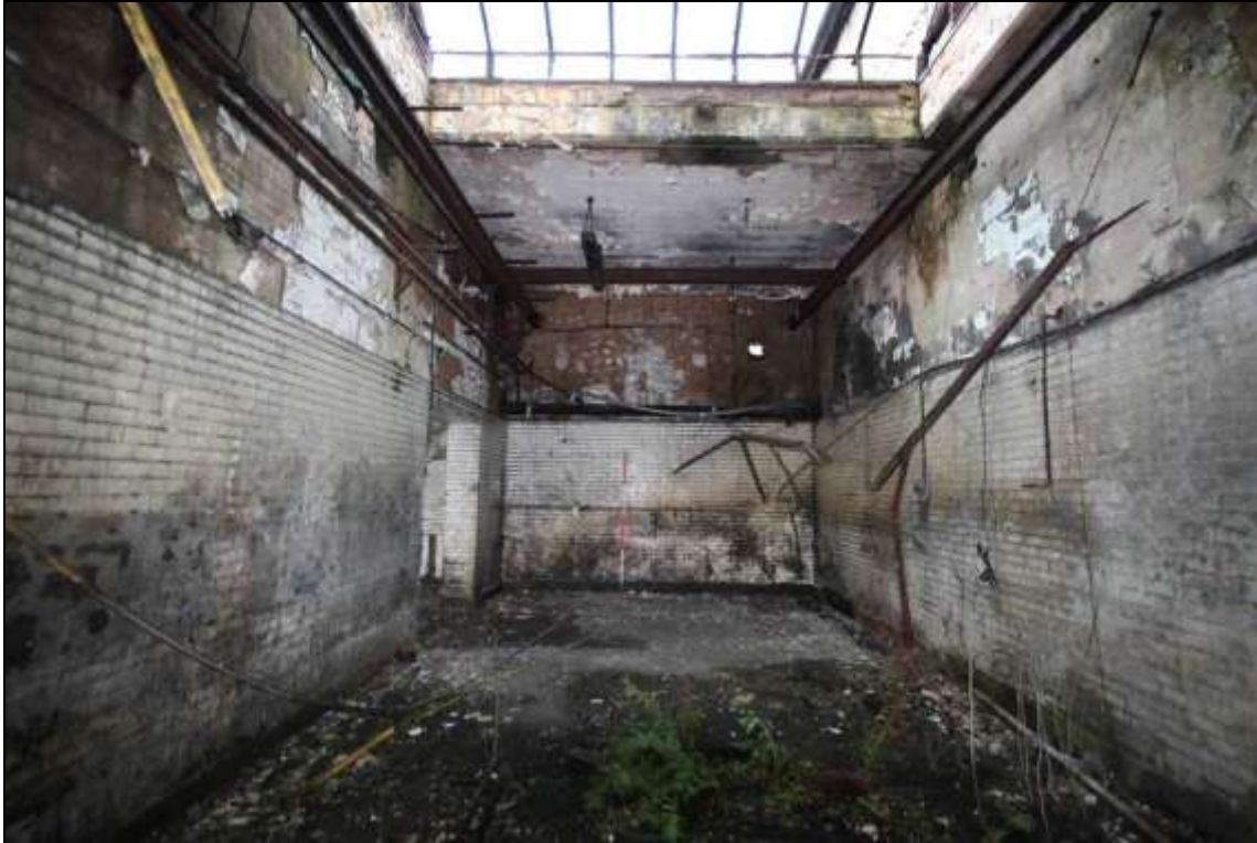
Figure 80: View of the south west corner of the former mule spinning shed with glazed tiles, 2m scale.
