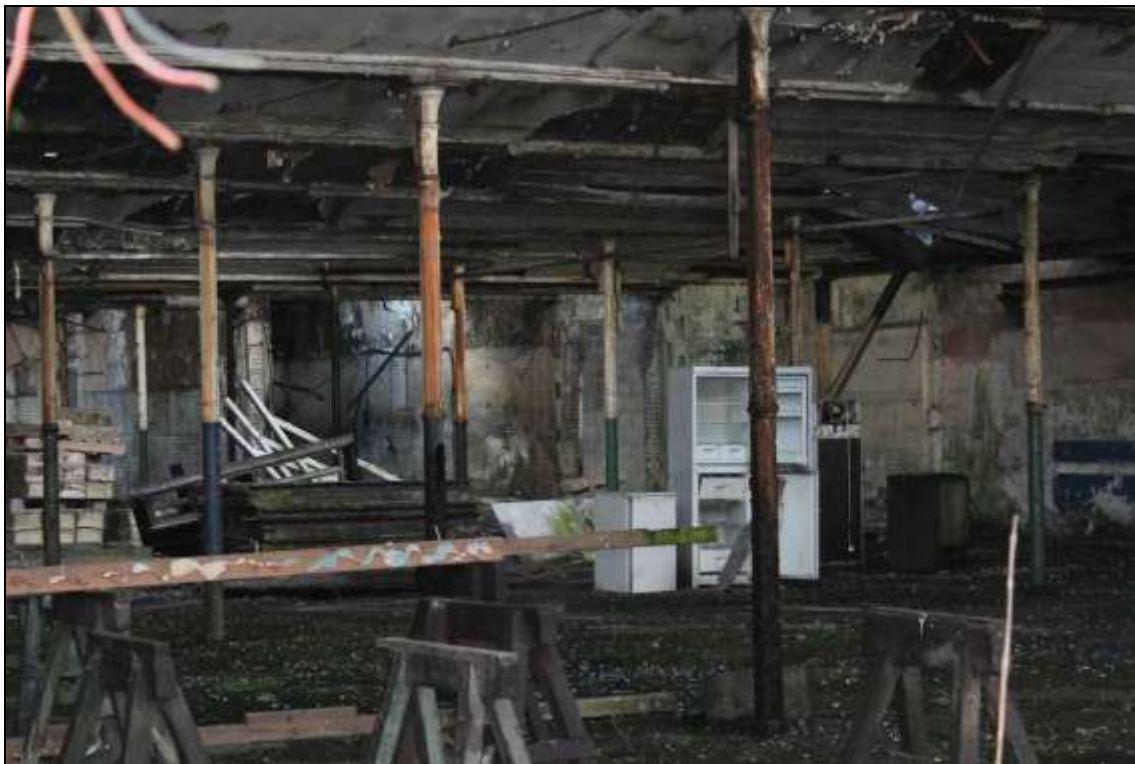
Figure 35: View of the interior of the former mule spinning shed, facing south west.
