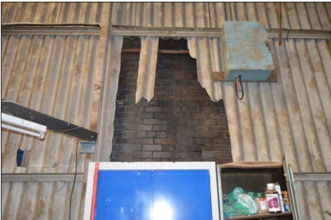
Figure 147: Detail view of the exposed brickwork to the lower section of the chimney east elevation.
