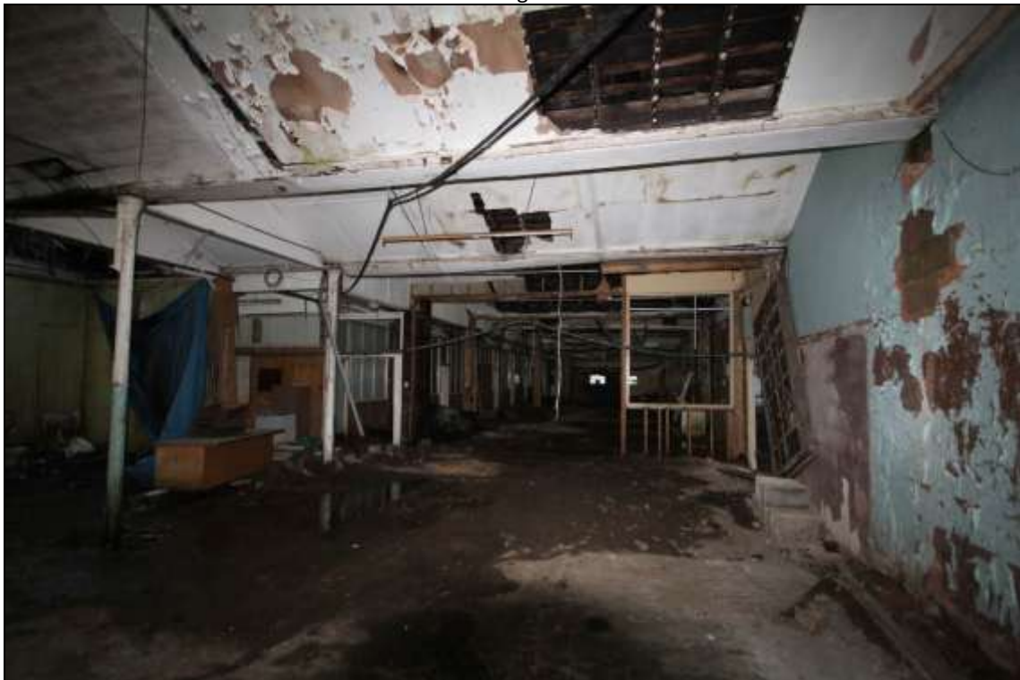
Figure 65: View of the eastern section of the former mule spinning shed, facing south.
