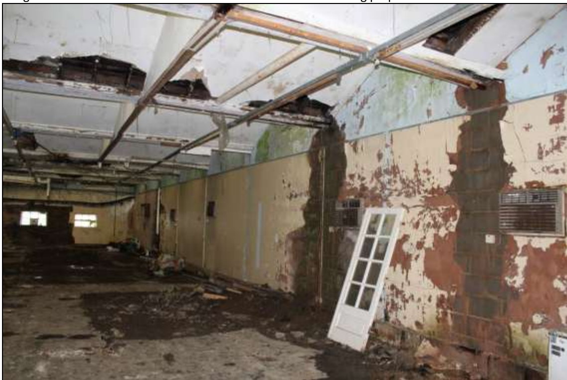
Figure 49: View of the later inserted concrete breeze block wall, facing south west.
