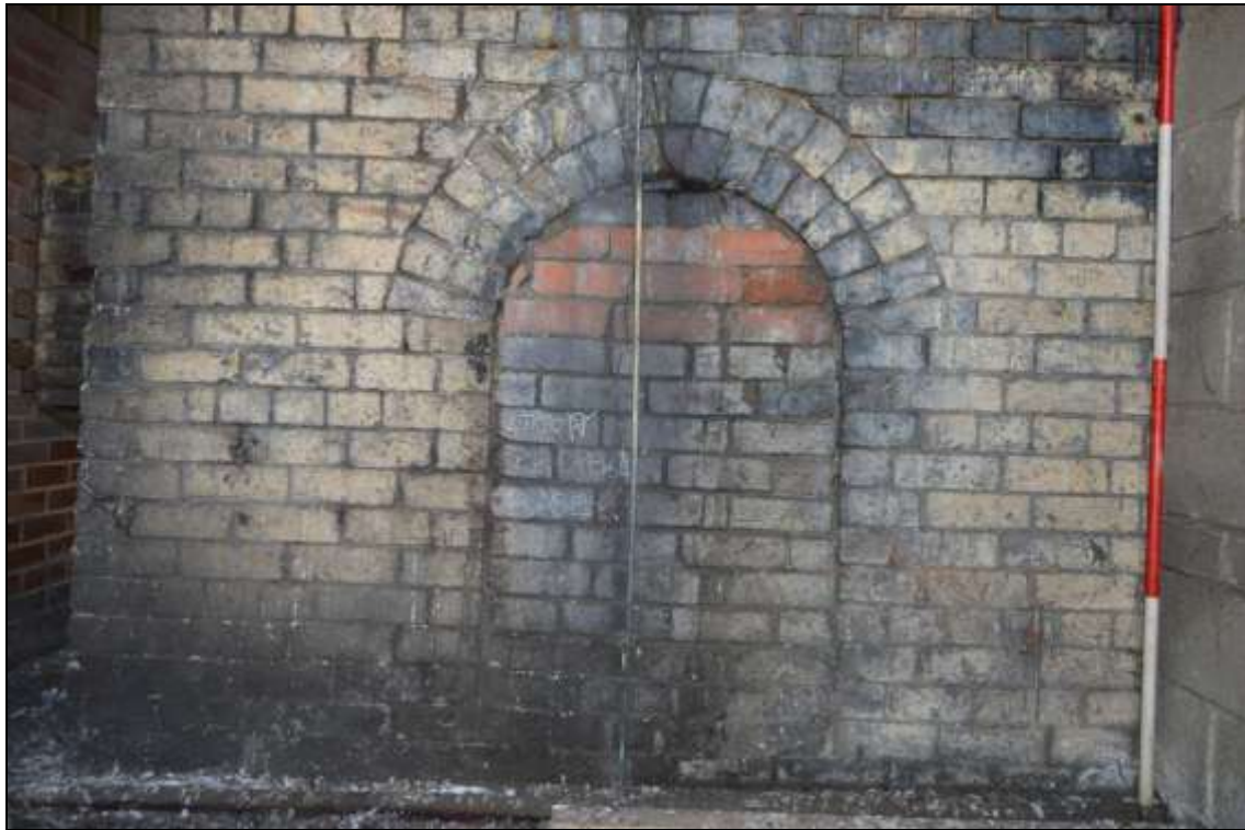
Figure 142: Detail of arch at the base of the brick chimney's west elevation, 2m scale.
