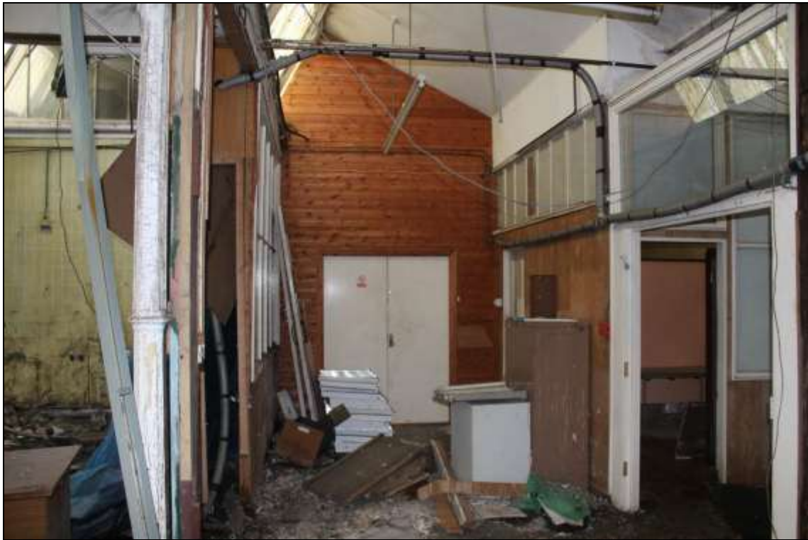
Figure 64: View of the inserted doorway allowing access between the former mule spinning shed and Fearnough House.
