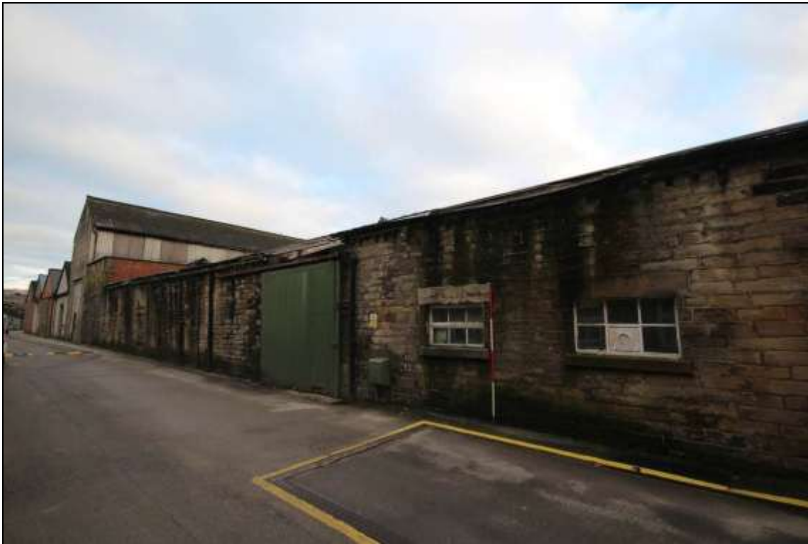
Figure 18: View of the southern elevation of the mule spinning shed, facing north west, 2m scale.
