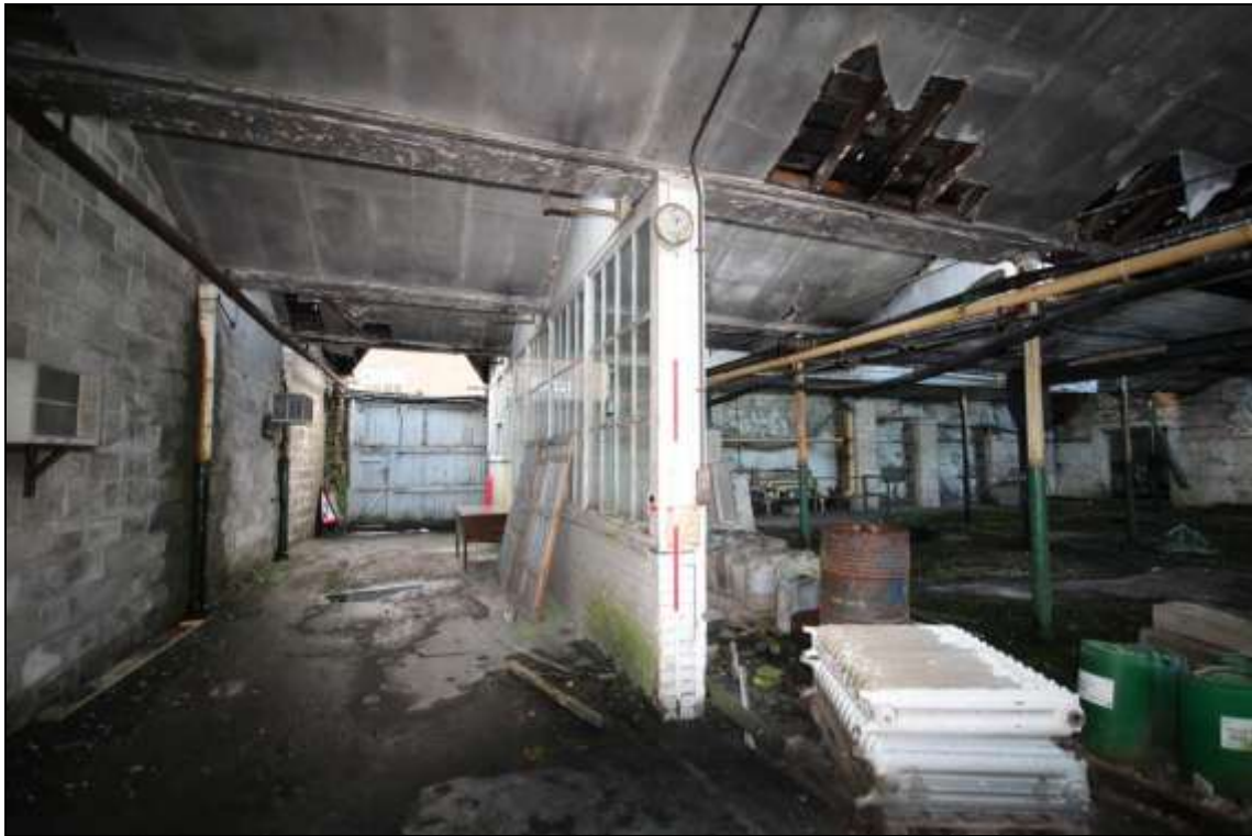
Figure 46: View of two inserted walls projecting from the southern wall to form a passageway, 2m scale.
