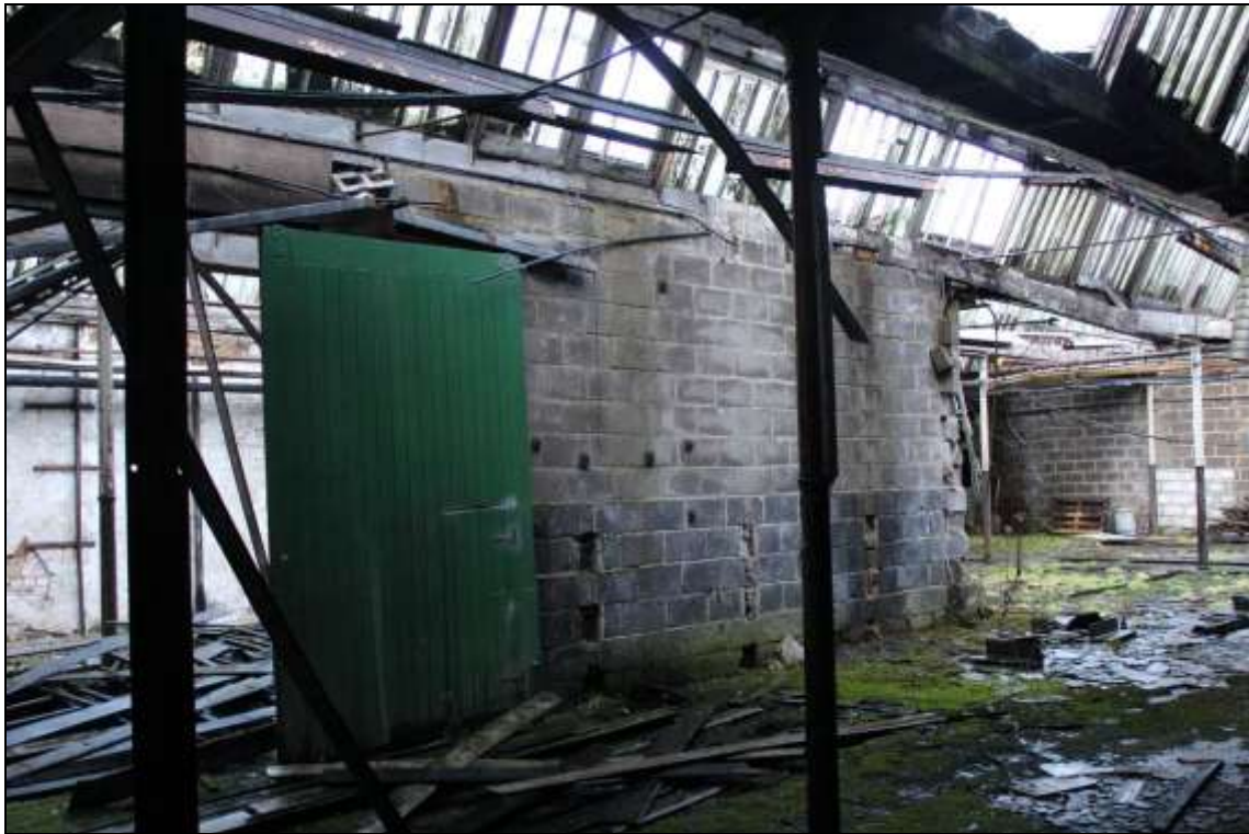
Figure 48: View of an inserted concrete breeze block wall running perpendicular to the western wall.
