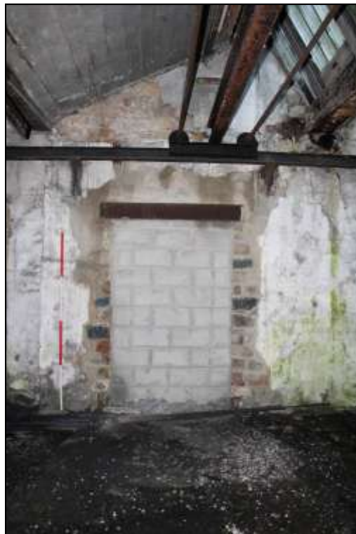
Figure 79: View of a later inserted aperture along the west wall of the former mule spinning shed, 2m scale.
