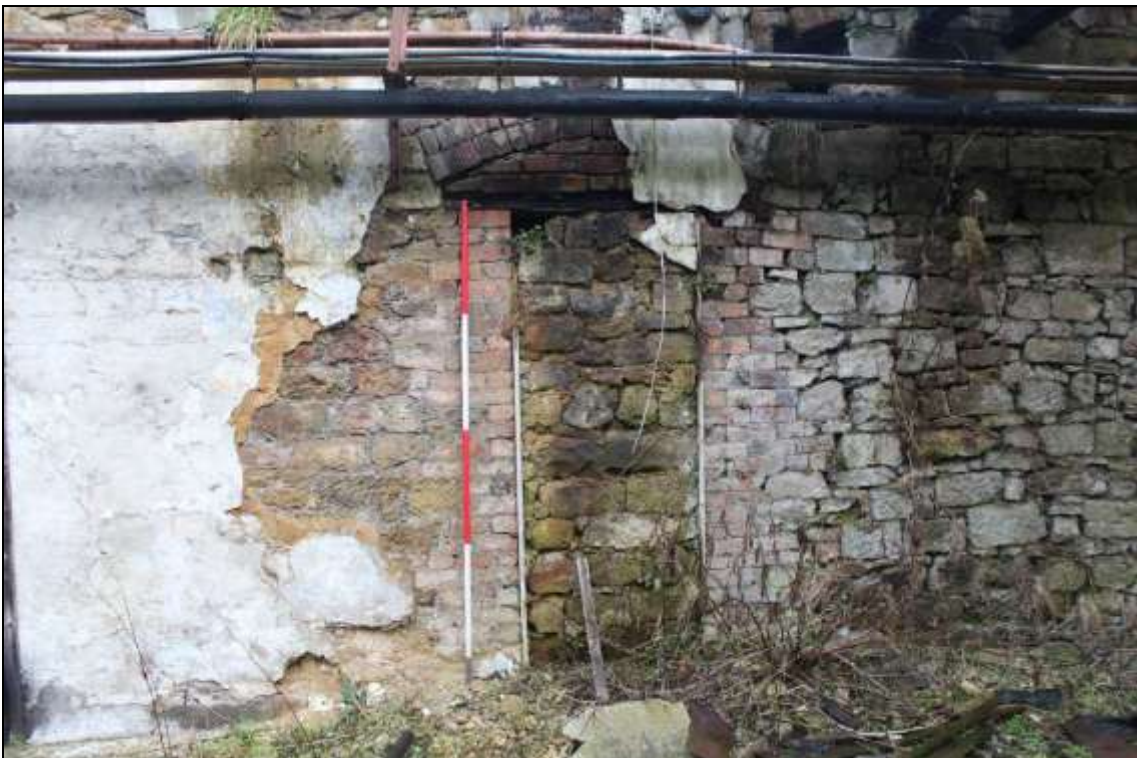
Figure 73: View of the modified northern wall of the former mule spinning shed, 2m scale.
