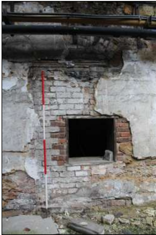
Figure 74: Numerous modified aperture along the northern wall of the former mule spinning shed, 2m scale.
