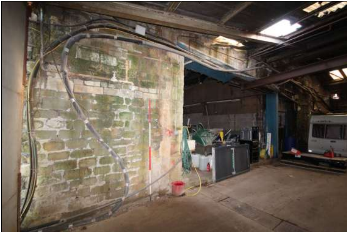
Figure 94: General view of the heavily modified western elevation of the retort house, 2m scale.
