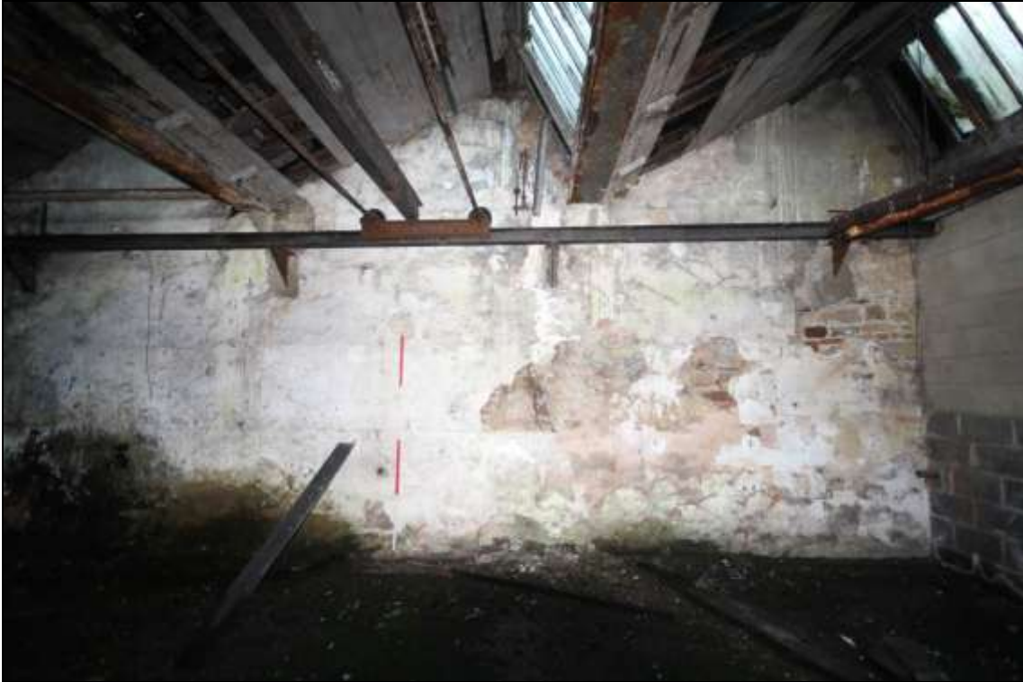
Figure 76: View of a section of the western wall covered in plaster, facing west, 2m scale.
