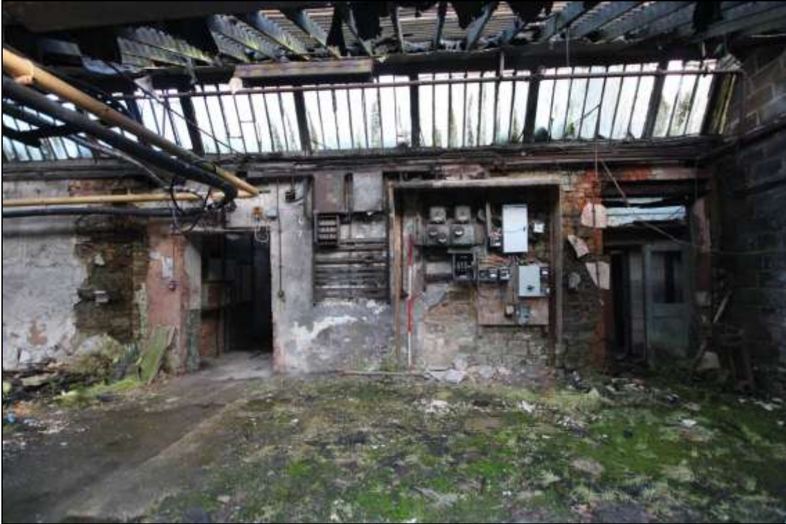
Figure 72: View of the modified northern wall of the former mule spinning shed, 2m scale.
