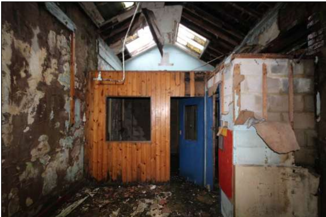
Figure 55: View of an inserted office block to the north of the mule spinning shed.
