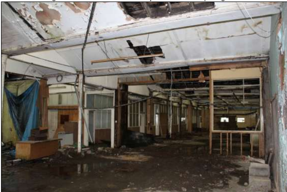
Figure 59: View of the eastern section of the former mule spinning shed with inserted stud offices.
