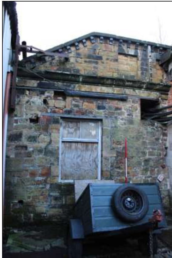
Figure 24: View of a section of the western elevation, showing detailing mirroring that of the eastern elevation and a modified doorway, 2m scale.
