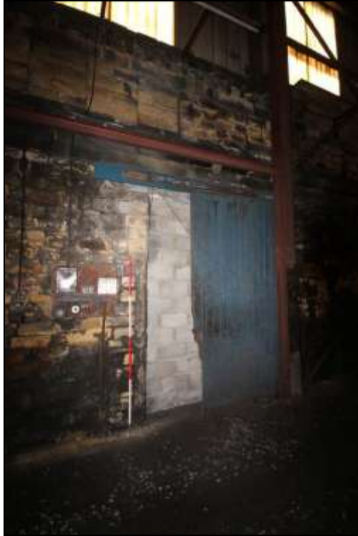
Figure 28: View of a blocked doorway along the former western elevation, 2m scale.
