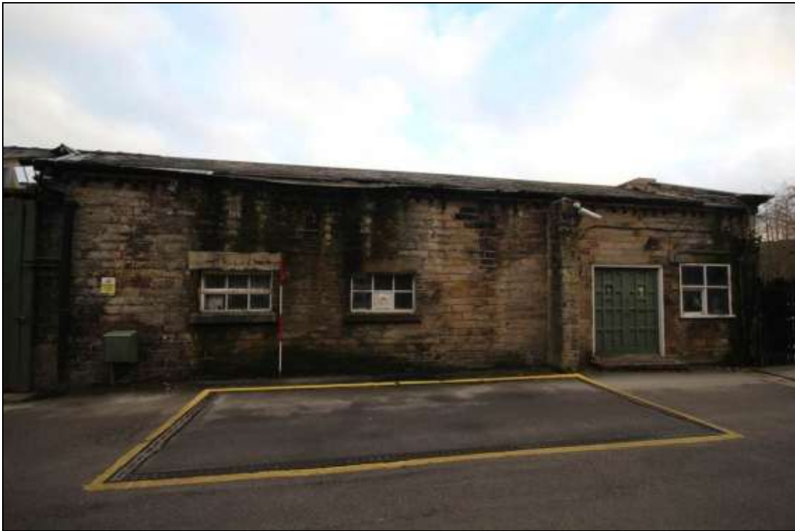
Figure 16: View of the weighing bridge adjacent to the south elevation of the former mule spinning shed, 2m scale.
