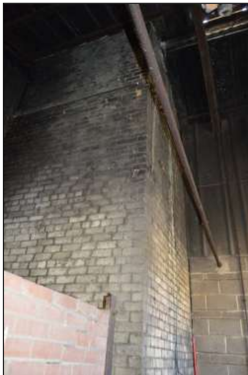
Figure 143: View of the lower north and west elevations of the brick chimney.
