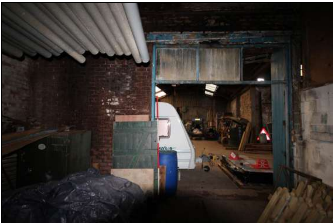
Figure 105: View of a later inserted large opening in the western wall of the retort house, 2m scale.
