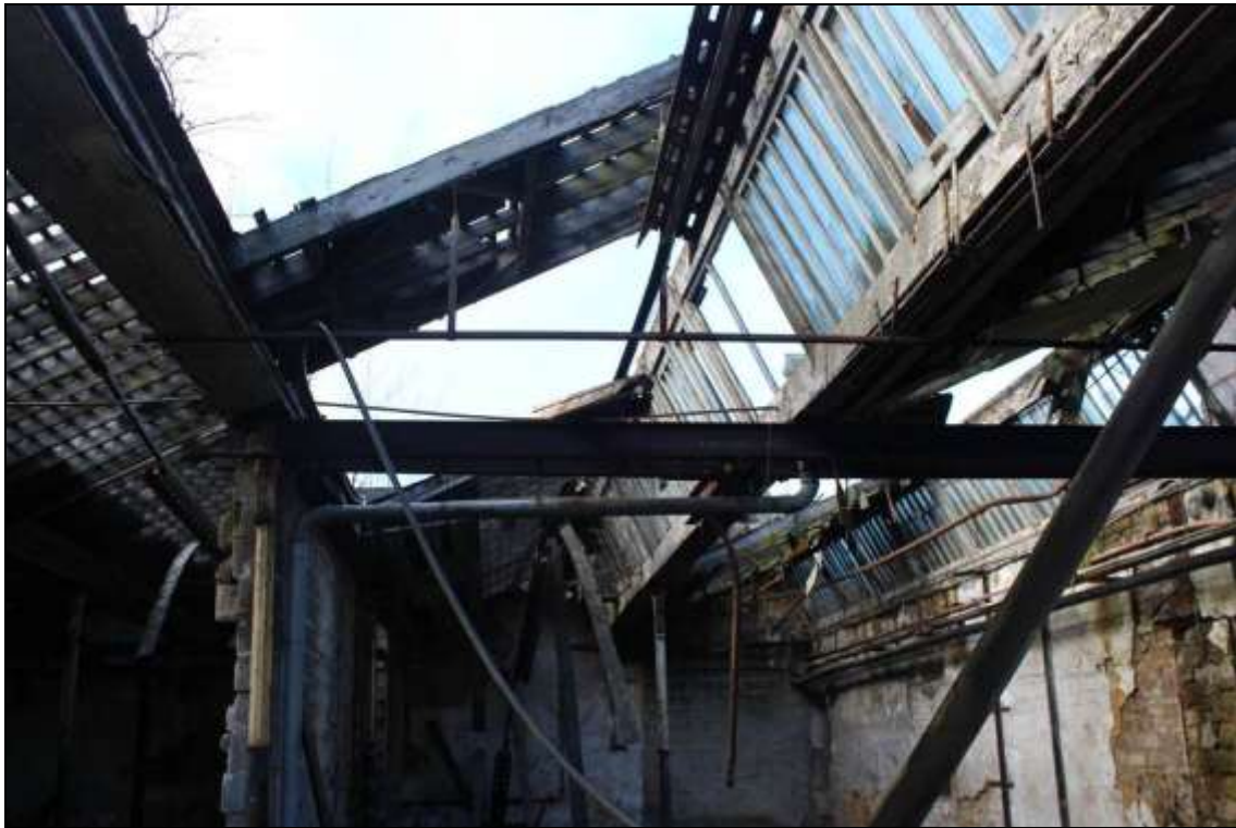
Figure 42: View of the deteriorating roof of the former mule spinning shed.
