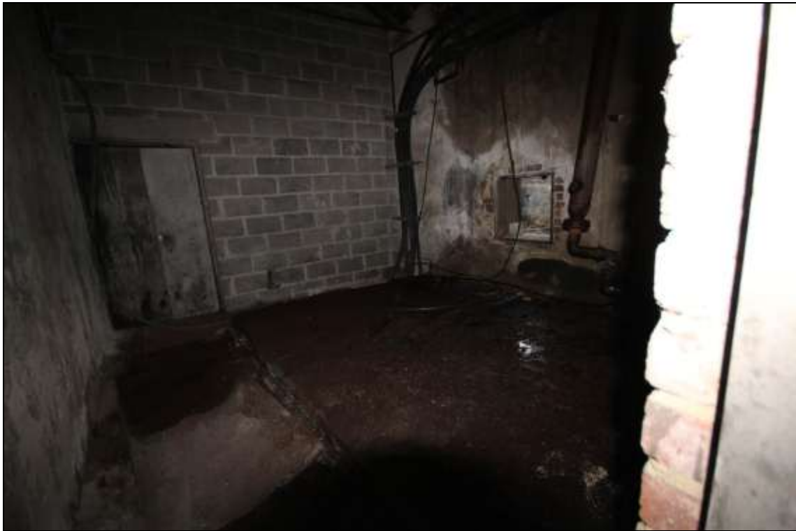
Figure 50: View of a room to the north of the main interior of the former mule spinning shed.
