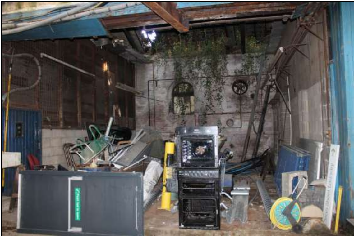
Figure 98: General view of the interior of the modified retort house, facing east.
