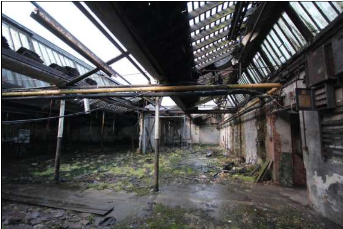
Figure 36: View of the northern portion of the former mule spinning shed, facing west.
