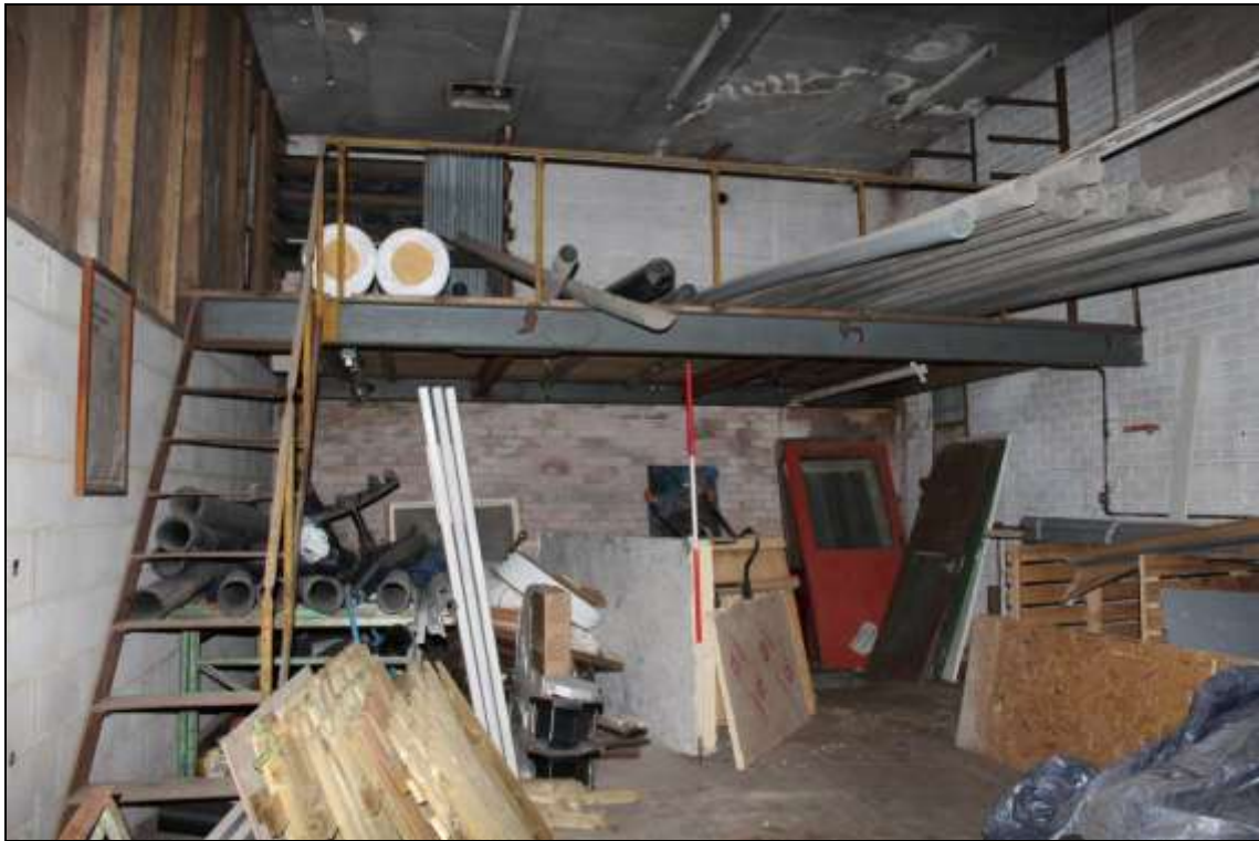
Figure 104: View of the southerly later created room of the Retort House, 2m scale.
