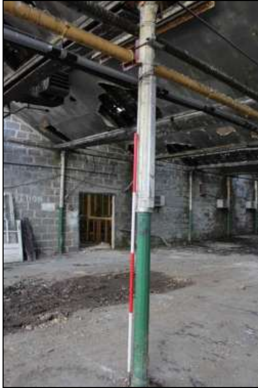
Figure 44: View of one of the cast-iron columns in the former mule spinning shed, 2m scale.
