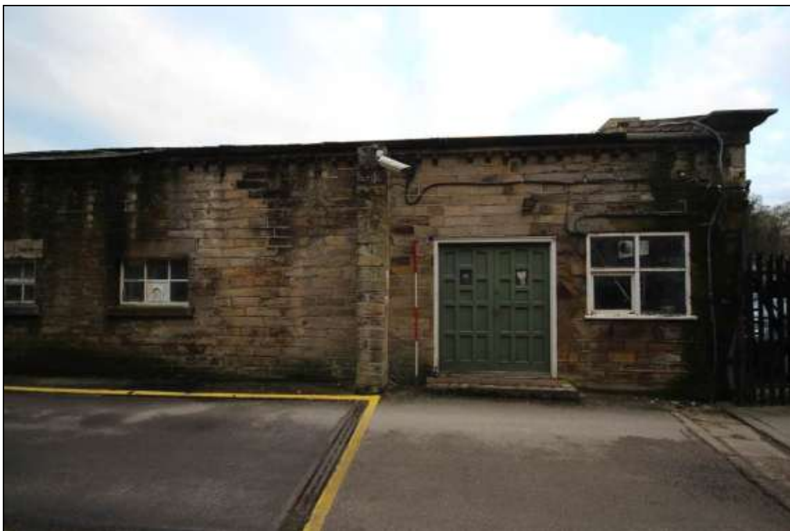
Figure 15: View of the easternmost section of the south elevation of the mule spinning shed, 2m scale.
