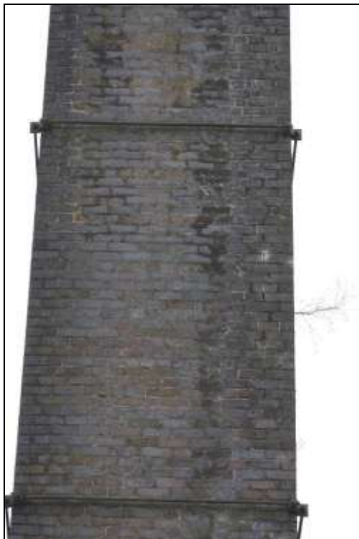
Figure 135: View of the northern elevations of the brick chimney at Riverside Business Park, Bakewell.
