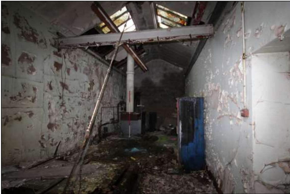
Figure 56: View of the former plant room with an inserted concrete breeze block western wall, 2m scale.
