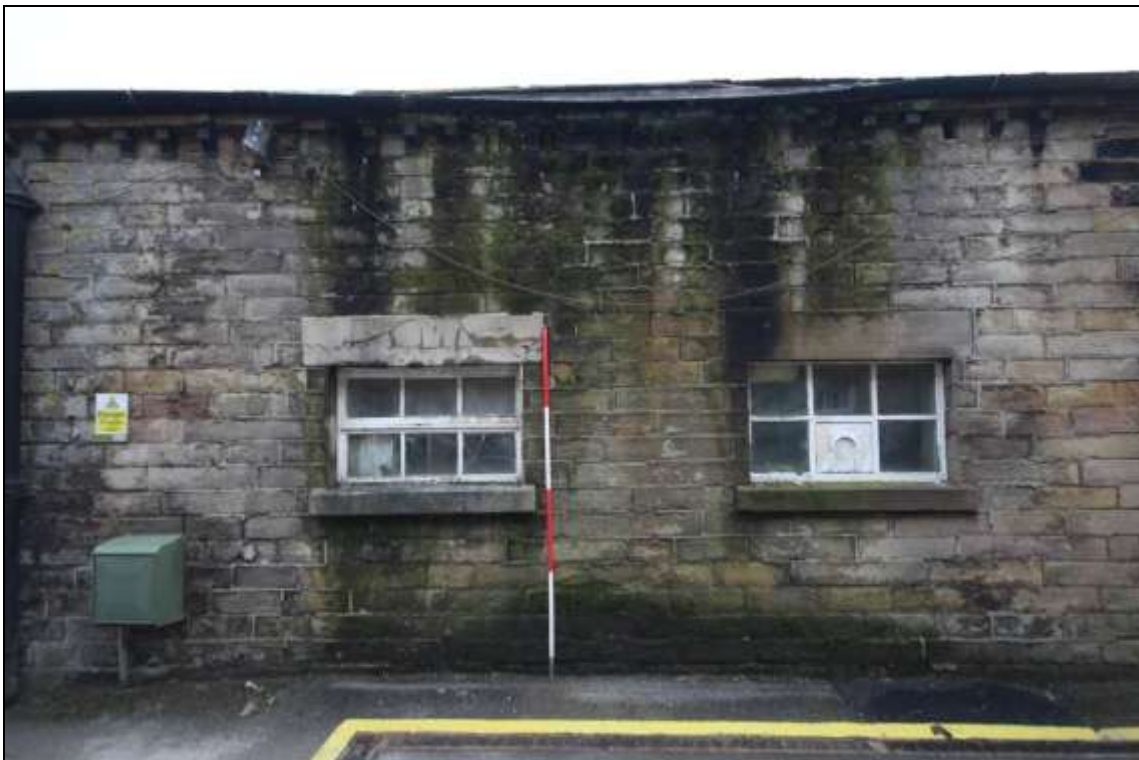
Figure 17: View of a later inserted window along the southern elevation of the former mule spinning shed, 2m scale.
