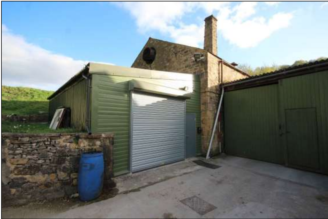
Figure 92: View of the northern elevation with a later lean-to addition, 2m scale.
