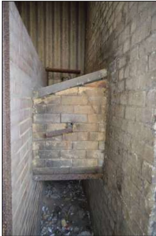
Figure 144: View of a connecting flue in lower north elevation of the brick chimney (right).
