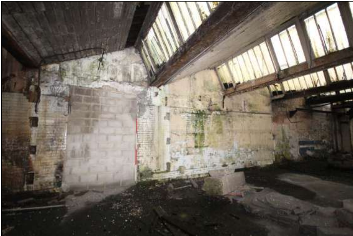
Figure 78: View of a section of the west wall of the former mule spinning shed, 2m scale.
