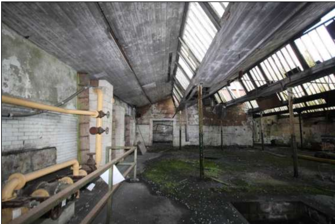
Figure 81: View of the southern section of the former mule spinning shed, facing west, 2m scale.
