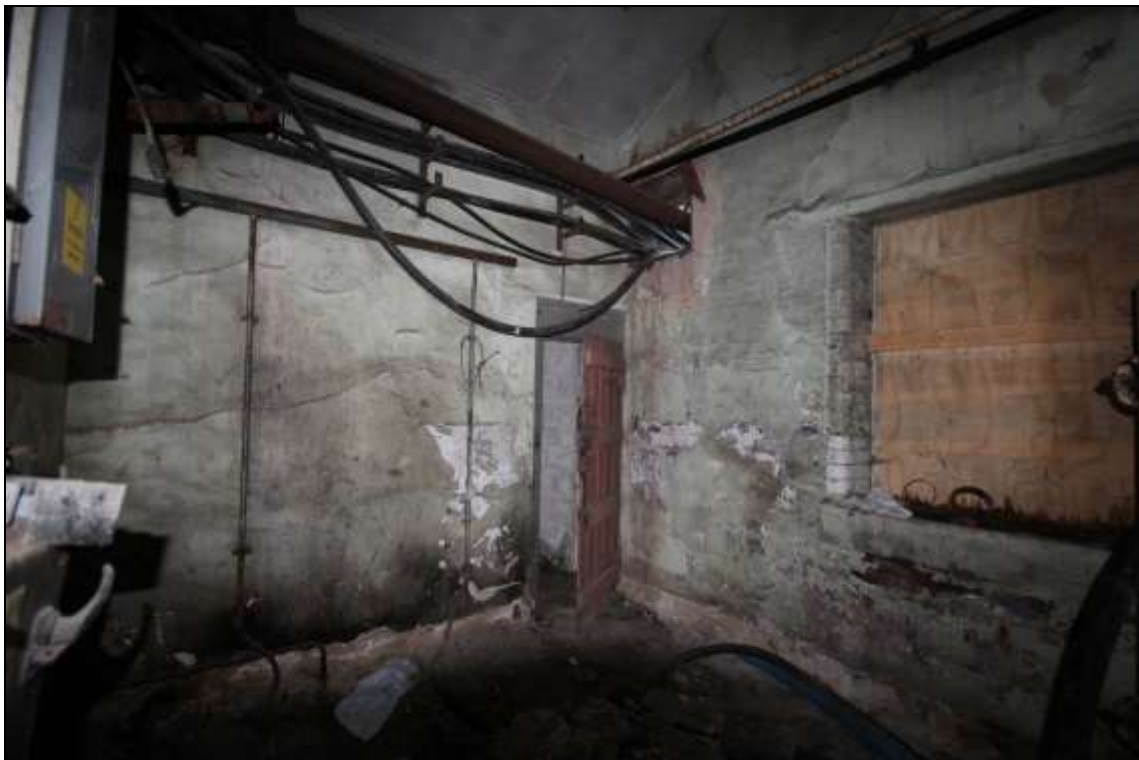
Figure 53: View of a utilities room to the north of the main mule spinning shed, 2m scale.
