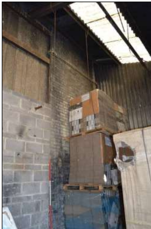
Figure 145: View of the lower section of the south elevation of the brick chimney, 2m scale.
