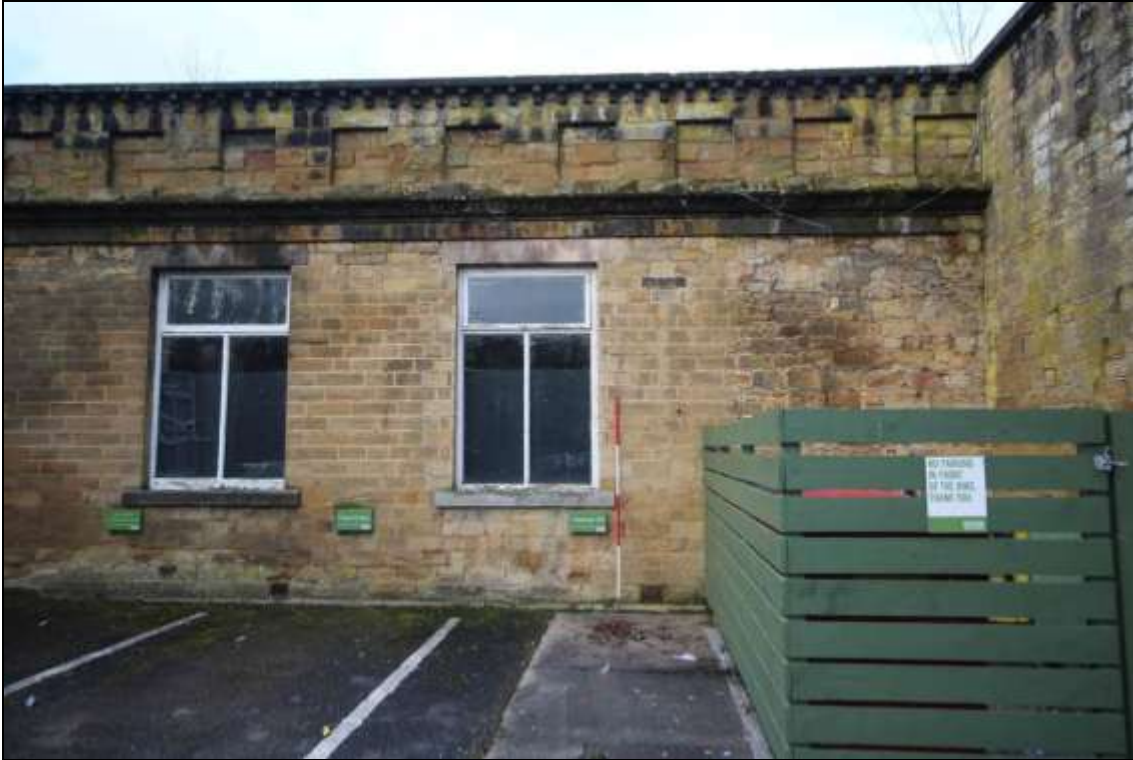
Figure 12: View of the 19th century sandstone blocks incorporated with the earlier 1777 structure, 2m scale.
