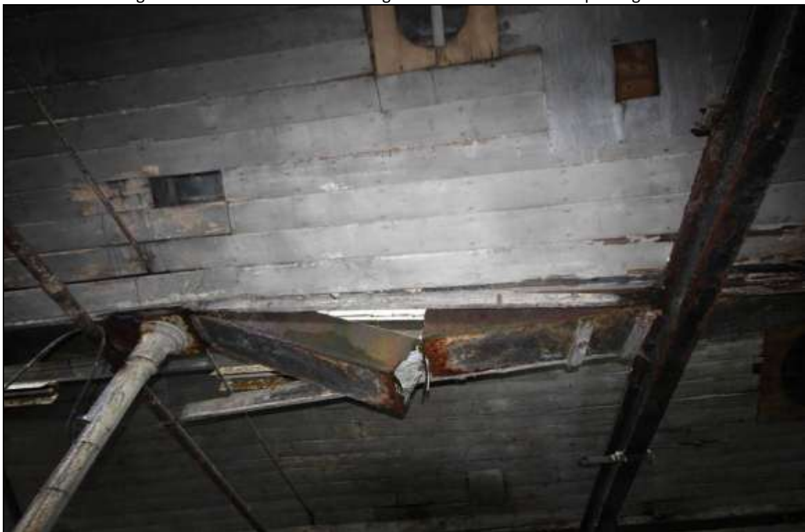
Figure 43: View of the deteriorating roof structure.
