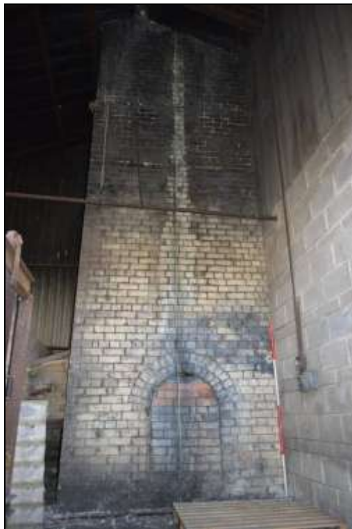
Figure 141: View of the lower section of the west elevation of the brick chimney from inside the surrounding buildings, 2m scale.
