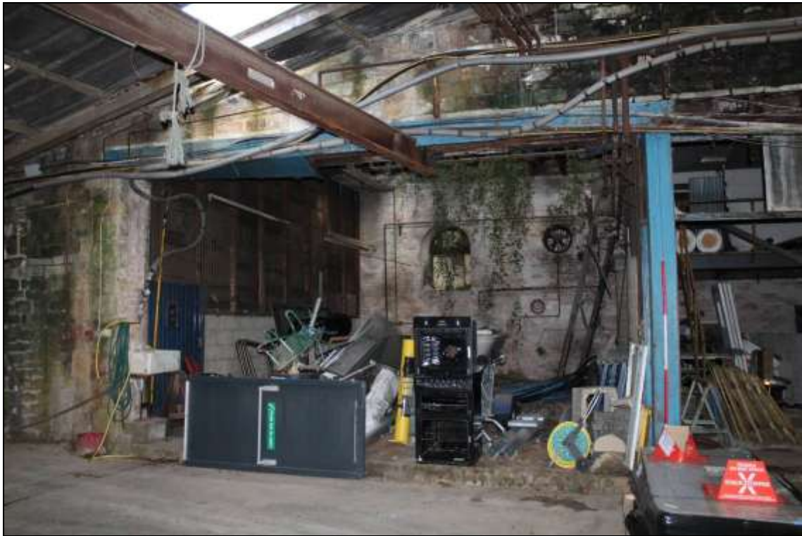
Figure 102: General view of the 'central' modified area of the Retort House, facing east, 2m scale.
