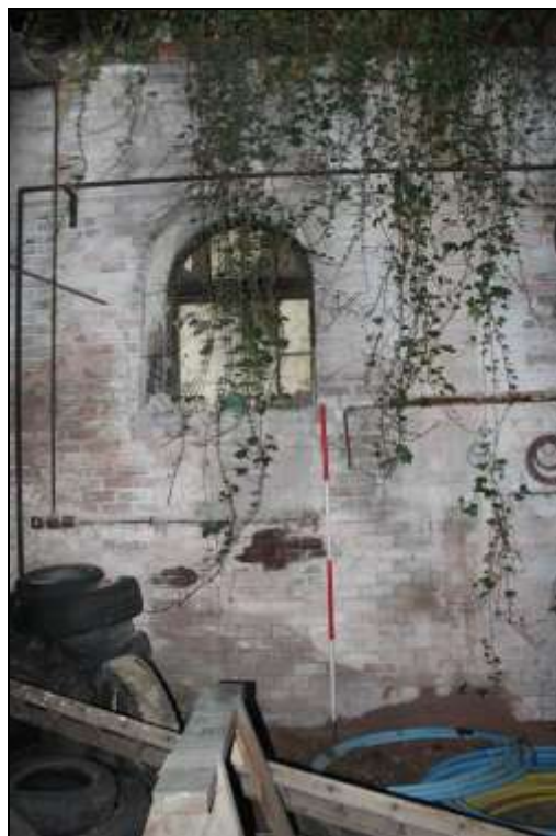
Figure 99: View of a blocked window along the eastern wall of the retort house, 2m scale.
