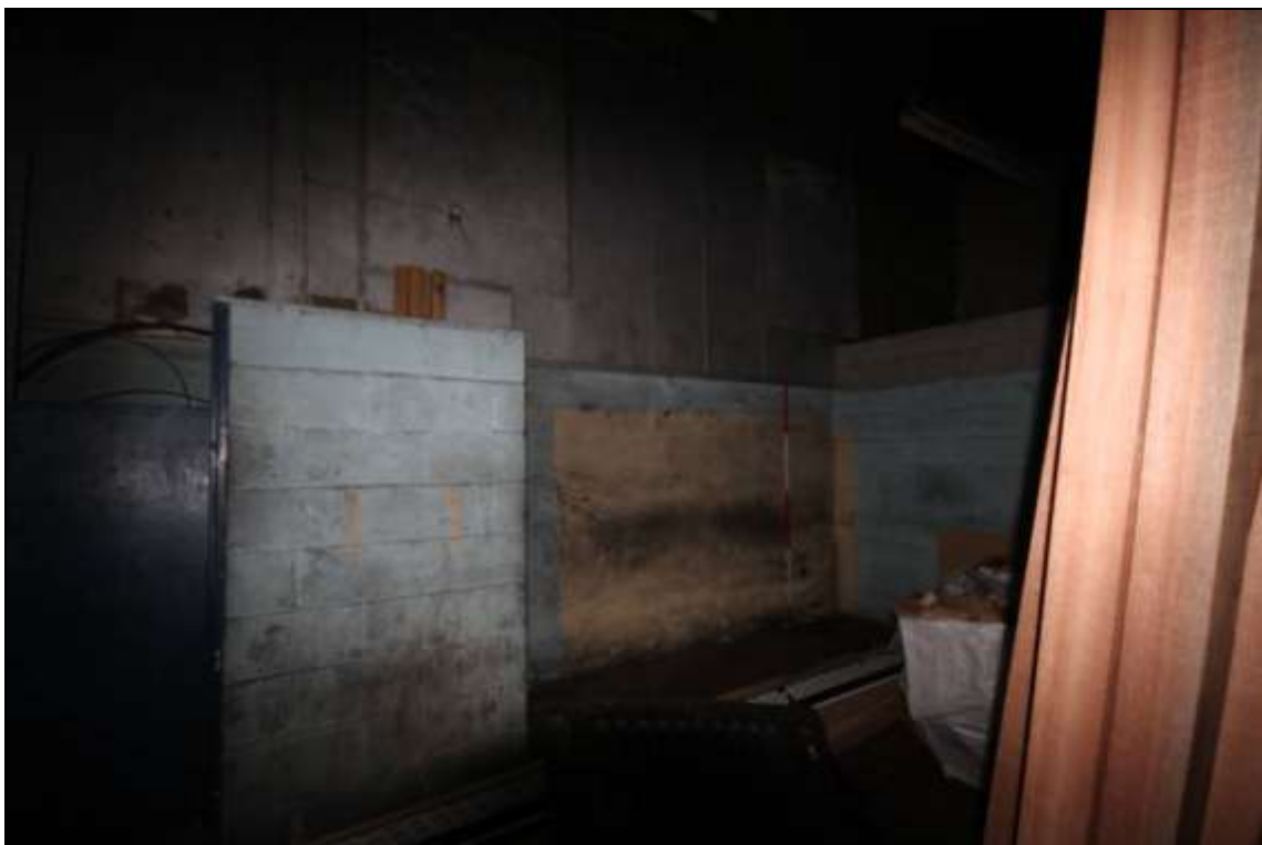
Figure 101: View of the northernmost later created room in the retort house, 2m scale.
