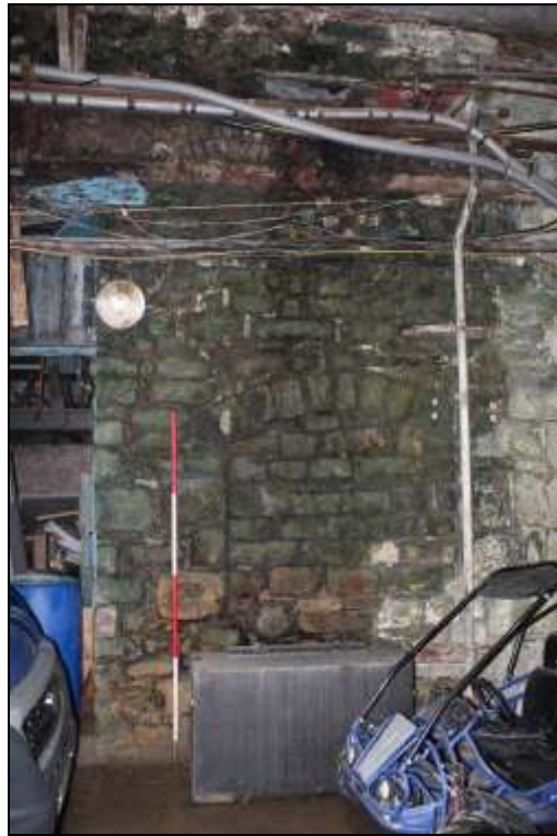
Figure 96: View of the segmental arched stone blocked doorway along the western elevation of the retort house, 2m scale.
