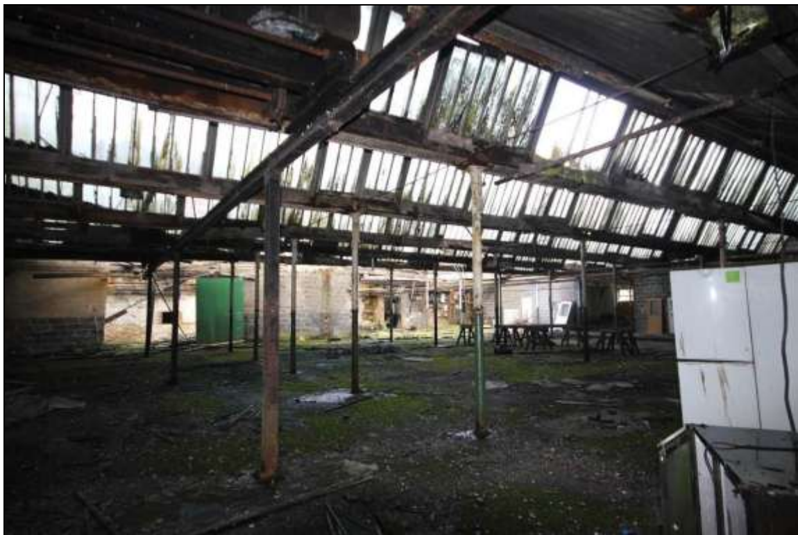
Figure 39: View of the interior of the former mule spinning shed, facing north east.
