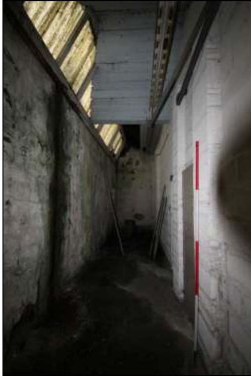
Figure 66: The insertion of a concrete breeze block wall has provided a separate room in the north east corner of the former mule spinning shed, 2m scale.
