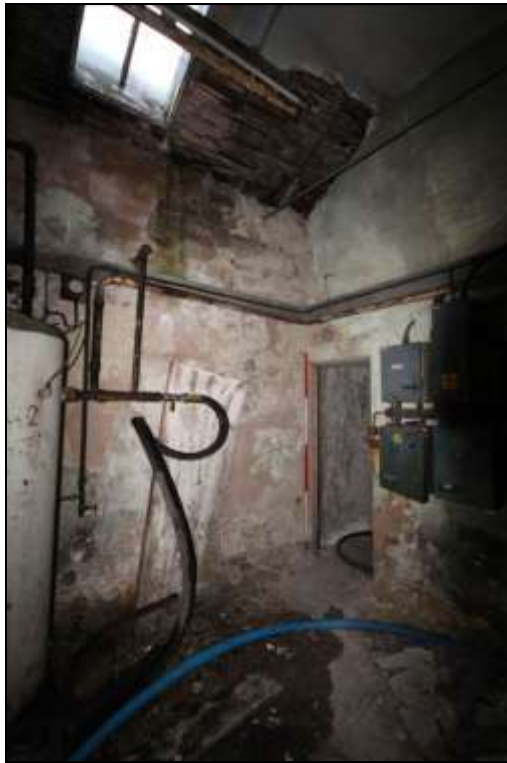
Figure 52: View of a utilities room to the north of the main mule spinning shed, 2m scale.
