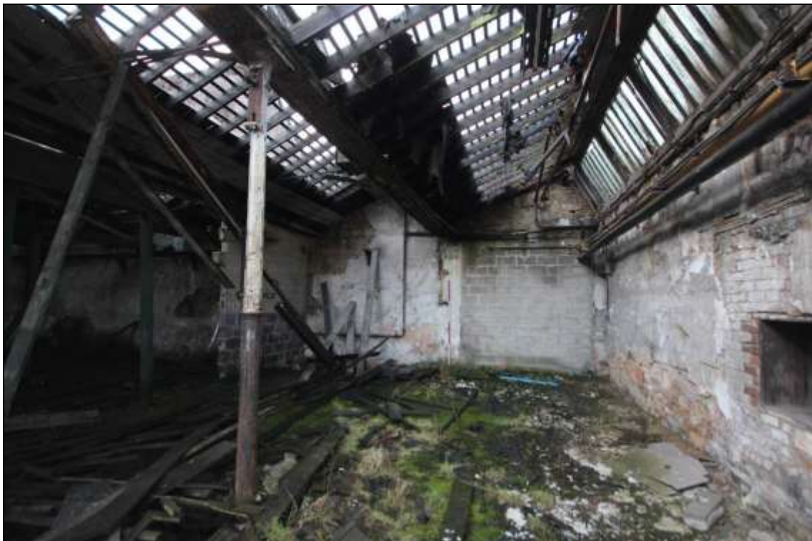
Figure 75: View of blocked aperture along the west wall of the former mule spinning shed, 2m scale.
