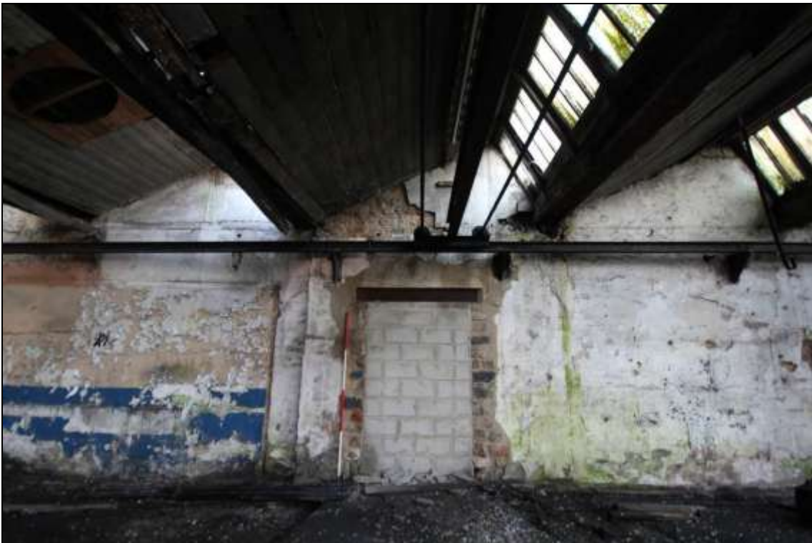
Figure 77: View of blocked aperture along the west wall of the former mule spinning shed, 2m scale.
