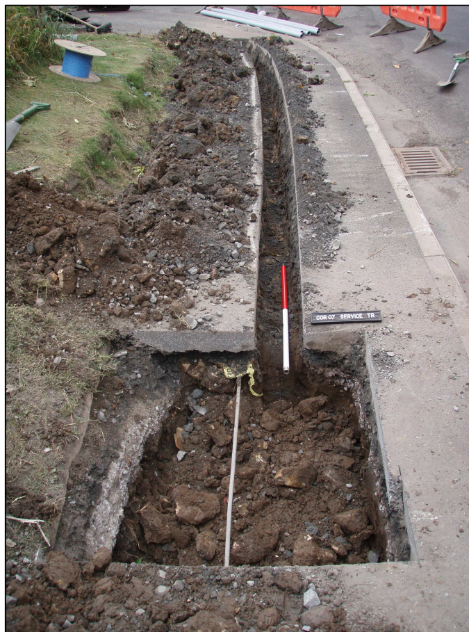
Fig. 3 Eastern end of trench, facing west, showing one meter square extension, scale = 1m
