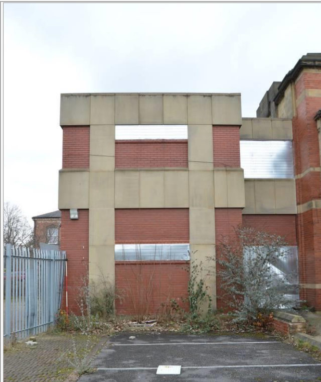
Plate 108.1: South elevation of the modern extension to the Canning wards (facing north west). Scale 2m.
