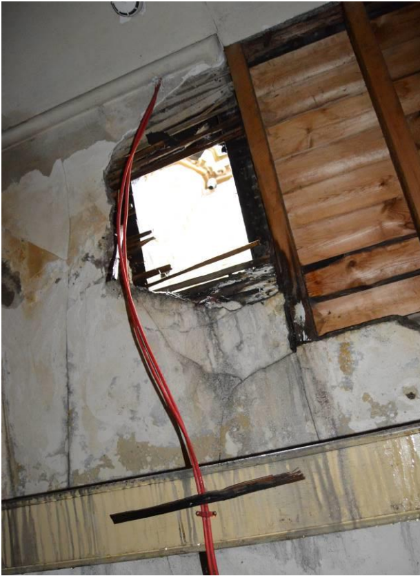
Plate 61.5: Damage to roof behind tower. Note later wood planks. Facing south east.
