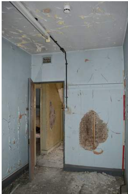
Plate 68.10: View within room S12, note the mesh construction behind the plaster. Scale 2m.
