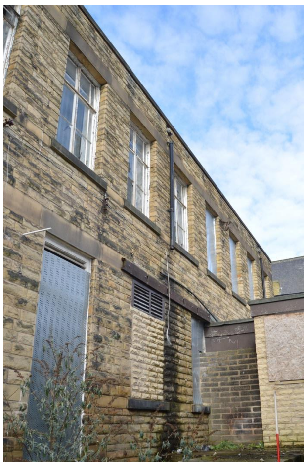
Plate 72.1: South elevation of the service wing extension, looking north west. Scale 2m.
