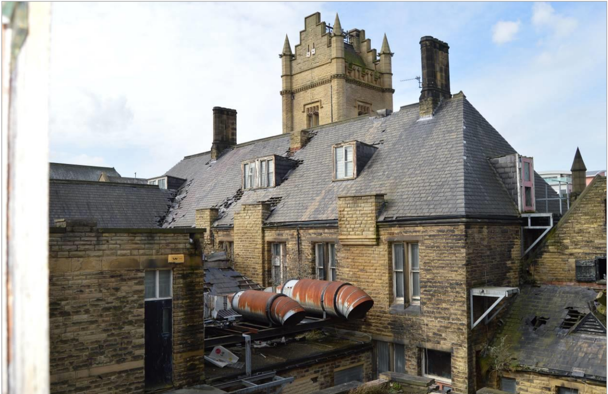
Plate 16: Rear view of the administration range looking north west. Note the truncated and capped chimney flues along the line of the eaves. Facing west.
