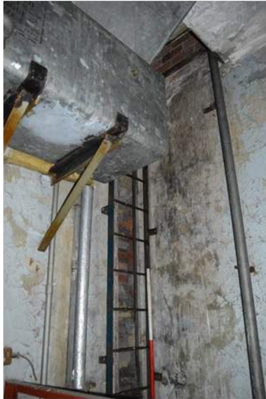
Plate 64.2: Later water tank to second floor tower room. Scale 2m.
