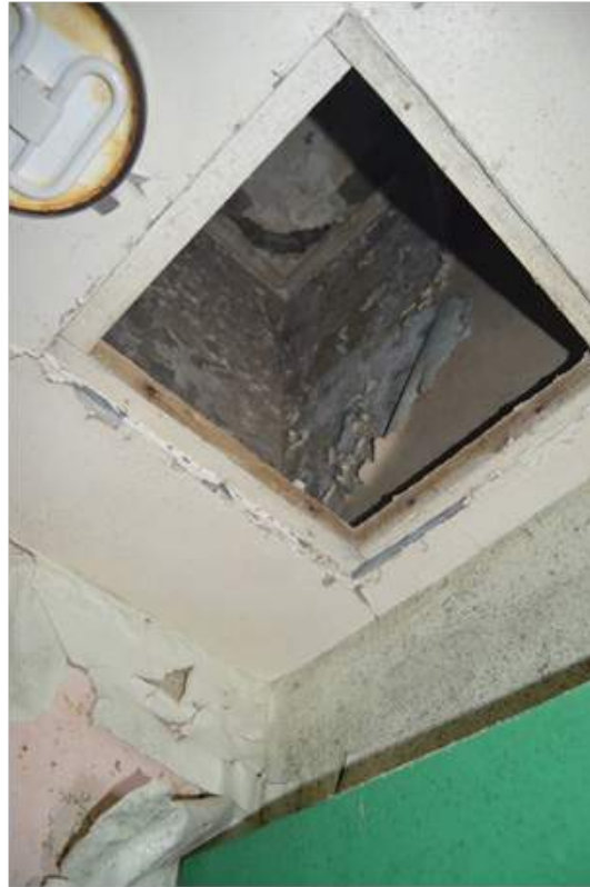
Plate 39: View of plaster coving to the museum room.
