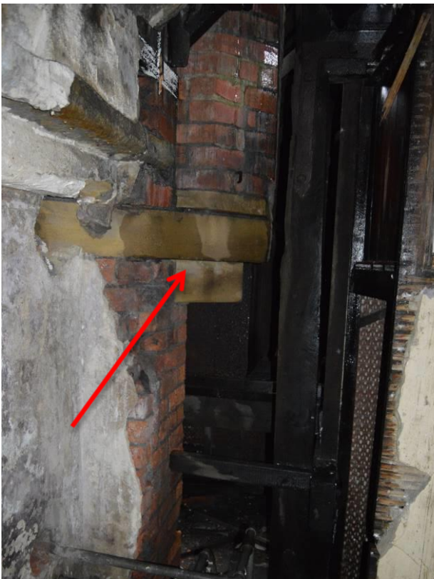
Plate 61.3: Stone corbel supporting the south west turret of the tower. Note the brick internal construction. Facing north east.
