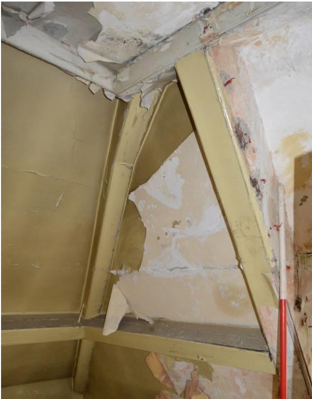
Plate 68.6: Trusses supporting the eastern hip incorporated into the interior space. Scale 2m. Facing south.
