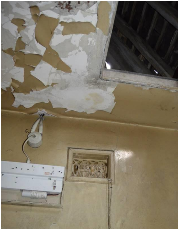
Plate 68.2: Vents above the doors to the rooms of the second floor accommodation. Facing south east.
