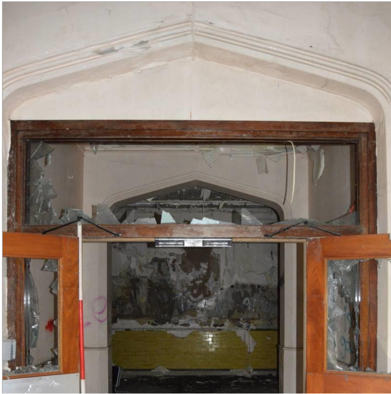
Plate 19: Internal arches in the visitor's hall. Note later insertion of glazed doors. Scale 2m. Facing south east.
