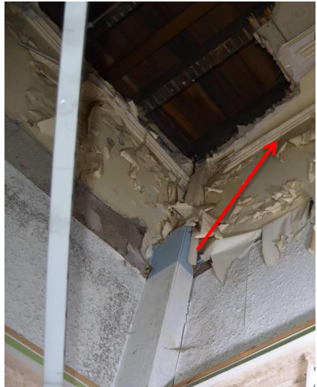
Plate 31: Surgeon's sitting room cornice in place above modern dumb waiter enclosure. Facing north east.
