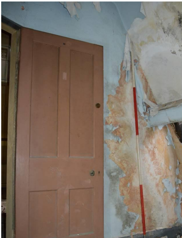
Plate 68.8: View within room S10, with four panel door. Scale 2m. Facing south west.
