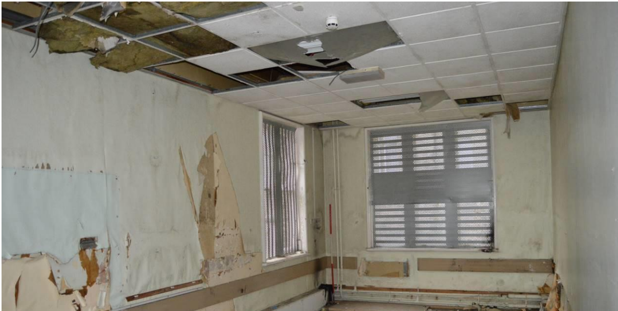
Plate 60.1: View facing west in the nurses' dormitory. Scale 2m. Facing south west.
