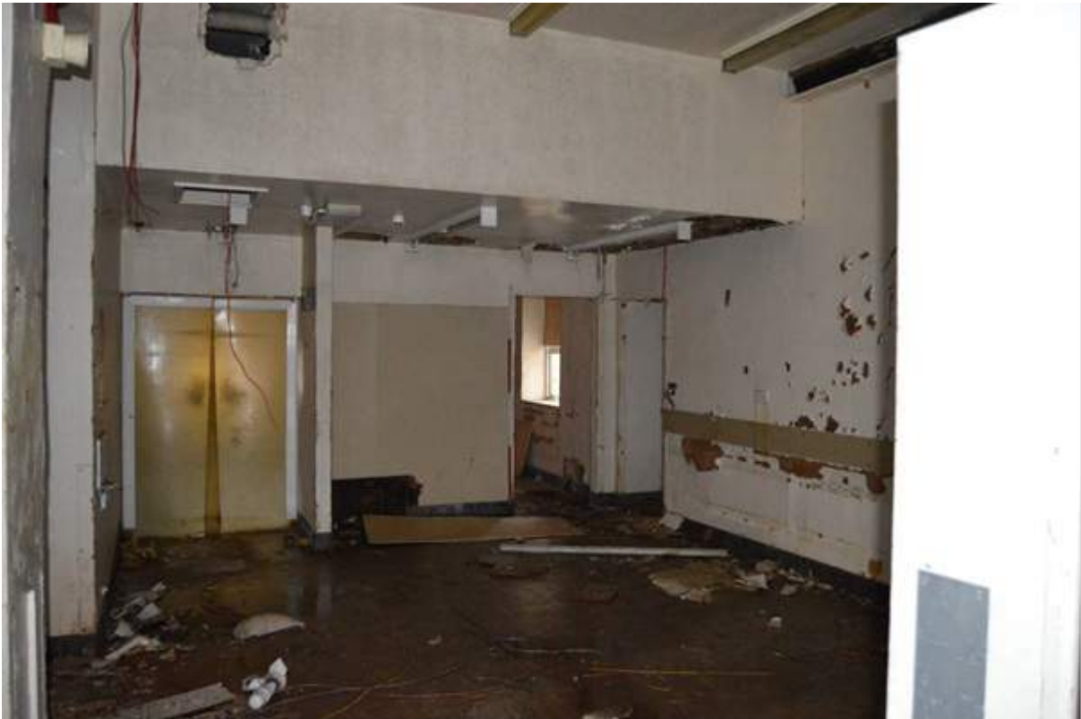
Plate 75: The modern kitchen area in the service range, the location of the staff dining room originally. The lowered ceiling is not a structural element, most probably housing modern services and equipment. Scale 2m.
