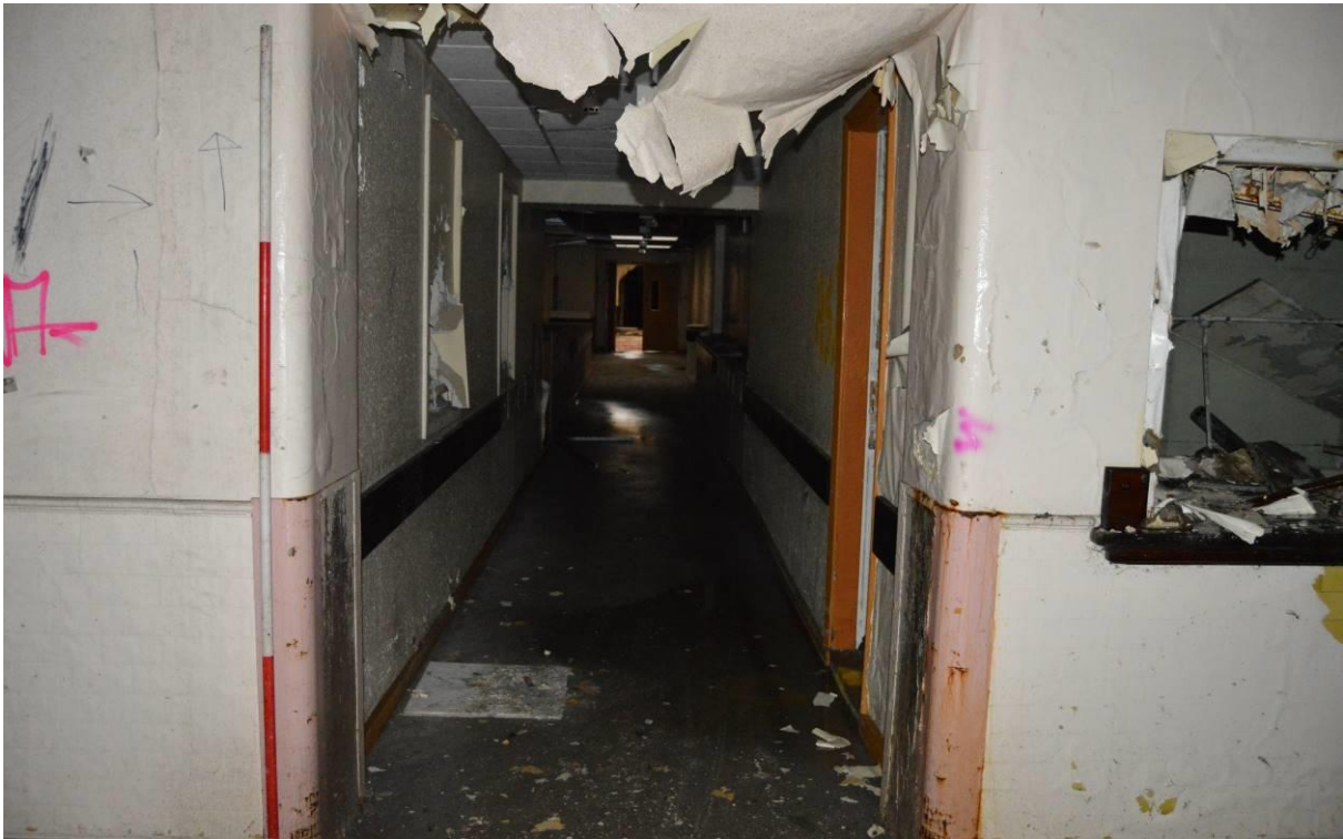
Plate 101.7: View of the later linking corridor from where it met the original axial corridor (facing north west). Scale 2m.
