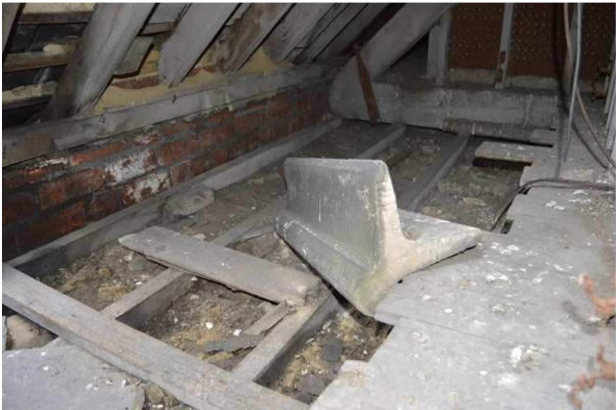
Plate 69.4: Ridge-stone fallen into roof space.
