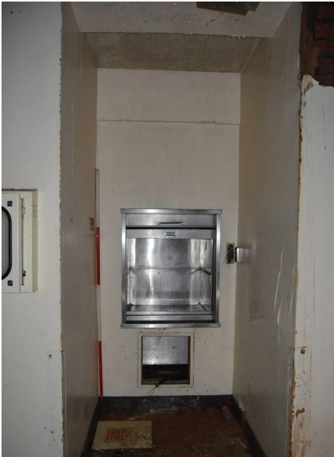
Plate 79.3: Detail of modern dumb waiter in room G11.1. Scale 2m. Facing south east.
