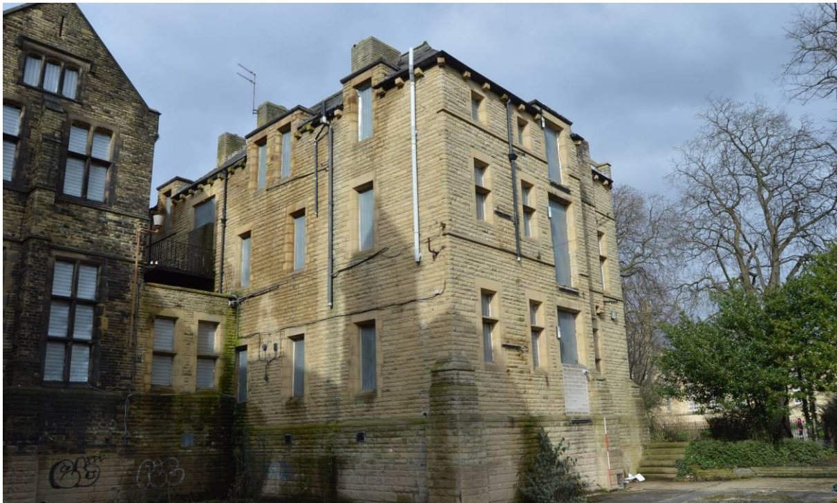
Plate 101: The rear and south facing elevations, along with its single story linking structure, of the Nurses' home (facing north). Scale 2m.
