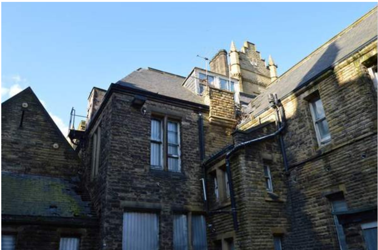
Plate 17: Rear view of the administration range looking north west. Note the truncated and capped chimney flues along the line of the eaves.
