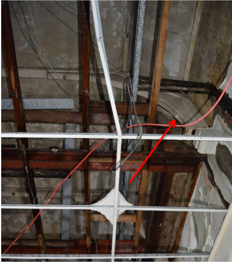
Plate 86.1: View of the board room ornate ceiling with hammer beam details (facing north west).
