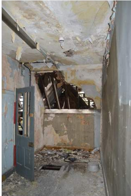
Plate 69.3: Room S13 looking north to the gable on the front projecting bay. Scale 2m.
