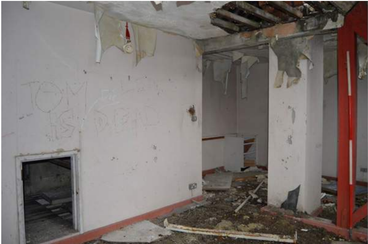
Plate 65.1: Room S3 with hatch to tower and chimney flue in the centre of the room. Scale 2m.
