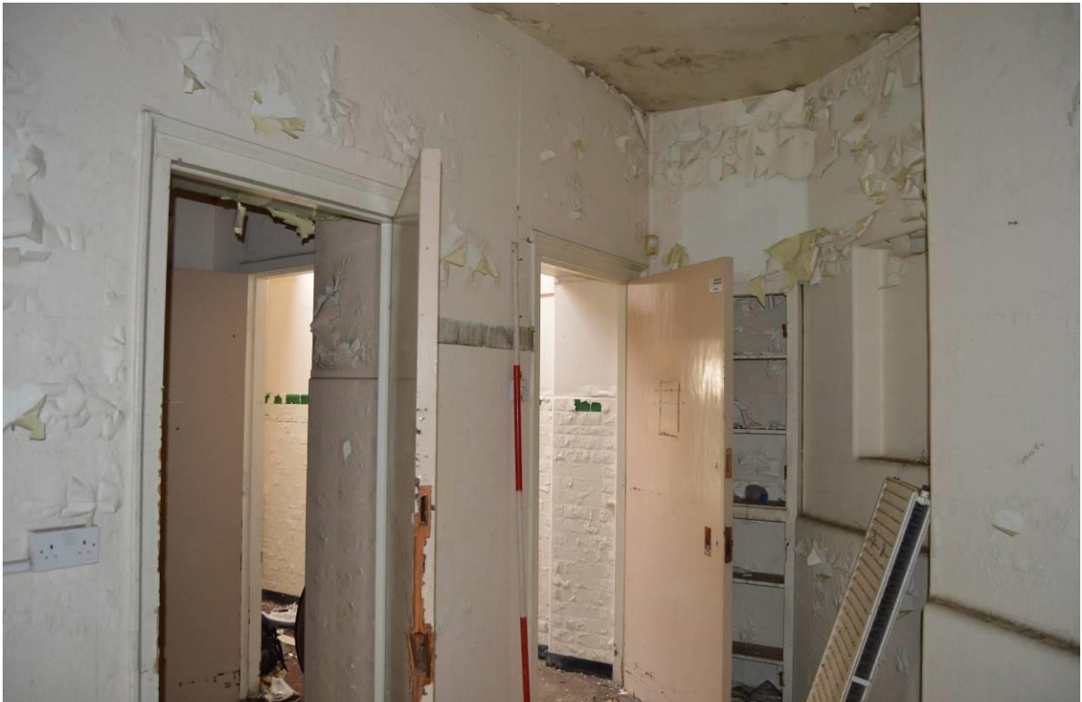
Plate 91.16: Room 26 formed by a later extension added to original east pavilion ward ground floor (facing north east). Scale 2m.
