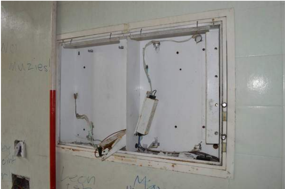
Plate 105.8: Operating theatre X-ray light fitting. Scale 2m.
