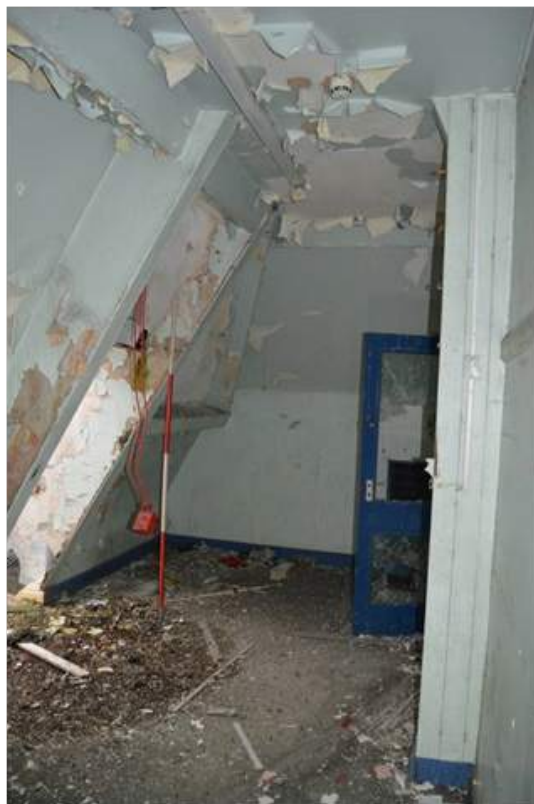
Plate 67.10: Room S8 below the west hip of the administration range. Scale 2m.
