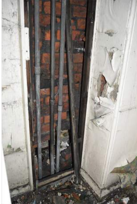
Plate 42.2: Old style pipes exposed in room F4, note the brick structure of the tower.
