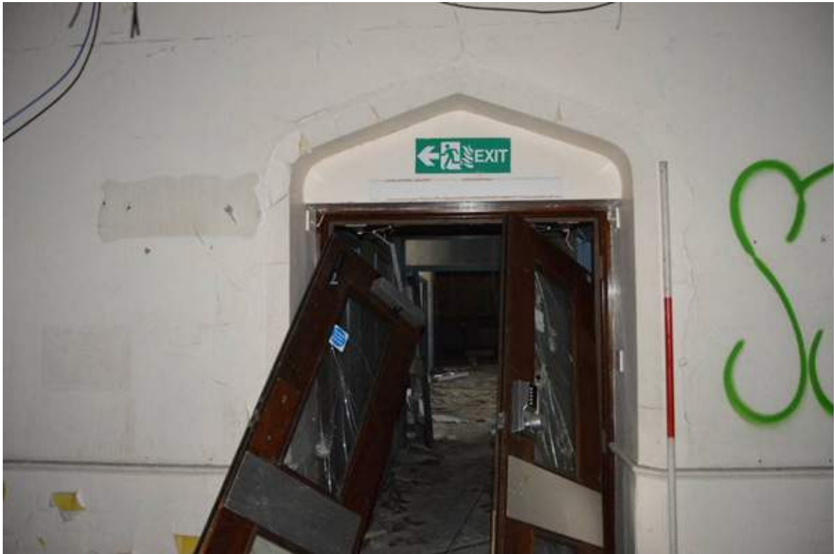
Plate 92.1: Tudor arch entrance retained to west pavilion ward, ground floor. Scale 2m.
