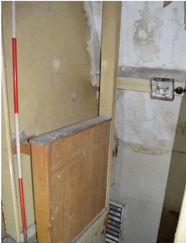
Plate 68: View towards staircase to section of second floor accommodation. Scale 2m. Facing south.
