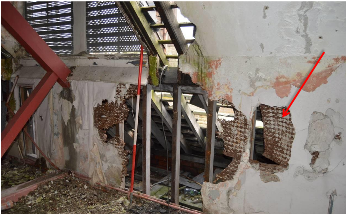
Plate 66.1: Room S3 with mesh and plaster wall construction. Scale 2m. Facing east.
