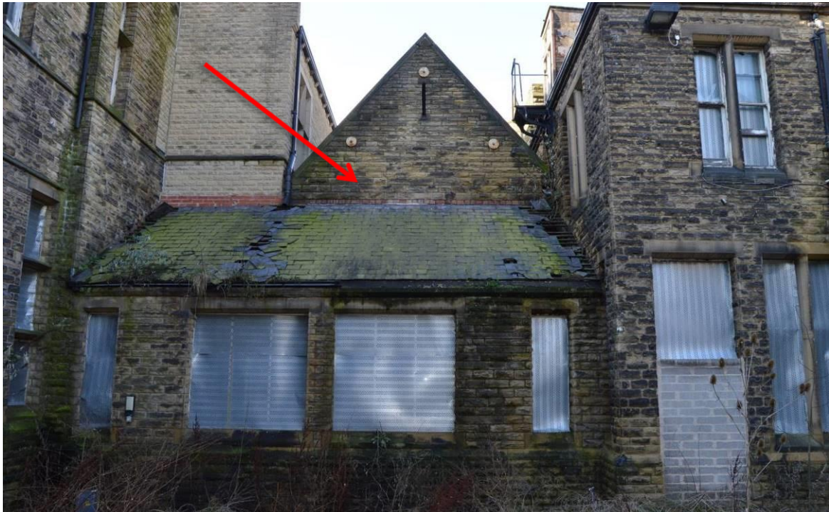
Plate 84: Rear view of the western linking range with the corridor in the foreground with the rear gable of the boardroom (facing north west).
