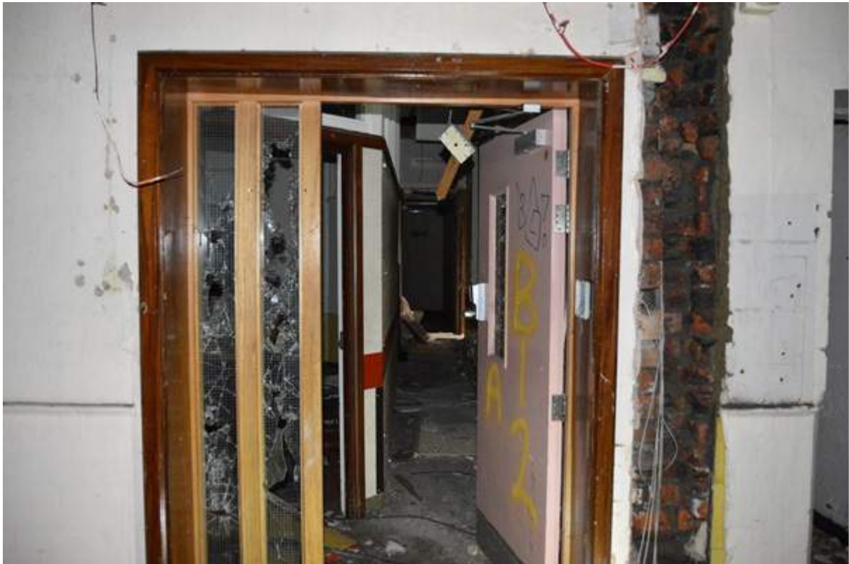
Plate 91.3: Modern entrance and corridors to ground floor of east pavilion ward, formerly out-patients dispensary and consulting rooms.
