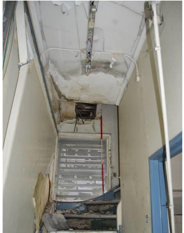
Plate 52.2: Stairs to the west of the nurses' accommodation. Scale 2m. Facing south west.
