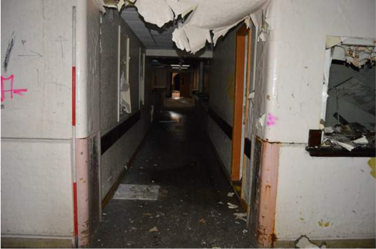
Plate 101.7: View of the later linking corridor from where it met the original axial corridor. Scale 2m.
