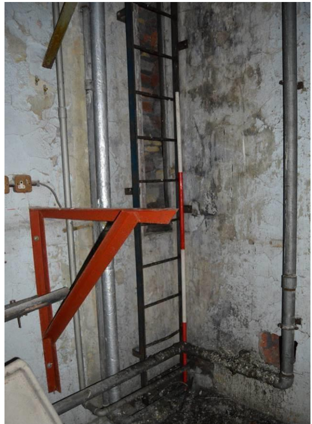
Plate 64.3: Ladder allowing access to the third floor of the tower. Scale 2m. Facing east.
