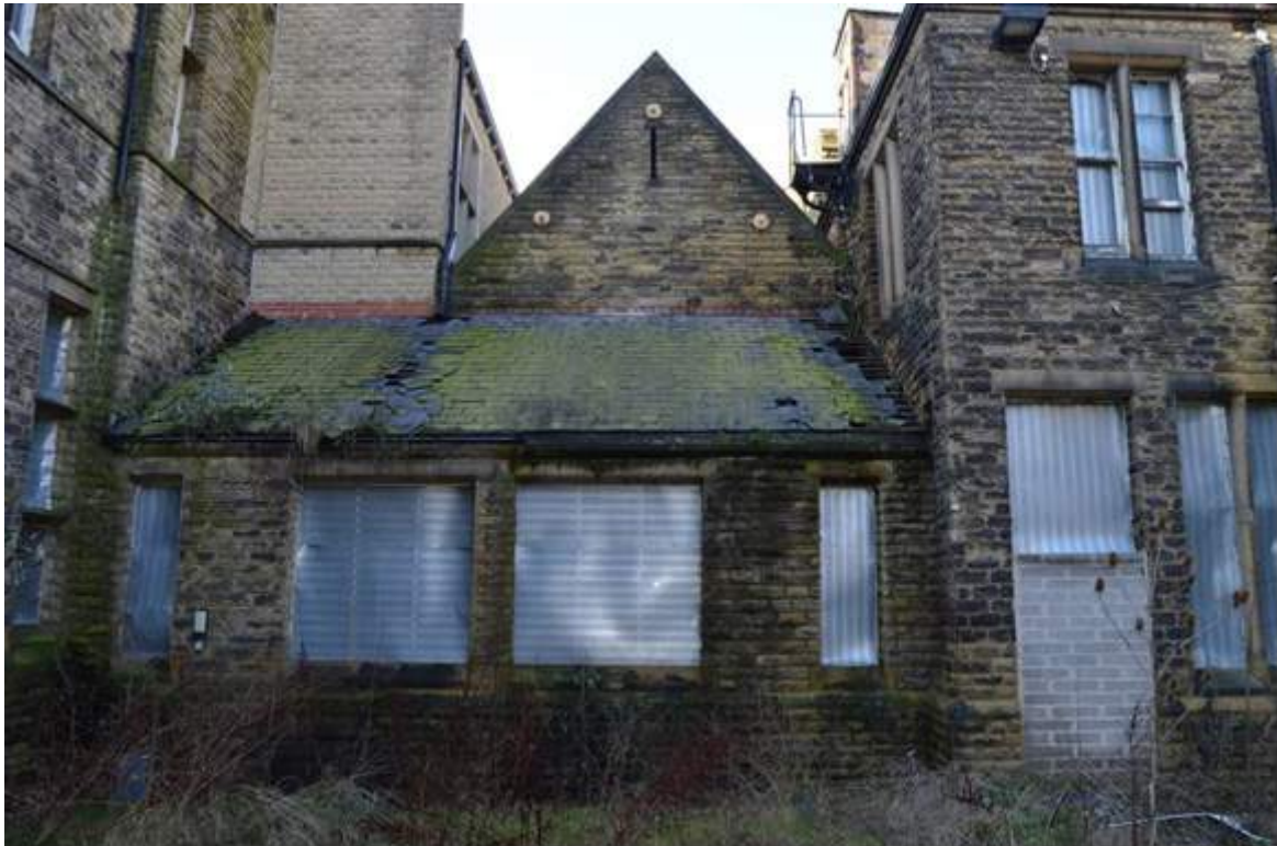
Plate 84: Rear view of the western linking range with the corridor in the foreground with the rear gable of the boardroom.
