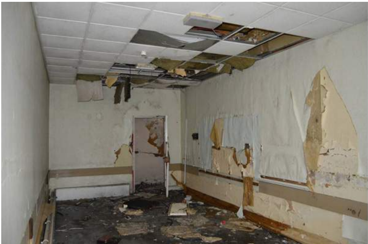
Plate 60.2: View facing east in the nurses' dormitory. Note the rough wall surface where the fireplace would have been located.
