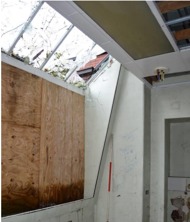
Plate 105.5: Detail of operating theatre window. Note the frame for secondary opaque glazing (facing north). Scale 2m.
