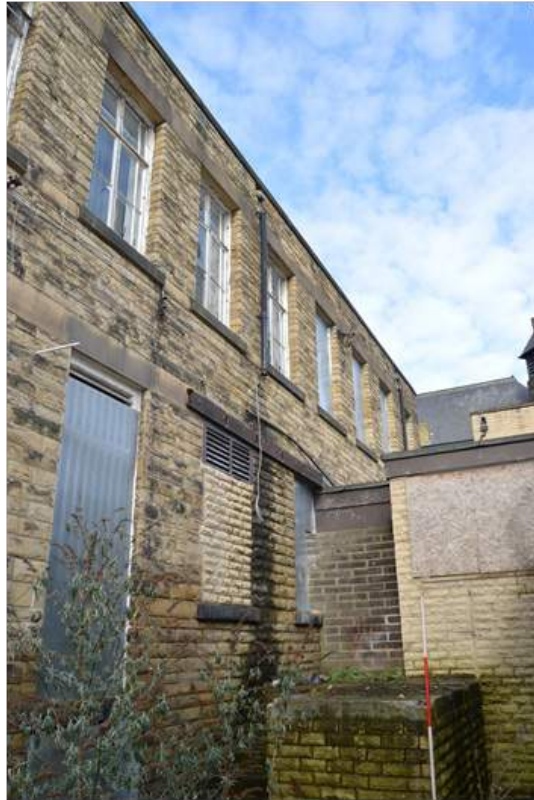
Plate 72.1: South elevation of the service wing extension, looking north west. Scale 2m.
