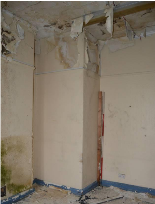
Plate 43.3: View of dumb waiter lift shaft from ground floor level. Scale 2m. Facing east.
