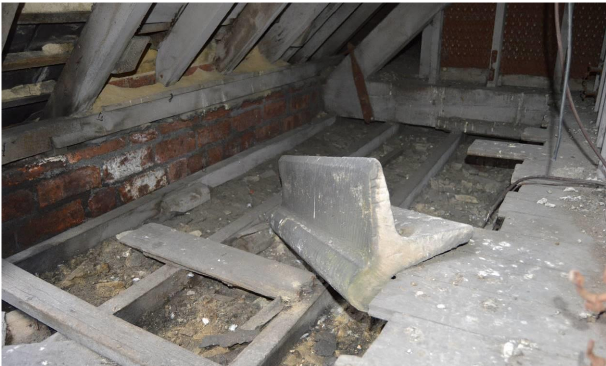
Plate 69.4: Ridge-stone fallen into roof space. Facing south.
