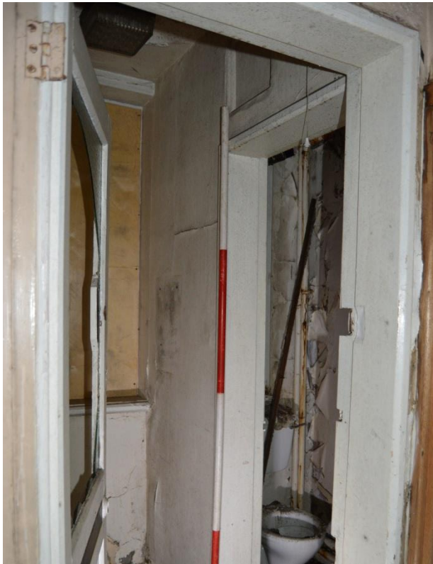
Plate 73.3: View into the W.C.. Note the vent above the door. Scale 2m. Facing south west.
