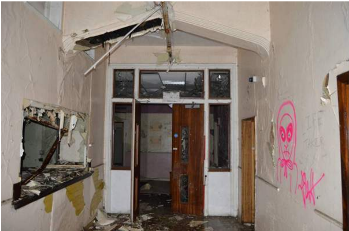
Plate 101.1: View from the axial corridor to the internal entrance to the Nurses' home.
