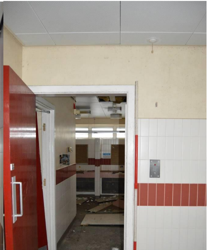
Plate 109.4: First floor interior of the modern extension to the Canning wards (facing north west). Scale 2m.
