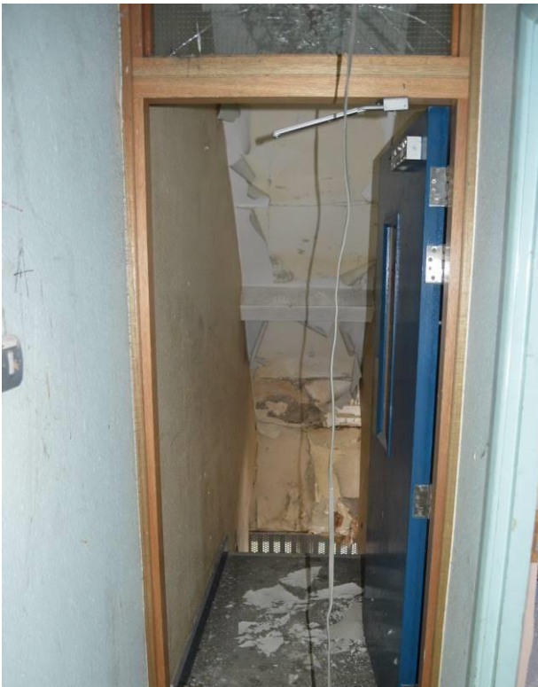
Plate 67.2: Modern fire door inserted into S4. Facing south east.
