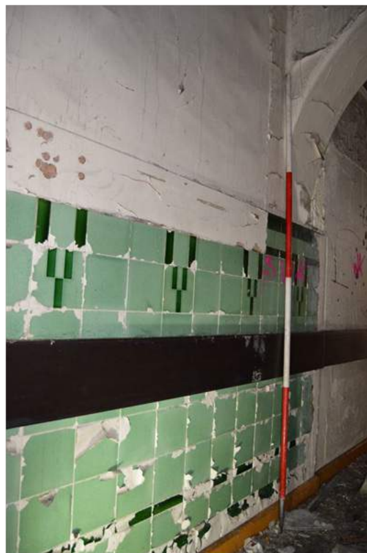
Plate 102.3: View of the out-patients linking corridor tiled finish below later paint finishes. Scale 2m.
