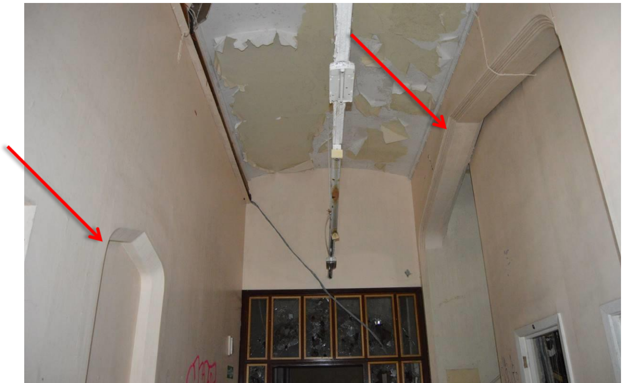
Plate 91.2: Tudor arch entrances to east pavilion ward and stairs, ground floor lobby (facing south west).
