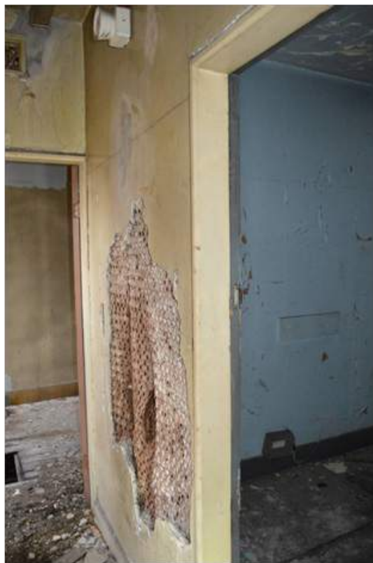
Plate 69: View of dividing wall to second floor rooms. Note the mesh layer.
