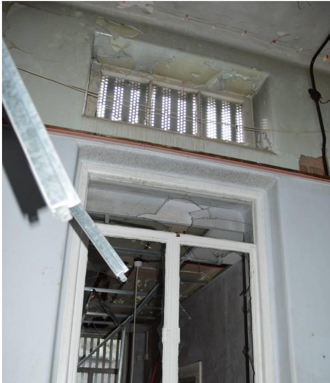
Plate 104.7: Detail of X-ray corridor window with internal and upper lights (facing south east).
