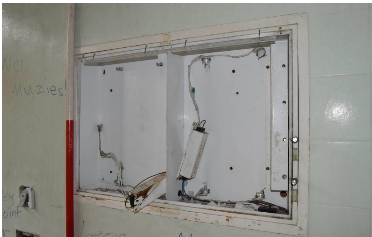
Plate 105.8: Operating theatre X-ray light fitting (facing north east). Scale 2m.
