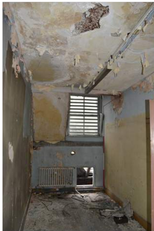
Plate 69.2: Dormer window to room S13, the window is adjacent to that in room S12. Scale 2m.
