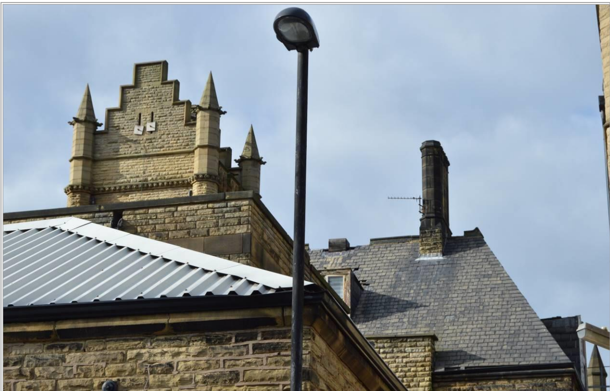
Plate 12: Rear gable of tower, note the less ornamented style and prominent parruss plates for internal tie rods. Facing west.
