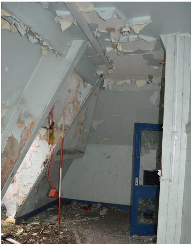
Plate 67.10: Room S8 below the west hip of the administration range. Scale 2m. Facing south east.
