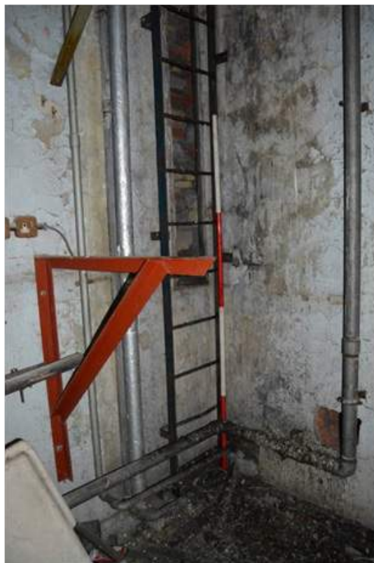
Plate 64.3: Ladder allowing access to the third floor of the tower. Scale 2m.
