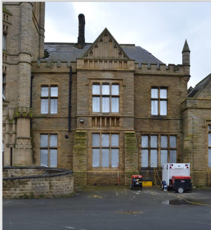
Plate 13: Front elevation view of administrative east range. Scale 2m. Facing south east.
