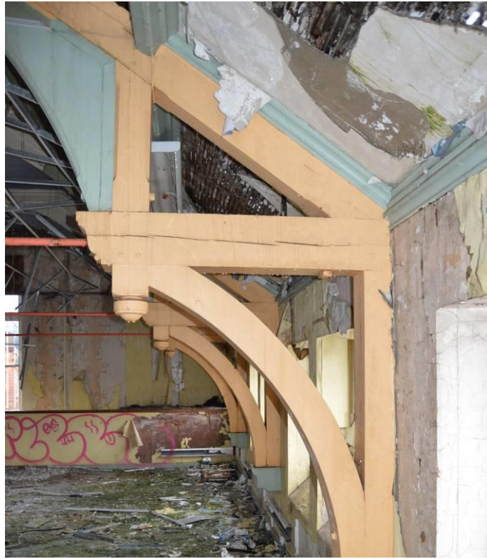
Plate 103: Upper level, retained ceiling features to out-patient's waiting room (facing north east).
