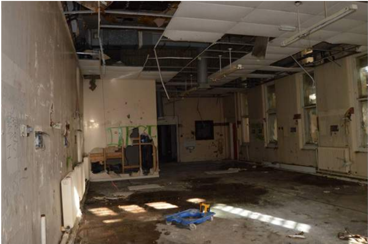
Plate 97.2: Plate 97.2: Reverse view of the ground floor of the children's ward. Scale 2m.
