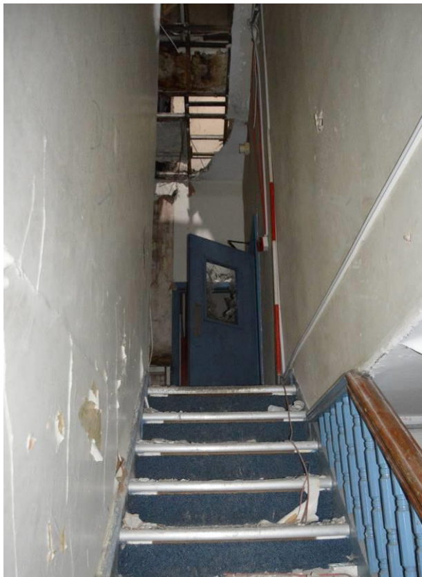
Plate 34: View up the stairs to room F1. Scale 2m. Facing north east.
