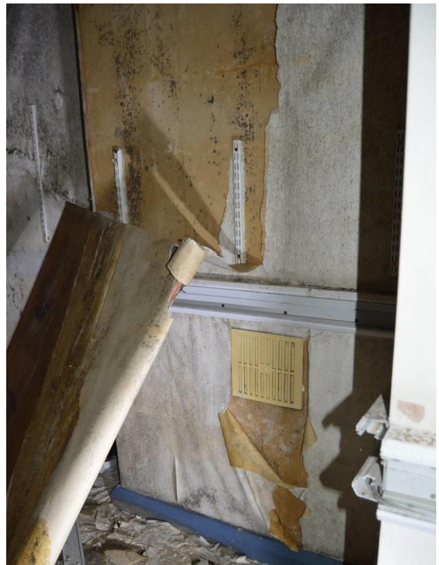
Plate 29.3: Blocked chimney with plastic vent. Facing north east.
