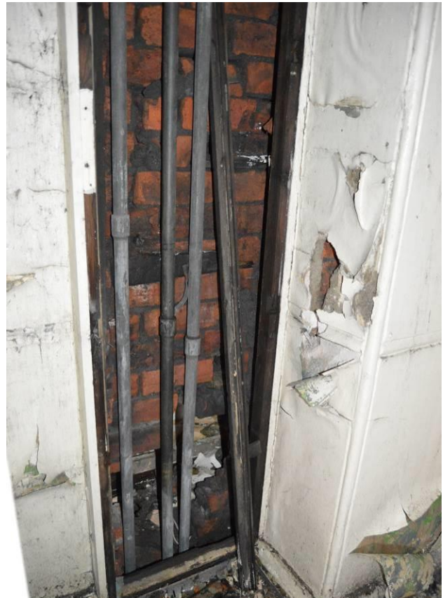
Plate 42.2: Old style pipes exposed in room F4, note the brick structure of the tower. Facing west.
