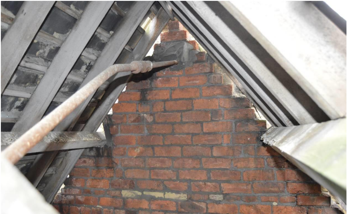
Plate 69.5: Brick construction behind the gable of the projection bay to front. Facing north west.
