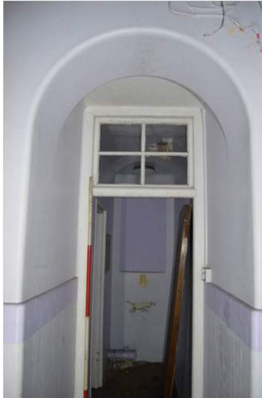
Plate 104.9: Sectional archway with rectangular fan light beyond, one of a series. Scale 2m.
