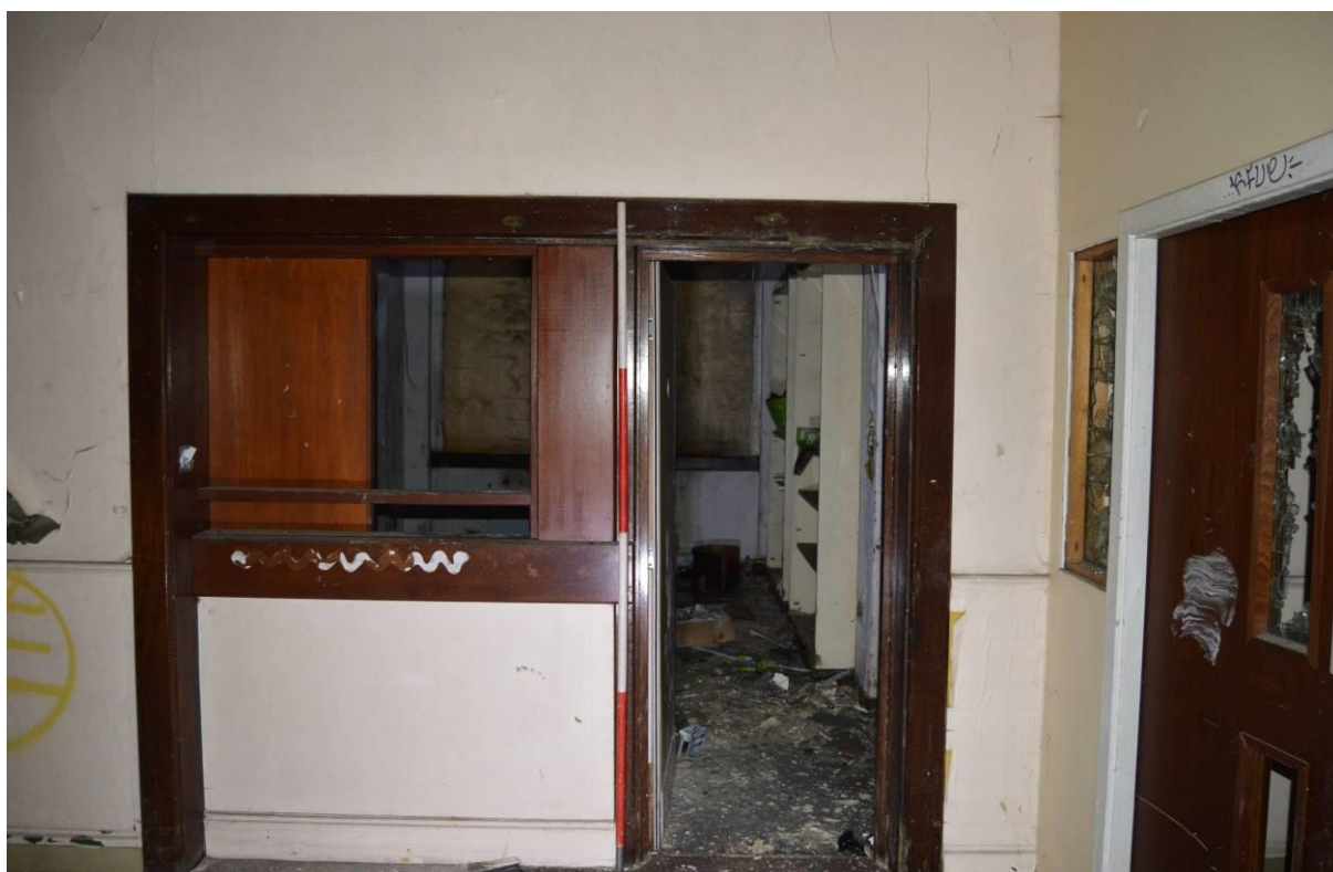
Plate 32: Counter/hatch and entrance from corridor into room G8. Scale 2m. Facing north west.
