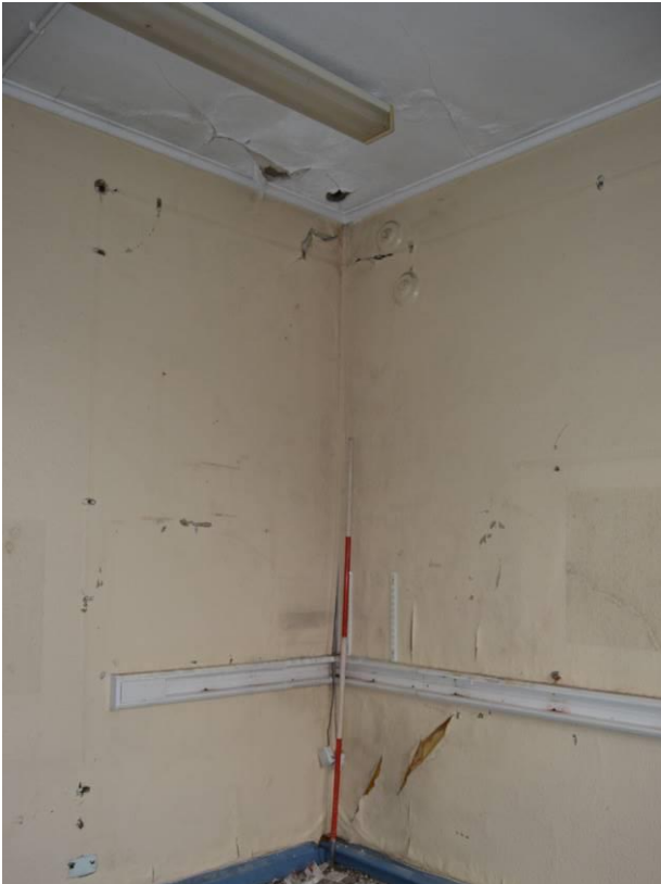
Plate 53.3: View of north east corner of F 11. Scale 2m. Facing north east.
