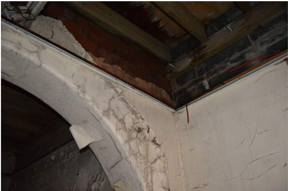
Plate 101.10: View of the later linking corridor from where it structurally joins the older building.
