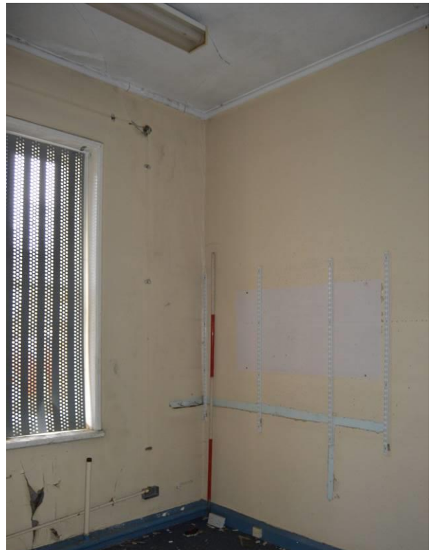
Plate 53.2: Nurses' bedroom. Note lack of corner chimney piece. Scale 2m. Facing south.
