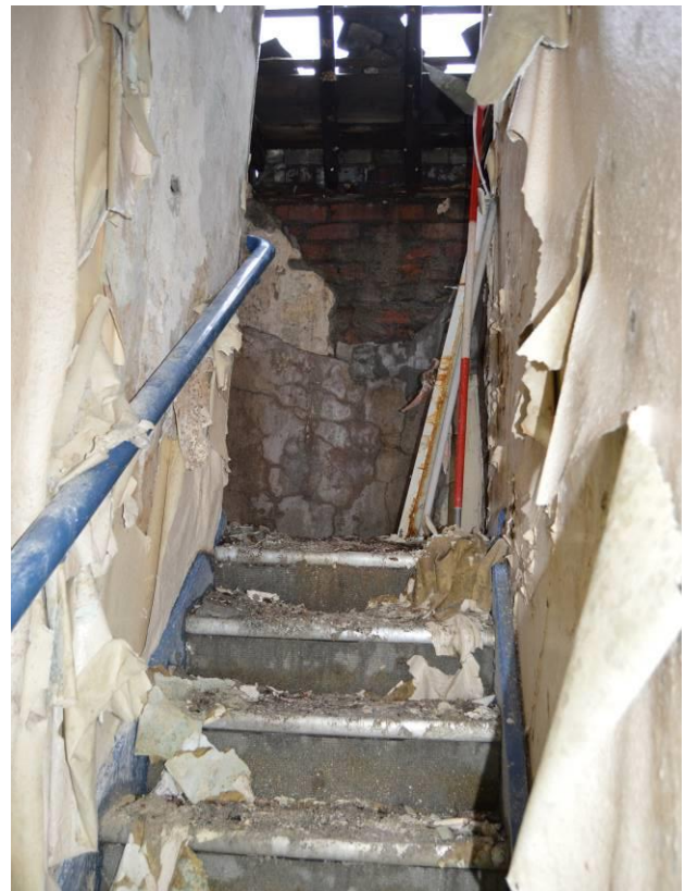
Plate 56.2: Half-landing/dog-leg of the stairs to the second floor. Scale 2m. Facing south east.
