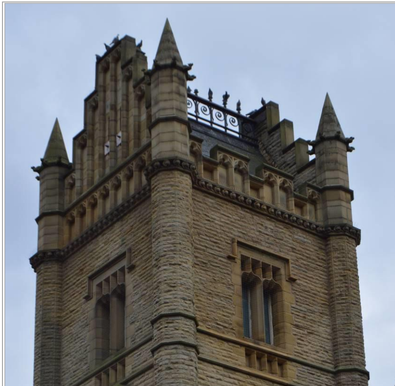
Plate 11: View of the top sections of the tower and its turrets. Facing east.
