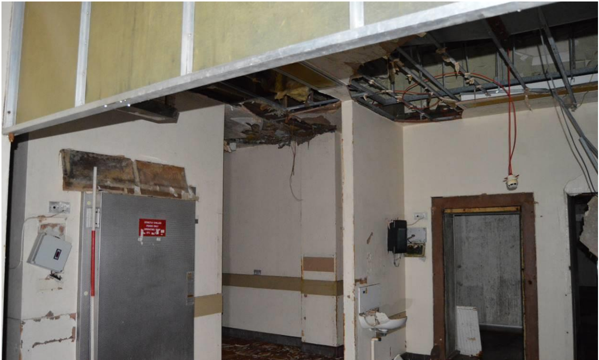
Plate 78: View towards the south back wall of the kitchen. Scale 2m. Facing south east.
