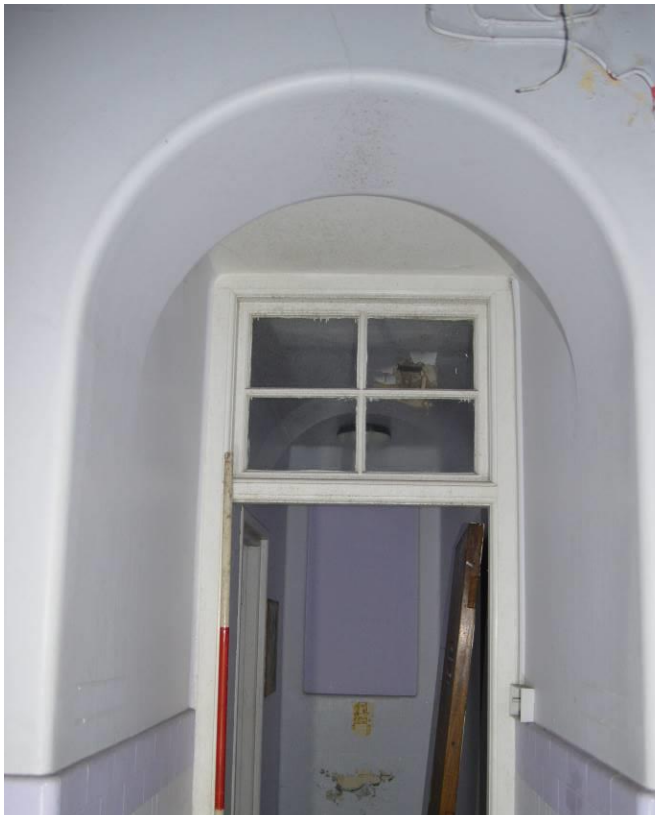
Plate 104.9: Sectional archway with rectangular fan light beyond, one of a series (facing south east). Scale 2m.
