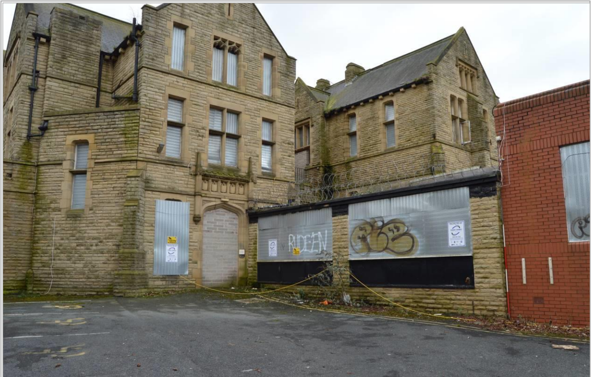
Plate 100: The Nurses' home extension to the east of the original hospital building (facing south). Scale 2m.
