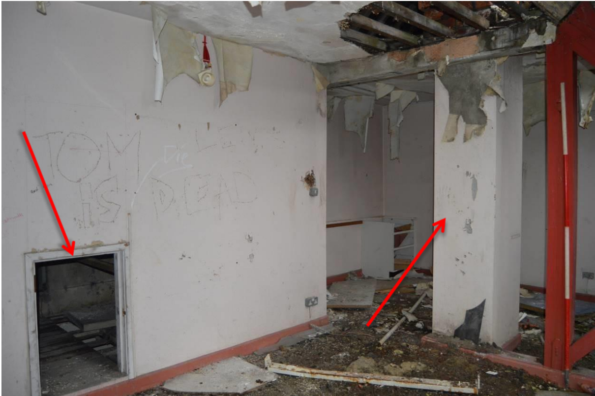
Plate 65.1: Room S3 with hatch to tower and chimney flue in the centre of the room. Scale 2m. Facing north.
