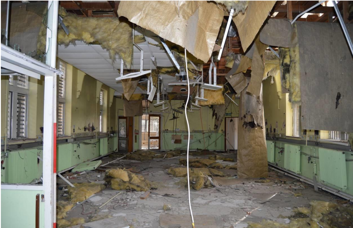
Plate 91.22: First floor ward of the eastern pavilion wing, facing south east. Scale 2m.
