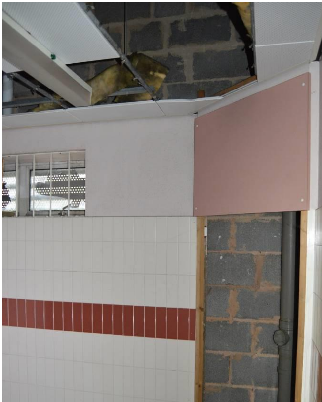
Plate 109.3: Detail of construction of the modern extension to the Canning wards (facing north west).
