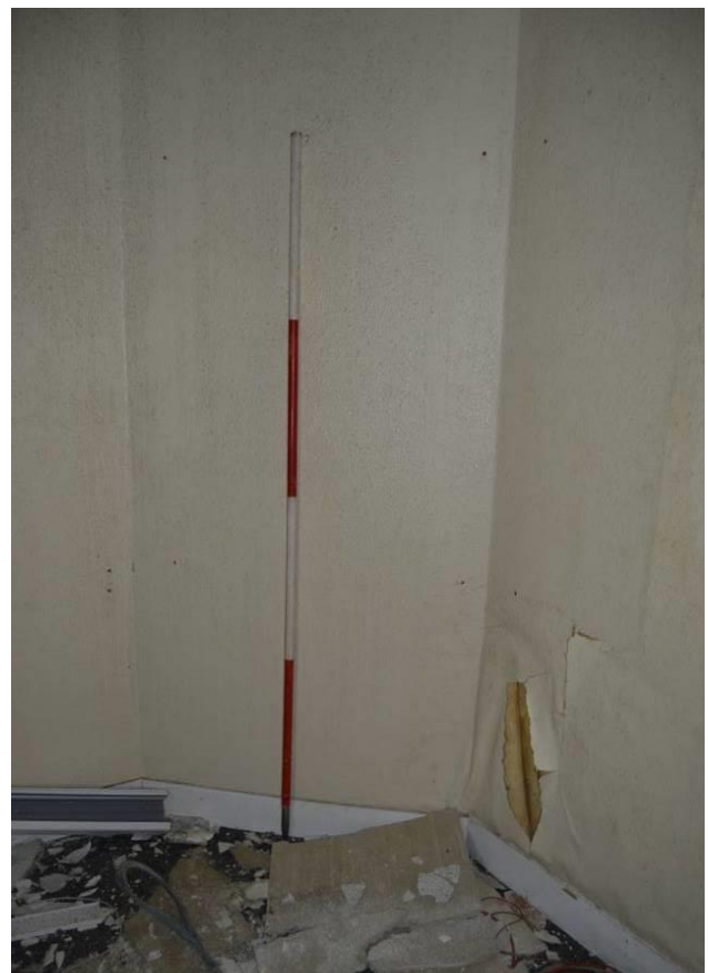
Plate 20.1: Corner chimney breast in visitor waiting room G2. Scale 2m. Facing south.
