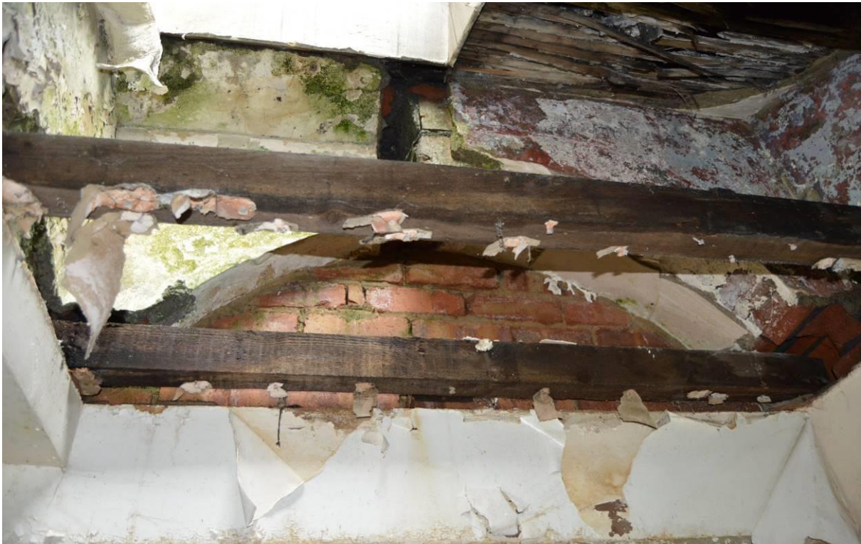
Plate 82: Arch above the half-landing of the nurses' stair half-landing, facing south west.
