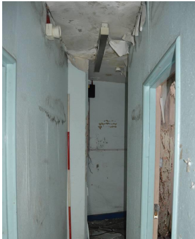
Plate 67.3: Facing east down the irregularly shaped corridor. Scale 2m. Facing north east.
