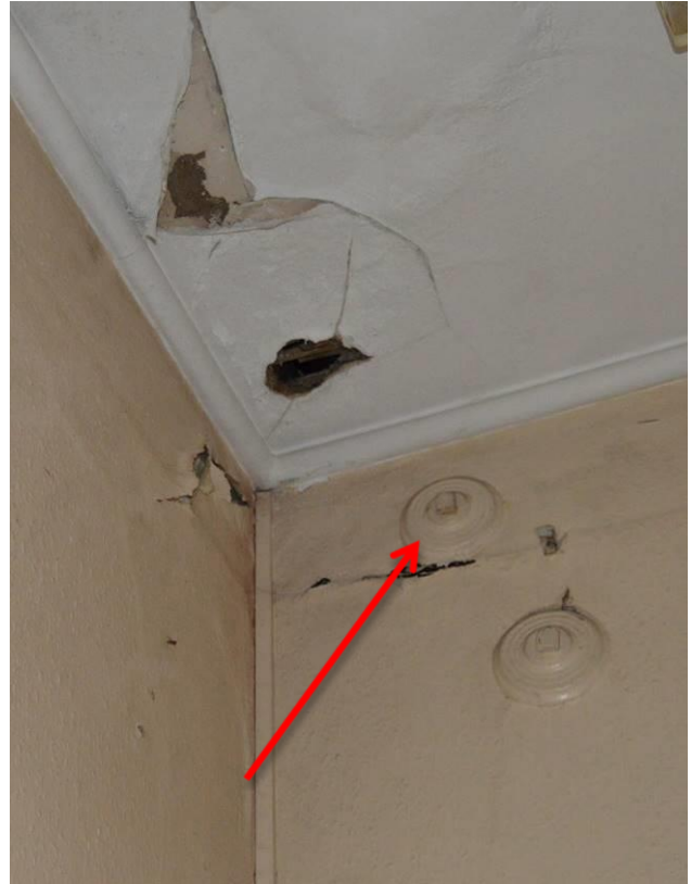
Plate 53.4: View of tie rod pattress plate fittings to room F11. Facing north.
