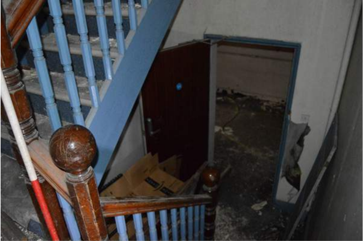
Plate 21: View from the half-landing in room G3 of the administration range. Scale 2m.
