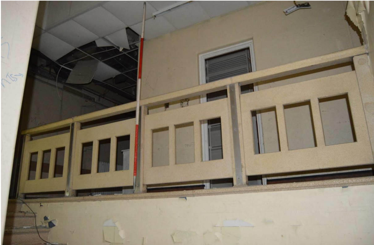
Plate 105.14: The Ann Canning Childs' Ward for Women stairs landing balustrade (facing south west). Scale 2m.
