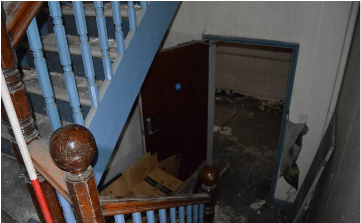
Plate 21: View from the half-landing in room G3 of the administration range. Scale 2m. Facing north.
