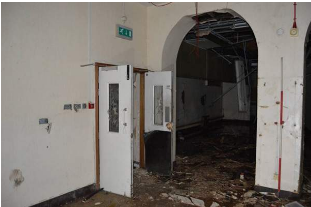
Plate 76: View back towards the entrance to the modern kitchen area. Note the opened up relieving arches which formed the east wall of the original staff dining room. Scale 2m.
