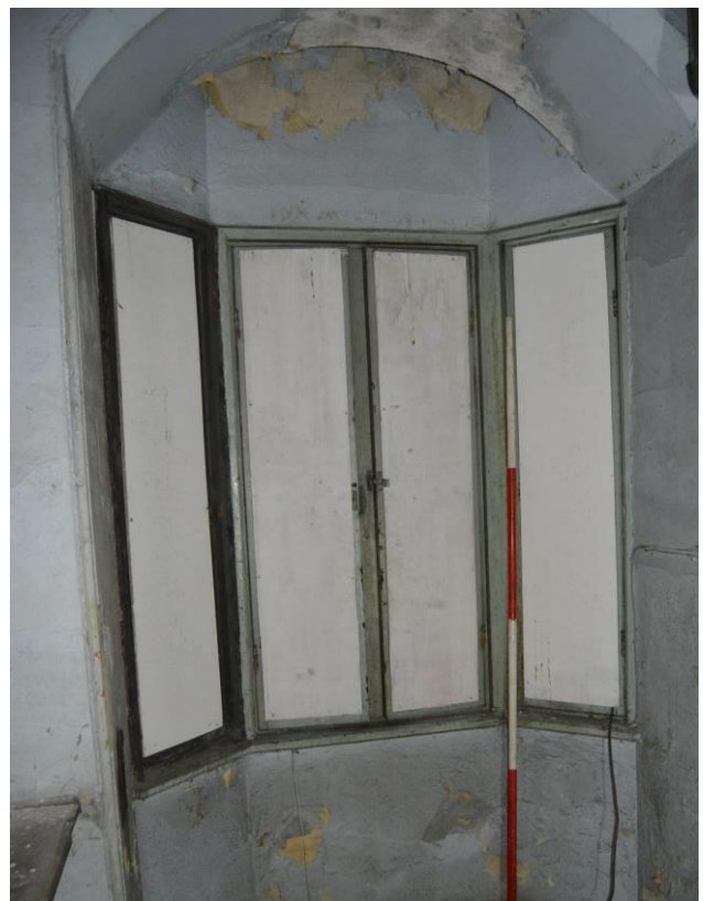
Plate 64.1: Top bay of the oriel window the tower with original shutters. Scale 2m. Facing north west.
