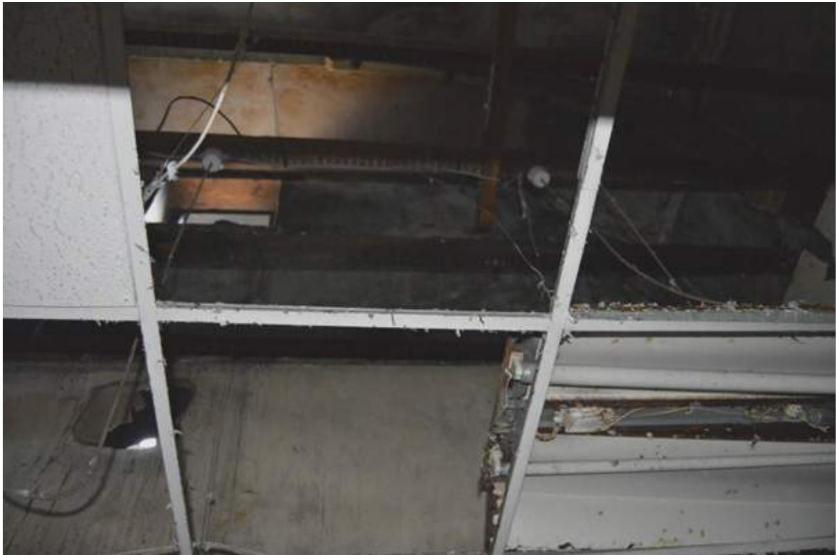
Plate 89.4: Section of operating theatre with two later ceilings below, including a lathe and plaster example. A hammer beam is just visible above.
