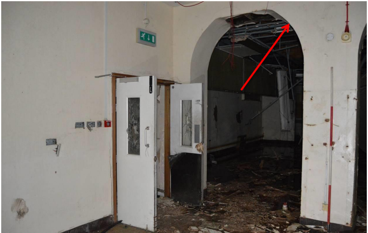
Plate 76: View back towards the entrance to the modern kitchen area. Note the opened up relieving arches which formed the east wall of the original staff dining room. Scale 2m. Facing north.
