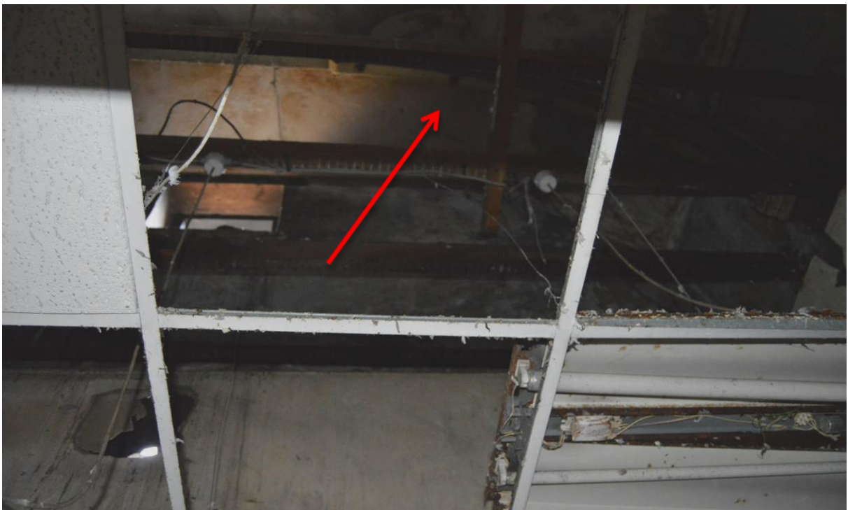
Plate 89.4: Section of operating theatre with two later ceilings below, including a lathe and plaster example. A hammer beam is just visible above (facing south east).
