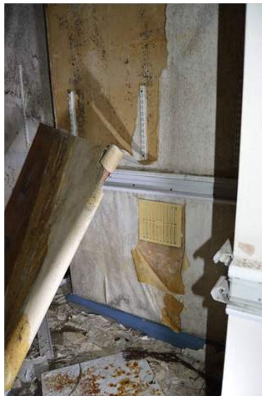
Plate 29.3: Blocked chimney with plastic vent.
