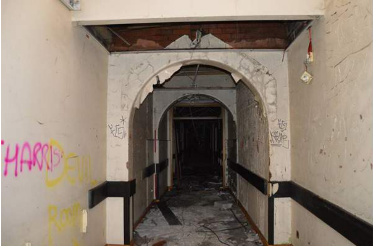
Plate 101.9: View of the later linking corridor from where it met the original out-patients' department. Scale 2m.
