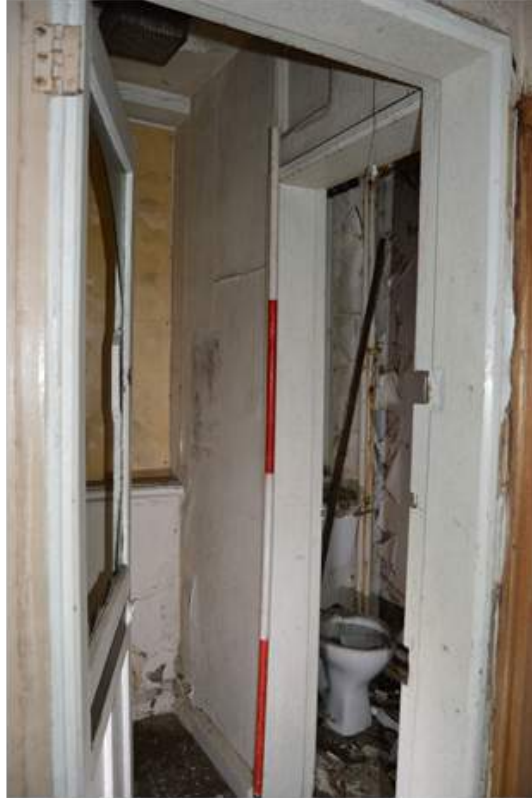
Plate 73.3: View into the W.C.. Note the vent above the door. Scale 2m.
