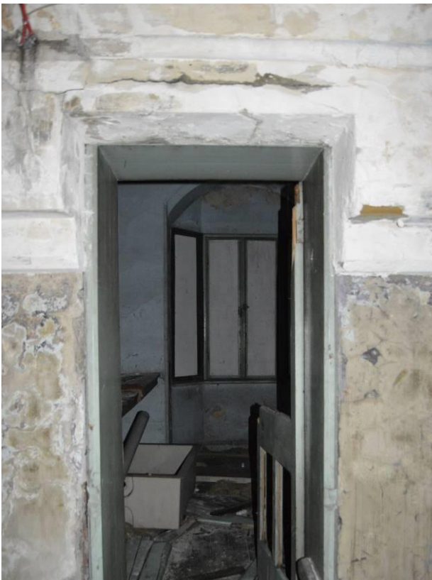
Plate 63: View into second floor tower room. Note the corbelled plasterwork at the door head. Facing north west.
