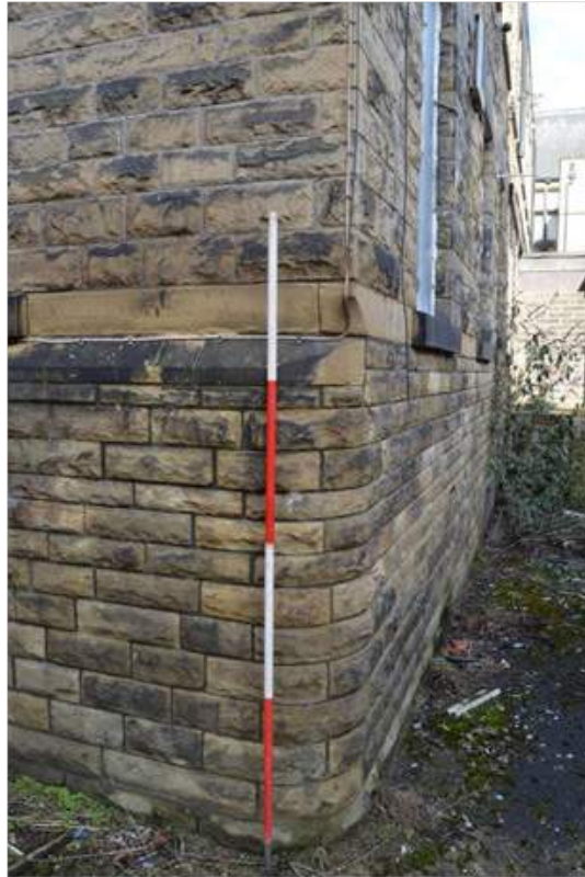
Plate 72.3: Filleted corner to south east corner of service wing extension. Scale 2m.
