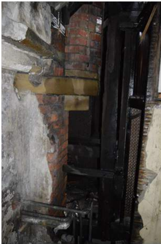
Plate 61.3: Stone corbel supporting the south west turret of the tower. Note the brick internal construction.
