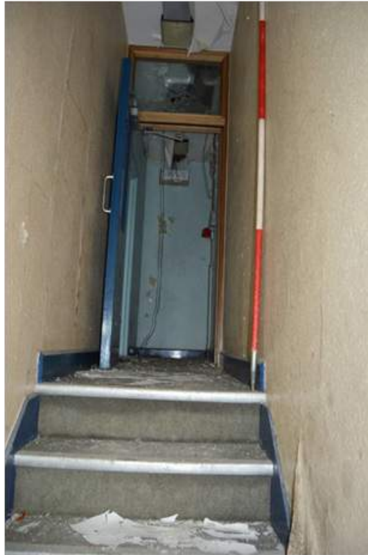
Plate 67.1: The corridor giving access to S3 and other rooms in the west section of the second floor accommodation. Scale 2m.
