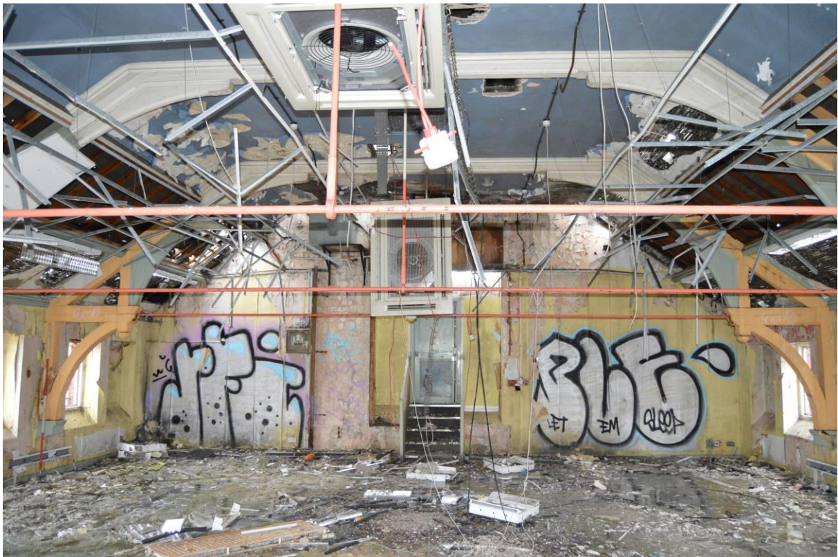
Plate 103.1: Upper level, retained the ceiling to out-patient's waiting room (facing south west). Scale 2m.
