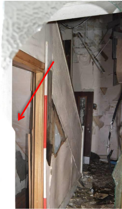
Plate 73.5: View of the staircase with door to basement stairs. Scale 2m. Facing north east.
