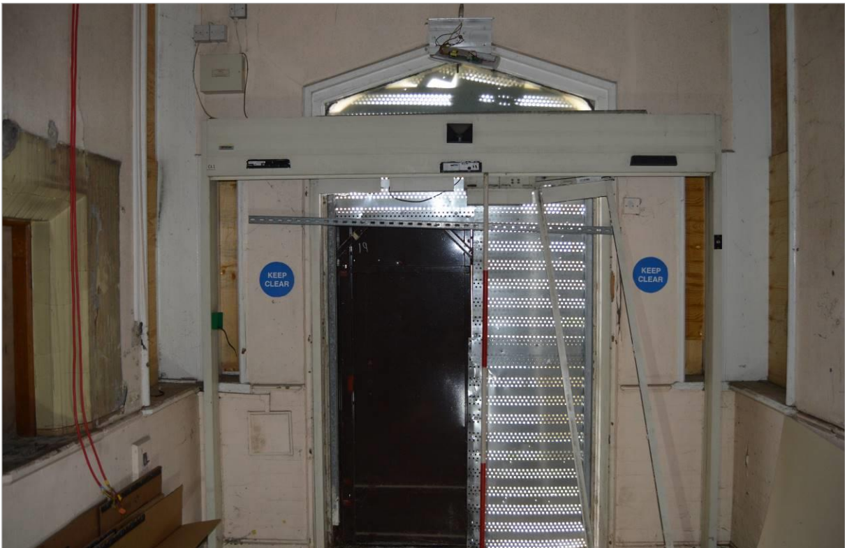
Plate 18: Internal view of the main entrance in the administration range. Scale 2m. facing north west.
