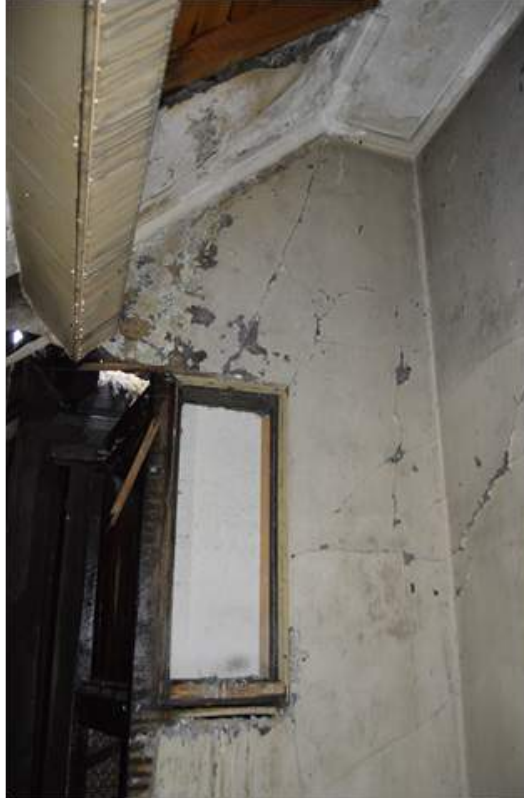
Plate 61.4: View of the lightwell plasterwork. Note the squint type opening in the far wall.
