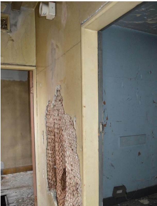
Plate 69: View of dividing wall to second floor rooms. Note the mesh layer. Facing east.
