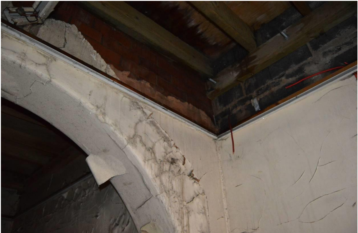
Plate 101.10: View of the later linking corridor from where it structurally joins the older building (facing north).
