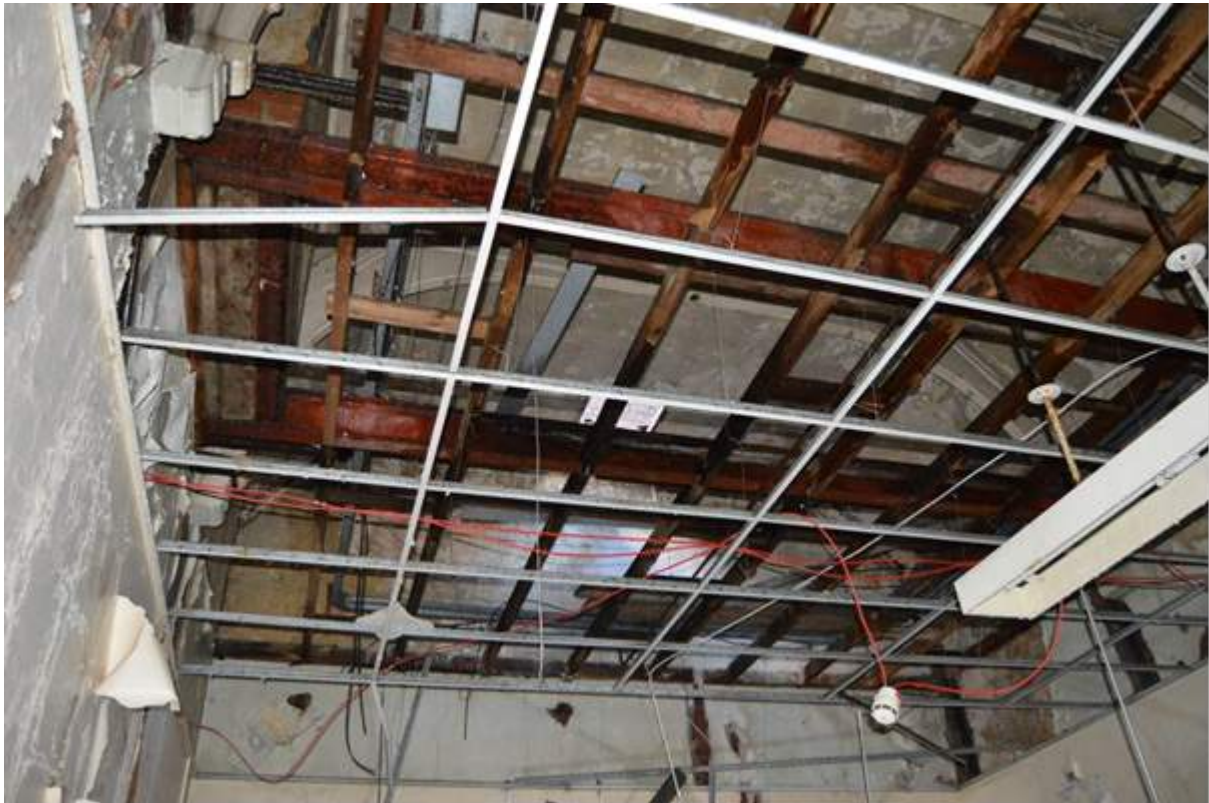
Plate 86.4: Rear of the board room ceiling. Note the hammer beam truss above the later ceiling framework.
