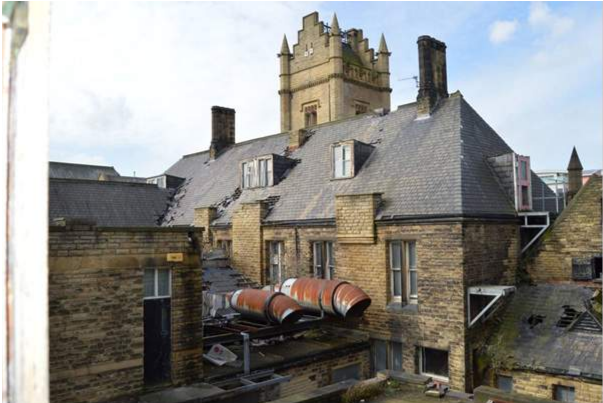
Plate 16: Rear view of the administration range looking north west. Note the truncated and capped chimney flues along the line of the eaves.
