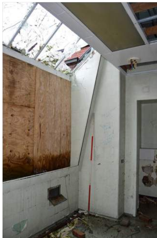
Plate 105.5: Detail of operating theatre window. Note the frame for secondary opaque glazing. Scale 2m.
