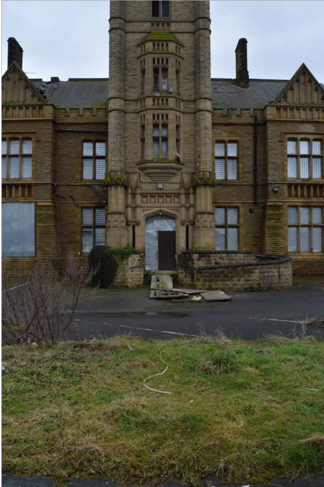
Plate 3: The front elevation of the tower with main entrance below of the administration range. Scale 2m.
