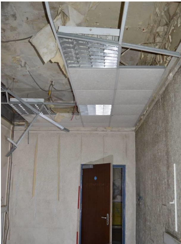
Plate 29.2: Modern door and suspended ceiling but with features above. Scale 2m. Facing south east.
