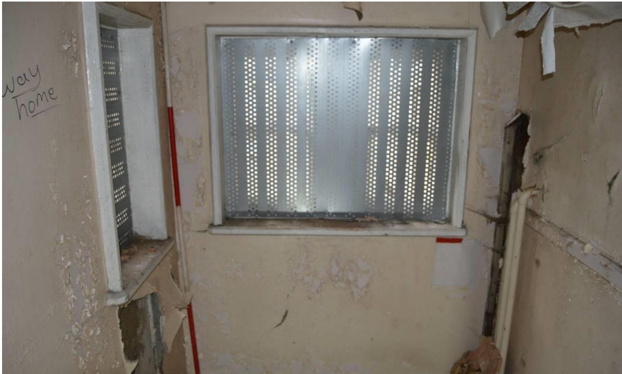
Plate 74.2: Windows to the half-landing of the service stair well. Scale 2m. Facing south west.
