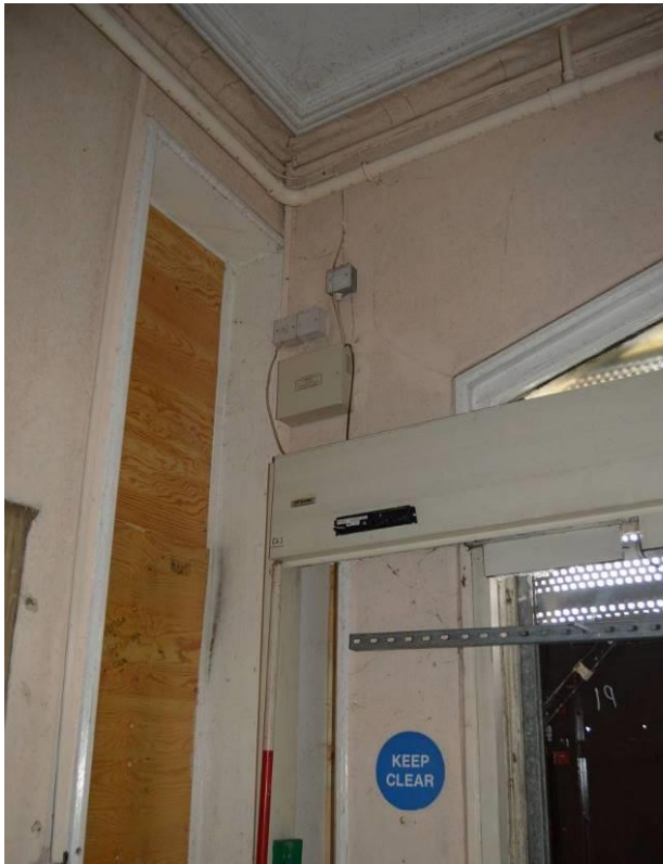
Plate 19.3: Detail of windows and coving to north corners of visitor hall. Scale 2m. Facing west.
