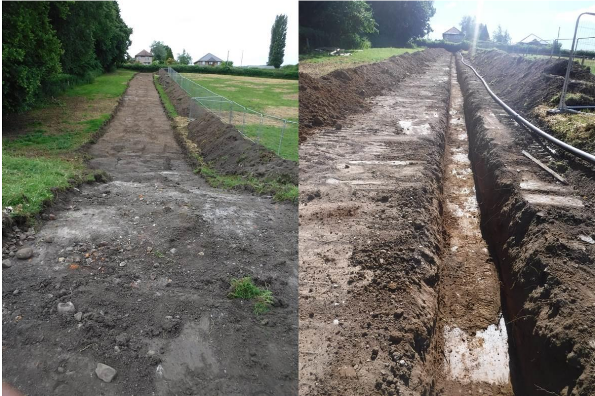
Figure 3. Left: Topsoil strip, looking southwest with exposed colliery spoil heap (004) in foreground; Right: Pipe trench, within stripped area, looking southwest
