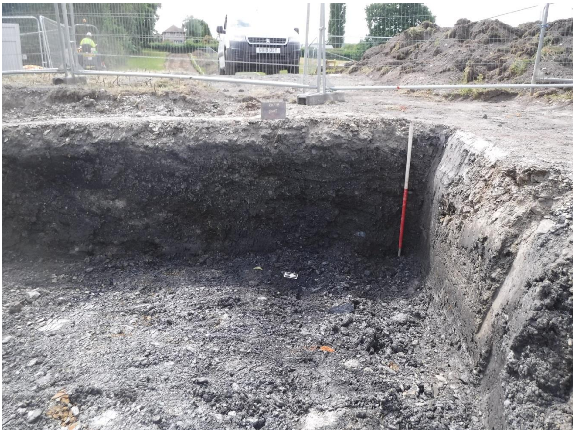
Figure 4. Excavation for footprint of pumping station, east and south facing sections through colliery spoil heap (004)
