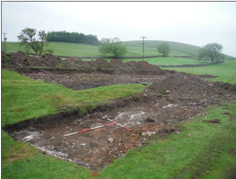
Figure 8: Location shot of Plot 2 (Septic Tank) and Plot 3 in the back (scale = 2m x 2m).
