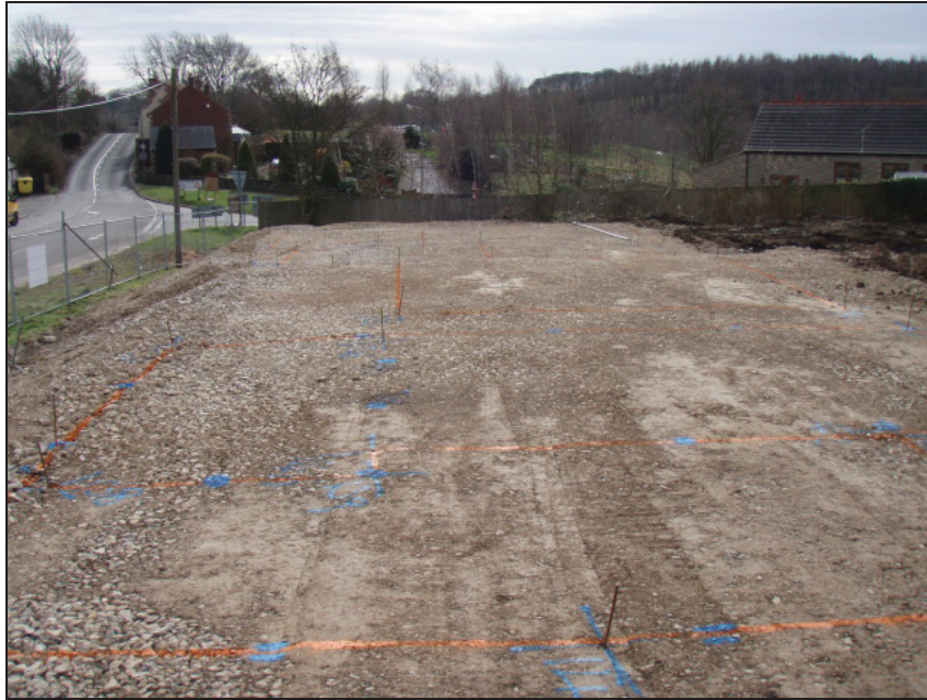
Fig. 7: Area B shown after the bank has been removed and a levelling layer of aggregate deposited ready for construction to begin.
