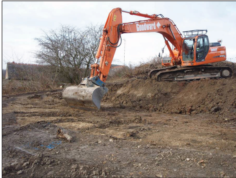
Fig. 4: Working shot of the removal of the soil to form a terrace for Area B.
