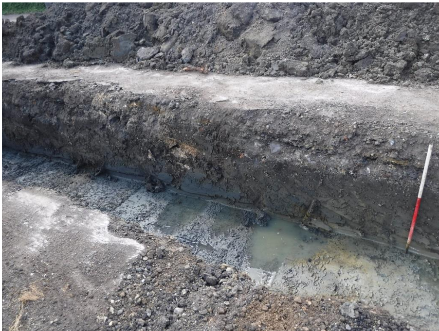
Figure 5. East facing section through Trench 1 showing modern surfaces over contaminated clay. Gravel backfill of modern pipe trench visible as an orange patch within the clay. Natural gravelly clay and ground-water in base of trench. Scales: 0.5m graduations.
