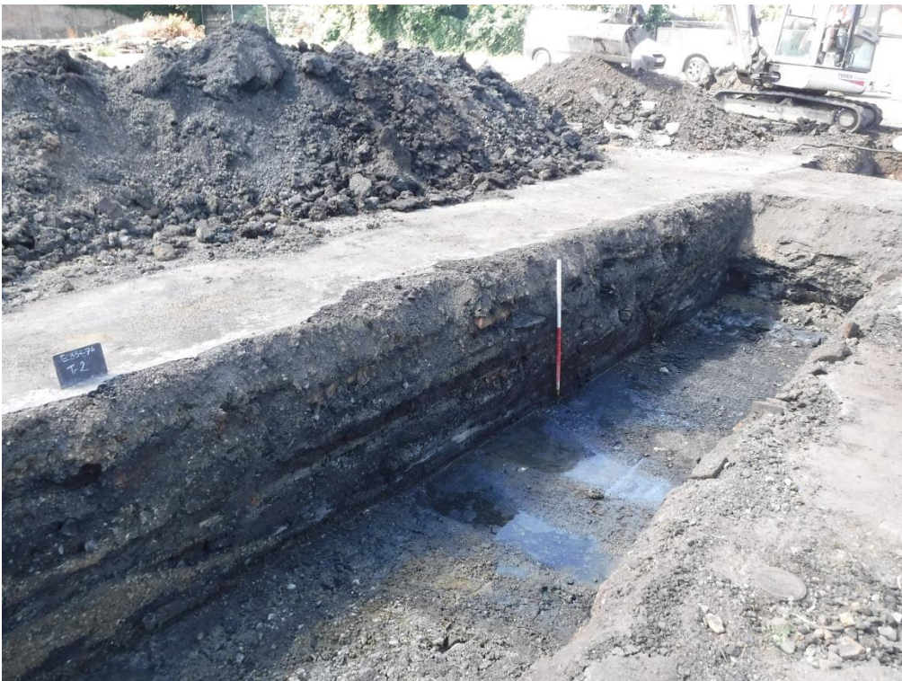
Figure 9. Contaminated deposits deeper than 1.2m meant that black sandy layer (210) formed base of trench after 9.8m of excavation. Possible cut [216] visible through gravel (211) in bottom left of photo. Scale: 0.5m graduations.
