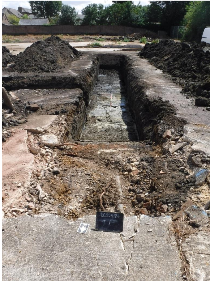
Figure 4. Trench 1 looking south, note the dog-legged service pipe beneath concrete in the foreground. Scale: 0.5m graduations.
