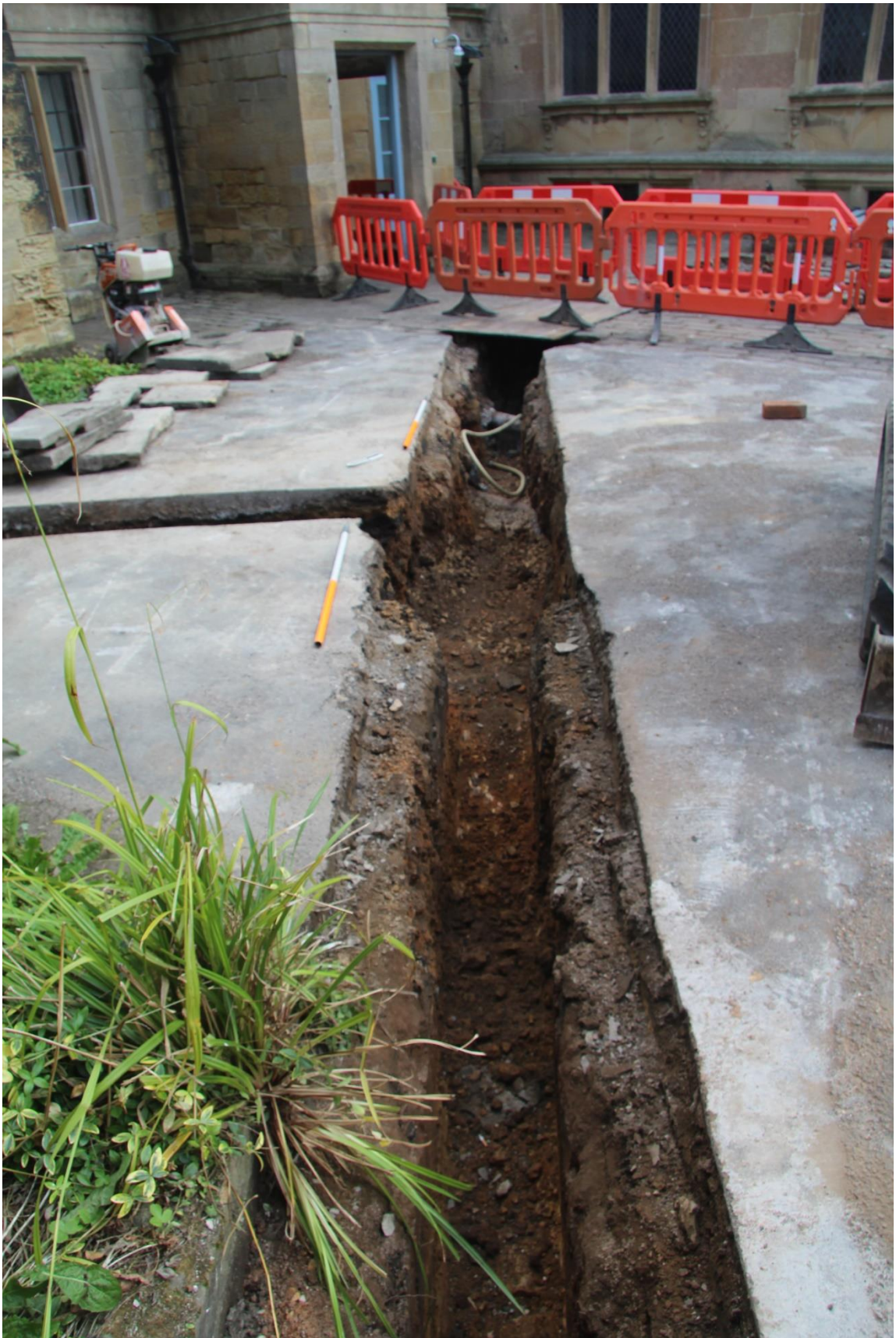
Figure 15. Excavations outside the National Trust offices (Scale 2x 1m in 0,5m gradations)
