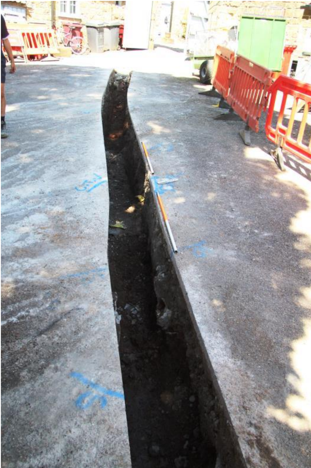
Figure 3. Trench excavation behind the Great Barn (the current National Trust restaurant) (Scale 2 x 1m in 0.5m gradations)
