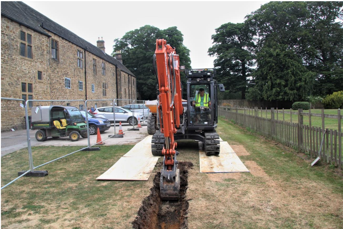
Figure 4. Trench excavation north of the Great Barn, with the listed cottages visible on the left hand side
