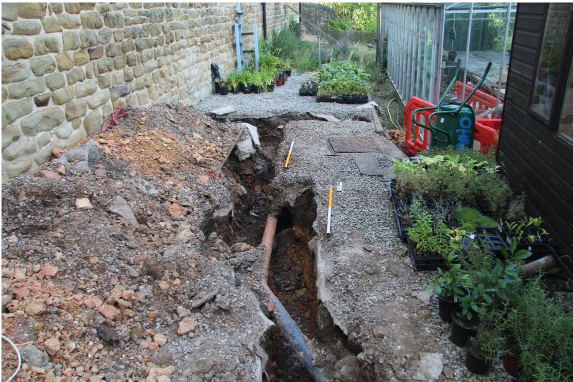
Figure 7. The pipe trench in the southern garden area, looking south (Scale 2 x 1m in 0,5m gradations)
