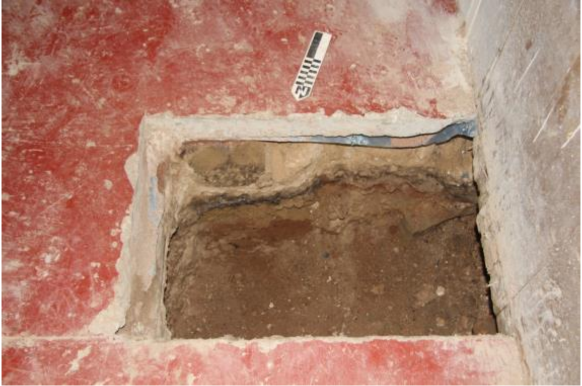
Figure 10. Section 5 - penetration through the wall and floor in the former stable building
