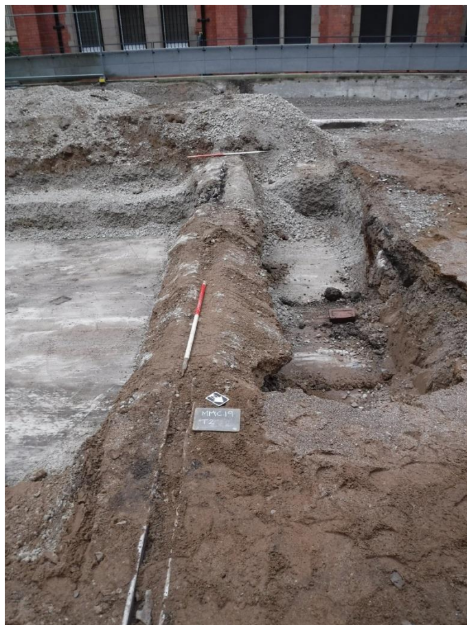
Figure 10. Concrete beam (204) carrying surface channel drain north-east/south-west across the courtyard. Scale: 2x1m.
