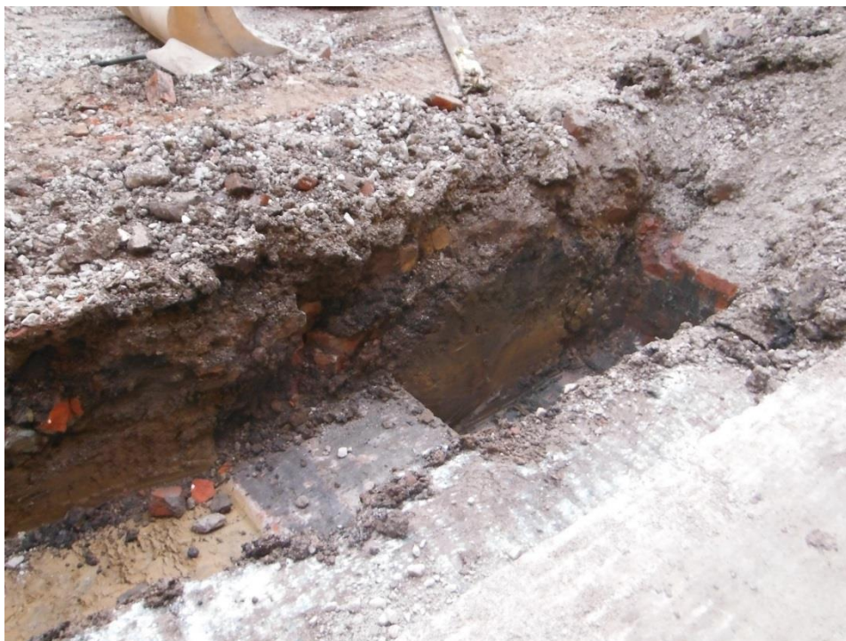
Figure 7. Oblique view of the south-west facing section during excavation of the engineering test-pit. Concrete slabs (103) and (105) visible in foreground. Brickcrete beam (107) and wall (106) visible in the centre. Wall (109) on concrete beam (110) visible on the right hand side of the photograph (south-east end of test-pit).
