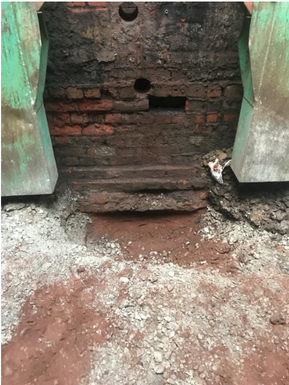
Stepped foundation of courtyard retaining wall, cut through and overlying natural clay
