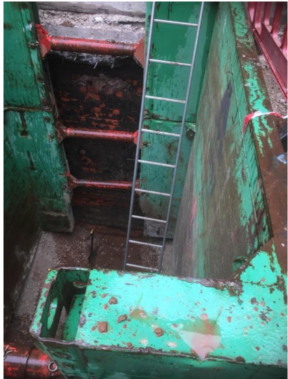
Depth of test-pit following removal of concrete slabs, made-ground deposits and natural clay to expose foot of wall
