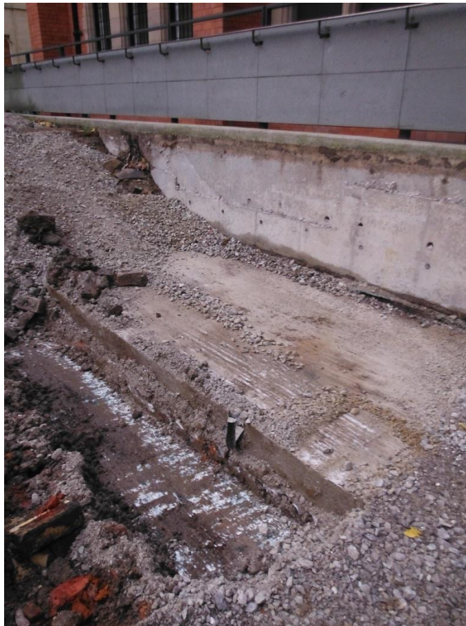
Figure 5. Foundation slab (103) for parapet wall around the courtyard, overlying lower slab (105) Found prior to excavation of the engineering test-pit. Looking south-west.
