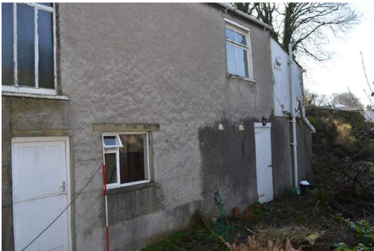
Plate 22: North west elevation of rear service range, looking south (Scale: 1 x 2m).
