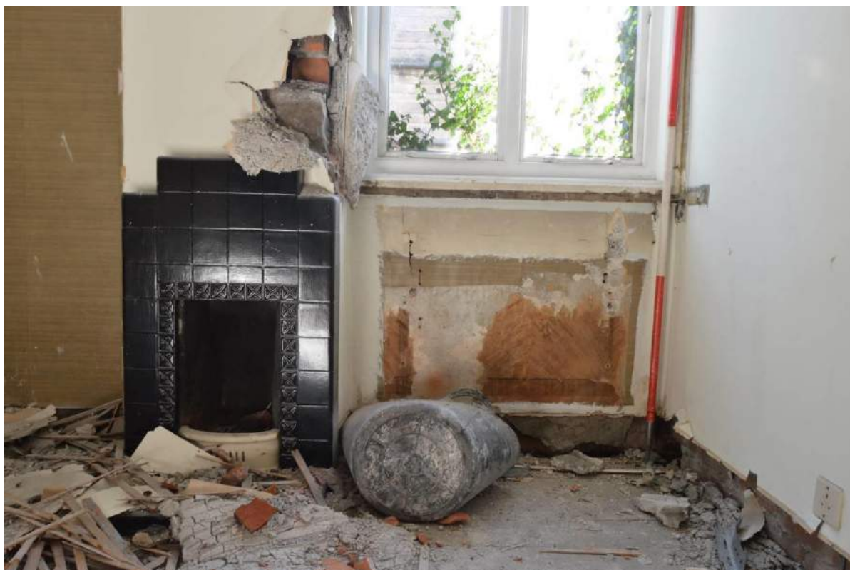
Plate 66: Fireplace in small first floor room. Note the trompe l'oeil wallpaper below the window (Scale: 1 x 2m).
