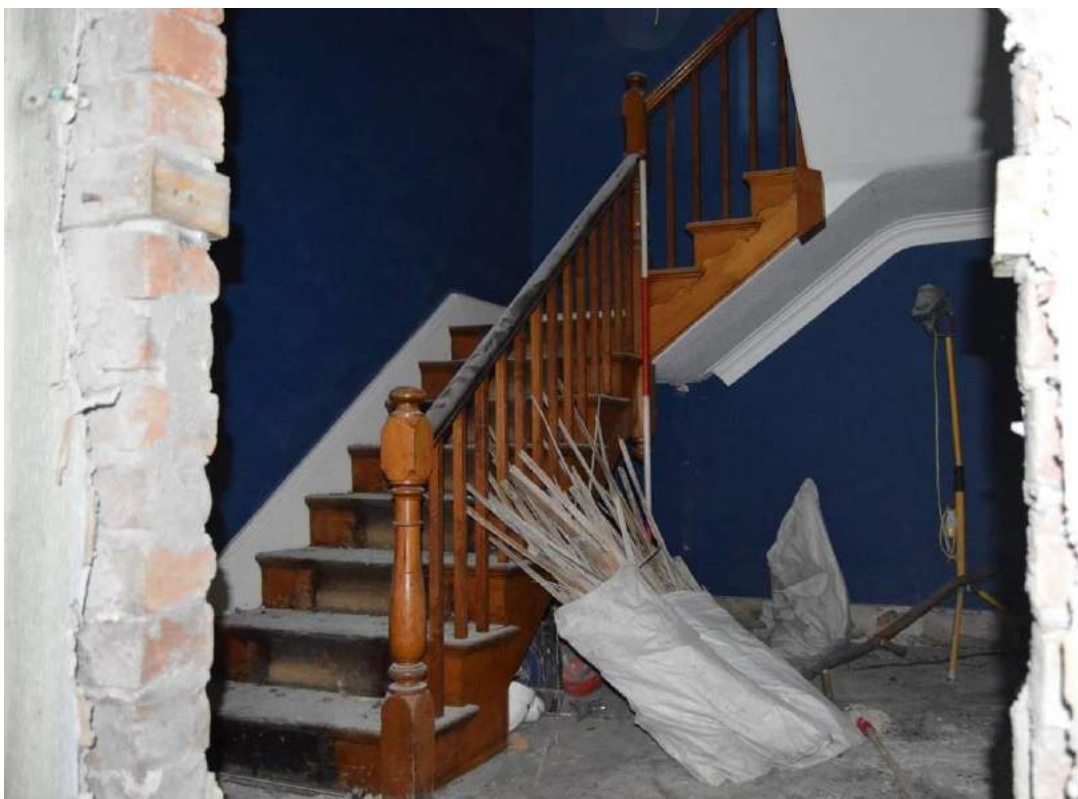
Plate 38: View of the lower flights of the staircase, from H1, facing west (Scale: 1 x 2m).
