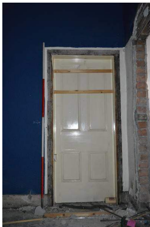
Plate 41: Sealed doorway which originally lead into the front room now occupied by the north shop (Scale: 1 x 2m).
