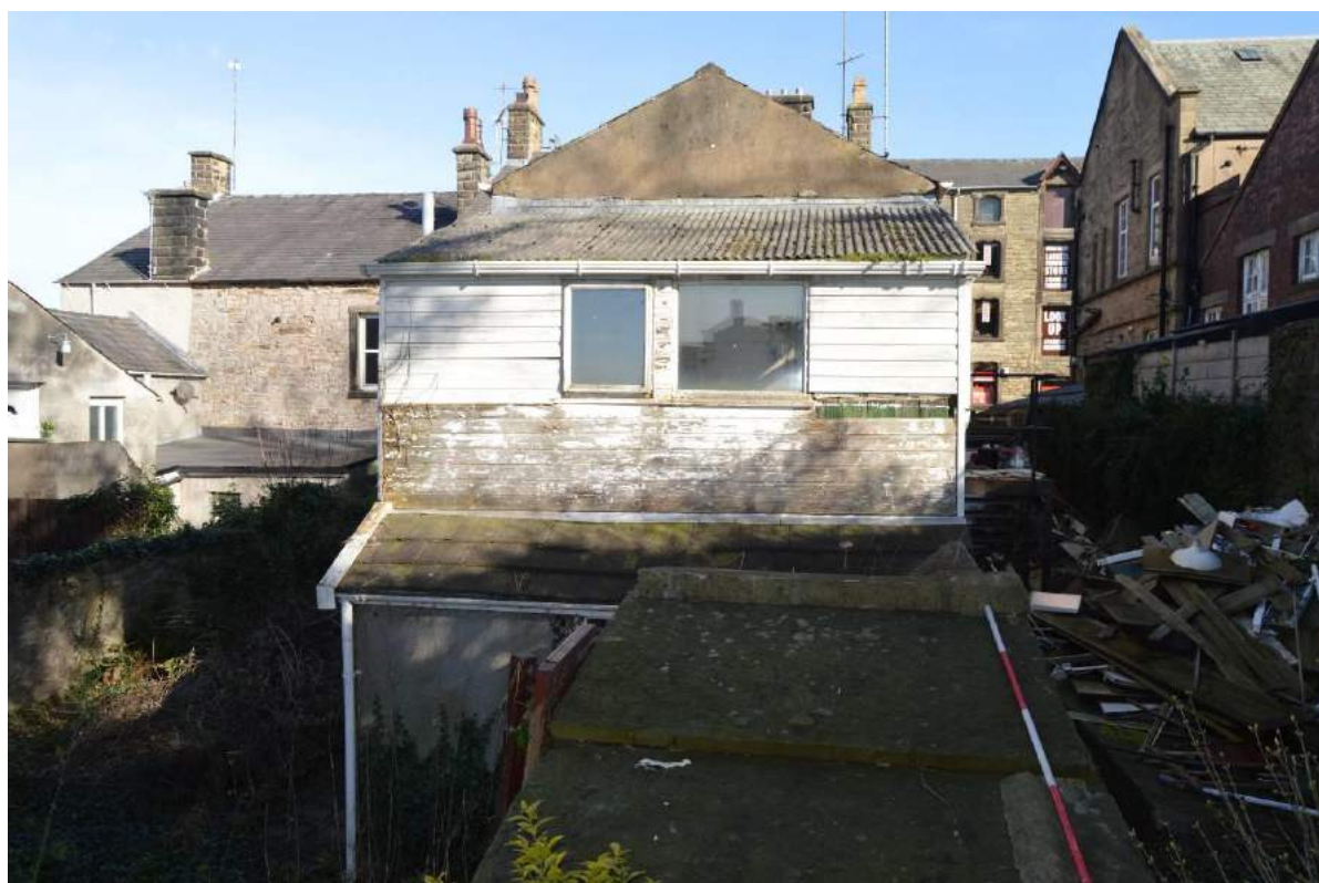
Plate 24: Rear gable wall of service range with timber frame projection (Scale: 1 x 2m).
