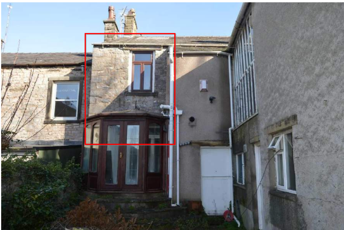
Plate 18: Exposed section of the principal building's rear elevation with the projecting rear service range to foreground (Scale: 1 x 2m).
