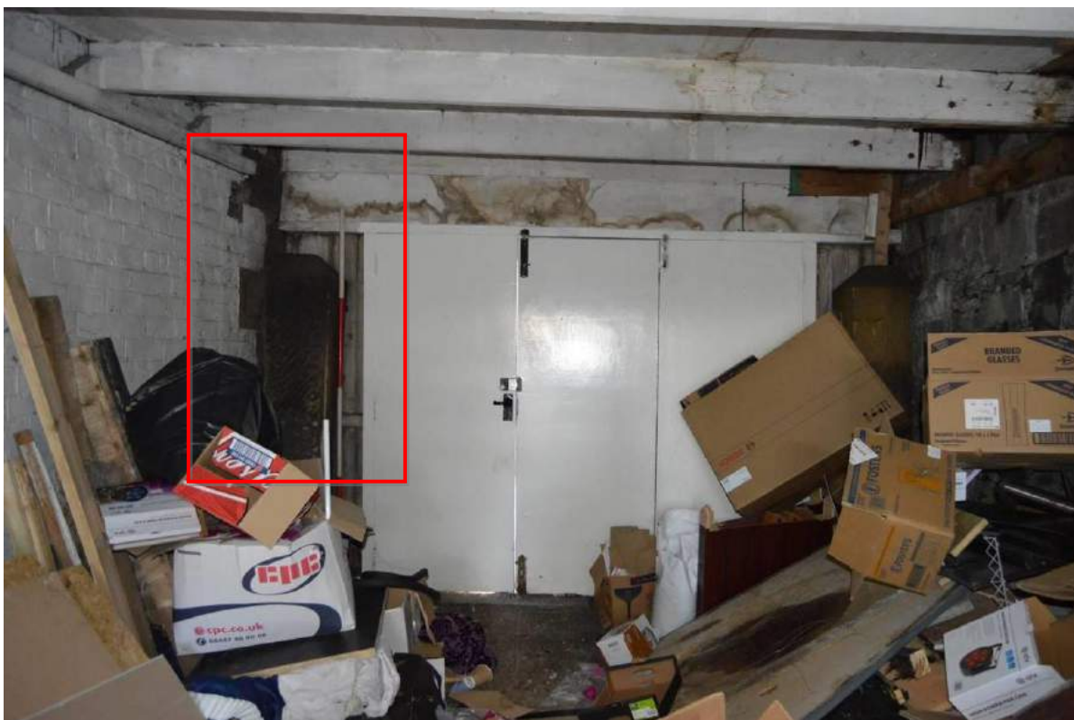
Plate 13: View north east of the side elevation, boundary wall and garage interior. Note to the left the quoins stones and the gate pillars (Scale: 1 x 2m).
