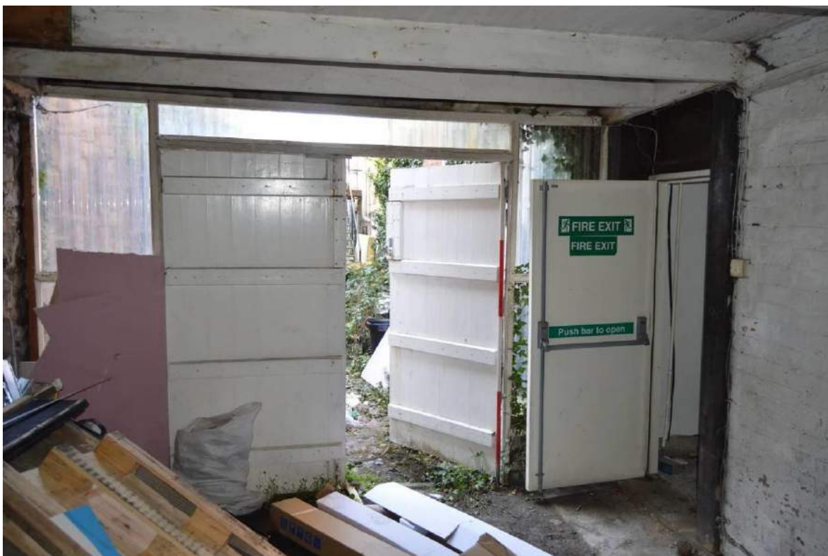
Plate 12: South east side elevation viewed from inside the garage. Note the dressed stone door surround to the side entrance of the building (Scale: 1 x 2m).
