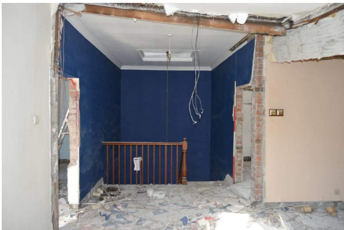
Plate 57: Landing, viewed from south east. Note the internal walls are missing (Scale: 1 x 2m).
