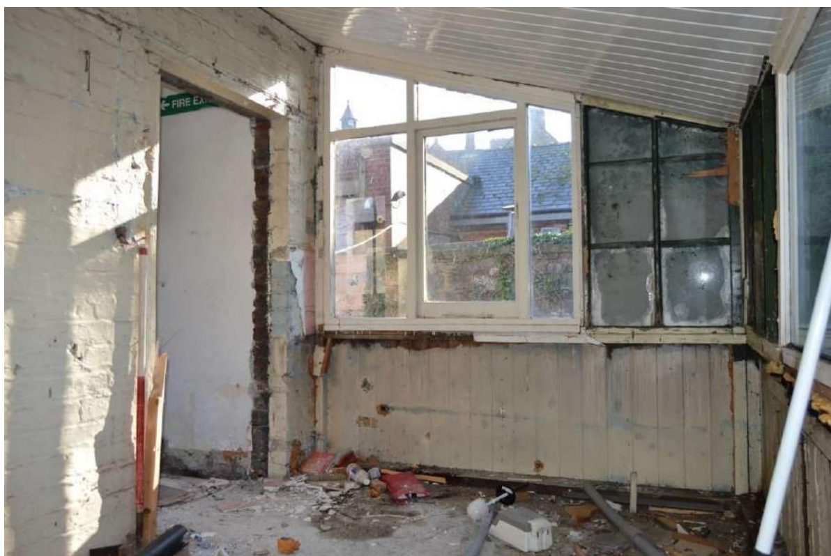
Plate 74: Interior of the 'glass room' at the rear of the rear service range (Scale: 1 x 2m).
