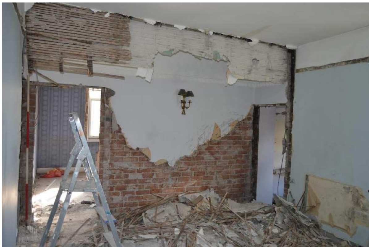
Plate 68: Interior of rear bedroom (F5). Note the lath and plaster dividing wall for the corridor (Scale: 1 x 2m).
