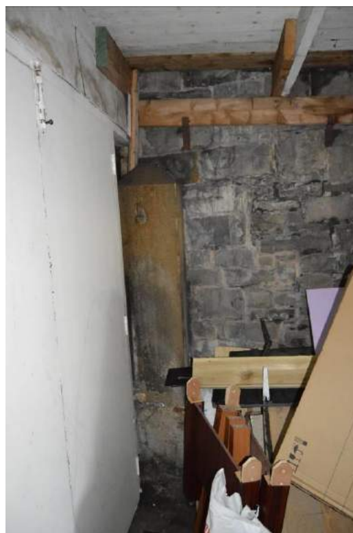
Plate 15: The opposing north east stone gate pillar, set against the boundary wall.
