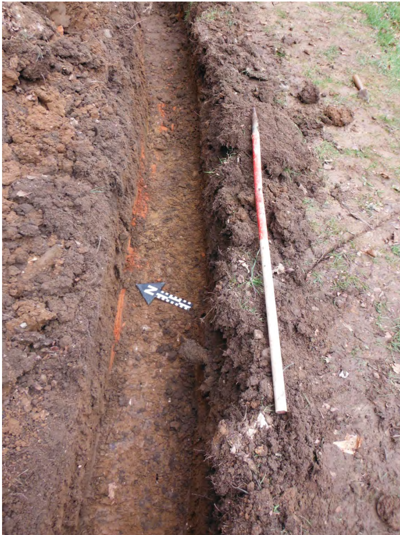
Figure 15 Drain (034) visible in the trench for the new storm drain, looking east
