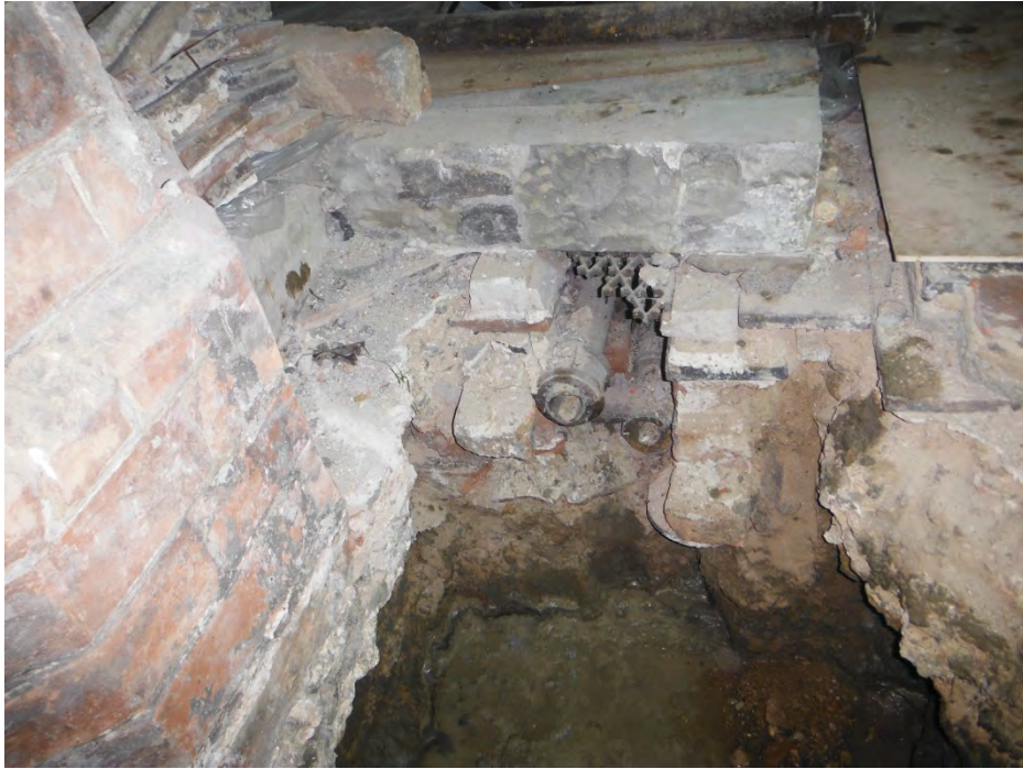
Figure 11 Heating duct [020] system overlaid by the concrete floor of the chancel
