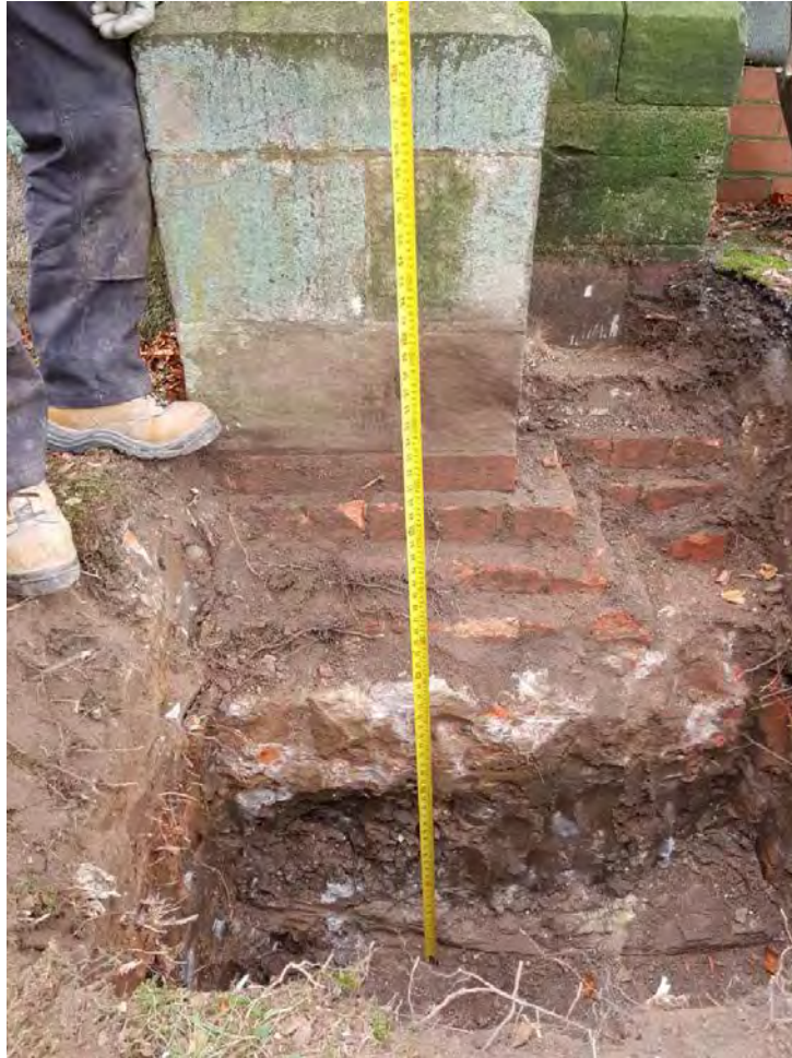
Figure 6 Stepped brickwork and concrete underpinning foundation underneath the east wall © Paul Mendham Stonemasons Ltd
