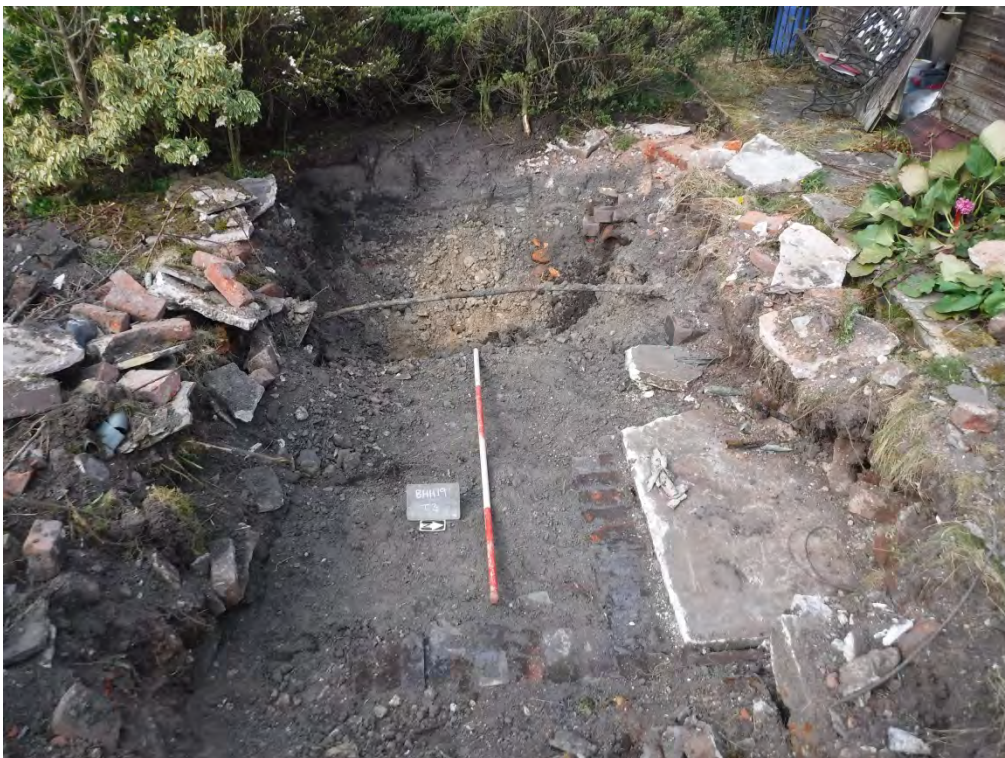
Figure 13. Trench 3, showing remains of a demolished 20th century building to the rear of the bungalow, looking west. Scale: 2m. Foundation courses of walls visible in the foreground alongside a concrete slab (304). Fragments of corrugated asbestos panelling observed in fill (some visible on edge of concrete slab), so trench was abandoned.
