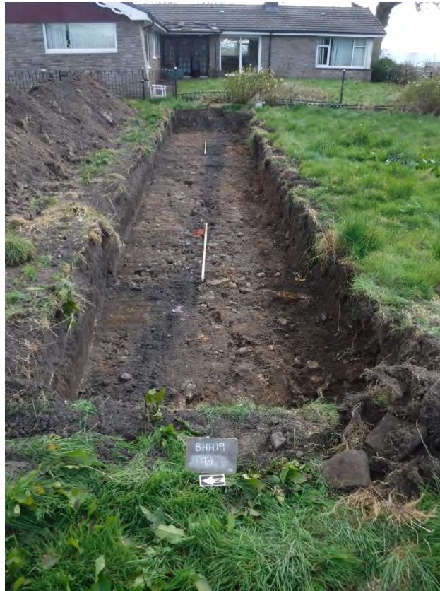
Figure 14. Trench 4, showing cut and fill of drainage soakaway [403]/(404) in the base, heading towards the modern manhole chamber of a foul-drain at the eastern end, looking east. Scale: 2x2m.
