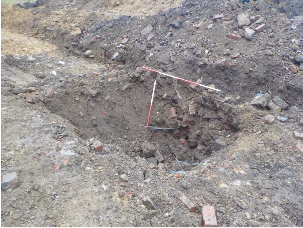
Figure 4. Modern Demolition Debris within fill (003). Note the abundance of brick, concrete, cabling and other modern detritus
