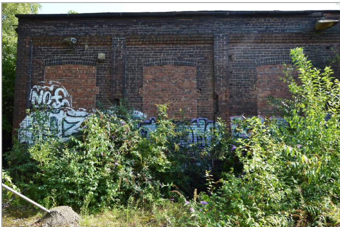
Plate 36: Three bays of the building showing the relief brickwork to Structure 9. Scale 2m.
