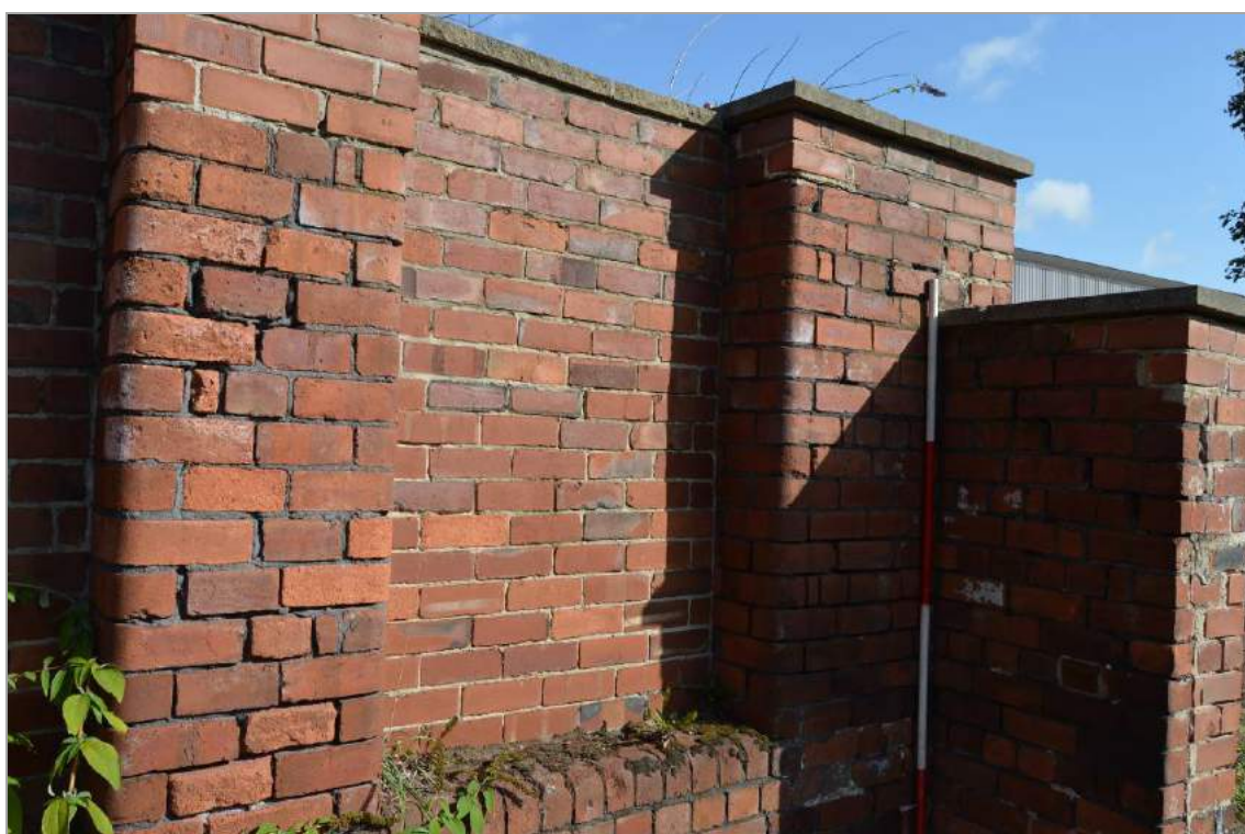
Plate 19: Ground floor window and other features in Structure 4, facing north east. Scale 2m.
