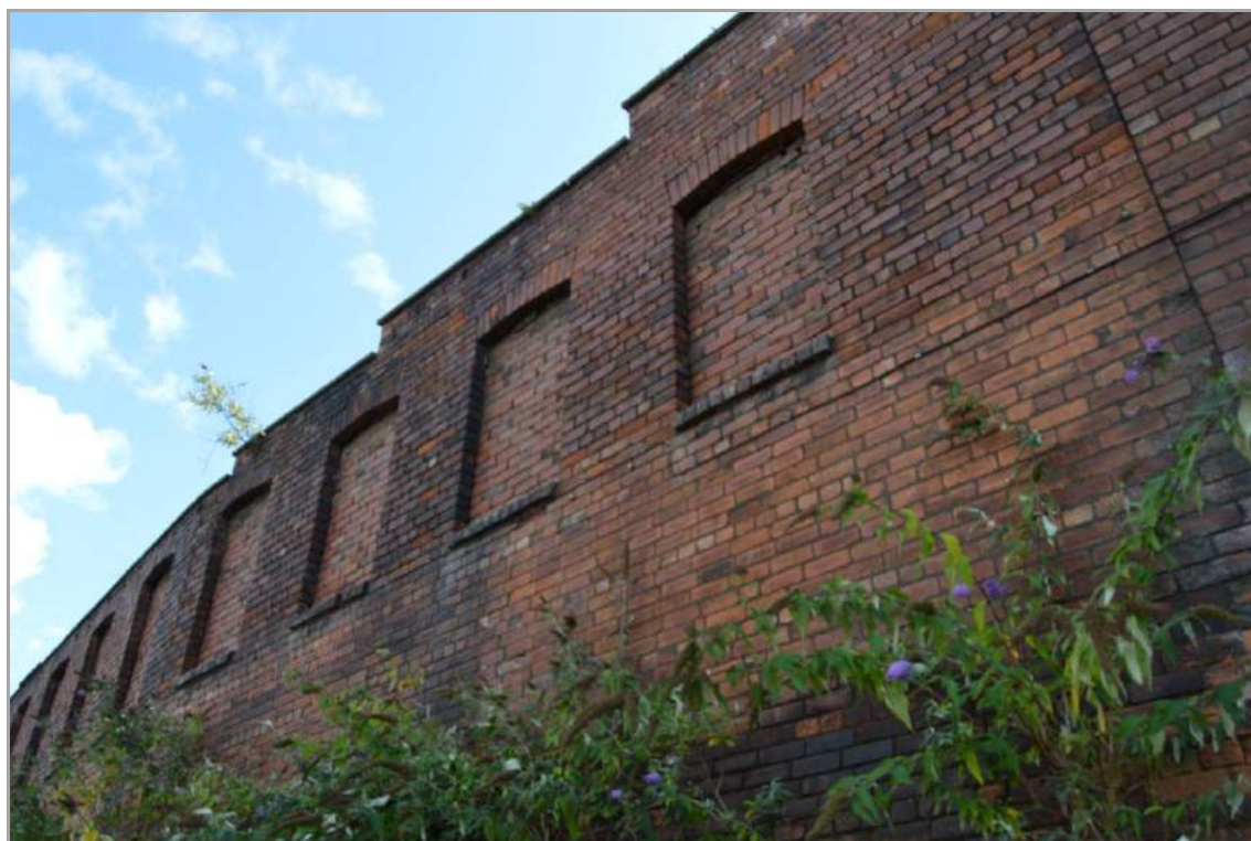
Plate 20: Detail north face of Structure 5 (facing east). Note the deviation in the course of the wall.
