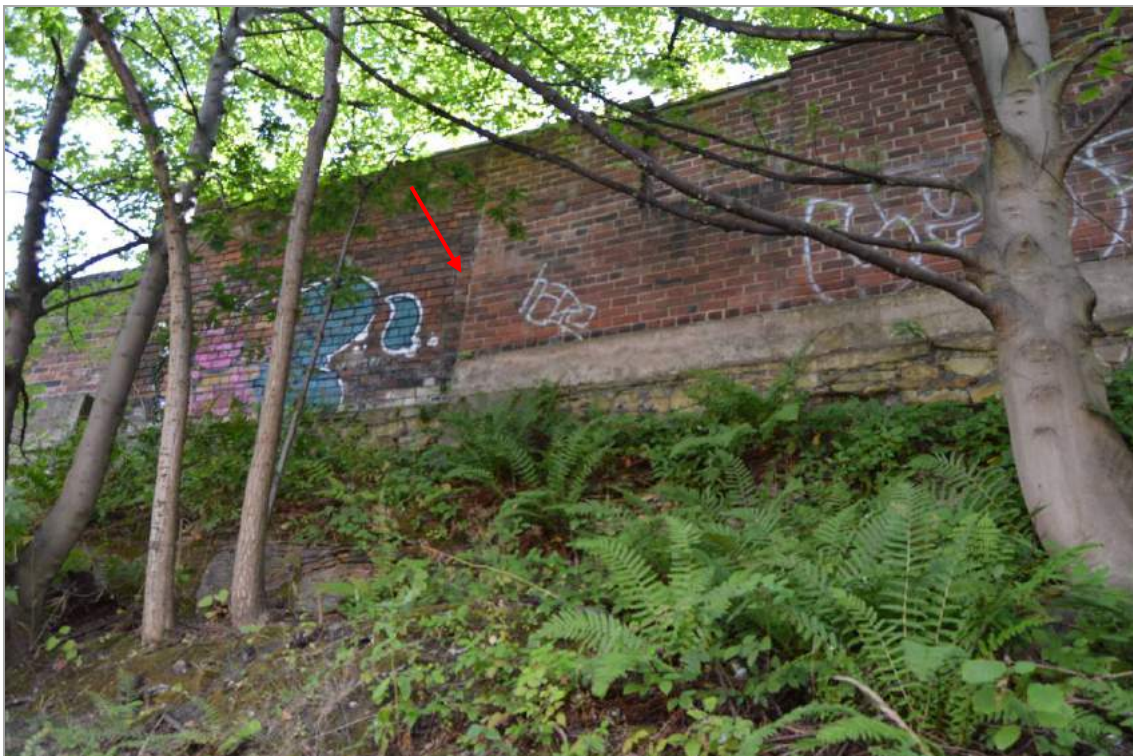
Plate 5: The north aspect of Structure 1 (facing south east) with construction break indicated (with structure 7, left).
