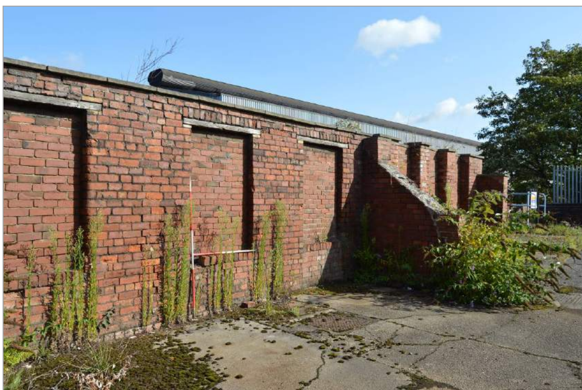
Plate 24: Blocked widows and east return of Structure 5. Scale 2m.
