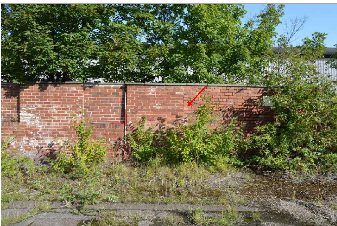
Plate 11: Structure 1, the north eastern corner of the former building, with construction break indicated (facing north). Scale 2m.
