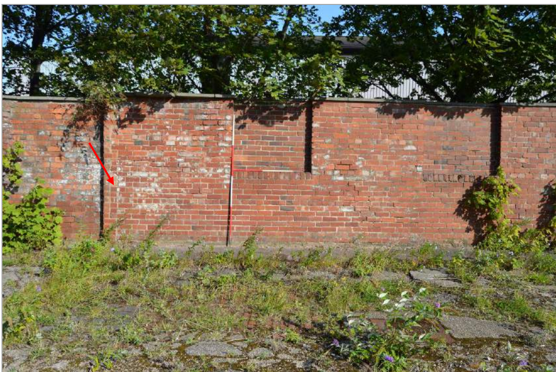
Plate 10: Structure 1, the north western corner of the former building, with the return indicated (facing north). Scale 2m.
