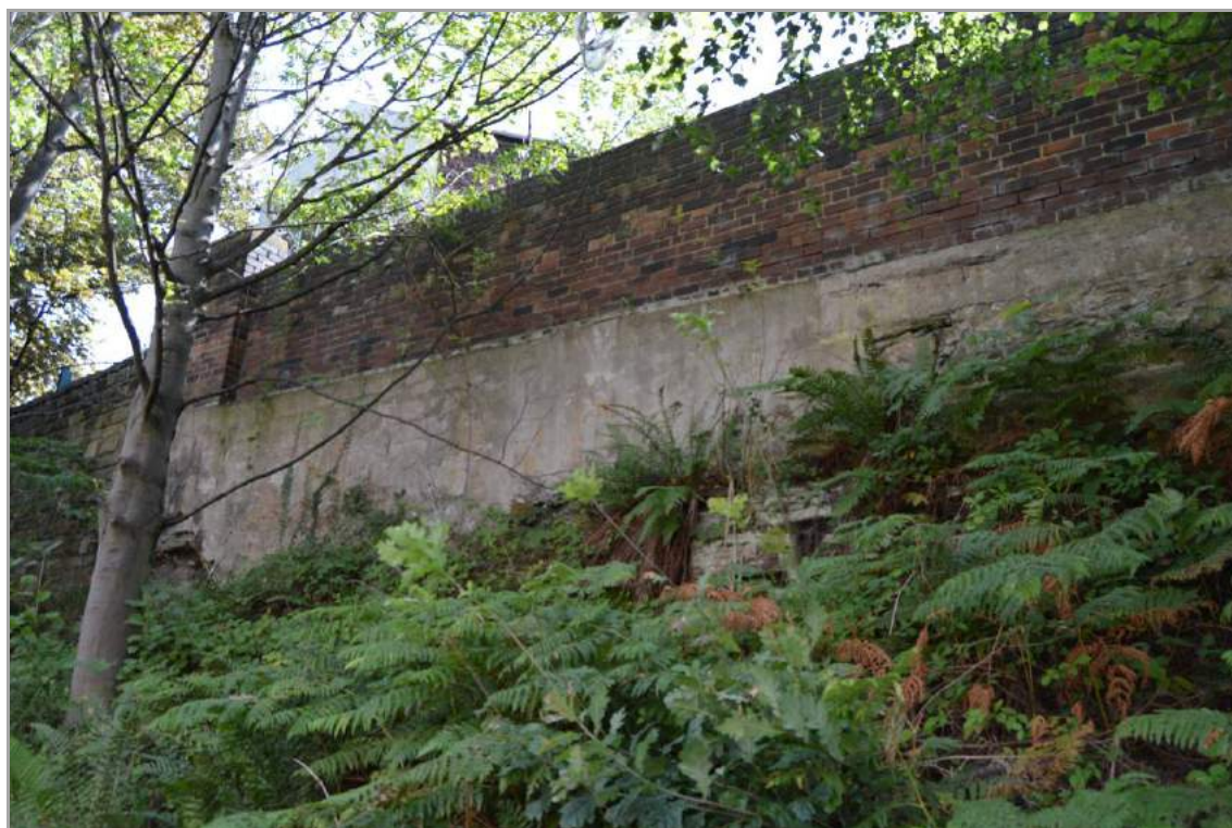
Plate 32: Structure 8, section of perimeter wall, from the canal towpath (facing south east)..
