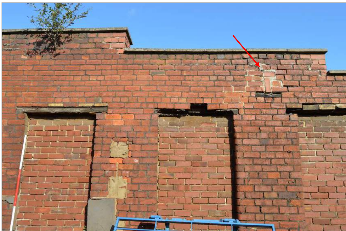
Plate 25: Blocked widows and truss slot (indicated) of Structure 5 (facing north). Scale 2m.
