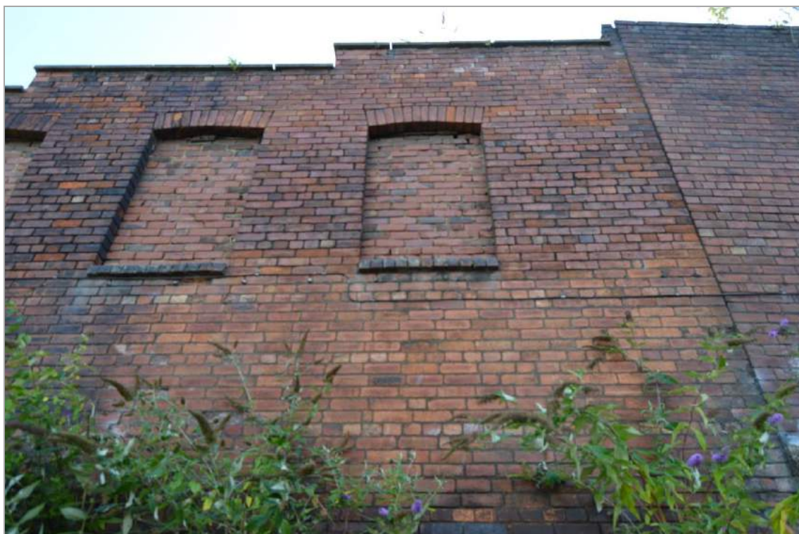
Plate 21: Blocked apertures to the north face of Structure 5.
