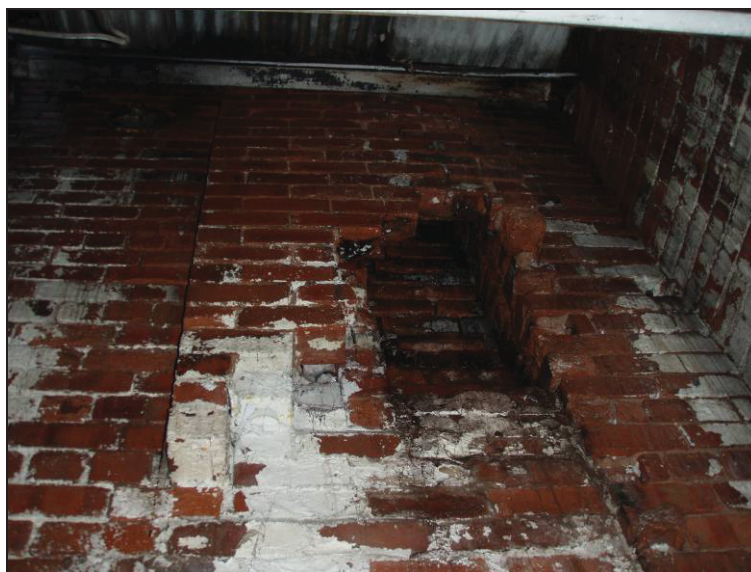
Fig. 25 Chimney breast located on the other side of the south wall of the chapel above the large entrance.
