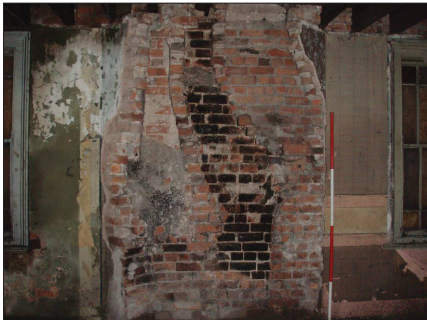
Fig. 28 East wall of the rectory showing the damaged central chimney breast. (Scale: 2m)
