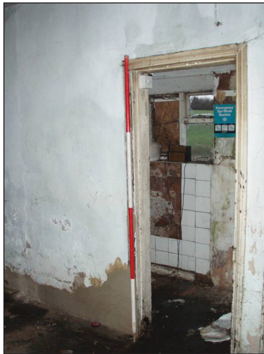
Fig. 43 Doorway to small extension on the east side of Room One. (Scale: 2m)
