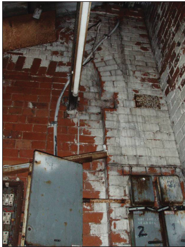
Fig. 26 Brick arch which would have framed an original window of the schoolhouse. Also note that the walls in the corner are not keyed in.
