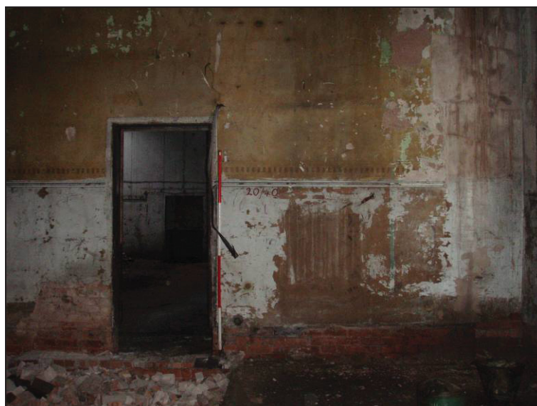
Fig. 13 Western doorway in the south wall giving access to the chapel from the school room. The brickwork at base of wall demotes height of original sloping floor level. (Scale: 2m)
