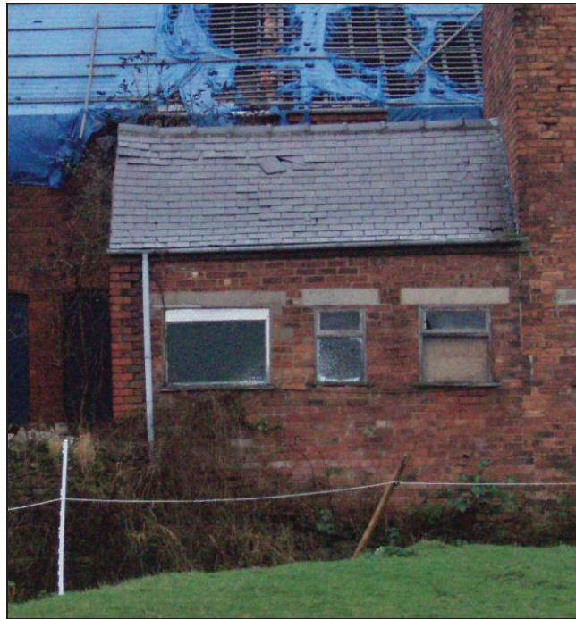
Fig. 65 East elevation of the office and toilet block showing where the wall abuts the rectory wall.
