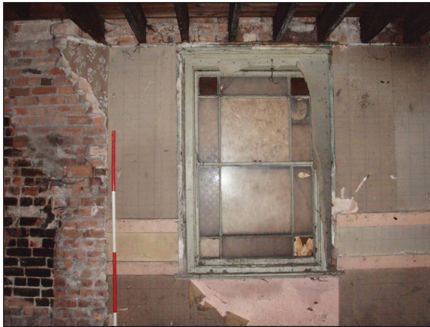
Fig. 29 One of the sash windows flanking the chimney breast on the east wall of the rectory. (Scale: 0.5m graduations)
