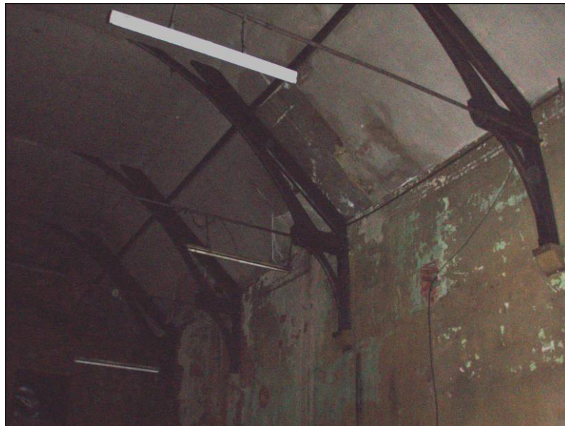
Fig. 7 Interior of Chapel showing the wooden ceiling beams on the south side.
