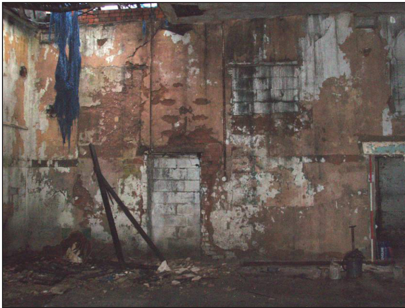
Fig. 20 The east wall of the schoolhouse showing the in-filled windows and doorway. (Scale: 2m)
