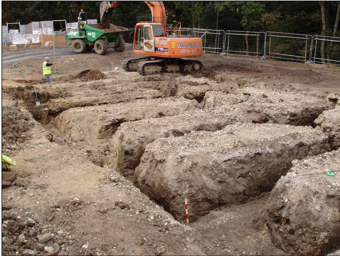
Figure 3. The extent of ground works across plots 9 through to 12 viewed facing north west.
