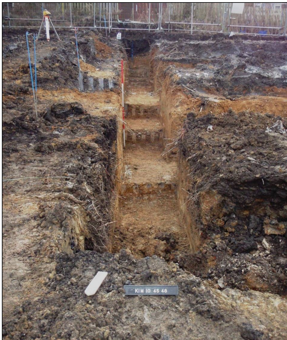
Fig. 2: North facing section of an eastern foundation trench within plots 45-48, showing maximum depth of ground reduction.
