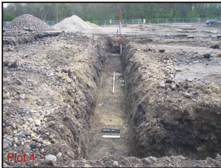
Fig. 4: Northern wall of Plot 4. The east end of the foundation trench shows the remains of the black made ground/organic level on top of the redeposited clay layer visible in the west and central areas of the trench.
