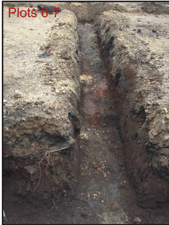
Fig. 6: General view of the foundations of the wall shared by Plots 6 and 7 (looking east).
