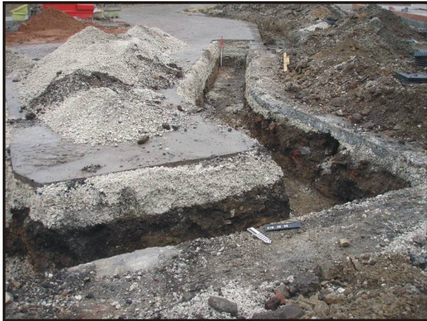
Fig. 29: General services trench cut through the new road. View of the west side, looking south.
