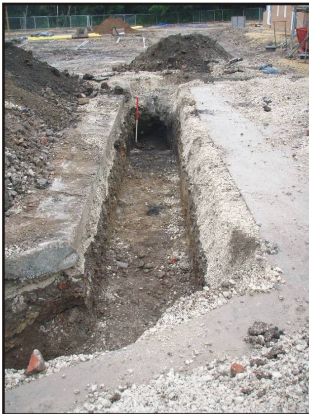
Fig. 30: General services trench, cut through the new road. View of the west side, looking west.
