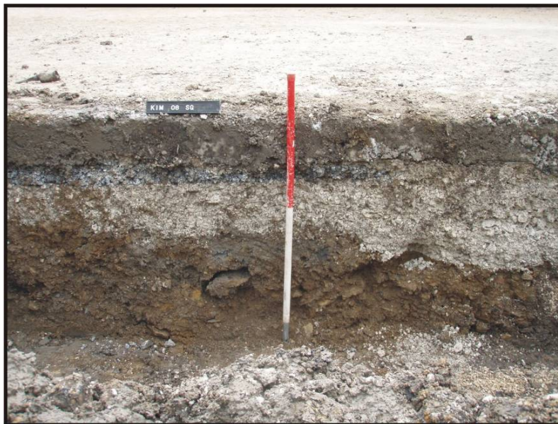
Fig. 26: Section of general services trench. The upper two levels correspond with the new road laid to service the dwellings.
