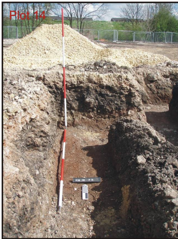
Fig. 12: North end of foundation trench for the eastern wall of Plot 14. The black made ground was redeposited in this area after being excavated in the west part of the development area.
