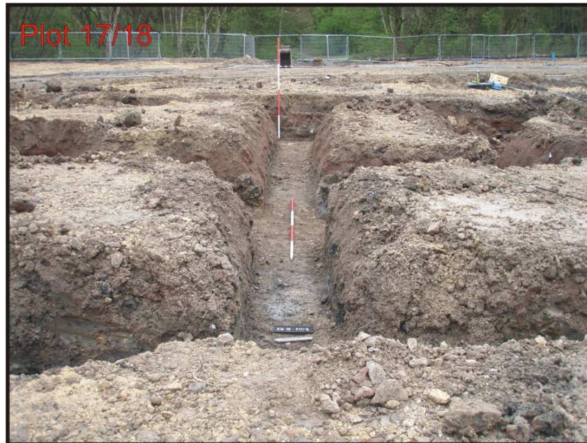
Fig. 17: Foundation for the wall dividing Plots 17-18. A thick layer of red sand can be seen in the eastern part of both Plots.
