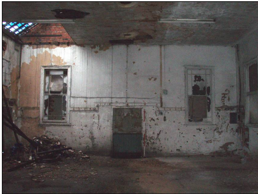
Fig. 22 South wall of the schoolhouse with the entrance at the centre. (Scale: 2m)
