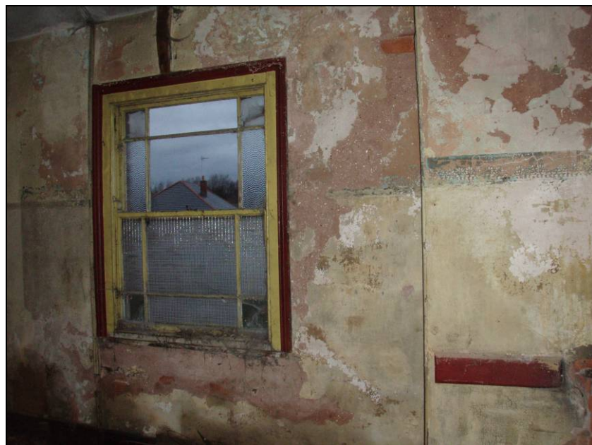
Fig. 34 Sash window on the east wall of the upper storey of the rectory.
