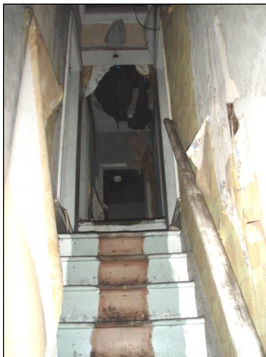
Fig. 46 Staircase in the 1908 extension showing the collapsed roof.
