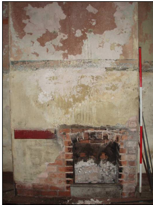
Fig. 33 Fireplace located on the east wall of the upper storey of the rectory. (Scale: 2m)
