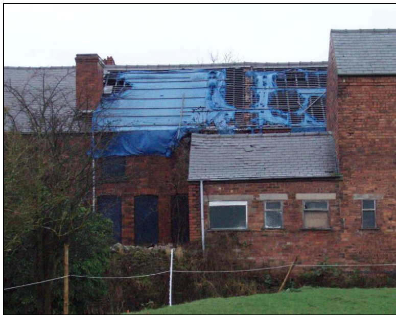
Fig. 62 East side of the schoolhouse roof showing damage.
