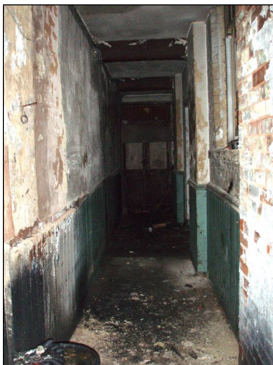
Fig. 24 The passage between the schoolhouse and the new living accommodation (looking west).
