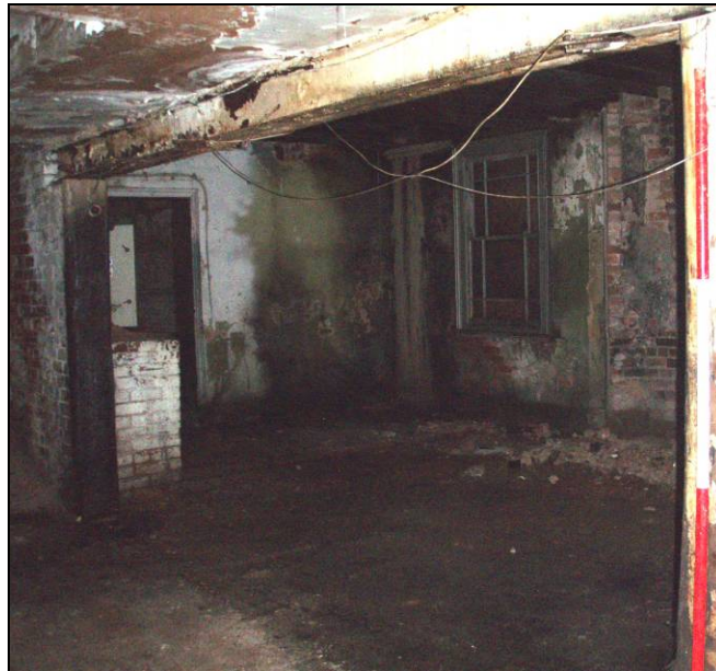
Fig. 30 Modern RSJ entrance to the rectory from the modern passage. (Scale: 0.5m graduations)
