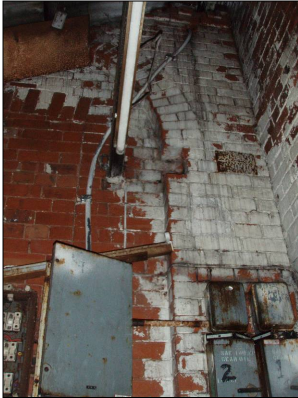
Fig. 26 Brick arch which would have framed an original window of the schoolhouse. Also note that the walls in the corner are not keyed in.
