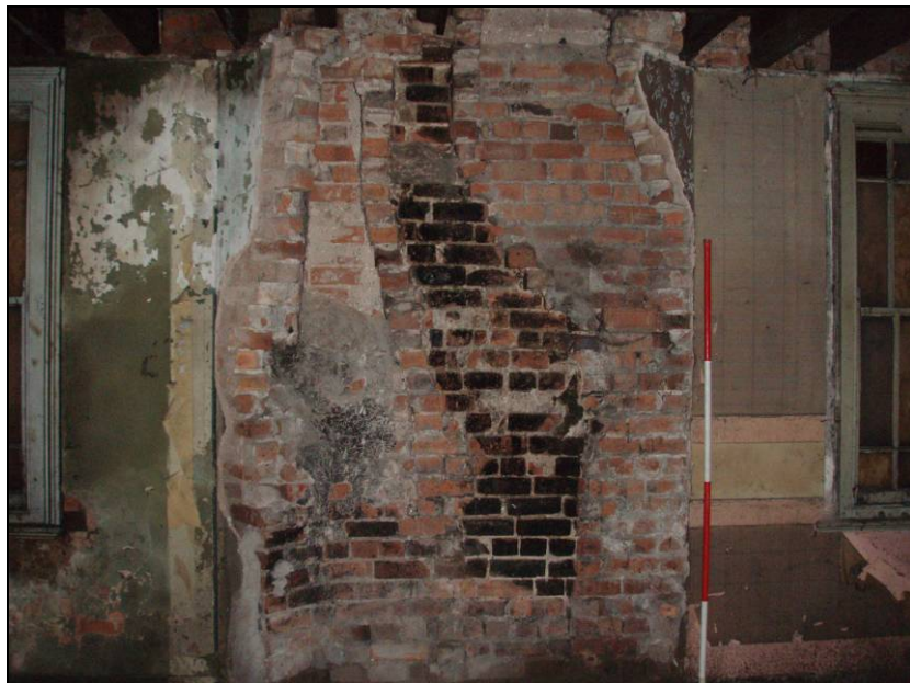
Fig. 28 East wall of the rectory showing the damaged central chimney breast. (Scale: 2m)
