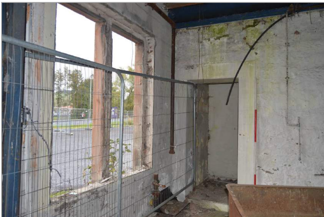
Plate 63: Interior of mullioned window in Building 2 with linking doorway to Building 1 (facing south east).
