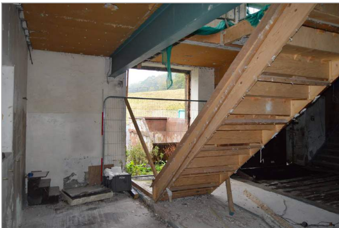
Plate 42: Rear view of the single flight of stairs adjacent the south personnel entrance (facing east). Scale 2m.
