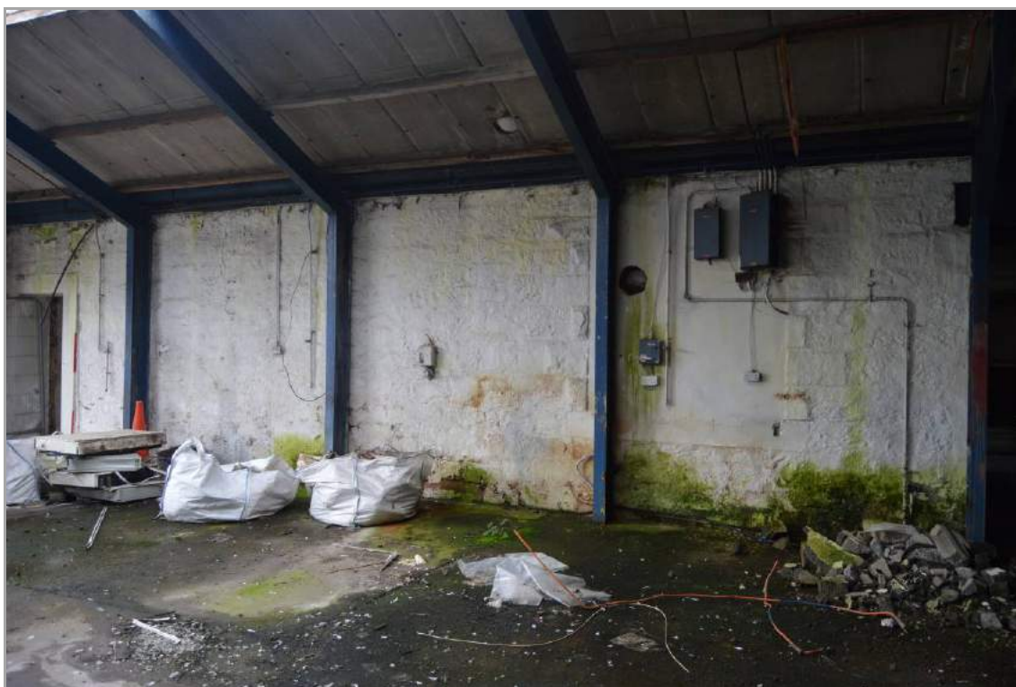
Plate 64: Former exterior wall of Building 1 internal to Building 2 (facing south). Note the blocked window. Scale 2m.
