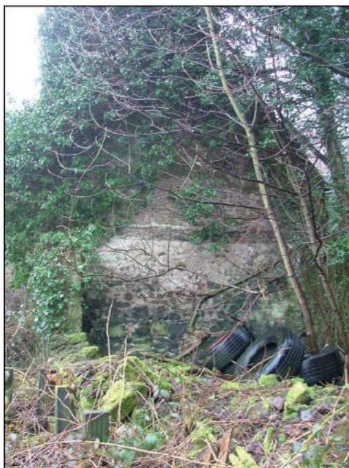
Plate 9: North elevation of Building A with the remains of a further building in the foreground
