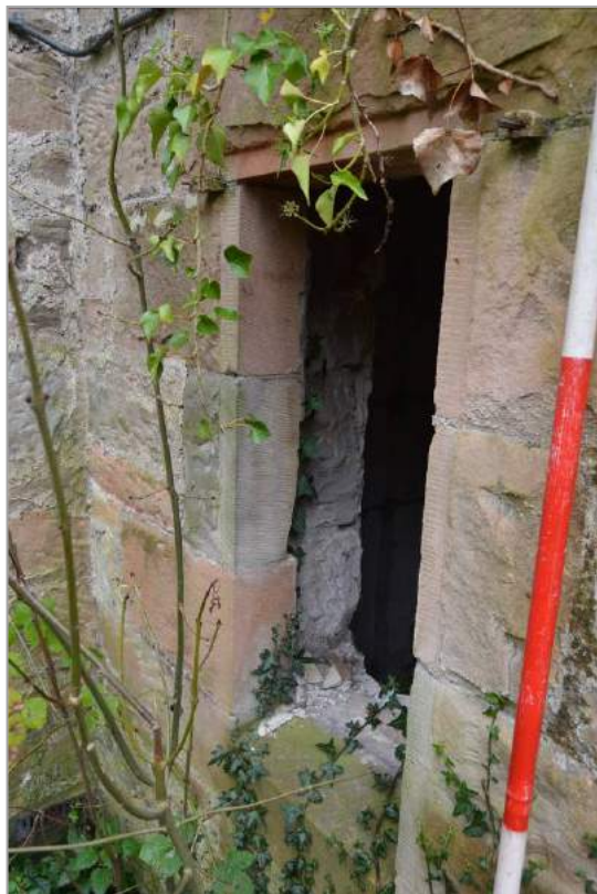
Plate 28: Window aperture in to north facing elevation of extension structure in front of west elevation (facing south east). Scale 2m.
