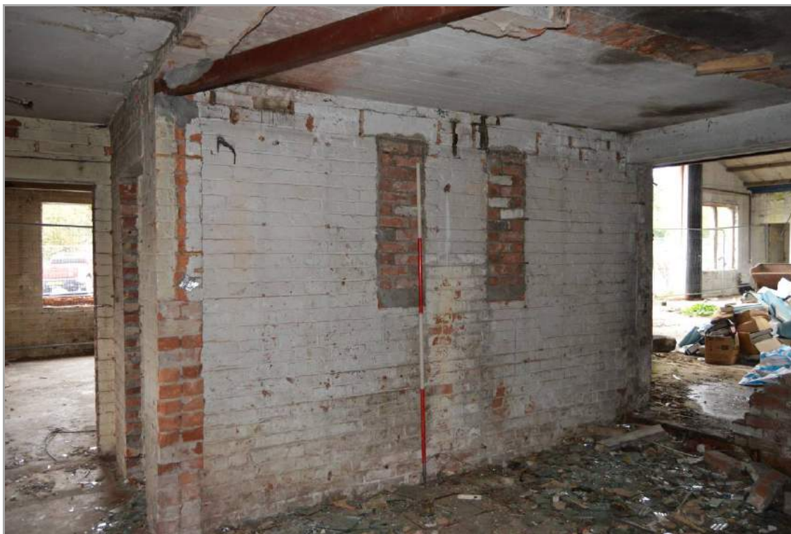
Plate 95: Interior of Building 4 (facing south east). Note the blocked windows to the interior wall. Scale 2m.
