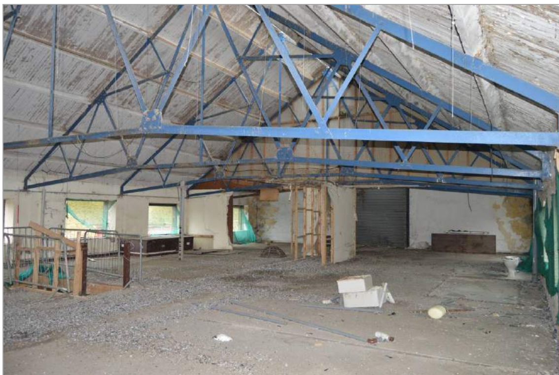
Plate 53: General interior view of Building 1, first floor (facing south west). Scale 2m.
