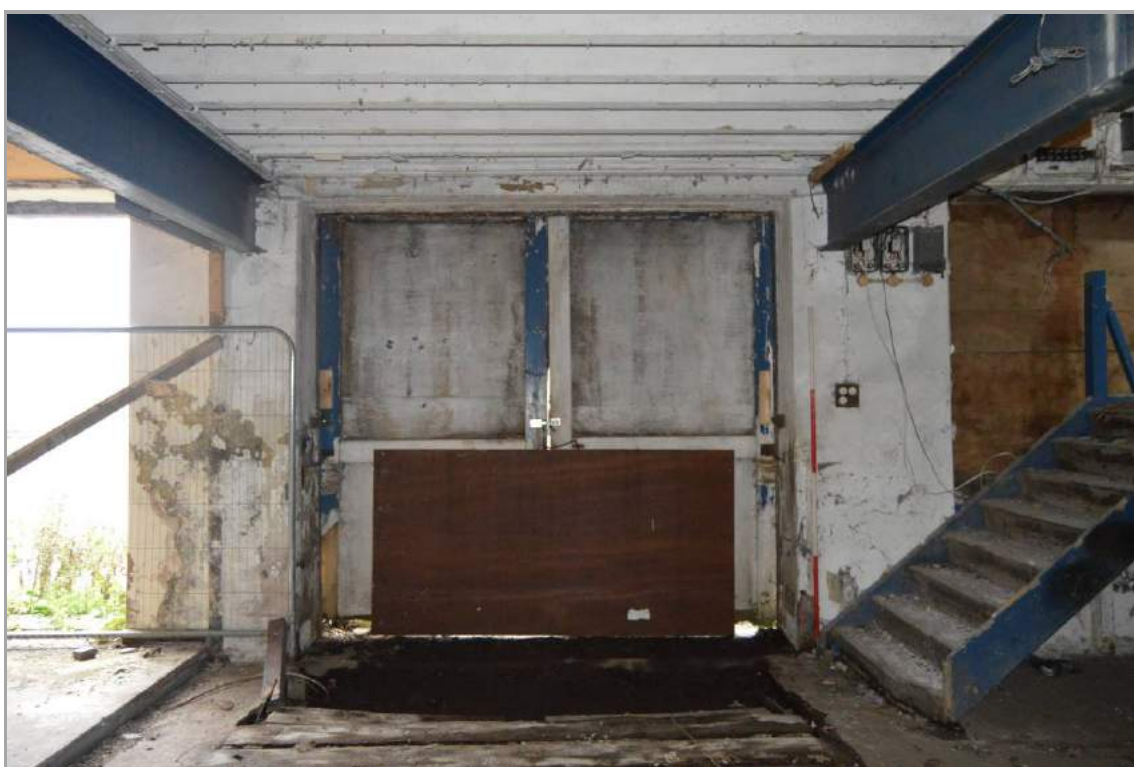
Plate 43: Interior of sliding good's doors (facing south). Note the timber plank flooring to the foreground. Scale 2m.
