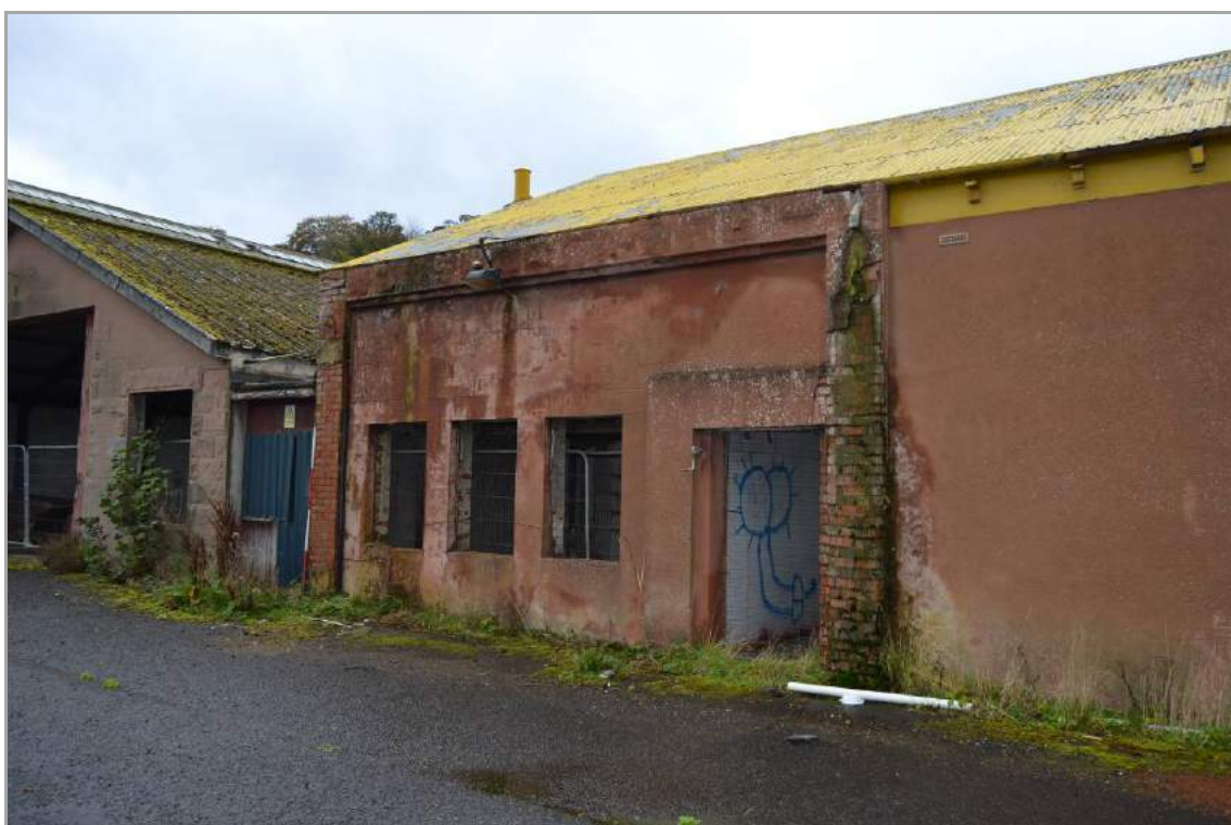
Plate 80: East elevation of Building 4 (facing south west). Note the different configuration of the façade as it relates to the range of ancillary/service rooms behind. Scale 2m.
