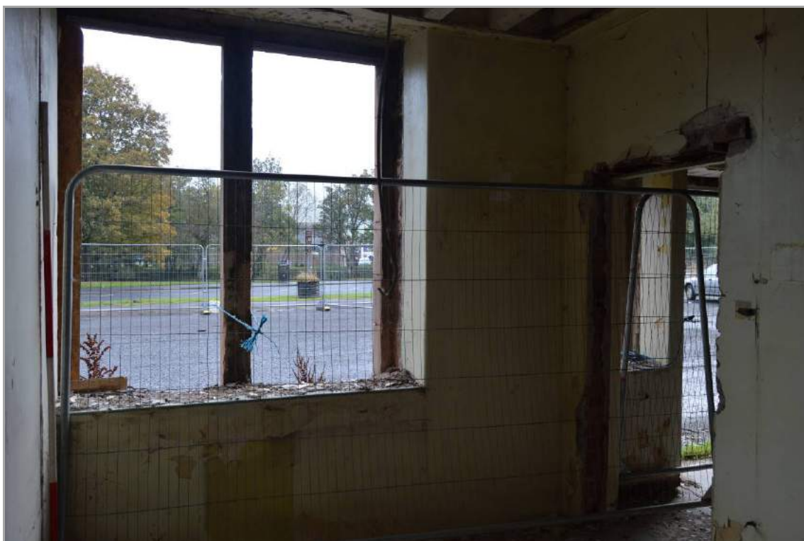
Plate 34: North room of the ground floor of Building 1 (facing east). Note the three light window has been bisected by addition of a later partition wall. (Scale 2m).
