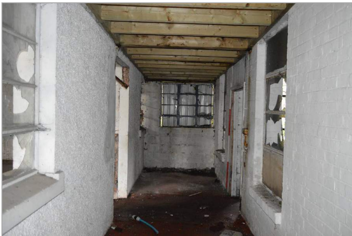
Plate 77: Interior of linking structure, Building 3 (facing west). Note the pebble dashed and brick side walls which were originally exterior elevations of Buildings 2 and 4. Scale 2m.
