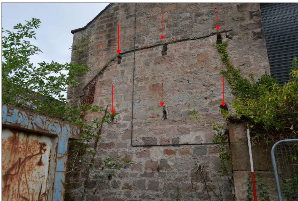
Plate 26: Joist and beam slots (indicated) for a covered external staircase to the west elevation (facing north east). A mortared flashing line is also visible. Scale 2m.
