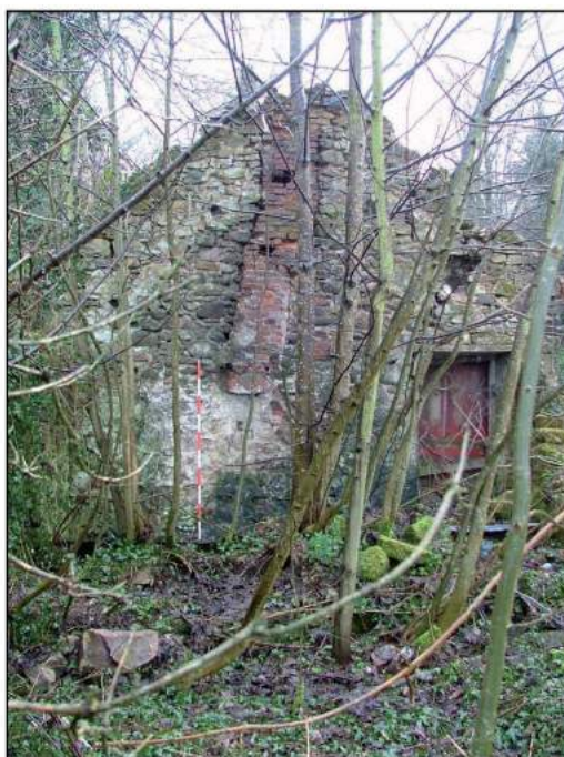
Plate 15: View looking west showing the internal cross wall which separated the two rooms of Building B (Scale = 2m)
