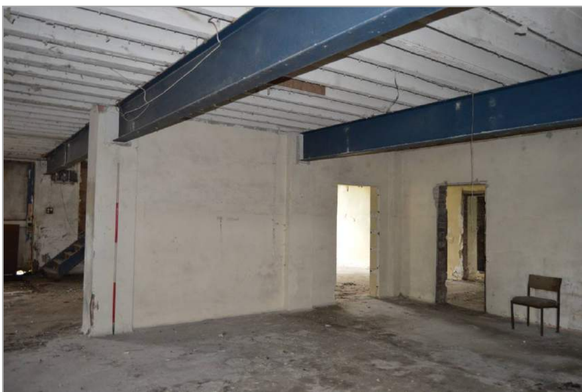
Plate 39: Ground floor space of Building 1 (facing south west) showing sections of internal dividing walls. Scale 2m.
