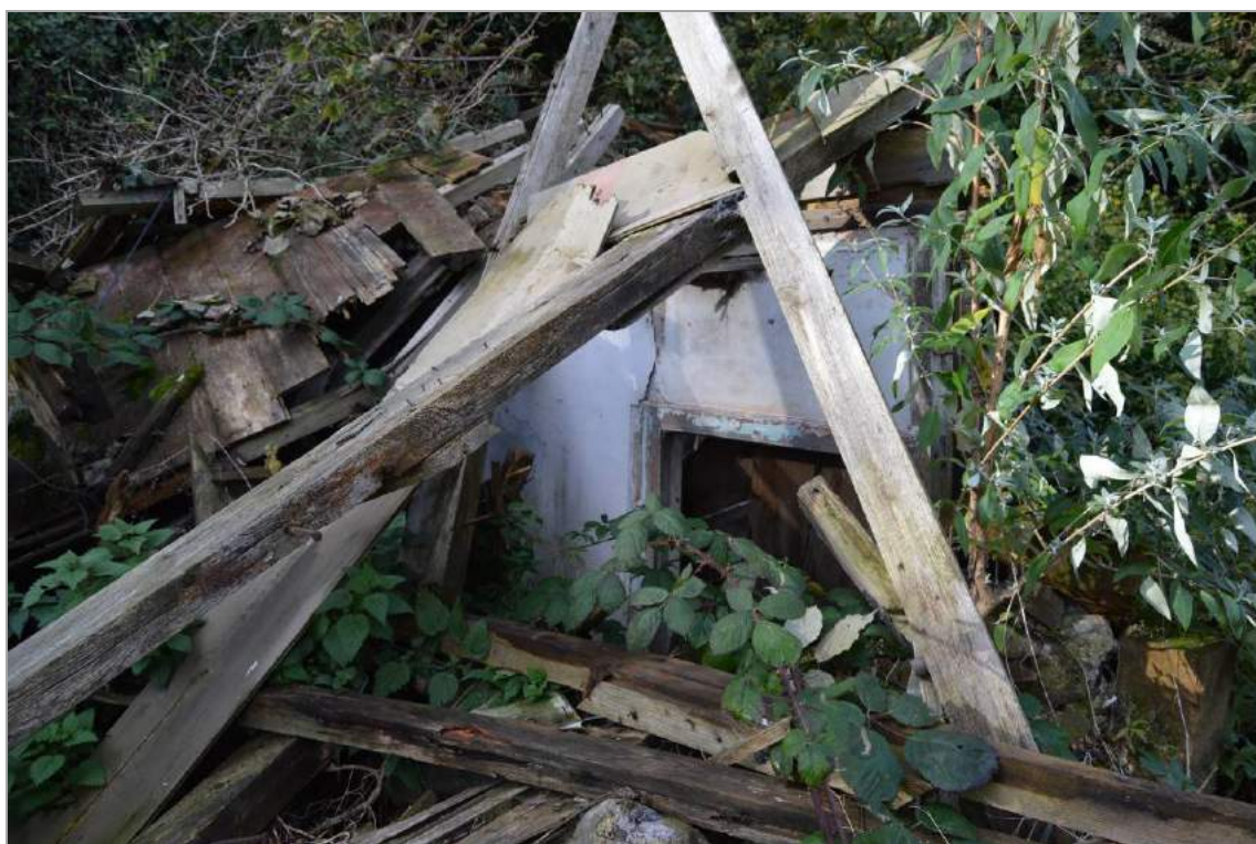
Plate 105: Collapsed interior of Building A.
