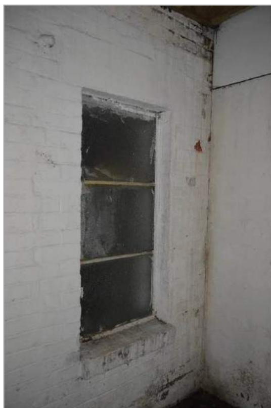
Plate 78: Interior of linking structure, Building 3, with previously outside facing window (north east). Scale 2m.
