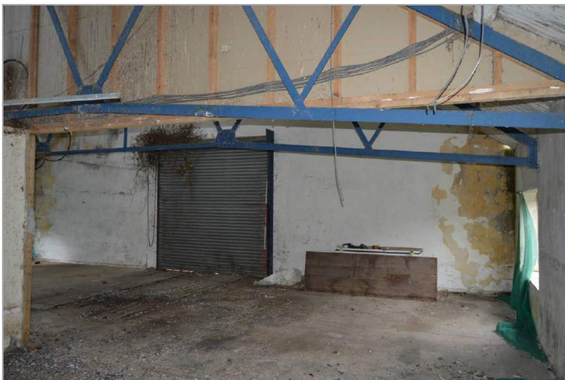
Plate 55: Roller shutter door to Building 1 first floor (facing south west). Scale 2m.
