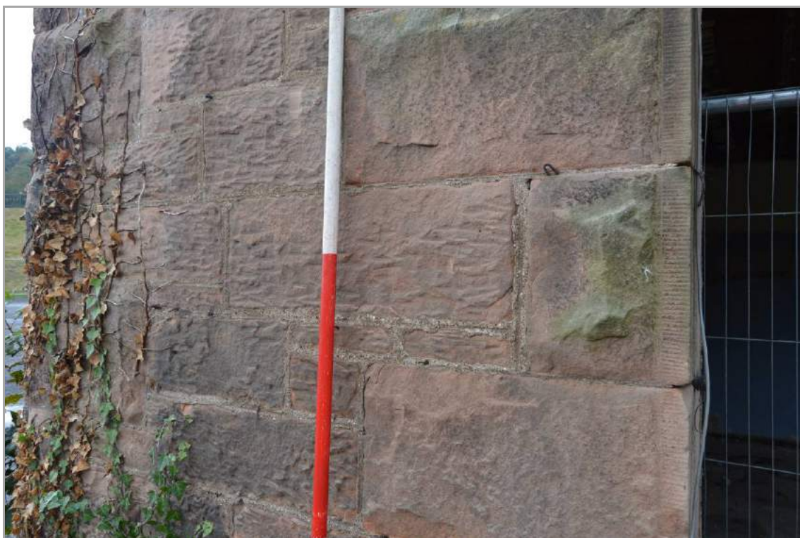
Plate 11: Roughly tooled ashlar and rusticated quoin detail to east elevation (facing north west). Scale 2m.
