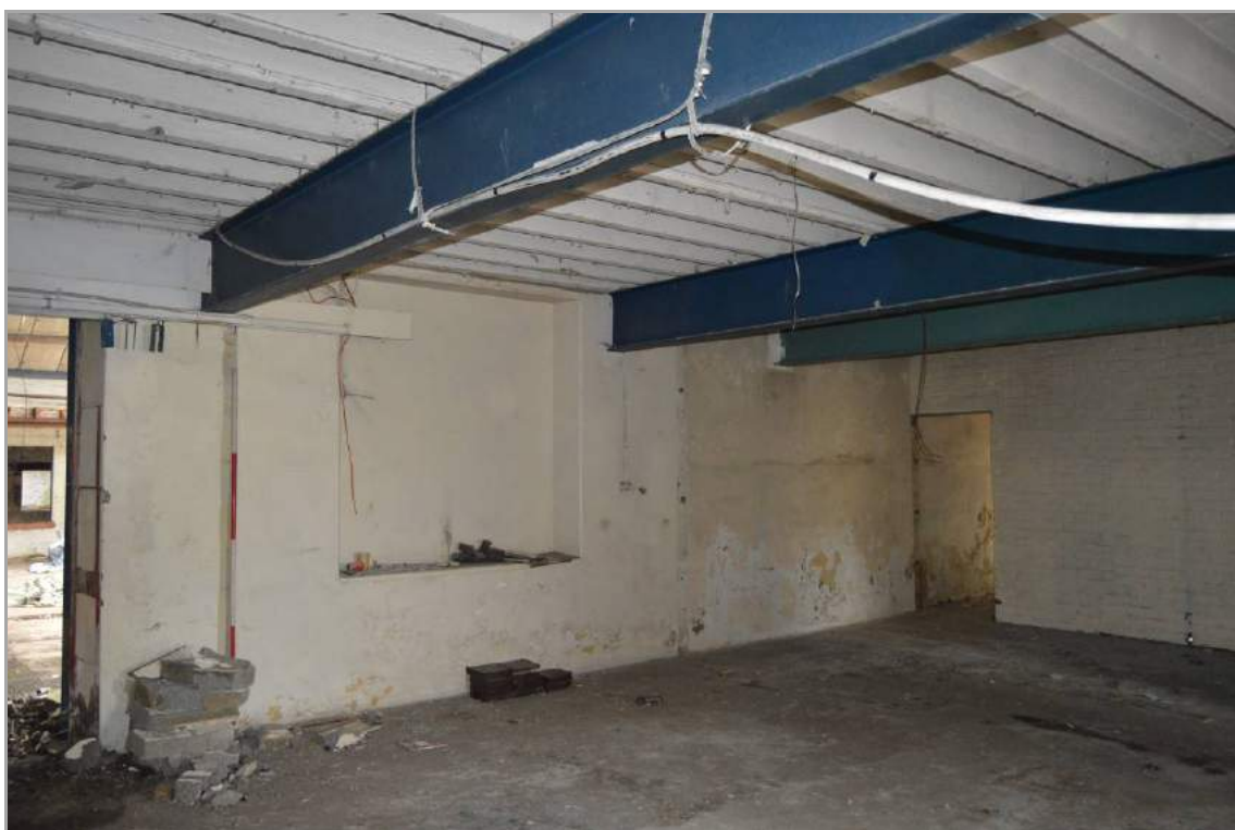
Plate 37: Ground floor space (facing north east). Note the blocked window aperture. Scale 2m.
