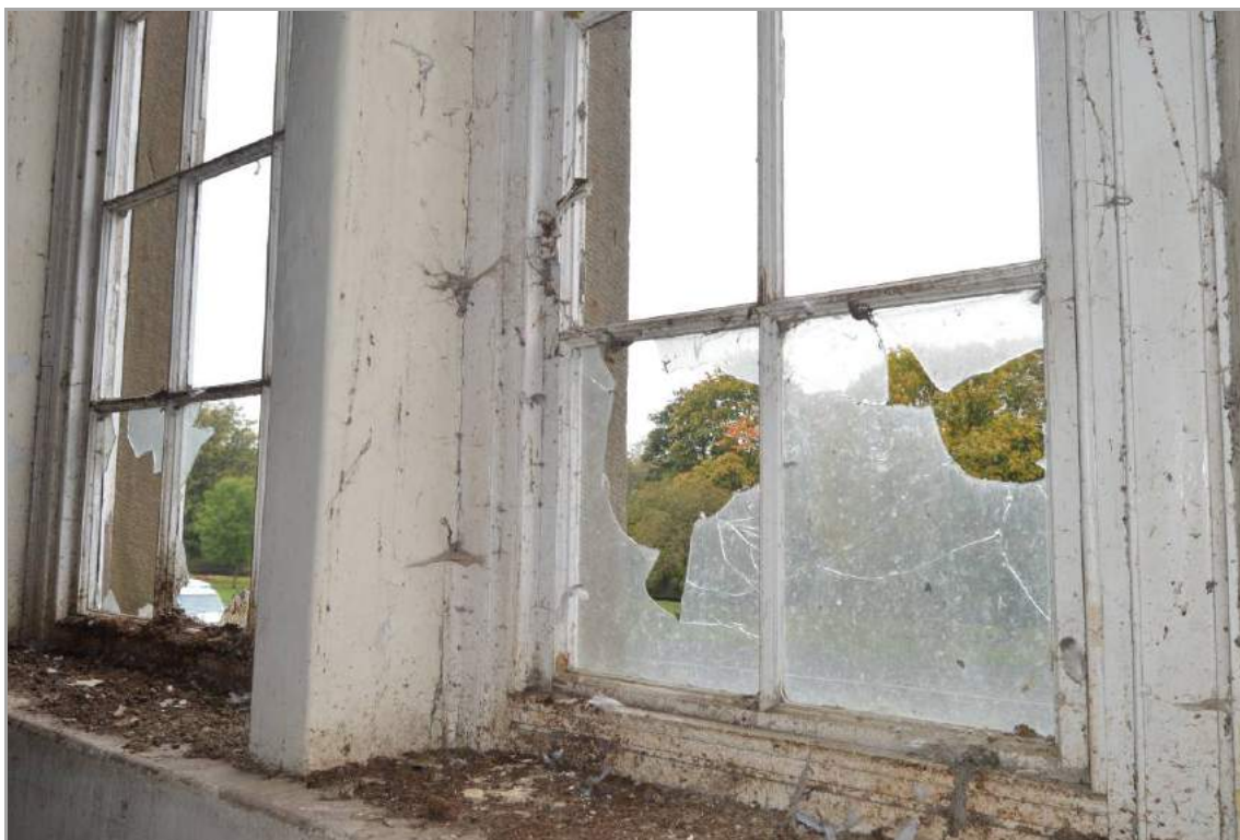
Plate 52: Internal detail of Venetian window to first floor of Building 1 (facing north east). Scale 2m.
