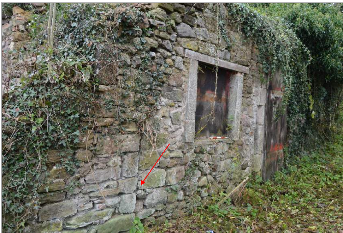
Plate 107: Former mill buildings to south (facing west). Construction break evident between the east and west building indicated.
