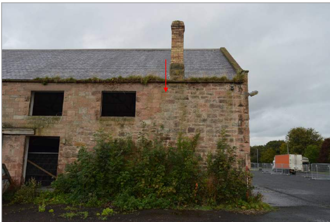
Plate 16: South elevation Building 1 (facing north). Note the difference in the appearance of the stonework. Scale 2m.
