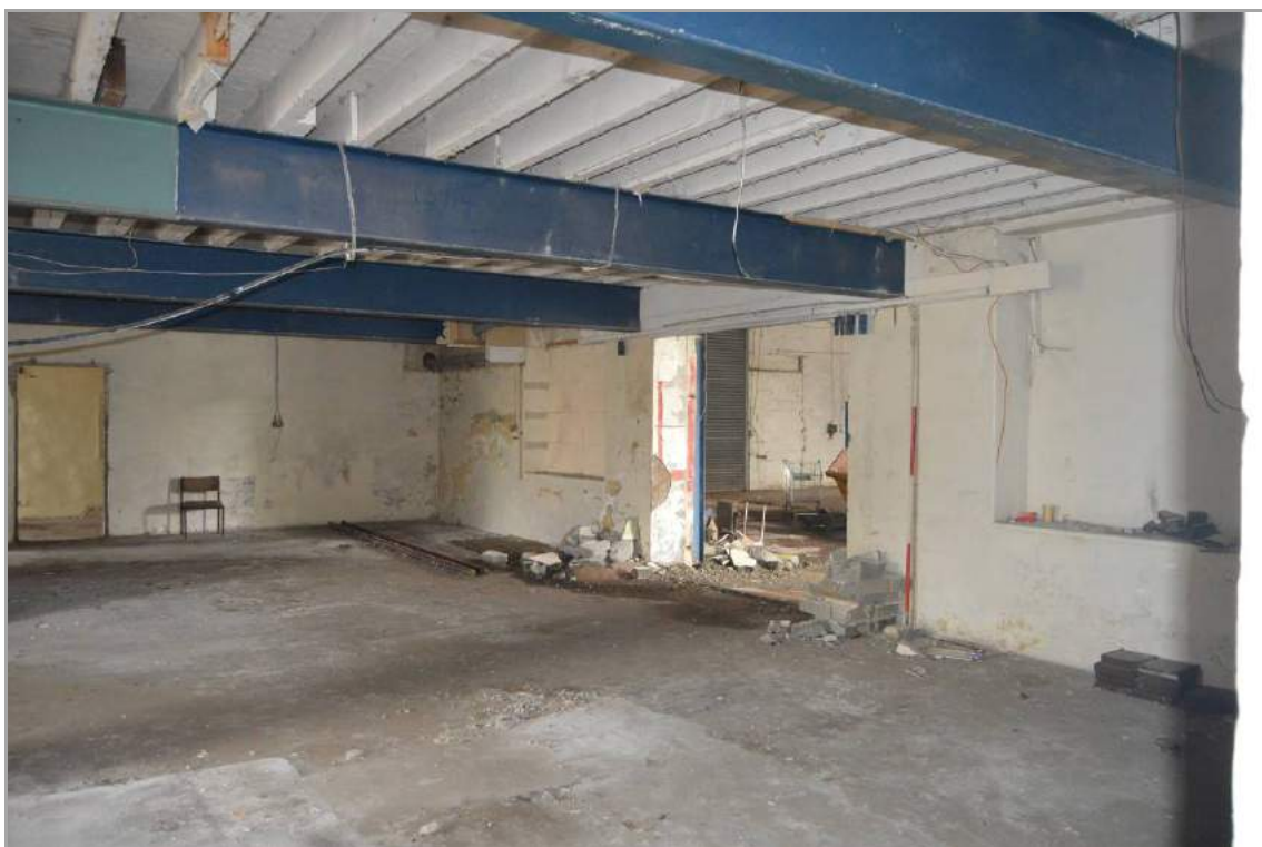
Plate 38: Ground floor space (facing south east) with internal doorway to Building 2. Scale 2m.
