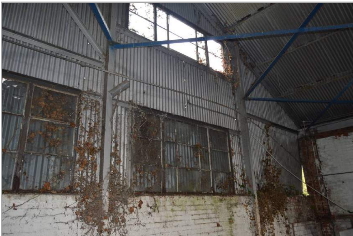
Plate 87: Interior of north elevation of Building 4 showing covered ground floor windows (facing south east).
