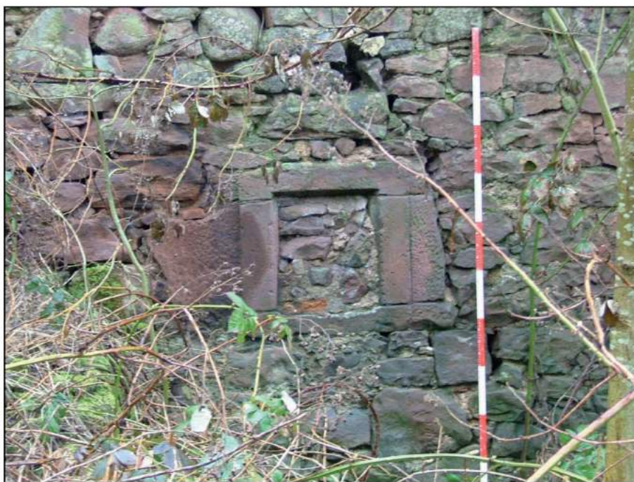
Plate 7: Blocked window in south elevation of Building A (Scale is in 20cm graduations)
