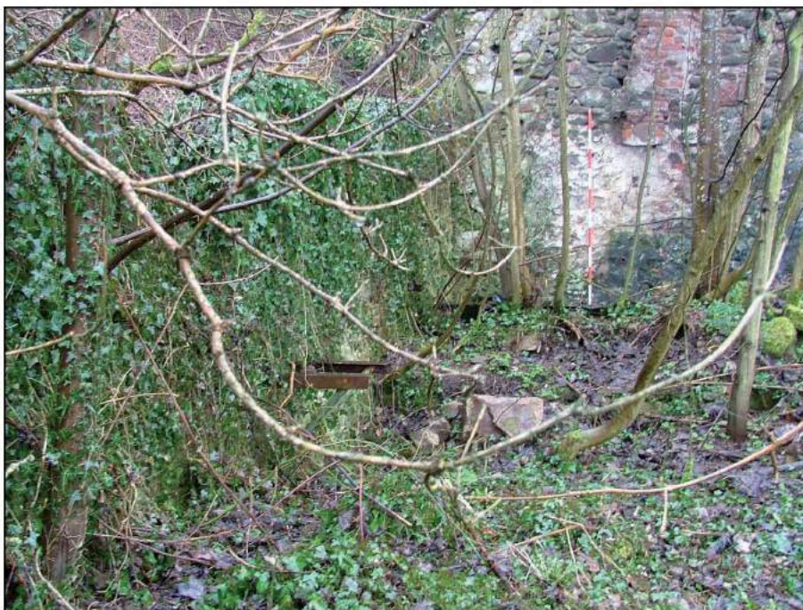
Plate 16: View looking west showing the interior of the east room of Building B with metalwork fixed into the south wall (Scale = 2m)
