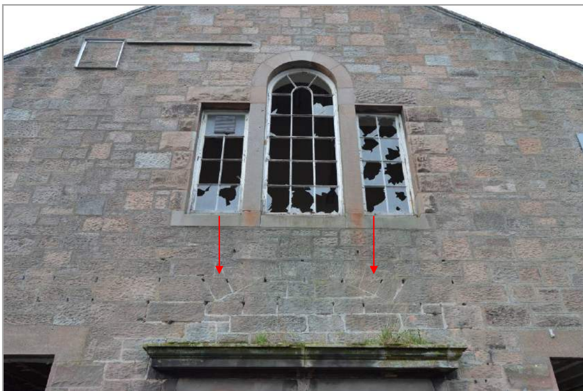
Plate 13: First floor window in east elevation (facing west). Note the stone voussoirs of a relieving arch.
