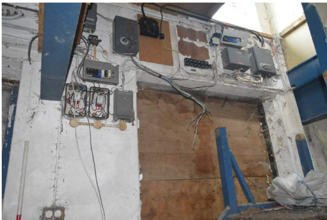
Plate 45: Electrical fittings adjacent dog-leg staircase to first floor of Building 1 (facing south). Scale 2m.
