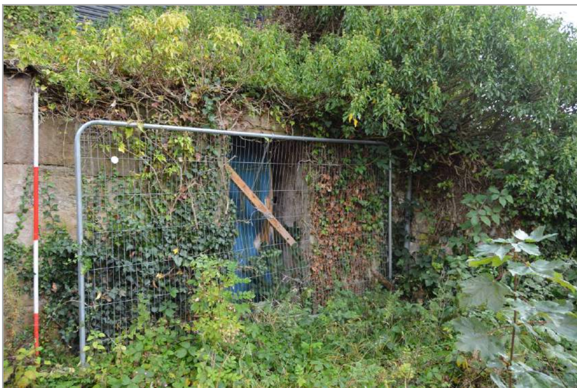
Plate 27: Extension structure in front of west elevation (facing south east). Scale 2m.
