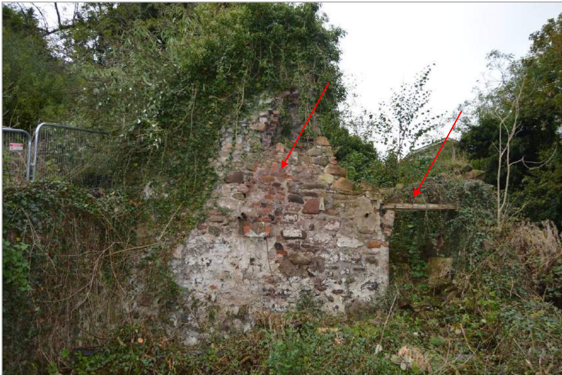
Plate 111: Interior of former Mill Building B (facing west). Note, the internal dividing wall with door and fire brick for chimney flue.
