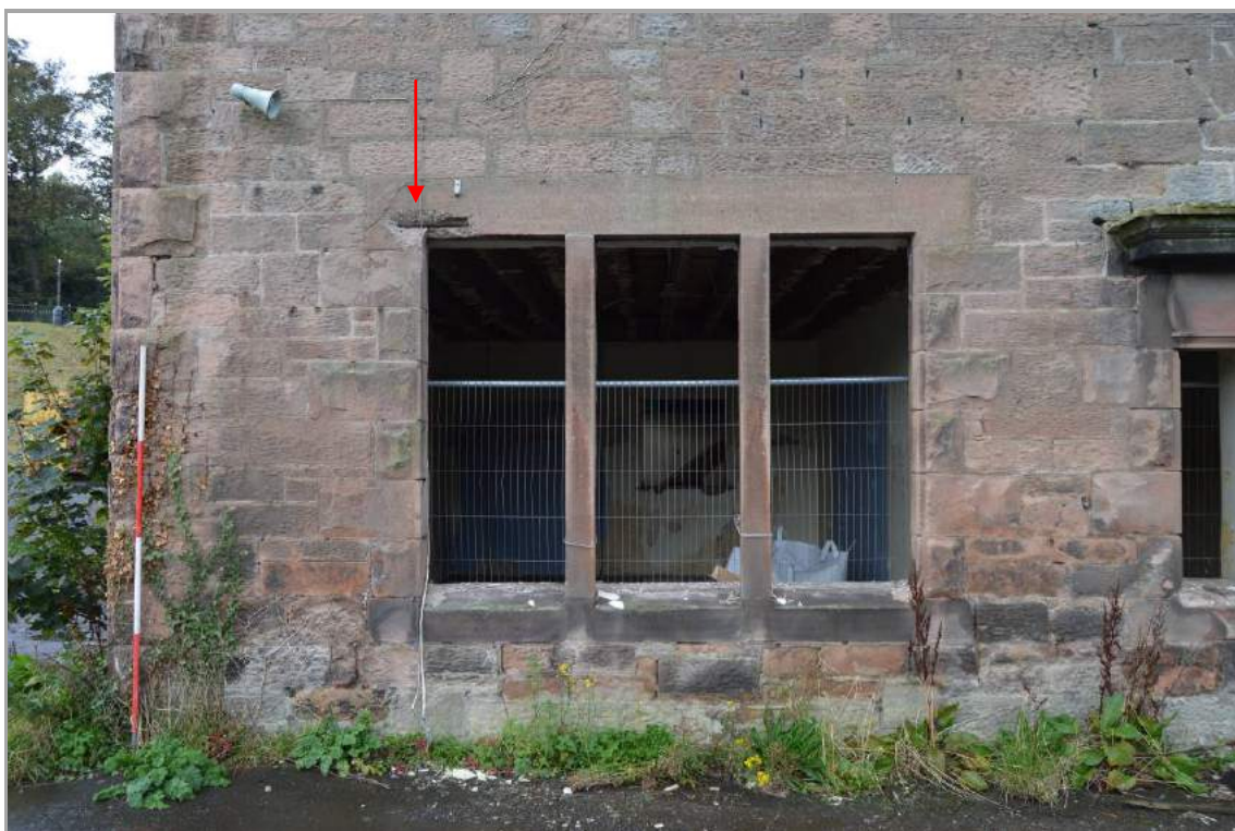
Plate 10: South window in east elevation (facing west). Note the reinforced concrete lintel. Scale 2m.
