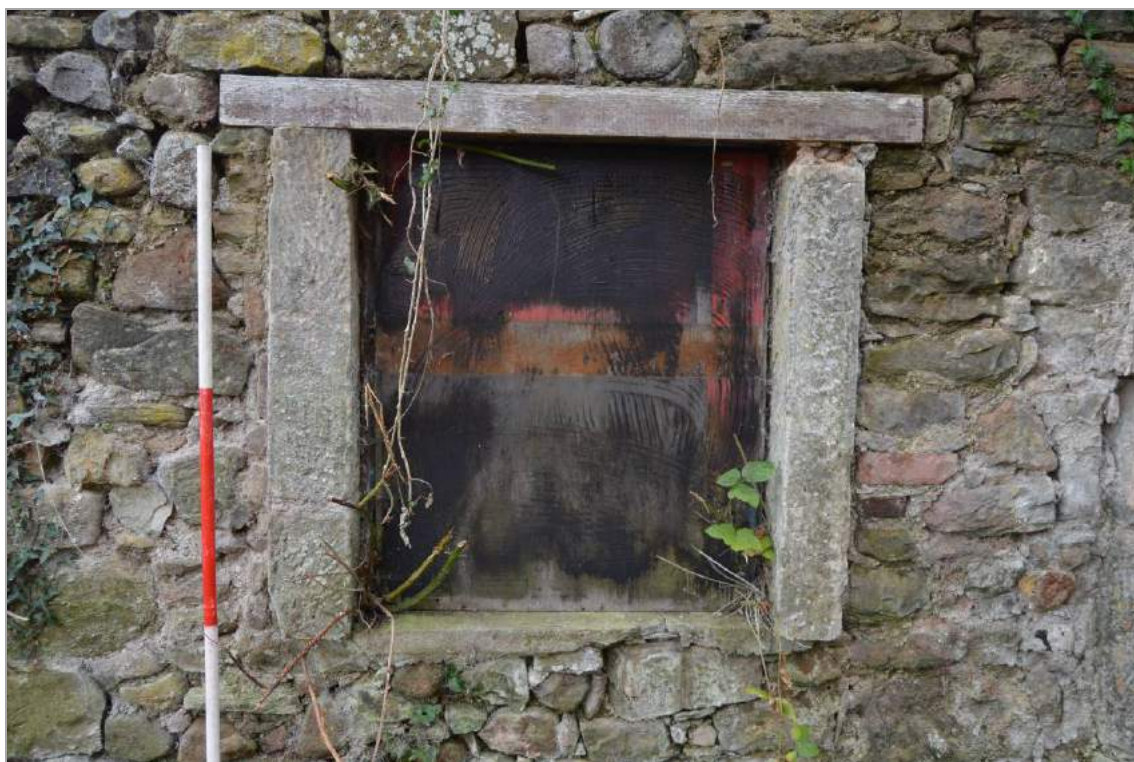
Plate 109: Former mill buildings to south, detail of north aspect window (facing south). Scale 2m.
