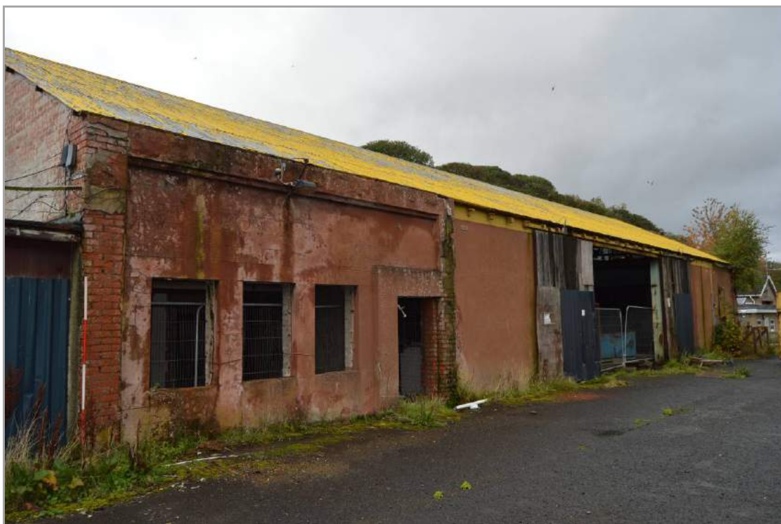
Plate 79: East elevation of Building 4, the largest building on the site (facing north west). Scale 2m.
