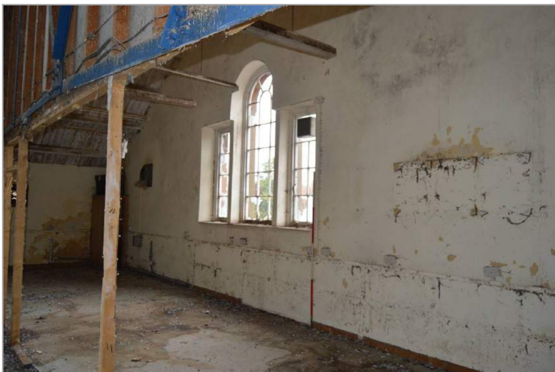
Plate 51: View of east window to first floor of Building 1 (facing north east). Scale 2m.
