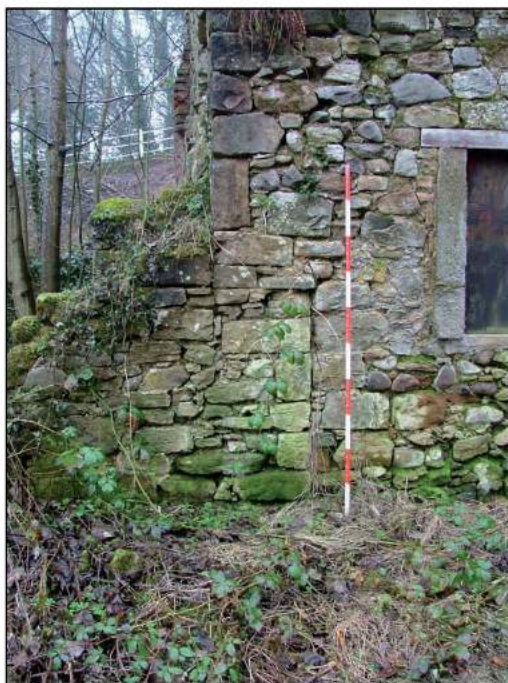
Plate 13: Vertical line of former quoins in the north elevation of Building B (Scale = 2m)
