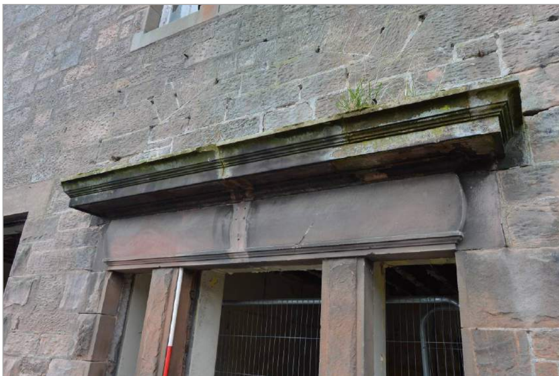
Plate 9: Oblique view of canopy over doorway in east elevation (facing north west). Scale 2m.
