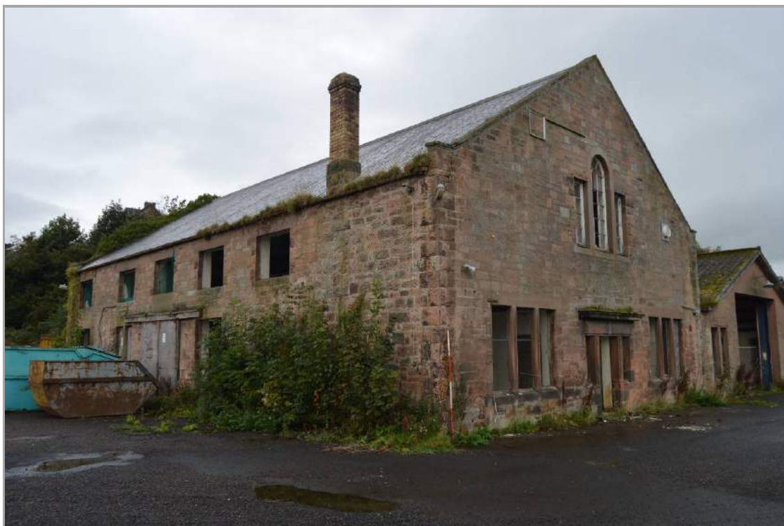
Plate 6: Oblique view of east and south elevations (facing south west). Scale 2m.
