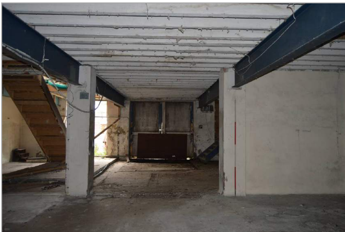
Plate 40: Ground floor space (facing south), looking towards the south goods entrance. Scale 2m.
