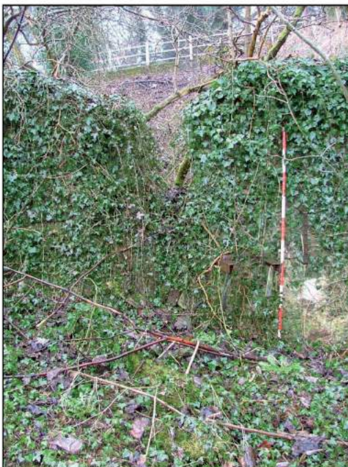
Plate 18: Hole in the south elevation of Building B for possible former water wheel axle (Scale = 2m)
