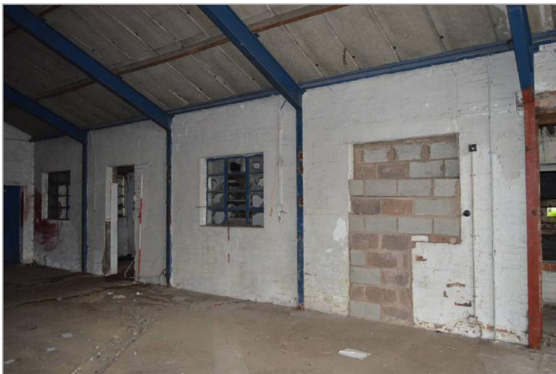
Plate 67: Former exterior wall of Building 2 (facing north west). Note the blocked door. Scale 2m.
