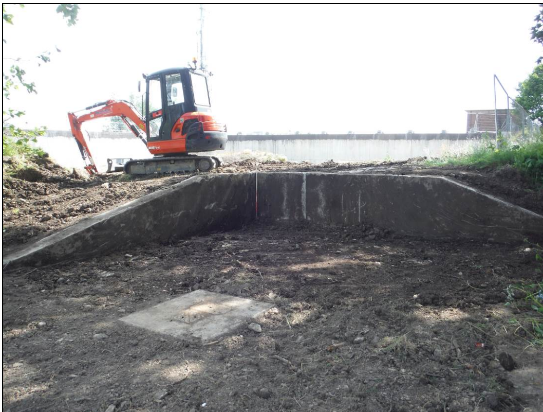
Figure 11. View looking west of concrete structure (505) (Scale = 1 x 1m in 0.5m graduations).
