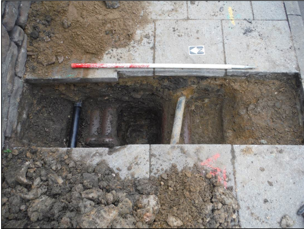
Figure 5. West facing section through Test Pit 2 (Scale = 1 x 1m in 0.5m graduations).
