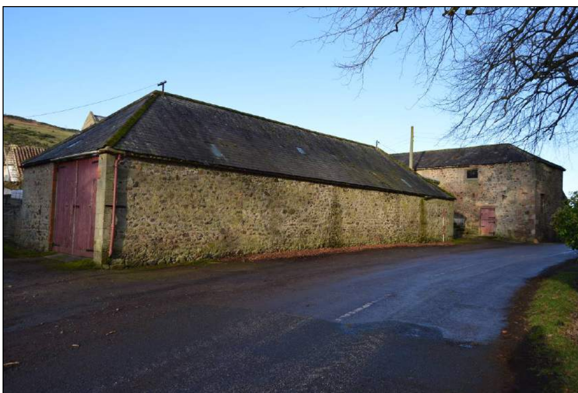
Plate 82: East elevation of the east farm range (facing south east). Scale 2m.
