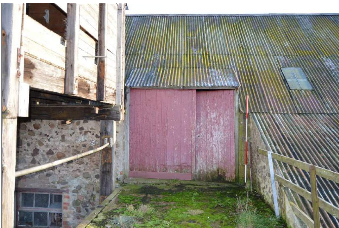
Plate 38: First floor barn entrance to the west elevation of the barn (facing east). Scale 2m.
