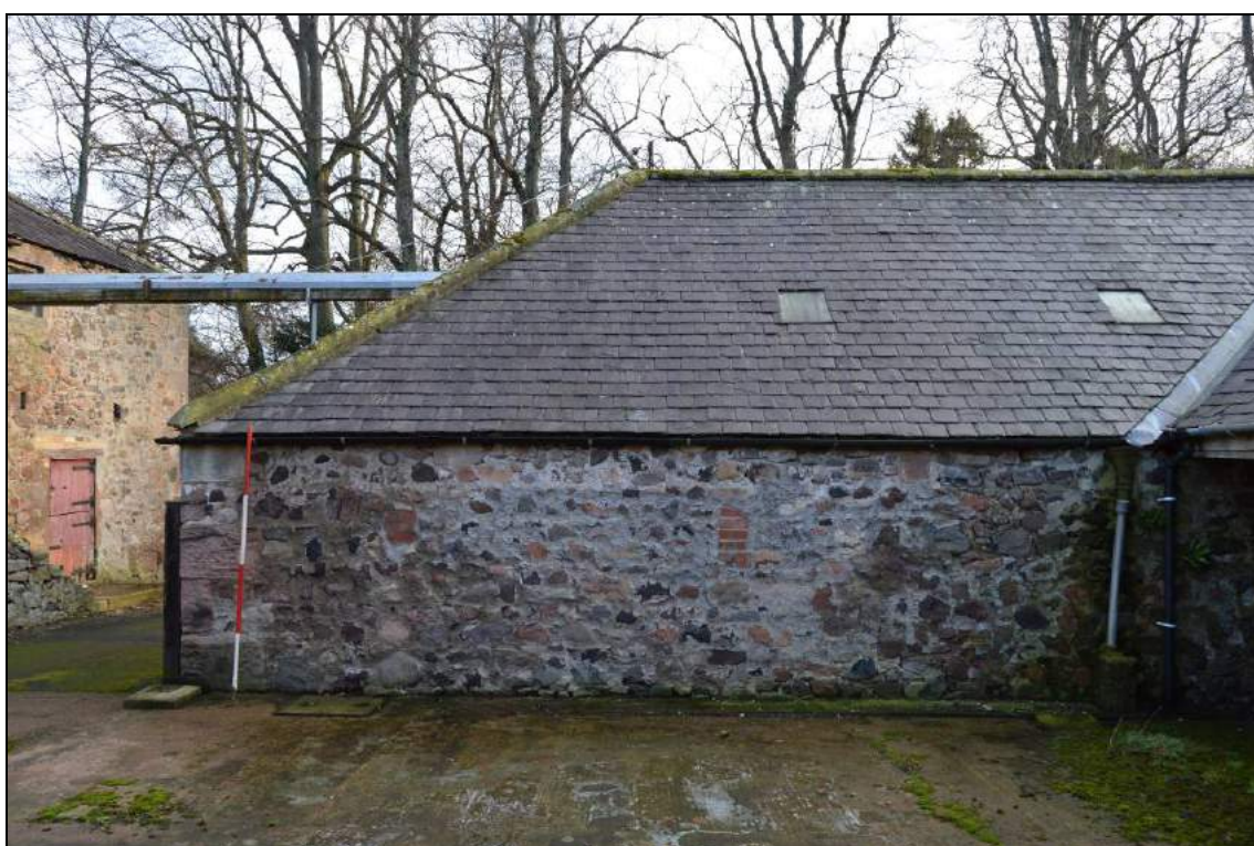
Plate 84: West elevation (facing south east) with small blocked openings indicated. Scale 2m.
