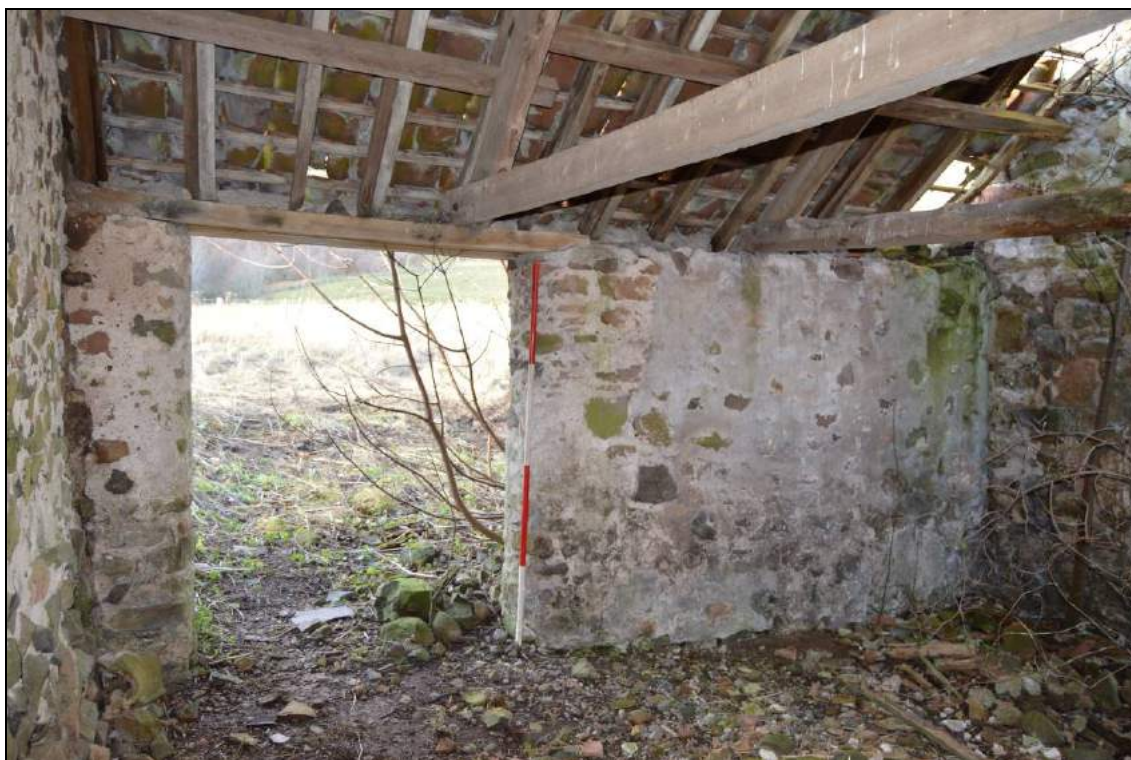
Plate 62: Interior of Hemmel building (facing west) with cattle door to west paddock. Scale 2m.
