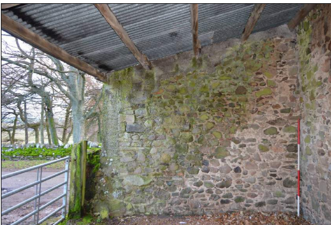
Plate 102: East elevation, of stone construction, of the shelter shed (facing east). Note. Scale 2m.
