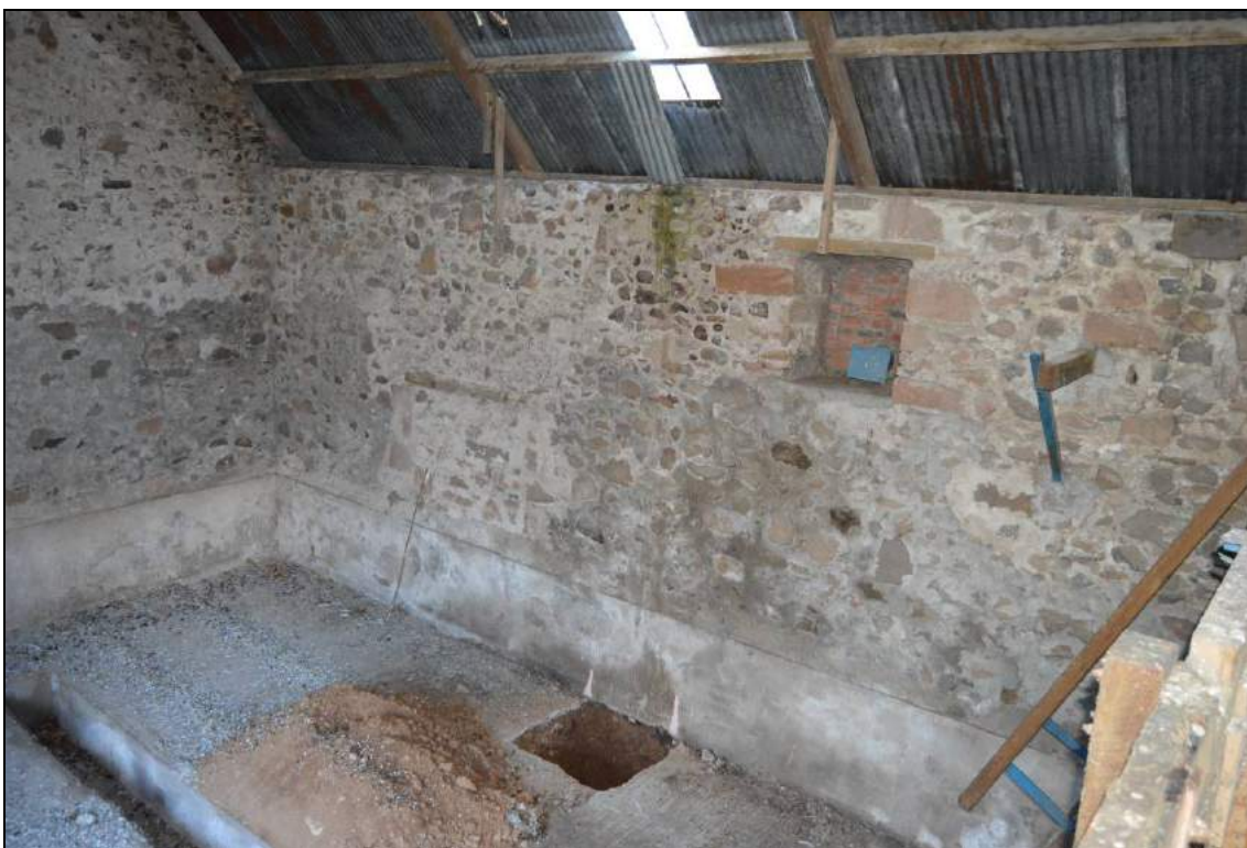
Plate 44: View of the open area to the interior of the barn (facing south west). Scale 2m.
