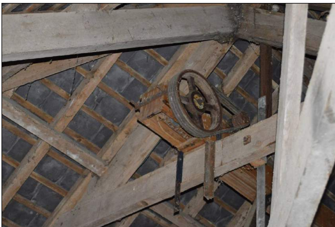
Plate 89: Grain conveyer mechanism in roof space of building (facing north west).
