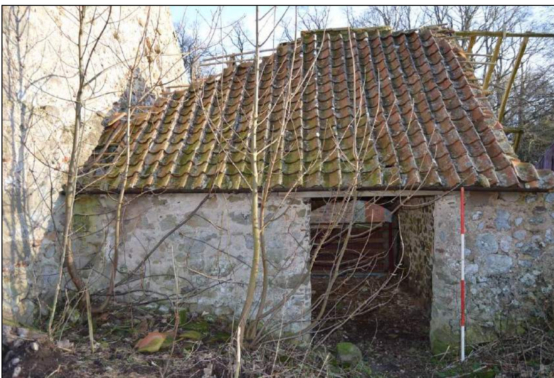
Plate 58: West elevation of hemmel building with cattle entrance (facing east). Scale 2m.
