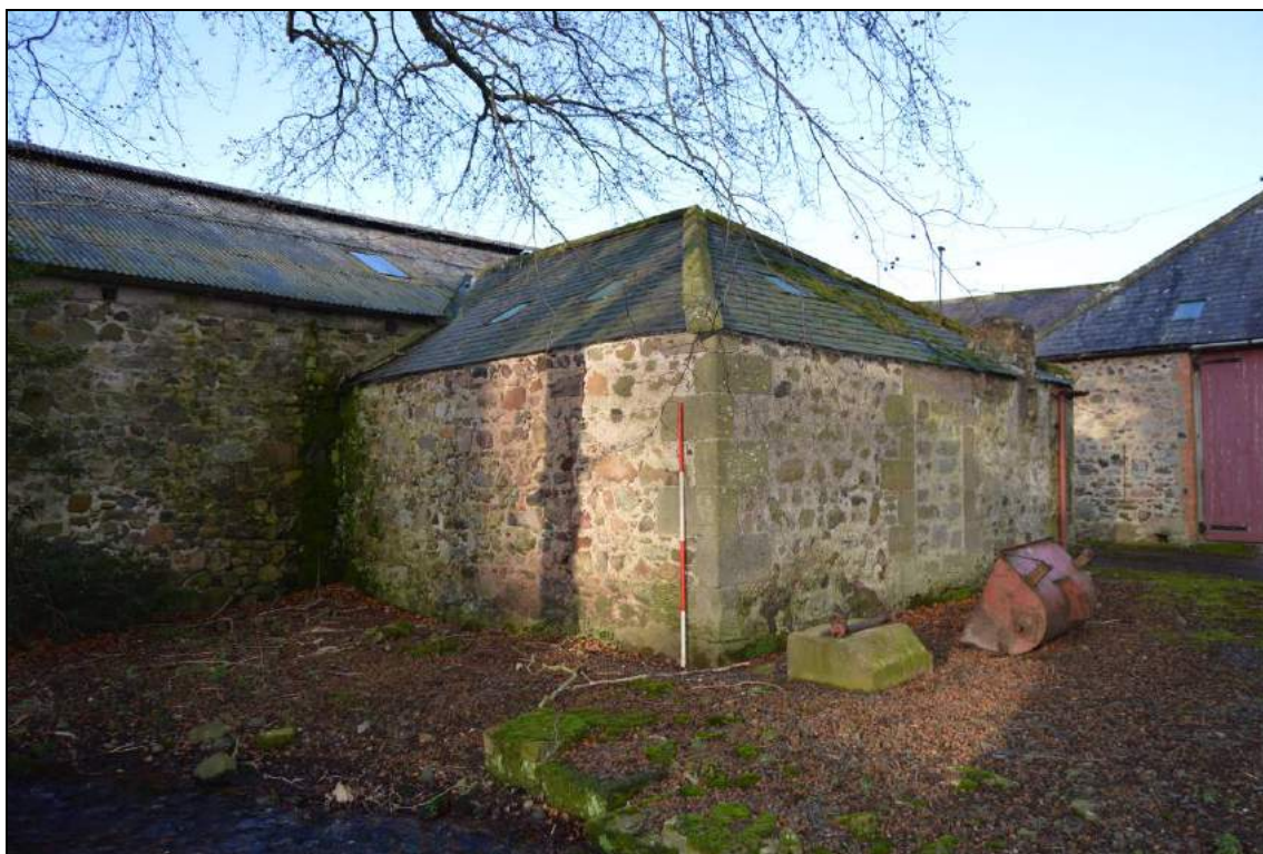
Plate 68: Projecting pavilion wing of south animal shed (facing north west). Scale 2m.
