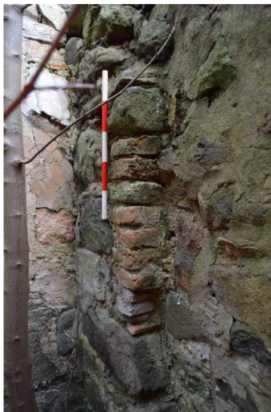
Plate 61: Interior of Hemmel building (facing north east) with red brick building material. Scale 0.5m.
