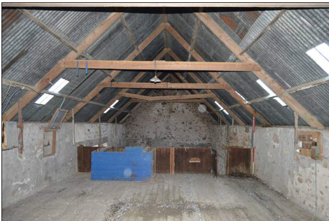
Plate 52: General view of the first floor of the barn (facing north). Scale 2m.
