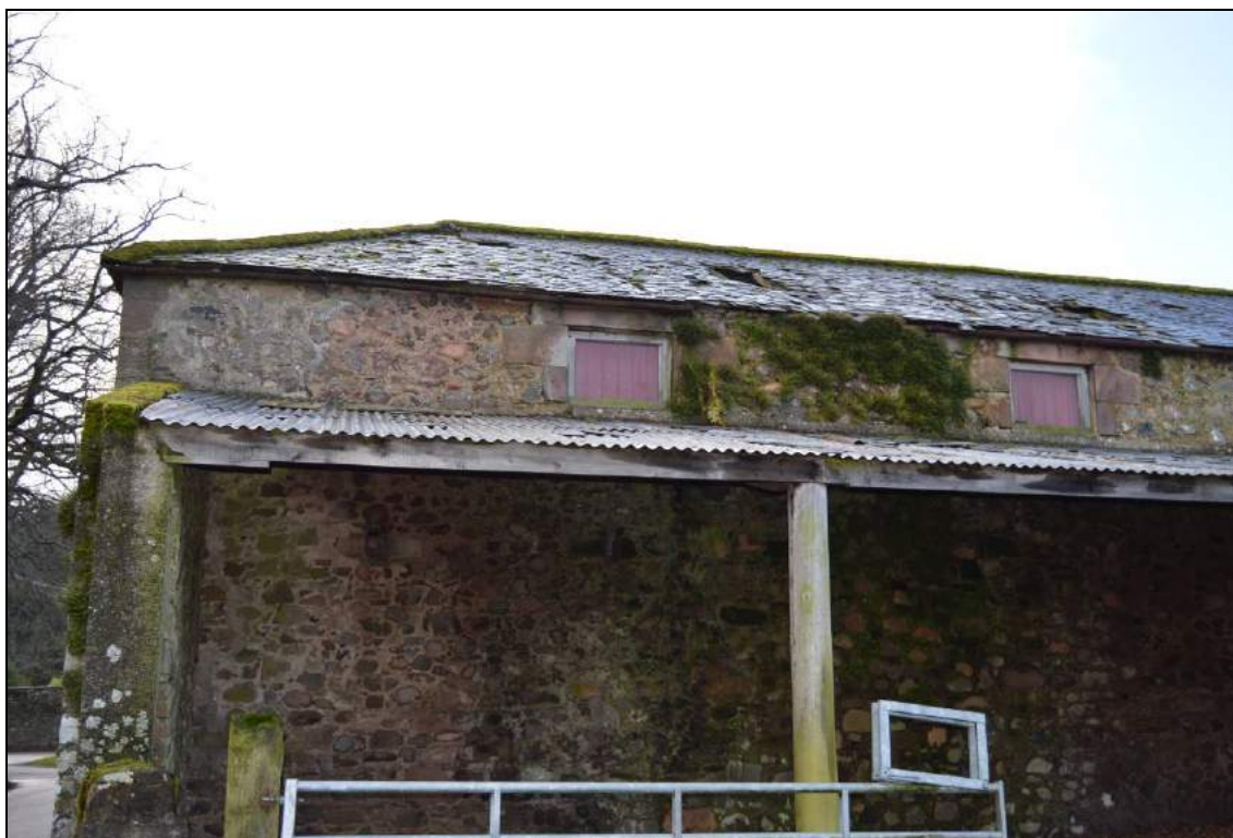
Plate 15: Eastern extent of the north elevation to the granary range (facing south). Scale 2m.
