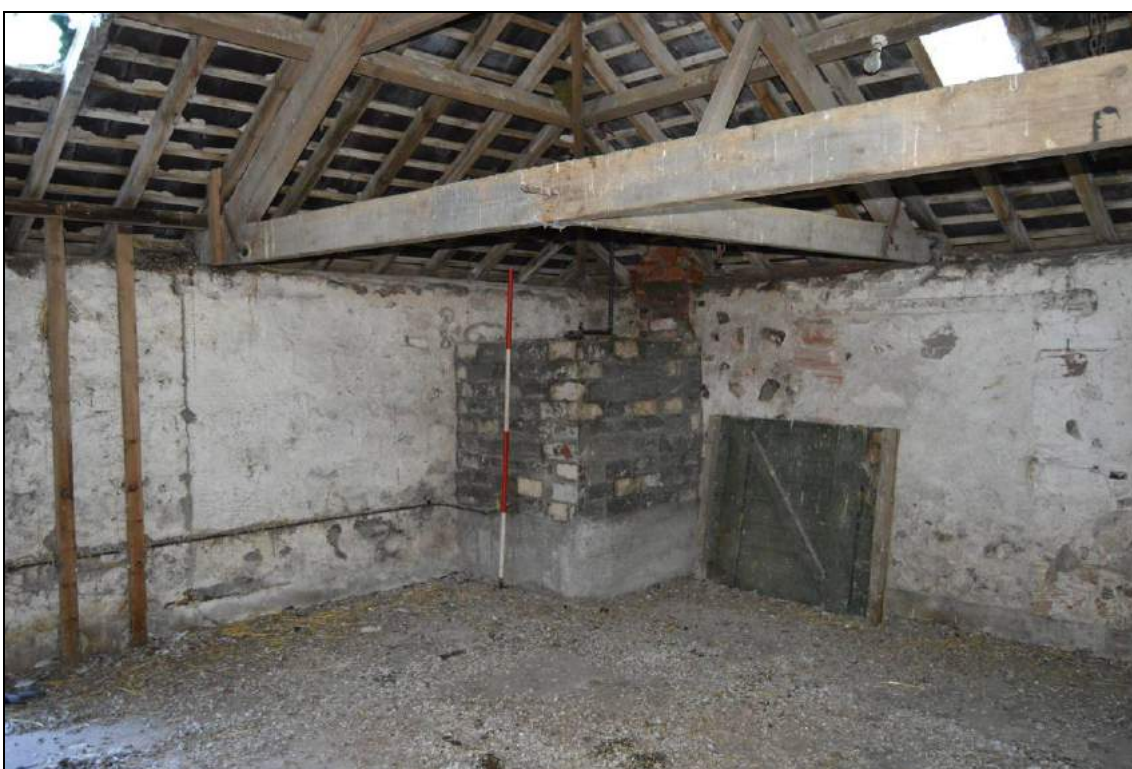
Plate 79: Interior of the project wing of the south animal accommodation (facing north east). Scale 2m.
