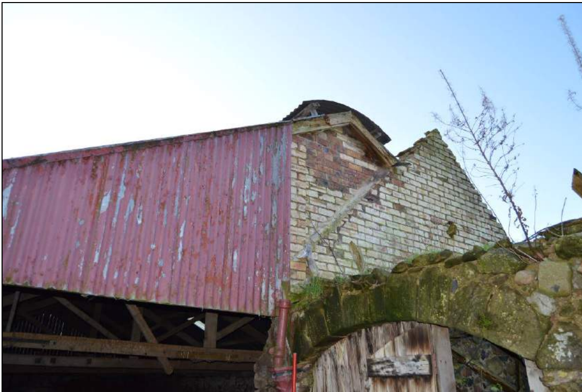
Plate 65: Detail of east gable to north elevation (facing south west). Note, the brick walling forms an internalised wall for the south elevation of the hemmel. Scale 2m.
