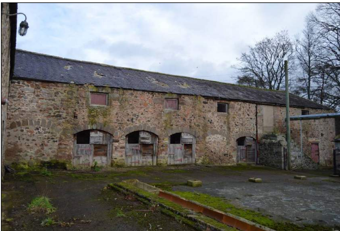
Plate 7: South elevation of the granary/cow-house from within the north foldyard. Scale 2m.
