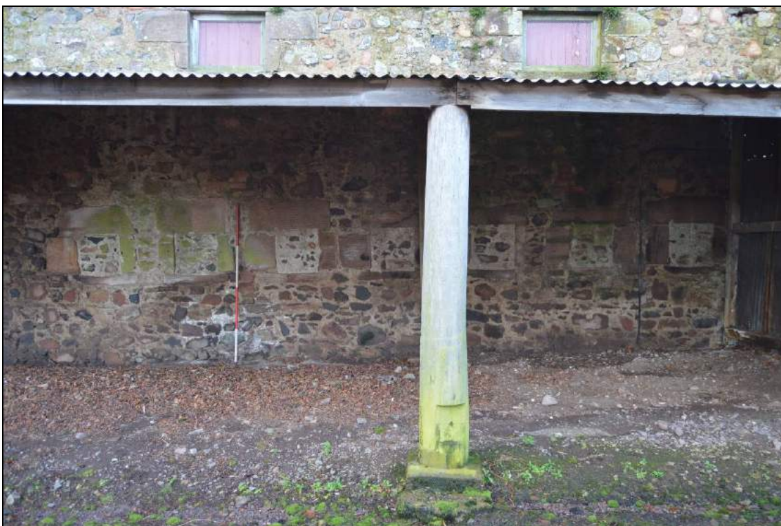
Plate 16: Seven of the cow-house apertures to the north elevation of the granary range. Scale 2m.
