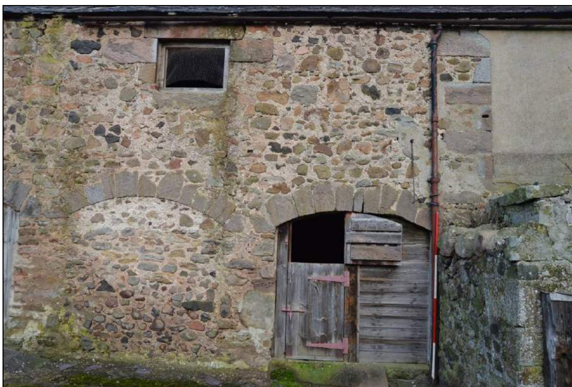
Plate 9: South elevation of the granary/cow-house with two of the former cattle entrances (facing north). Scale 2m.
