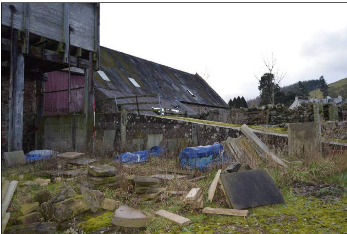
Plate 39: View towards the west facing elements of the barn (facing west) with its concrete ramp to foreground. Scale 2m.
