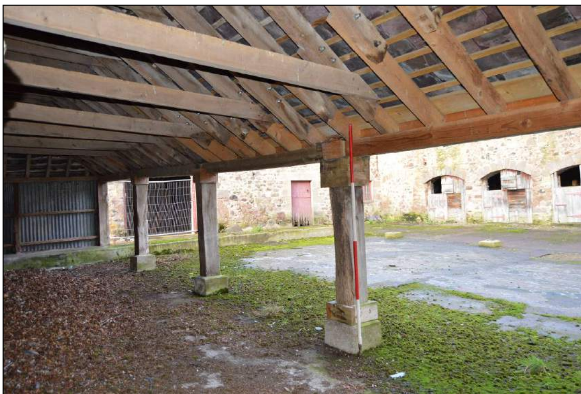
Plate 92: Interior of north shelter shed with supporting columns to front (facing north west). Scale 2m.
