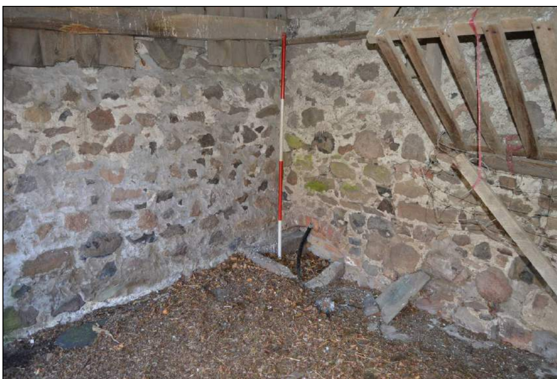
Plate 94: Interior of north shelter shed with drain (facing south east). Scale 2m.
