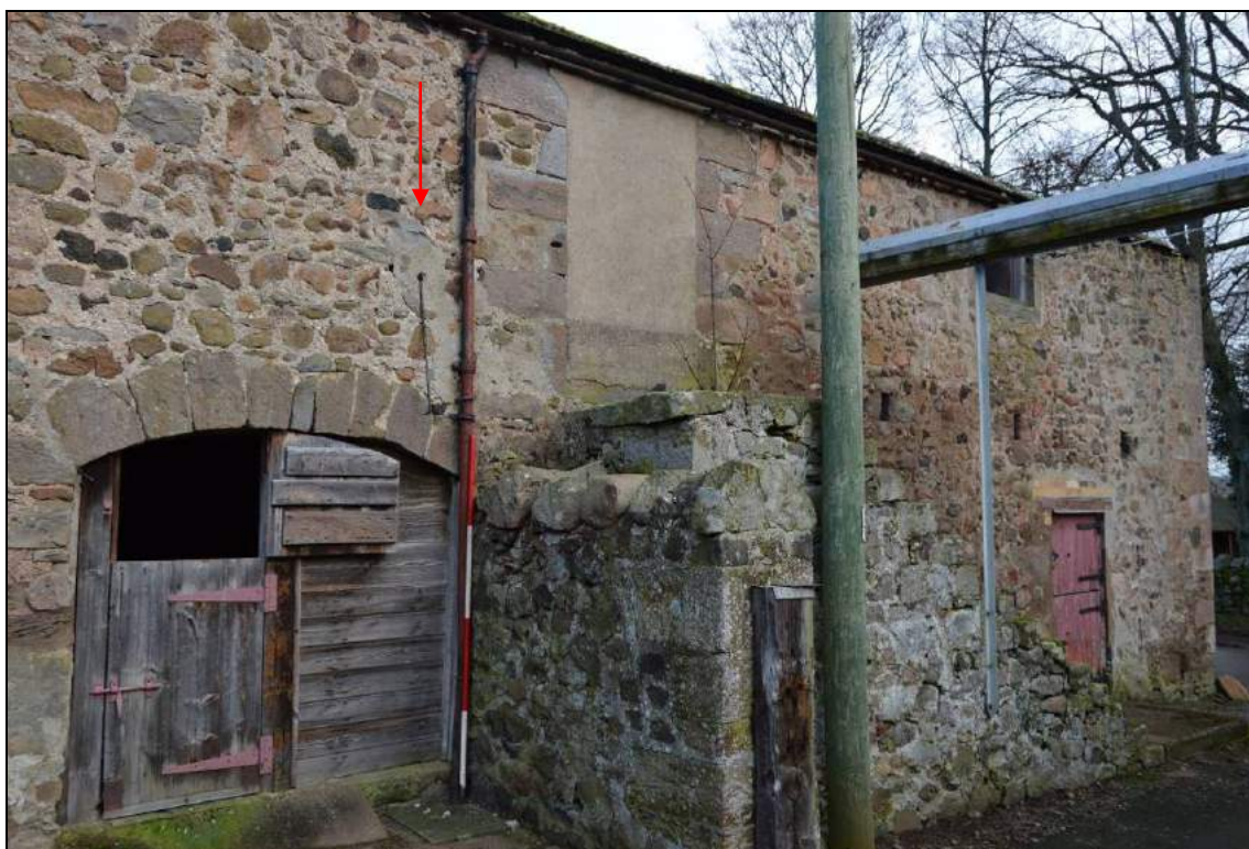
Plate 10: South elevation (facing north east) towards the east section of the granary/cow-house. Note the cement rendered blocked doorway to the first floor. Scale 2m.
