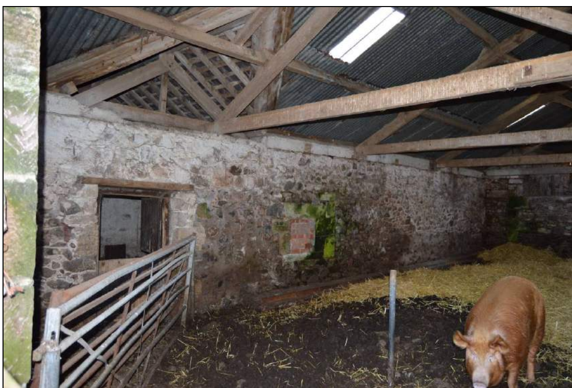
Plate 77: Interior of the southern animal accommodation range with connecting door to eastern structure (facing south east).
