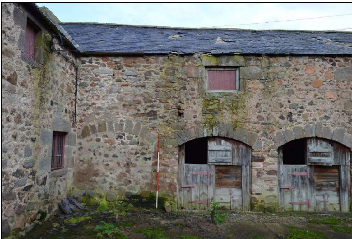
Plate 8: South elevation of the granary/cow-house with three of the former cattle entrances (facing north). Scale 2m.
