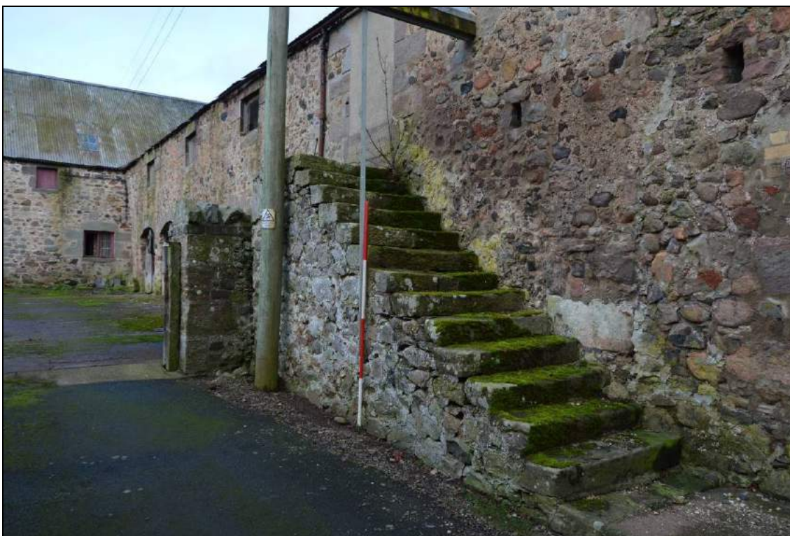
Plate 11: South elevation (facing north west) towards the granary/cow-house external steps. Scale 2m.
