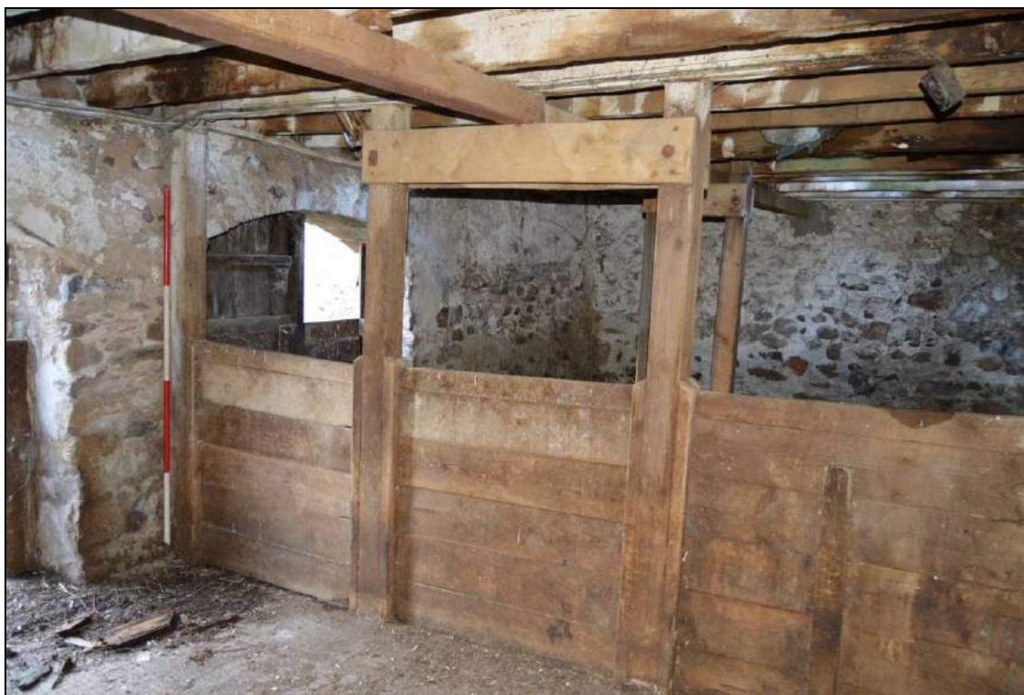
Plate 21: Animal stalls to west (facing west), with the blocked door contributing to a larger space. Scale 2m.
