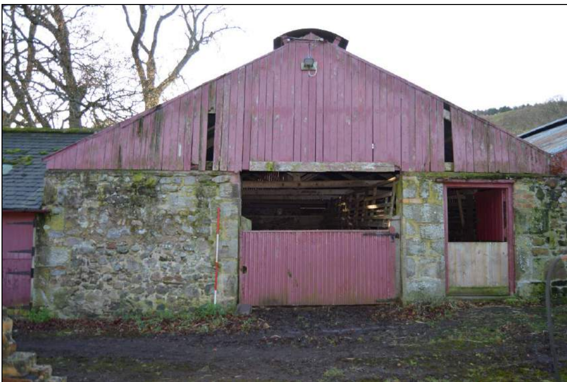
Plate 66: North elevation of south animal shed, east gable (facing south). Scale 2m.
