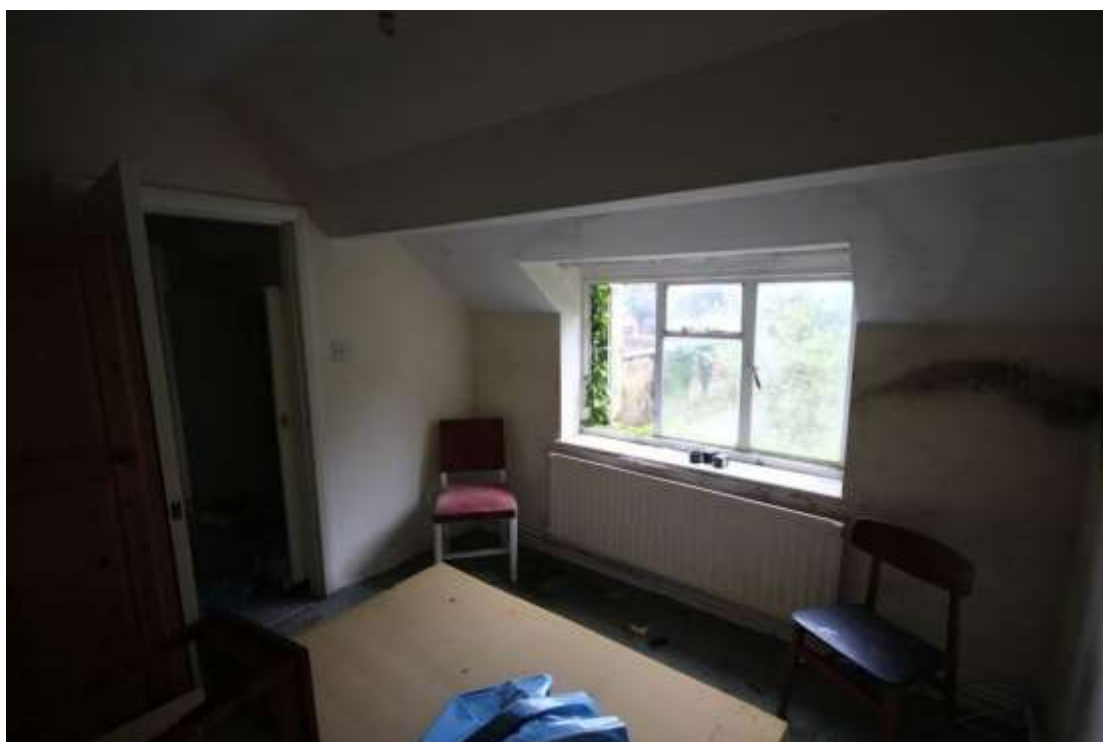
Plate 132: View of the first floor southern bedroom, facing north east. The original roof timbers have been covered here by plasterboard, visible above the window.
