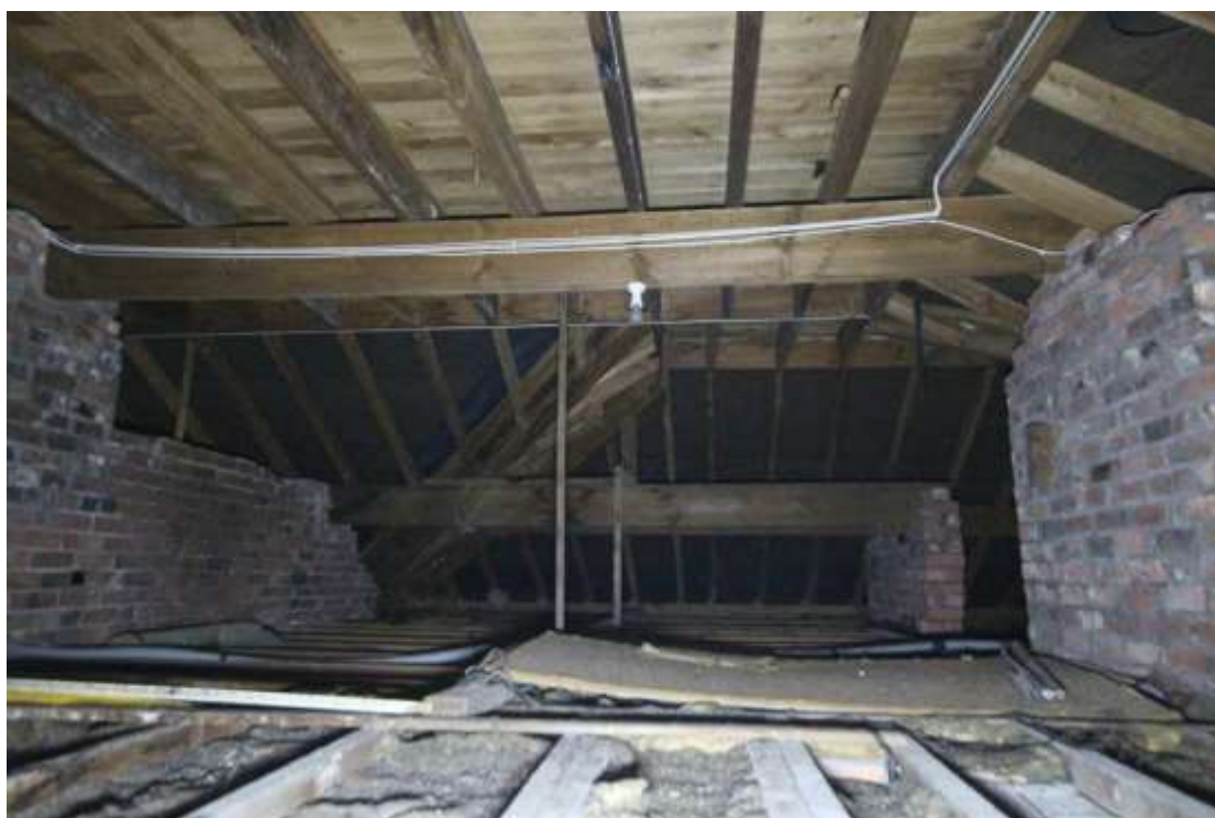
Plate 93: View of the unconverted attic space above the western part of Block A, facing west. These brick walls carrying the roof timbers are part of the original construction of the hall in the early 19th century.
