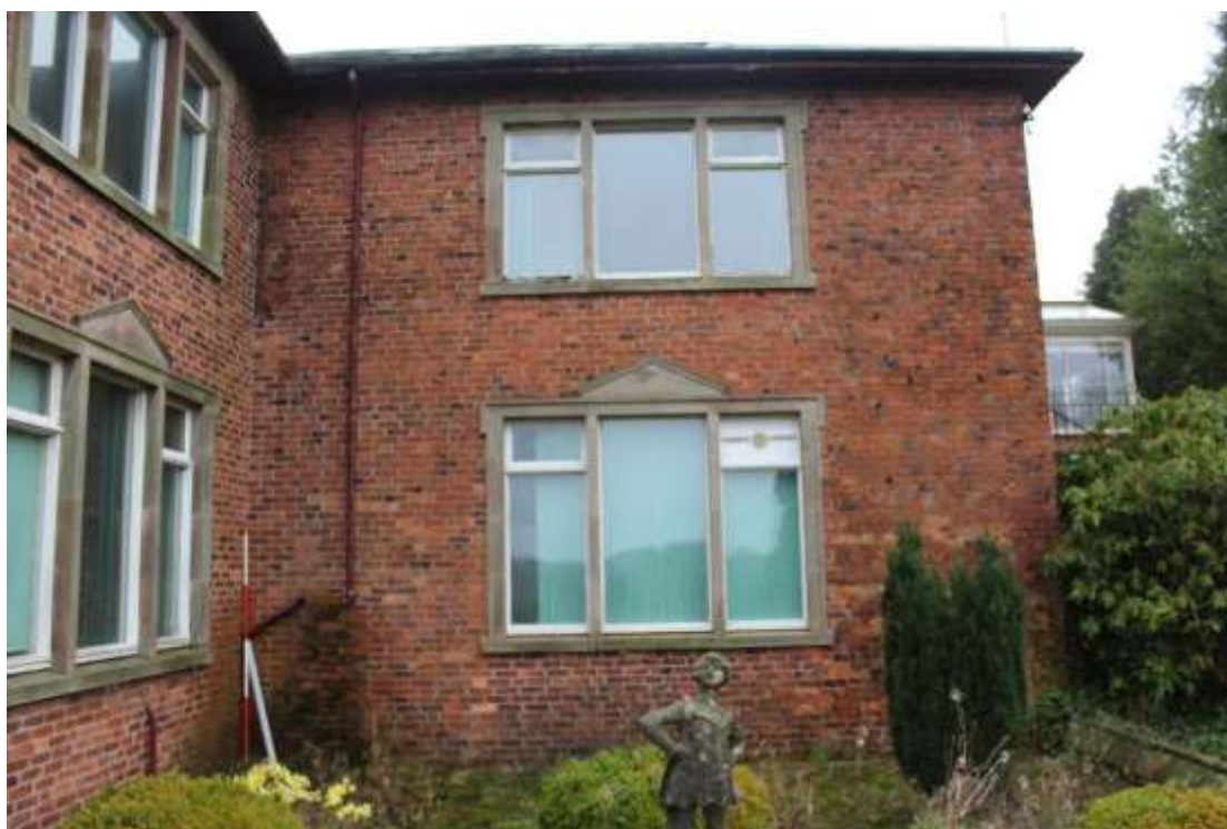
Plate 1: View of the eastern bay of the southern elevation of Block A, facing north. Scale 2m.
