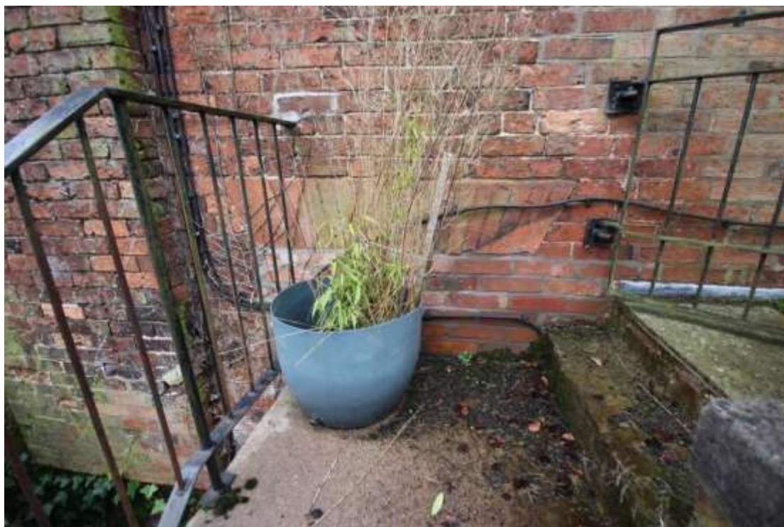
Plate 12: Detailed view of the now blocked ground floor window visible at the top of the stairs, facing west.
