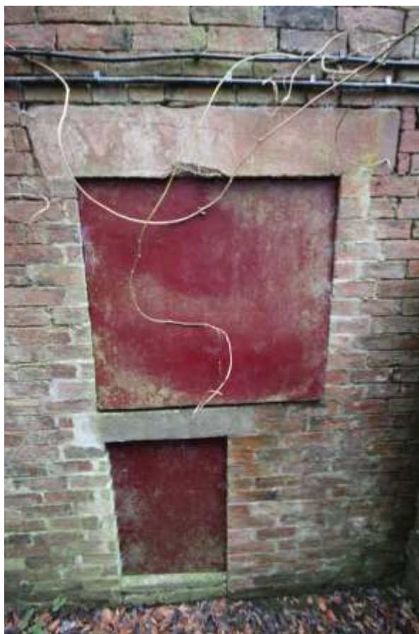
Plate 14: Detailed view of the openings in the eastern extension to Block A, facing west.
