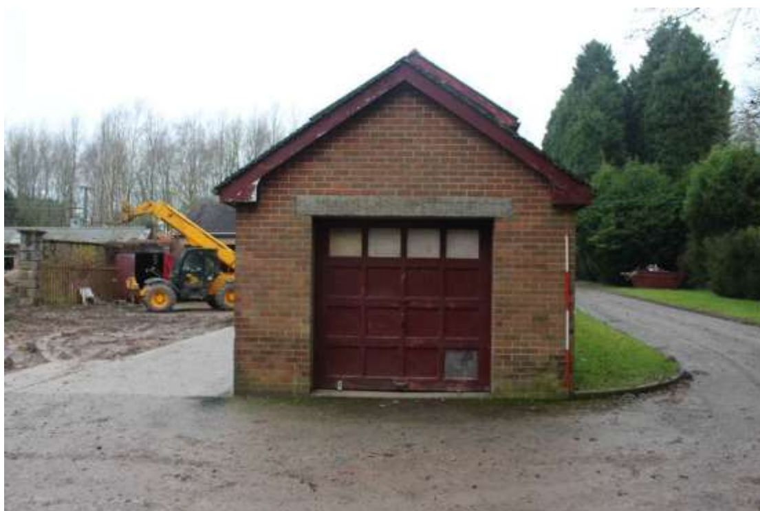
Plate 115: View of the southern gable end of the eastern block of the Gardener's Workshop, facing north.
