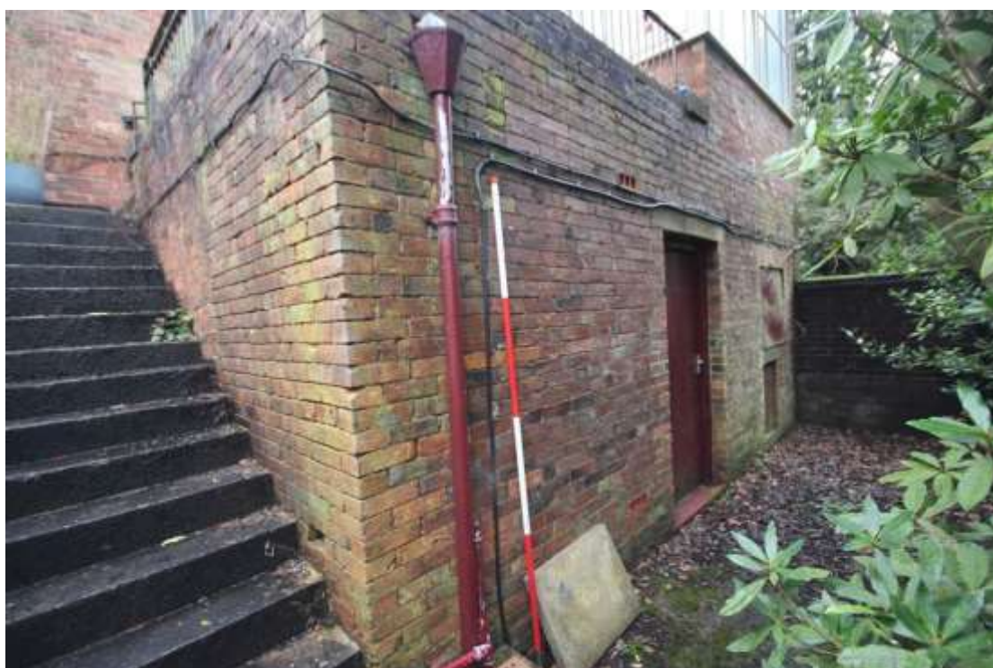
Plate 11: View of the southern side of the eastern extension added to Block A, facing north west. Scale 2m.
