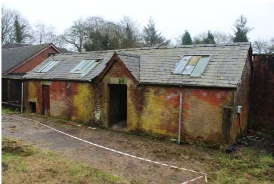
Plate 103: View of the northern elevation of the Potting Shed, facing south. Scale 2m.
