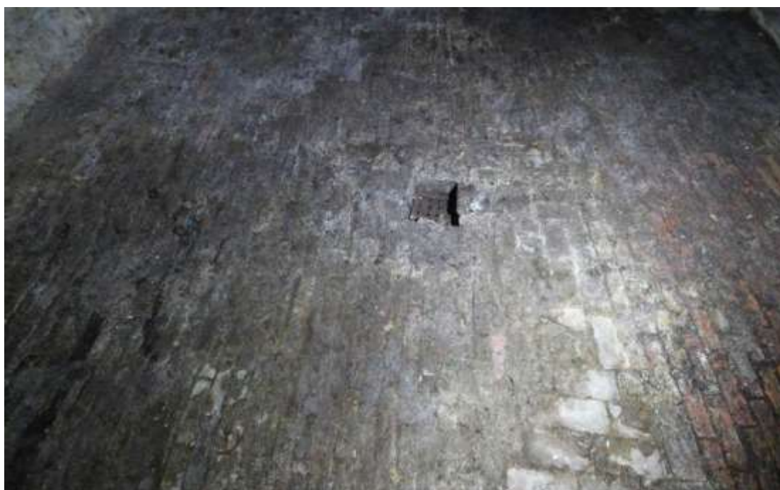
Plate 77: View of the central grate in the floor of the northern Store room, facing north.
