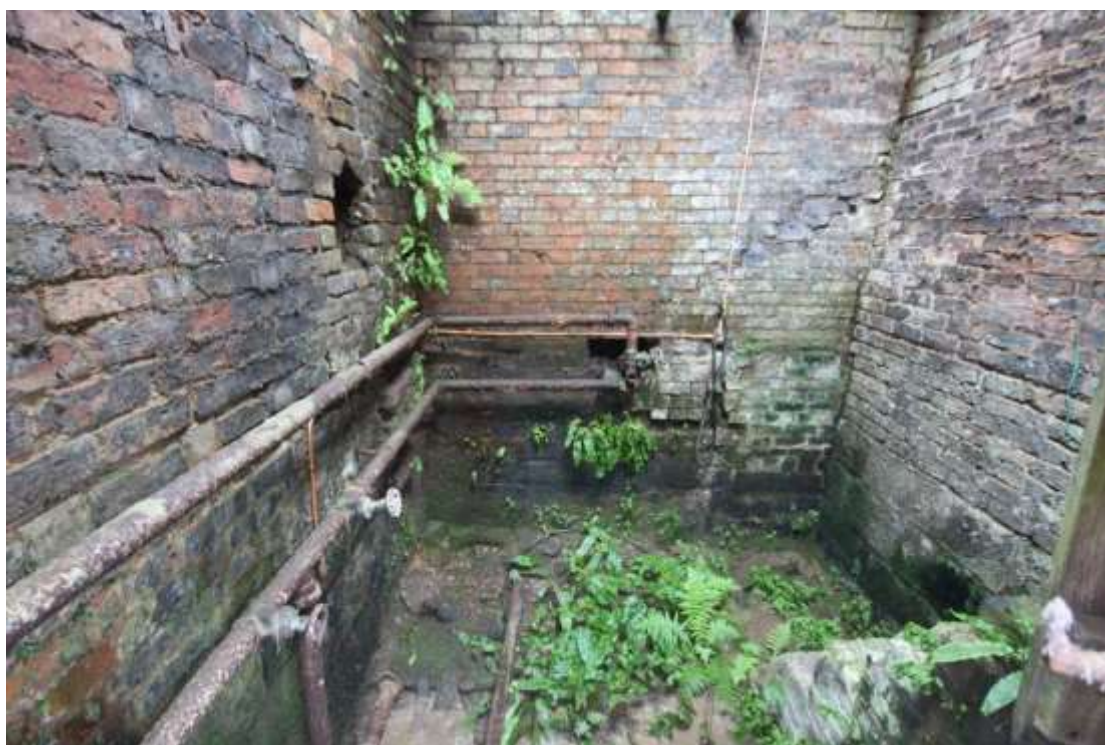
Plate 111: General view of the lower part of the southern interior wall of the eastern 'boiler room' adjacent to the Potting Shed, facing south.
