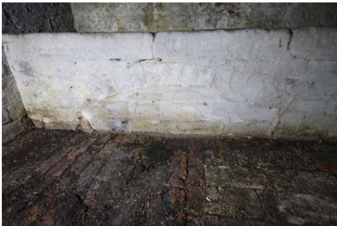
Plate 87: Detailed view of one of the relieving arches underneath the bench in the southern Store room, facing south.
