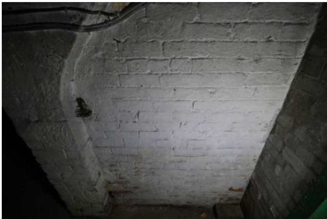
Plate 70: Detailed view of the blocked opening next to the entrance to the store, facing south.
