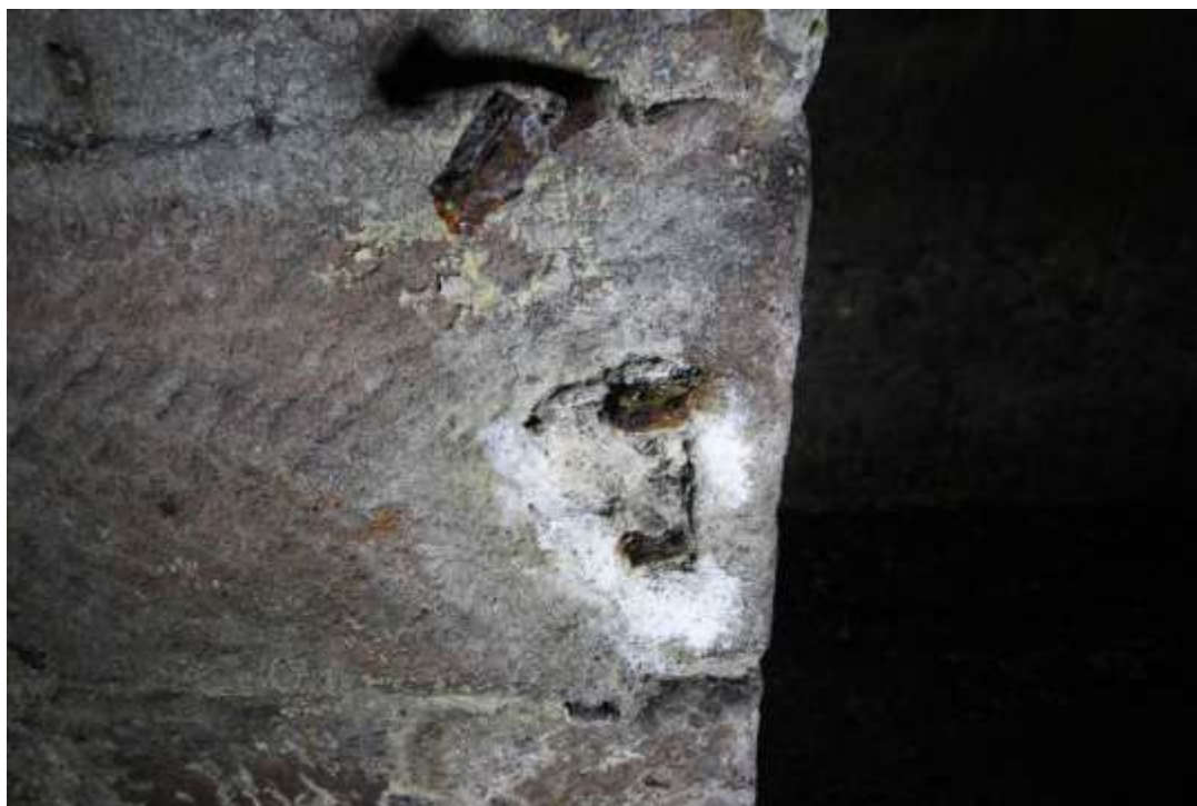
Plate 75: Detailed view of the latch fastener visible in the northern elevation of the north Store, facing north.
