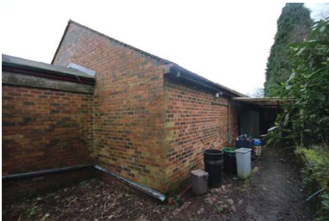
Plate 94: General view of the southern elevation of the south western extent of the Halcyon Room, facing north east. This is part of the late 1960s/early 1970s construction.
