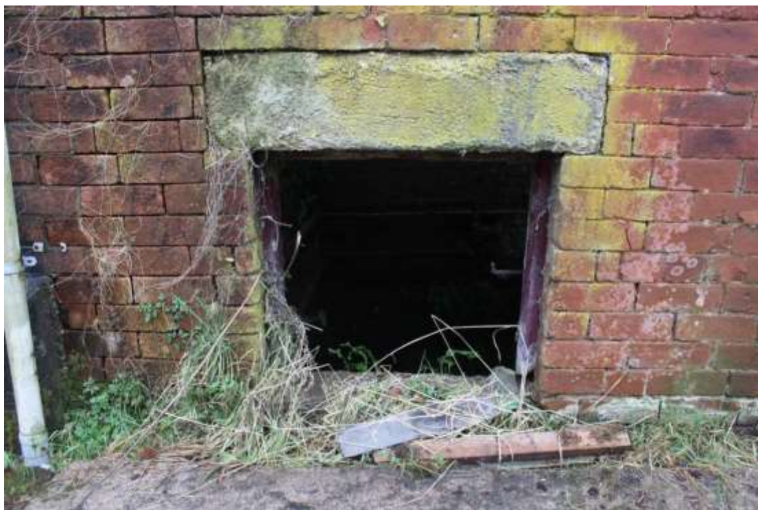
Plate 104: Detailed view of the low opening in the eastern side of the northern elevation, facing south.
