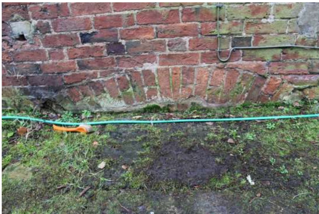
Plate 6: Detailed view of the blocked opening at the base of the northern elevation of the western wing, facing south.
