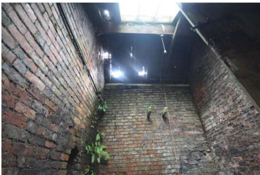
Plate 112: General view of the upper part of the southern interior wall of the eastern 'boiler room' adjacent to the Potting Shed, facing south.
