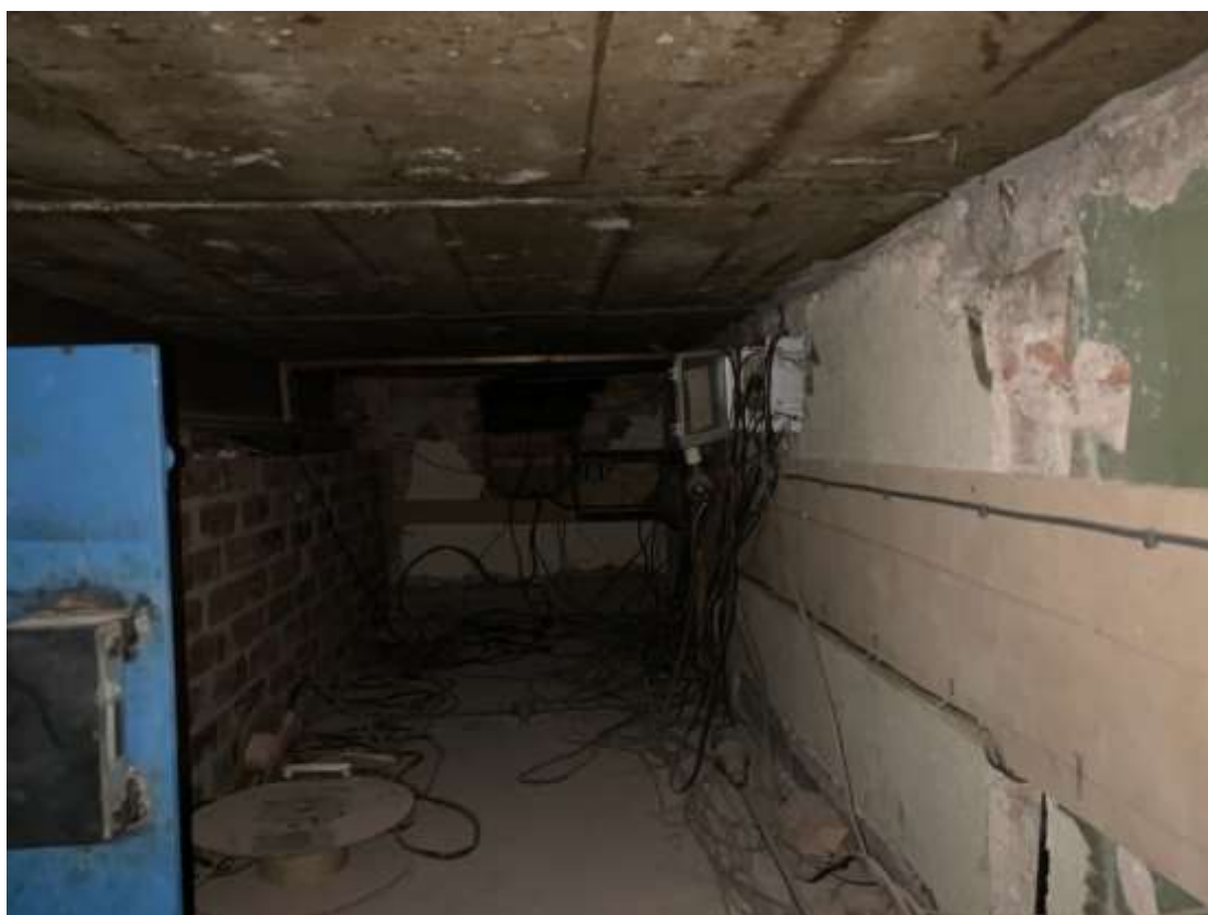
Plate 61: View of the Crawl Space directly underneath Bedroom 1, facing south. The wall on the left side of this photograph is most likely remnants of the original dividing walls in this wing of the hall building.
