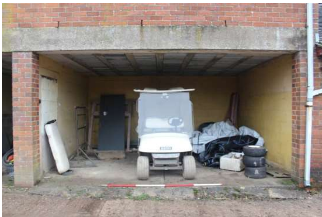
Plate 117: View of one of the open storage areas at the ground floor level of the eastern block of the Gardener's Workshop, facing east.
