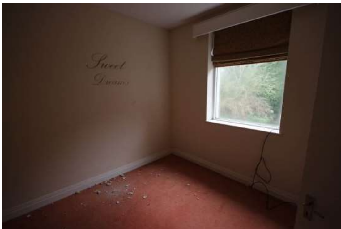
Plate 38: View of the first floor Bedroom in the eastern part of Block A, facing north west.
