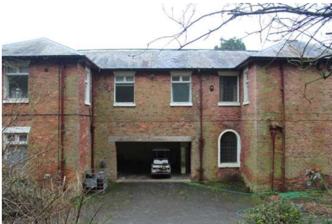
Plate 4: View of the northern elevation of Block A, facing south. Scale 2m. This is what remains of the original late Georgian U-shaped house, with the central northern elevation flanked by the eastern and western wings.
