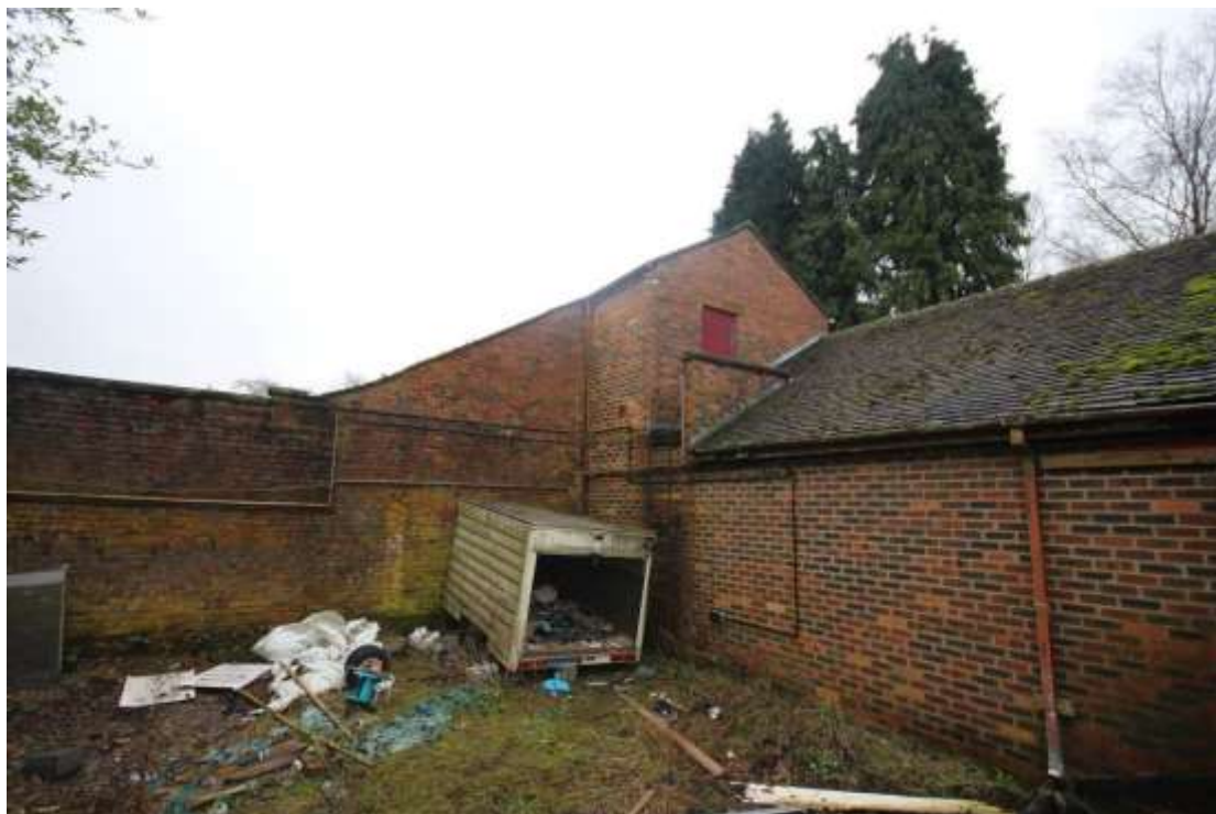
Plate 95: View of the north western extent of the Halcyon Room, facing south east. This is part of the late 1960s/early 1970s construction.
