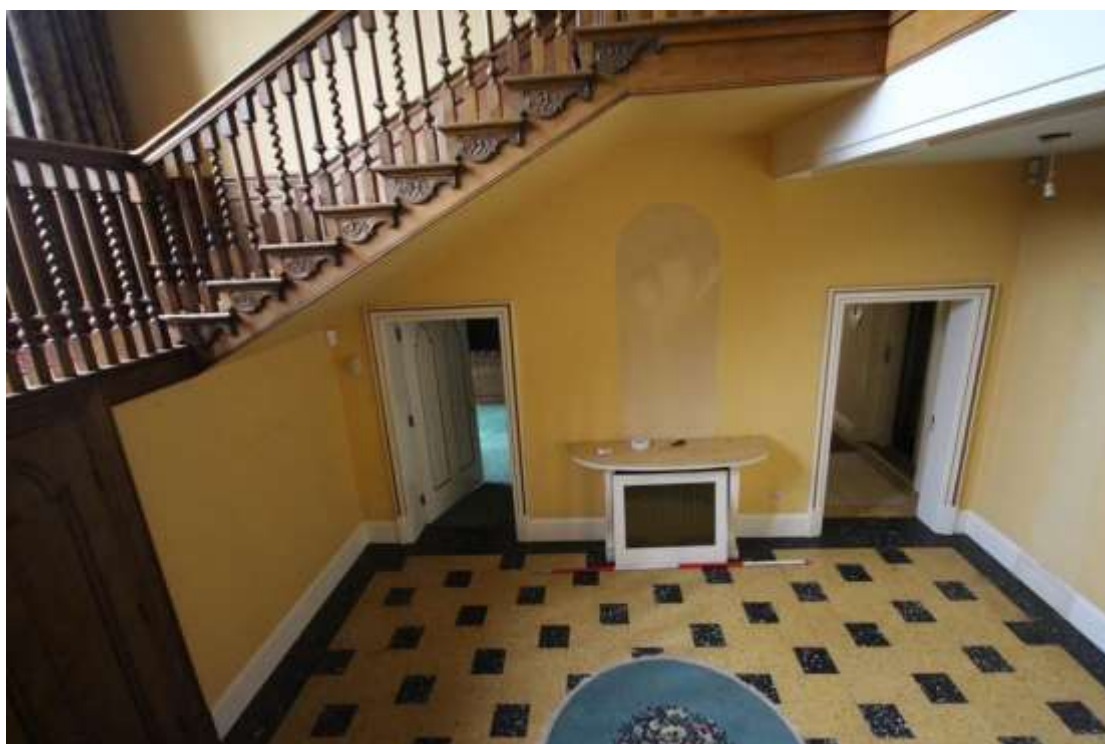
Plate 40: View of the northern elevation of the Reception Hall in Block B, facing north. Scale 2m.
