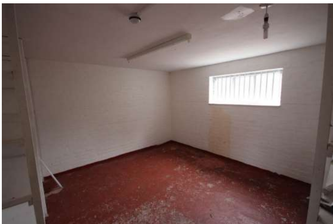
Plate 100: View of the north eastern room in the Halcyon Room, facing north east. This forms part of the modern extension that is to the north of the Coachman's Halt.
