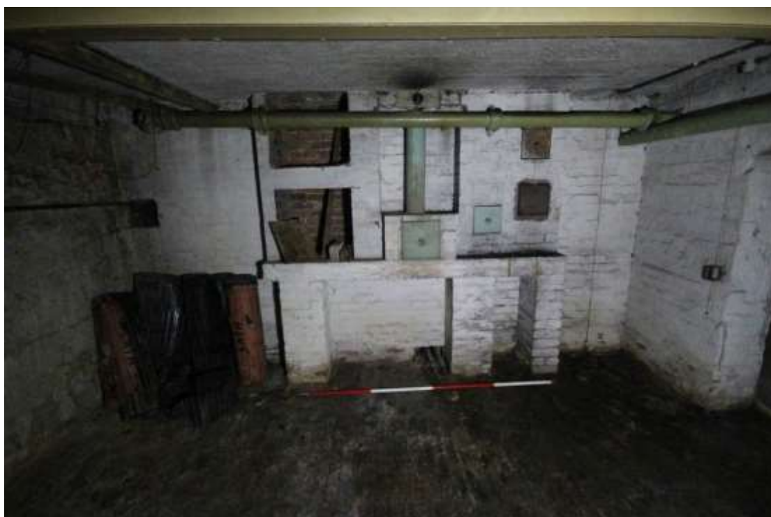
Plate 89: View of the northern elevation in the southern Store room, facing north. Scale 2m. These hatches are likely ash boxes, linked to the flue network.
