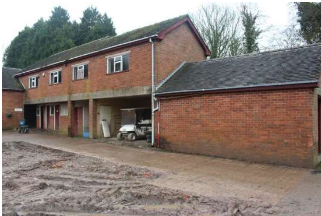
Plate 116: View of the western elevation of the eastern block of the Gardener's Workshop, facing north east.
