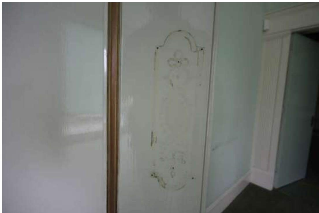
Plate 49: Detailed view of the shadow of the former handle plate on the doorway between the Dining Room and Drawing Room in Block B.
