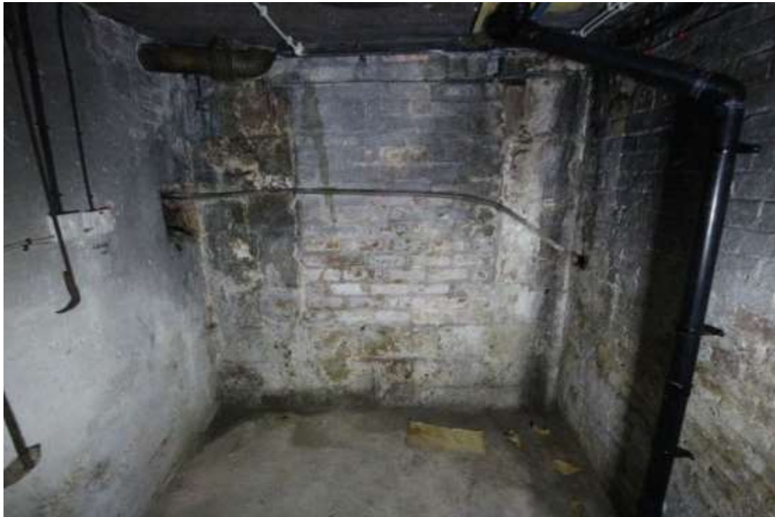
Plate 84: View of the western wall containing the blocked feature in the Boiler Room, facing west.
