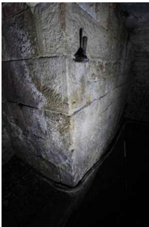
Plate 76: Detailed view of the iron pintel visible in the northern elevation of the north Store, facing north east.
