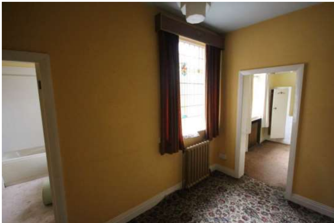
Plate 34: View of the Hallway in the western part of the first floor of Block A, facing north east.
