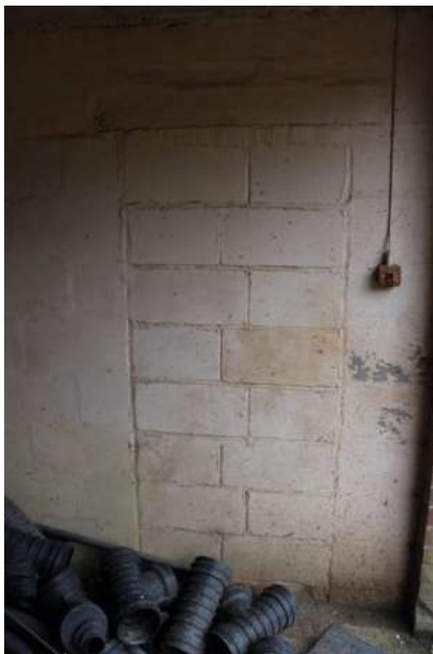
Plate 118: Detailed view of one of the ground floor blocked doorways in the eastern block of the Gardener's Workshop, facing south.
