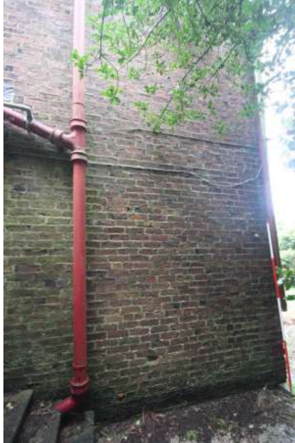
Plate 128: View of the southern elevation of the Coachman's Halt, facing north east. Scale 2m.
