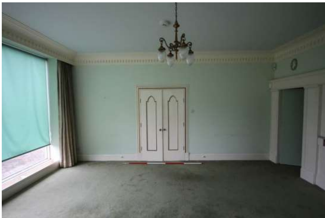
Plate 51: View of the west elevation of the Dining Room, facing north. Scale 2m.
