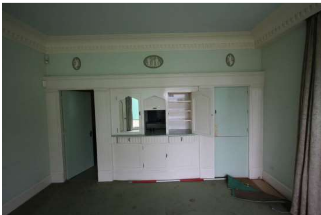
Plate 50: View of north elevation of the Dining Room, facing north. Scale 2m.
