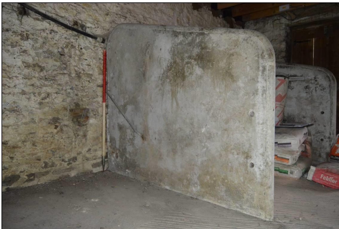
Plate 28: Concrete stall partition and additional features. Note the halter bar and remnants of a cow drinker (facing east).
