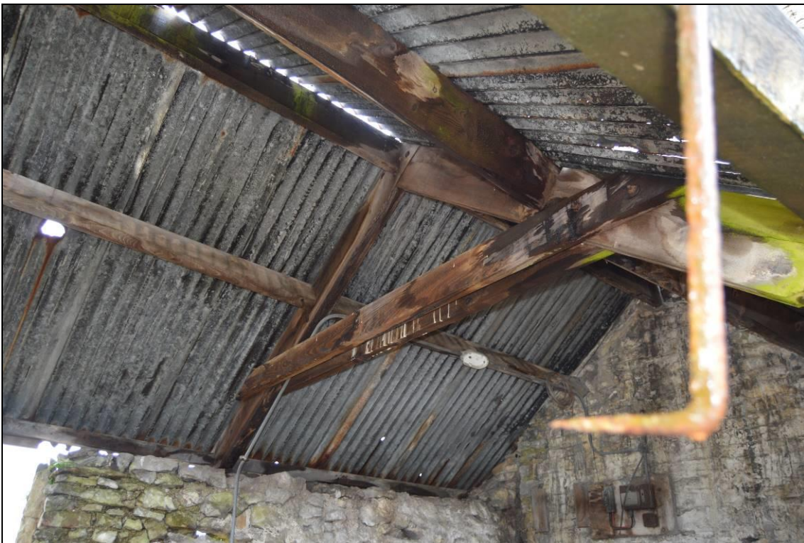
Plate 44: Building 2 roof structure with single tied truss. Note the iron bracket to the foreground which supported the wall plate. Scale 2m.
