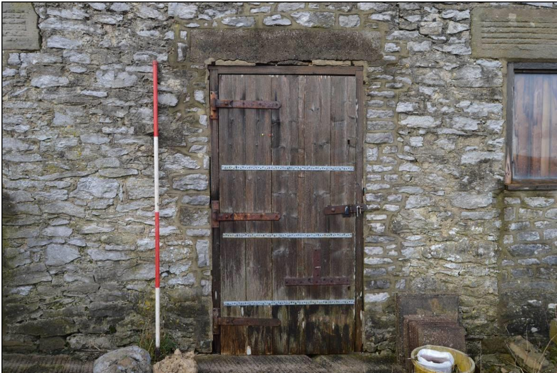
Plate 17: Five of the cow-house apertures to the north elevation of the granary range (facing north west). Scale 2m.
