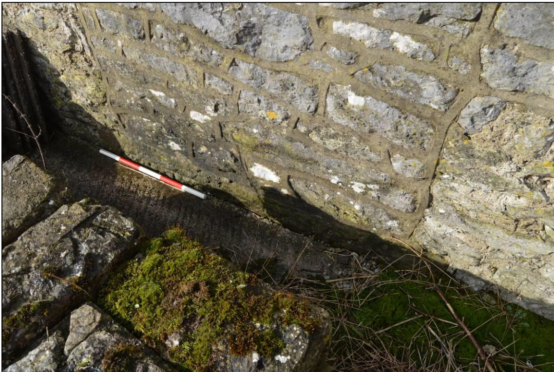
Plate 16: Moulded stone step to the south elevation two original apertures to the north elevation of the granary range. Scale 2m.
