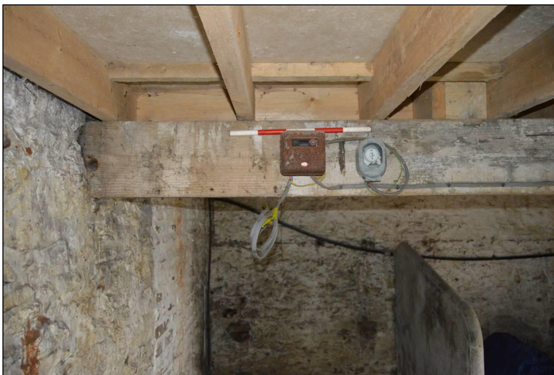
Plate 29: Electrical fittings to interior of building 1 (facing east). Scale 05m.
