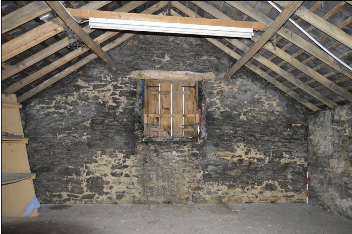
Plate 33: Interior of the west elevation of the barn (facing west). Scale 0.5m.
