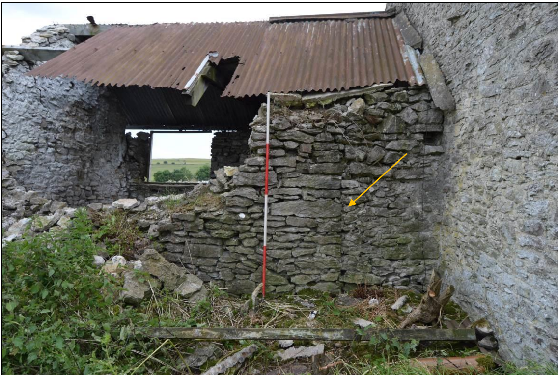
Plate 38: The collapsed north elevation of building 2 (facing south). A vertical break is evident to the right (indicated). Scale 2m.
