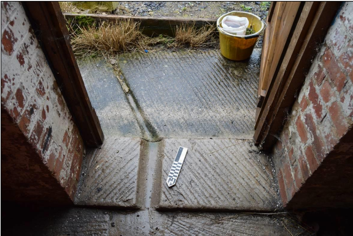
Plate 27: Concrete step with drain to ground floor of building 1 (facing south). Scale 0.2m.
