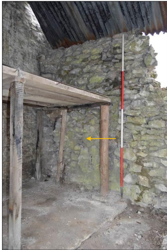
Plate 39: Interior of building 2 with construction break (indicated) adjoining possible wall core to right (facing north west). Scale 2m.
