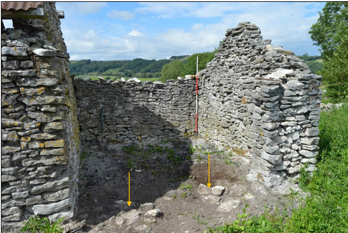
Plate 47: View from the yard into building 3 with foundations (indicated) for a south wall with smaller doorway (facing north east). Scale 2m.
