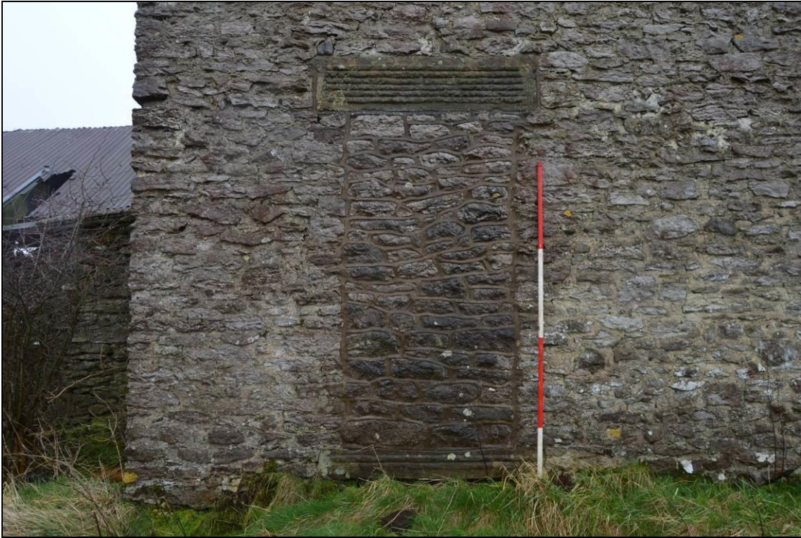
Plate 5: View of the blocked doorway in the north elevation in building 1 facing south. Scale 2m.
