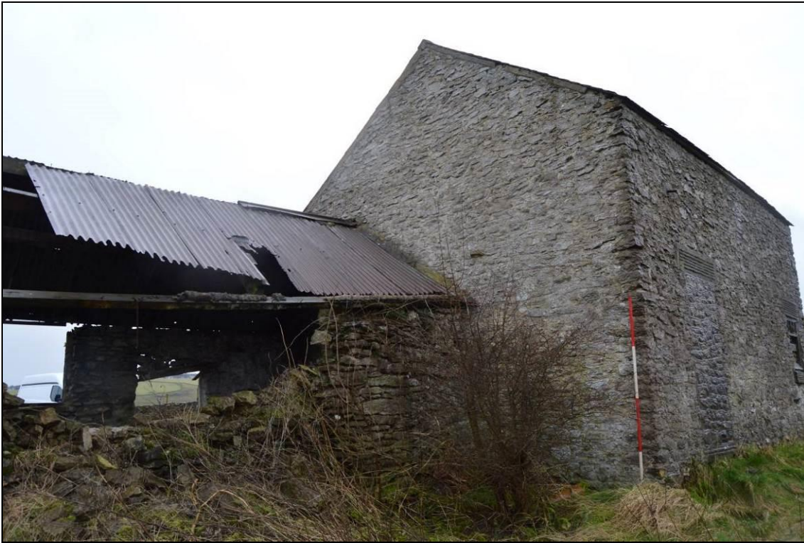
Plate 19: Oblique view of east elevation from the lane (facing south east). Scale 2m.
