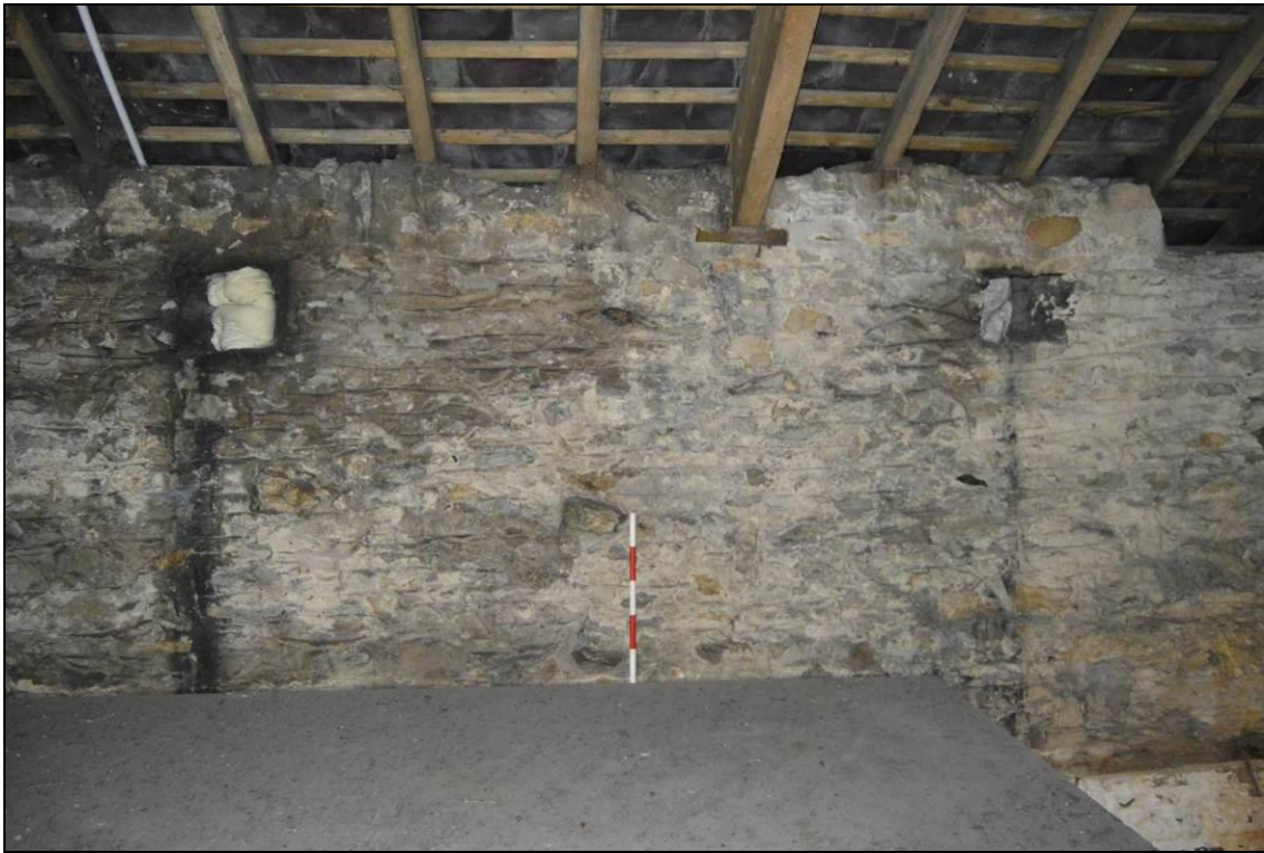
Plate 34: Interior of north elevation, first floor of the barn (facing north) showing the splayed vent openings. Scale 0.5m.
