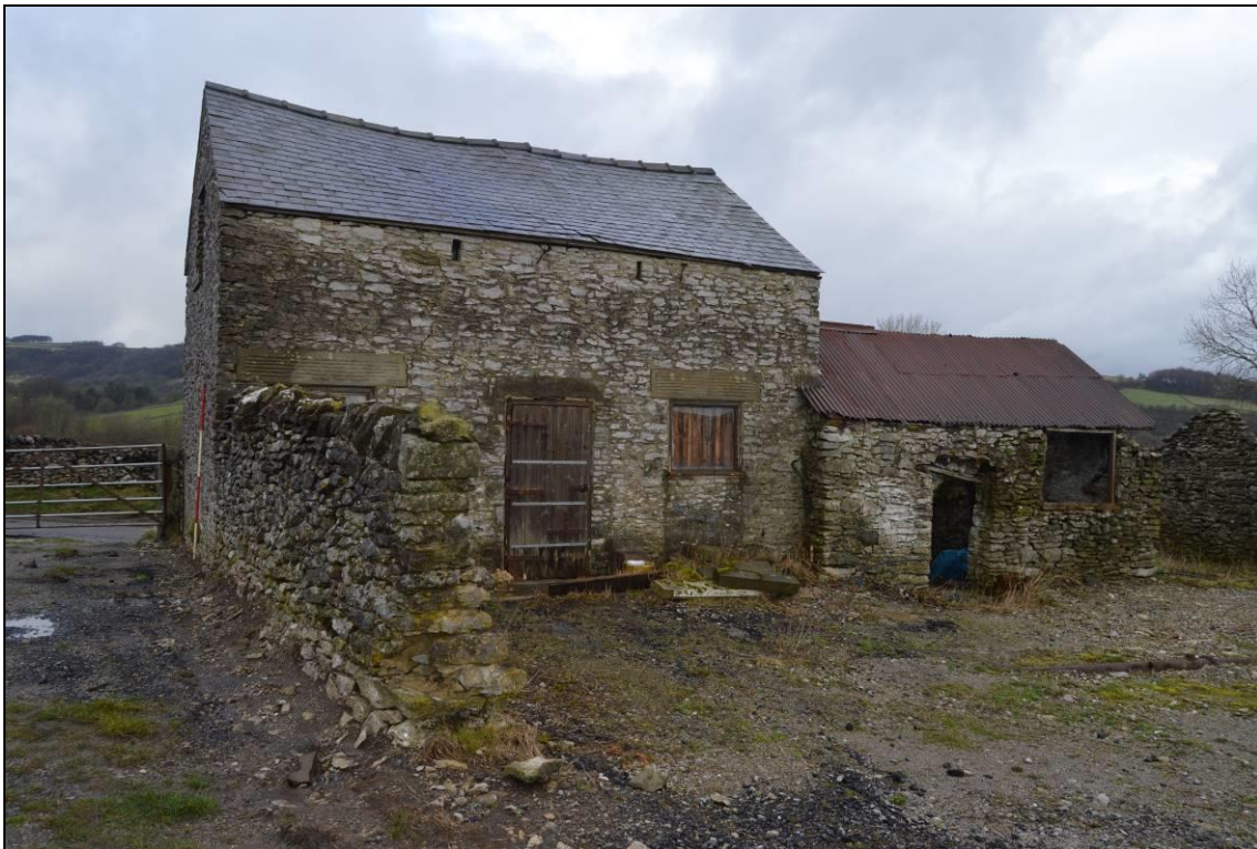
Plate 12: South elevation of building 1, with buildings 2 and 3 to the right (facing north). Scale 2m.
