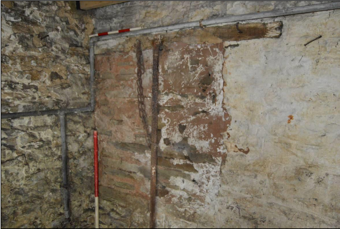
Plate 26: Interior of blocked window to north elevation (facing north west). Scale 1m.
