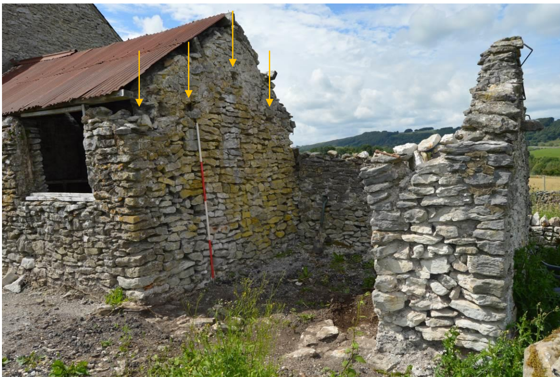
Plate 48: The adjoining gable wall between buildings 2 and 3. Note the sockets (indicated) for the former roof of building 3, with bag-rubbed lime mortar pointing above (facing north west). Scale 2m.
