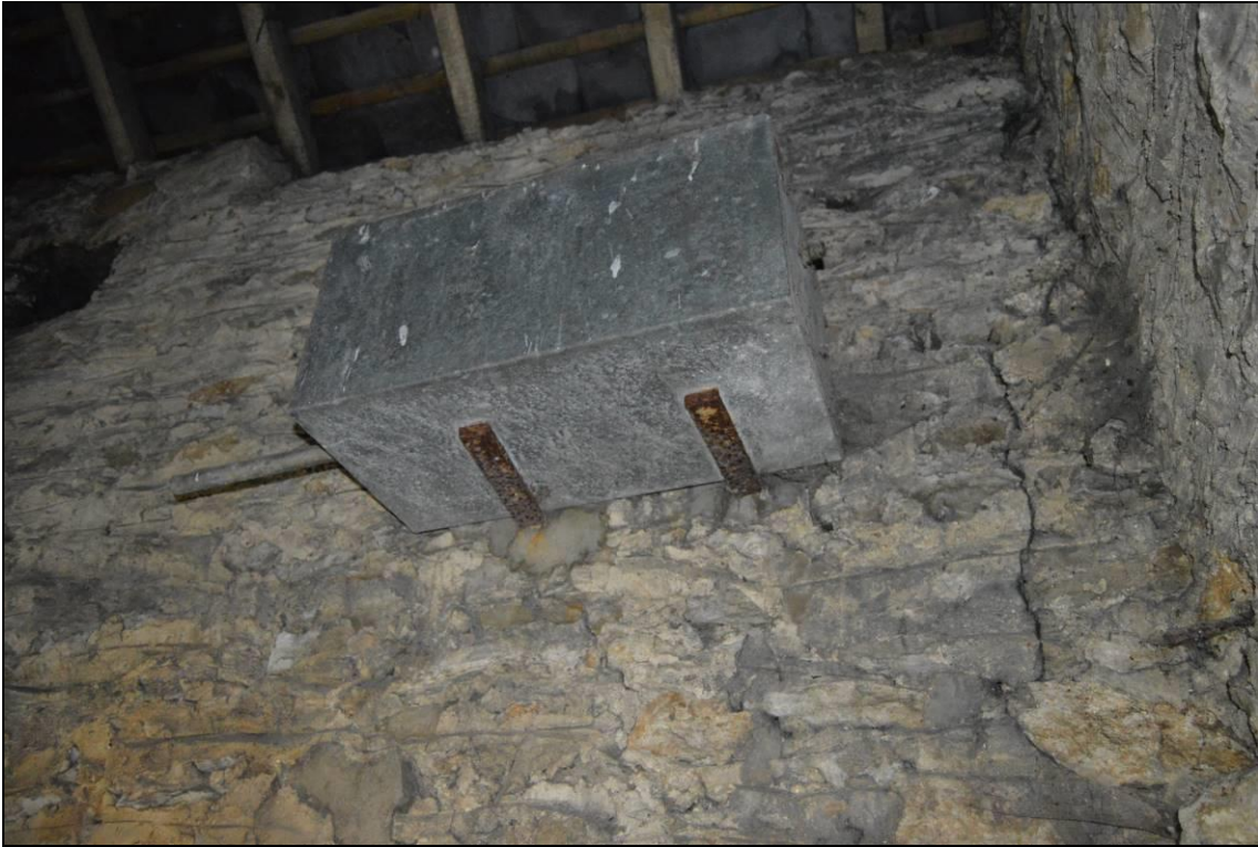
Plate 30: Water tank to interior of building 1 (facing north). Scale 2m.
