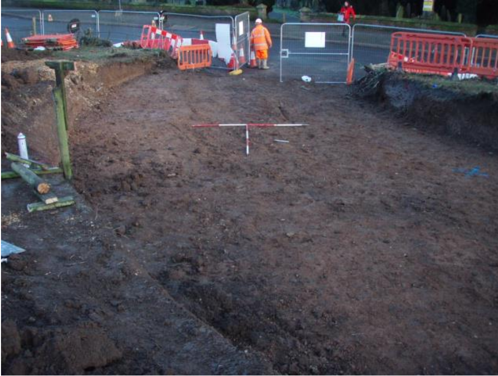
Figure 13: Haul road entrance linking to Mayfield Road/Church Street. View north-east. Scale 2x2m in 0.5m graduations.
