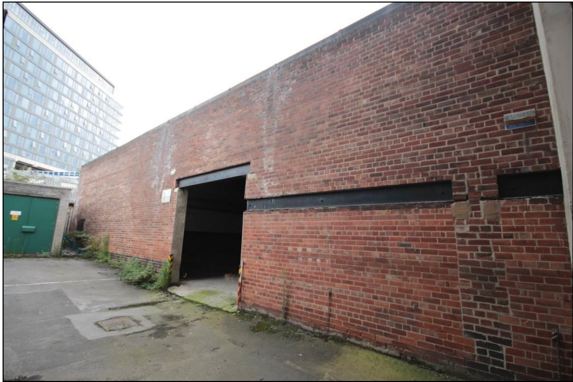
Plate 7: The eastern end of the north western elevation, facing south east. Scale 1m.
