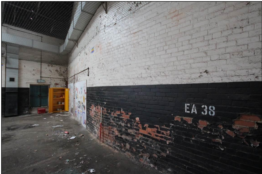
Plate 21: A different view of the north eastern wall showing the curve, facing north. Scale 1m.
