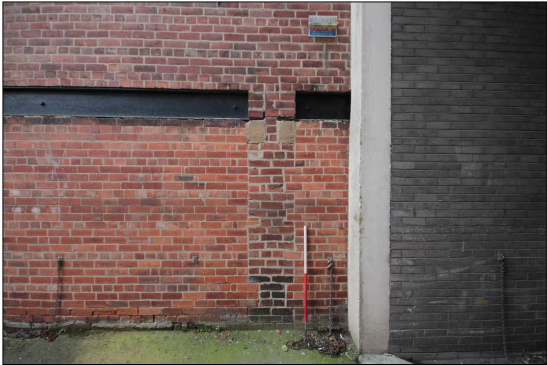
Plate 9: The feature situated to the right of the large goods entrance in the north western elevation, facing south east. Scale 1m.
