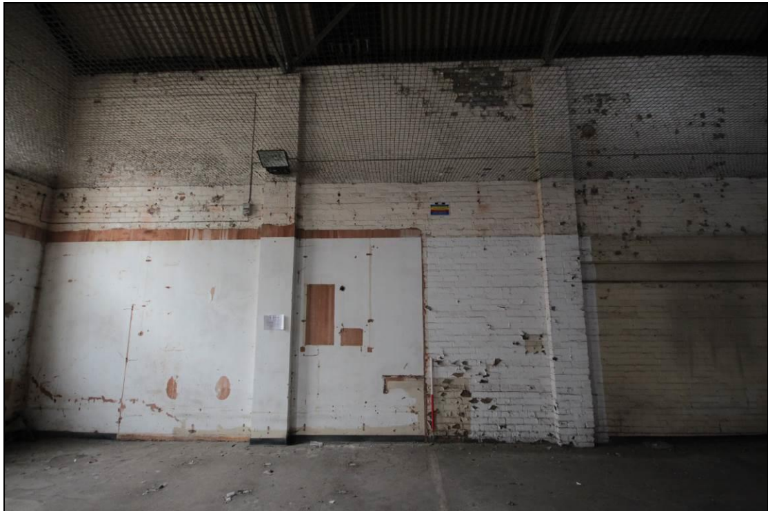
Plate 15: The far western end of the north western internal wall, facing north west. Scale 1m.
