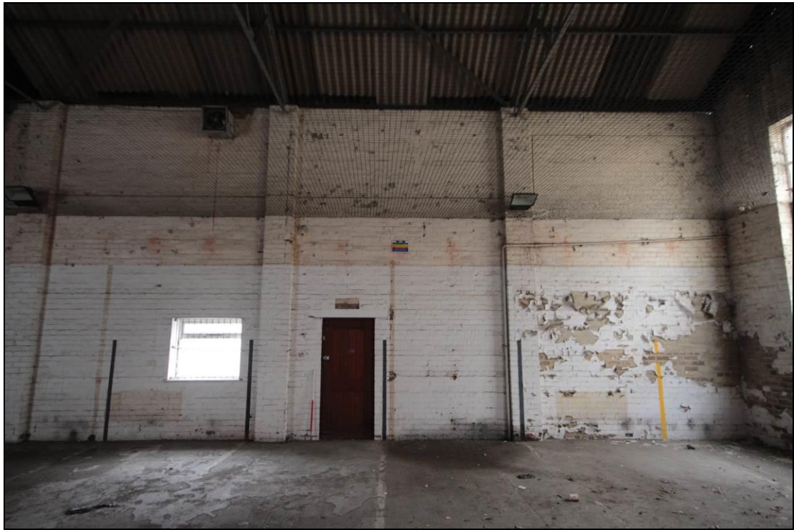
Plate 24: The western end of the south eastern wall, facing south east. Scale 1m.
