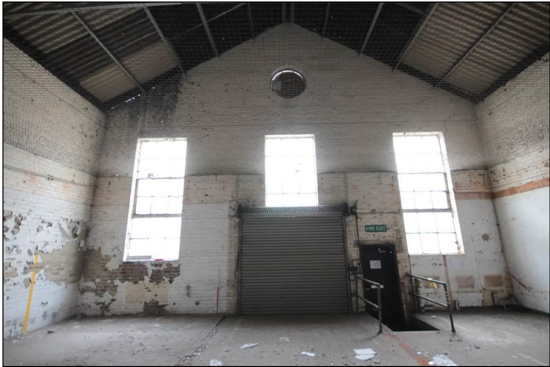
Plate 14: The south western internal wall, facing south west. Scale 1m. Note the brickwork on the floor to the right of this photograph. This may define an earlier access ramp.
