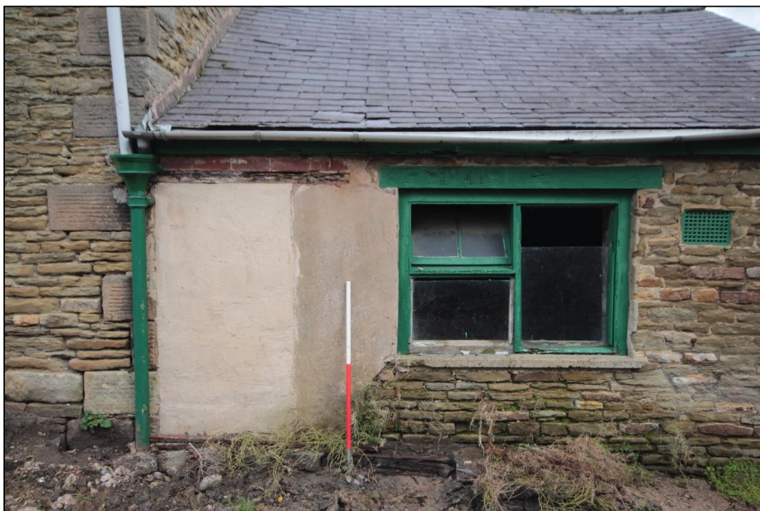
Plate 65: Blocked up doorway on the first extension, with 1m scale.
