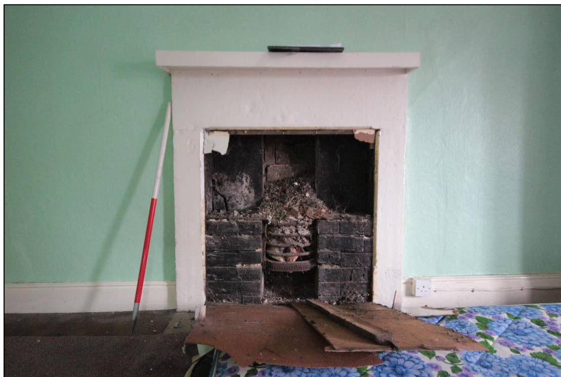
Plate 55: Fireplace in the northern-most bedroom of the farmhouse, taken facing north with 1m scale.
