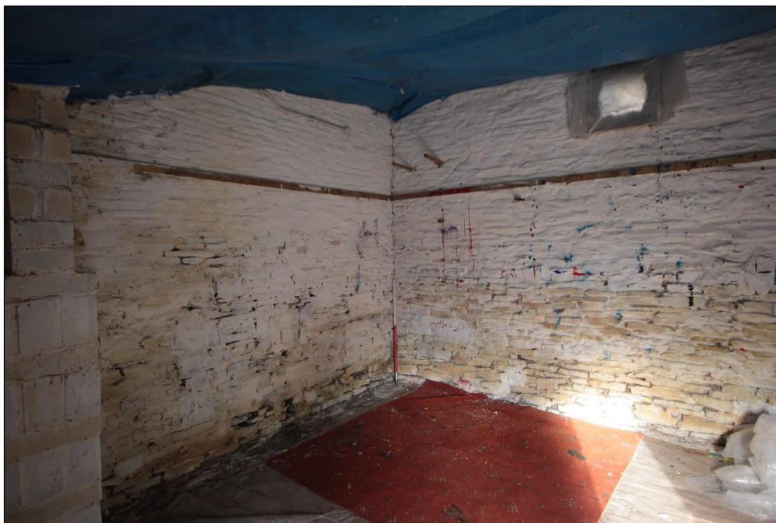
Plate 137: View of the north and west interior walls of the shelter shed extension, with 1m scale.
