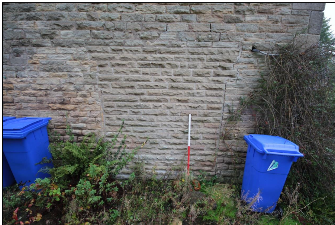
Plate 6: Blocked doorway on the southern facade of the farmhouse, facing north-west, with 1m scale.
