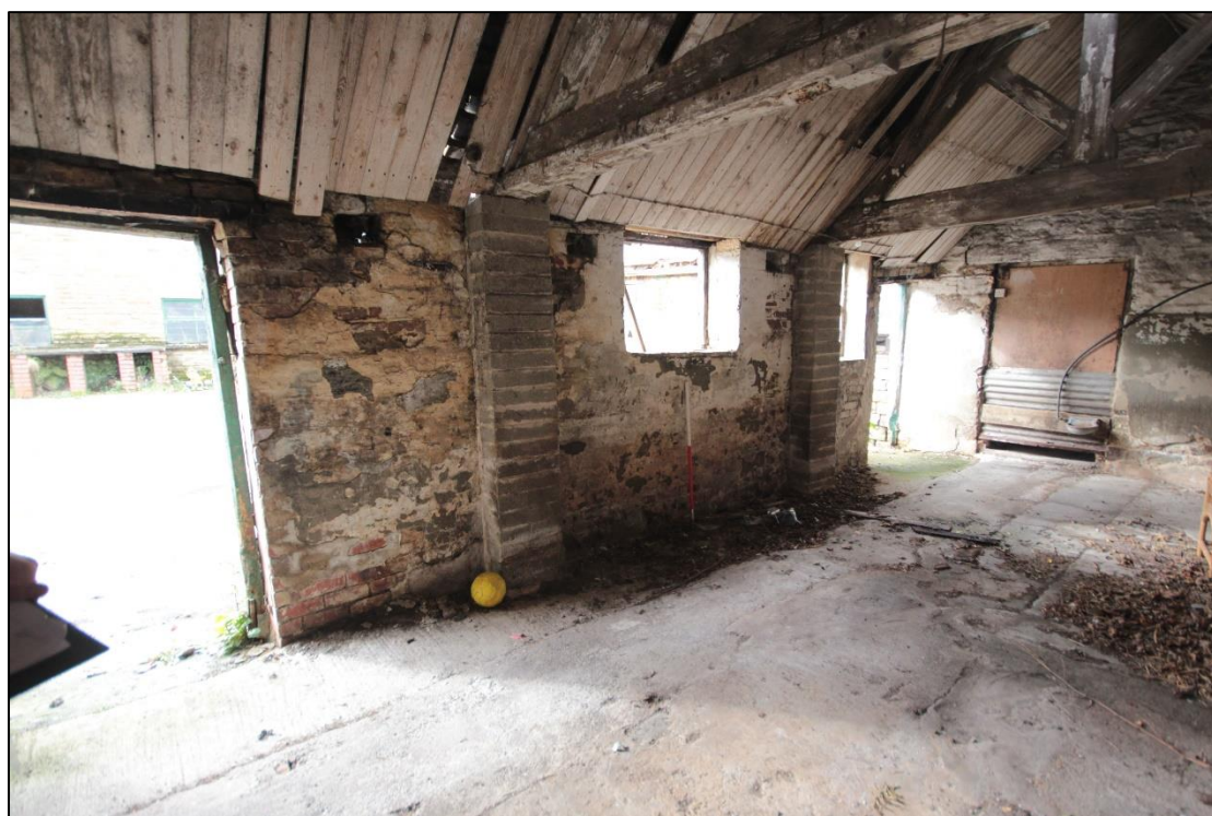
Plate 87: Oblique view of the western wall within the north-east building of the farmyard complex, with twin cinderblock plinths supporting the roof. Taken with 1m scale.
