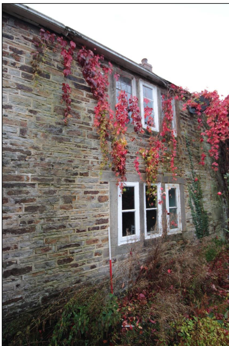
Plate 20: The northern extent of the eastern elevation of the farmhouse. Taken facing west with 1m scale.
