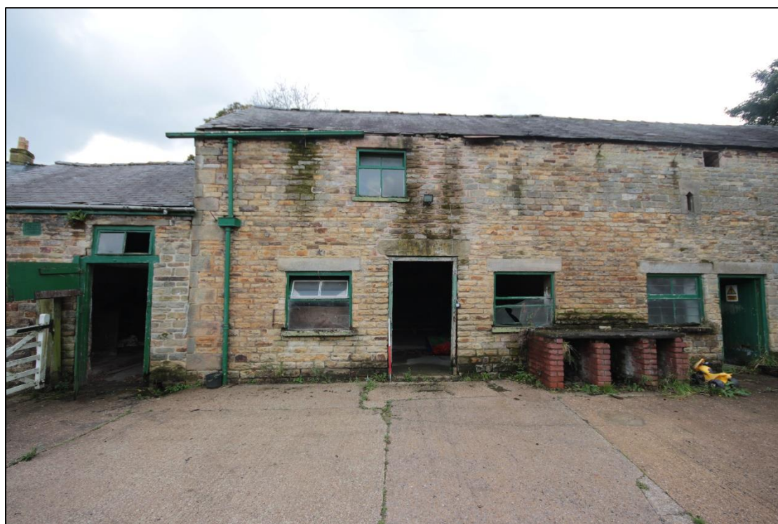
Plate 70: The internal eastern elevation of the western wing's main building, with 1m scale.
