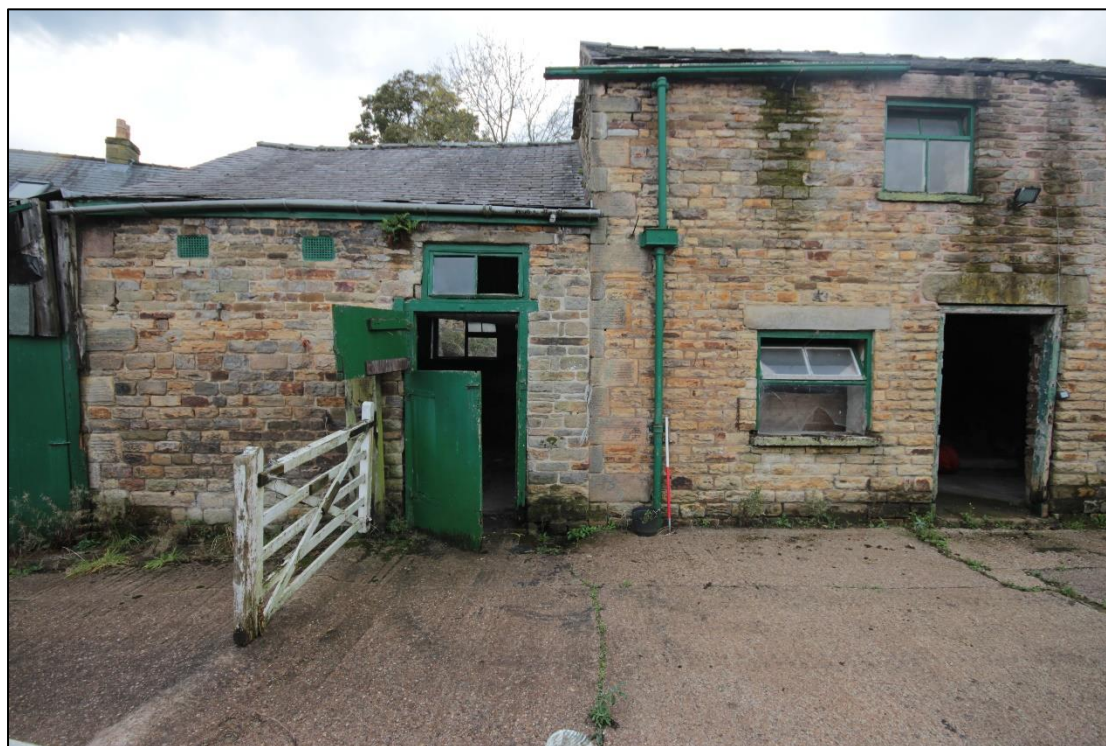
Plate 69: View of the internal eastern elevation, highlighting the extension added to the main western wing building. Taken with 1m scale.
