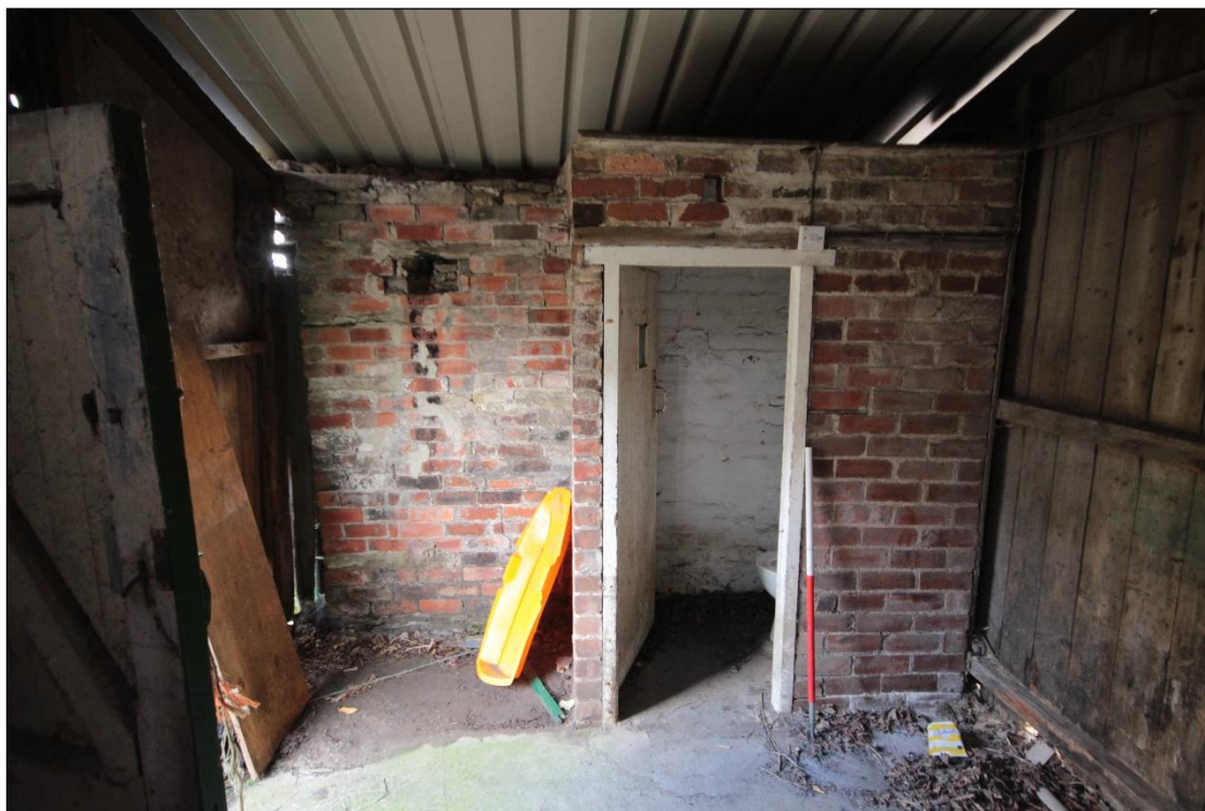
Plate 122: Modern brick built interior extension on the south-east interior of the end extension, with 1m scale.
