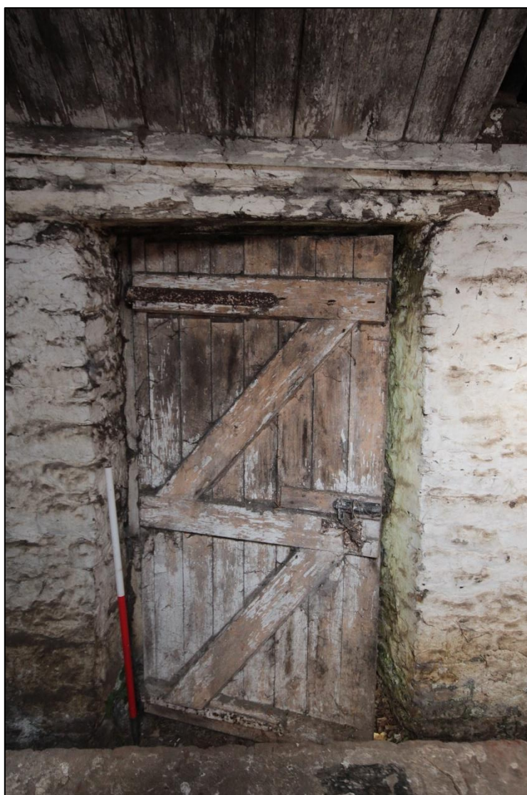
Plate 100: Timber door behind the low brick wall on the northern exterior of the north wing's interior, with 1m scale.
