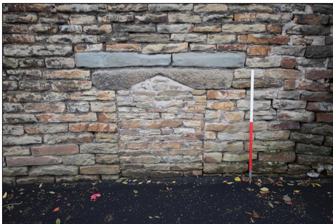
Plate 82: Previous opening on the east elevation from the road, with 1m scale.
