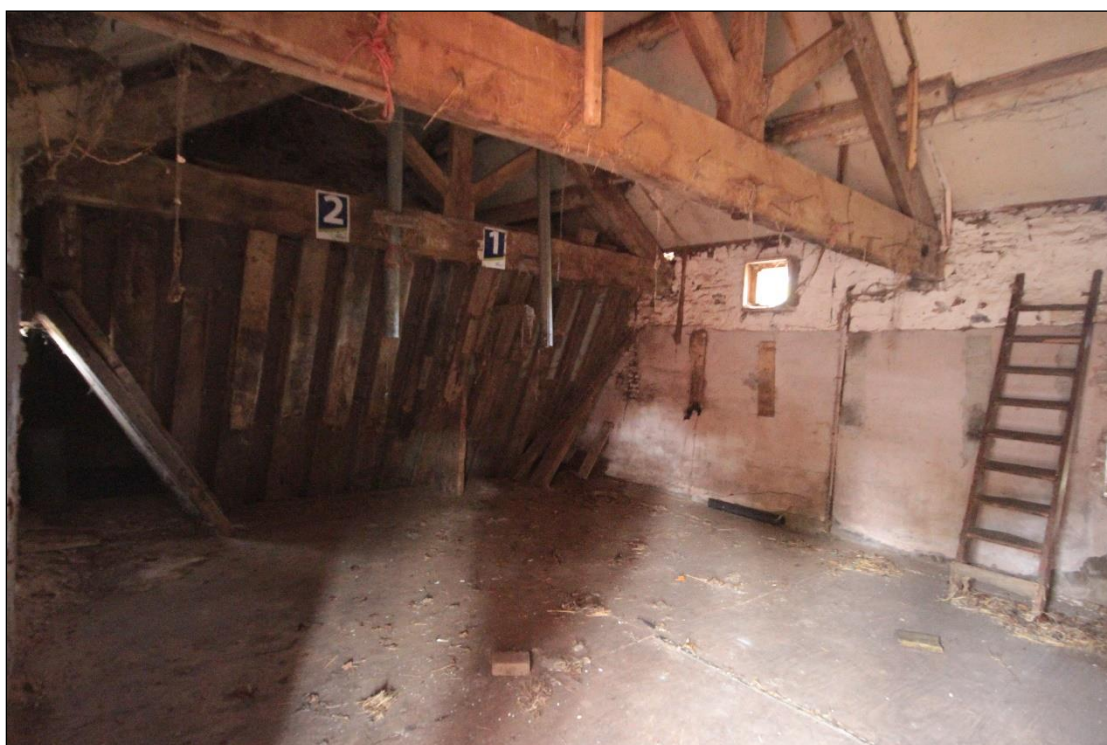
Plate 127: Northern extent of the first floor western room within the western wing, featuring timber apparatus connecting to lower grain chutes.
