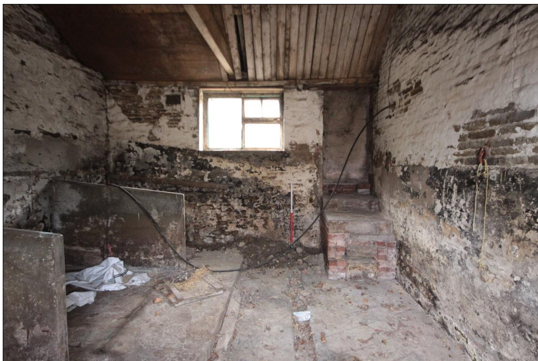
Plate 116: Western wall of the western extension, featuring raised blocked door, with 1m scale.
