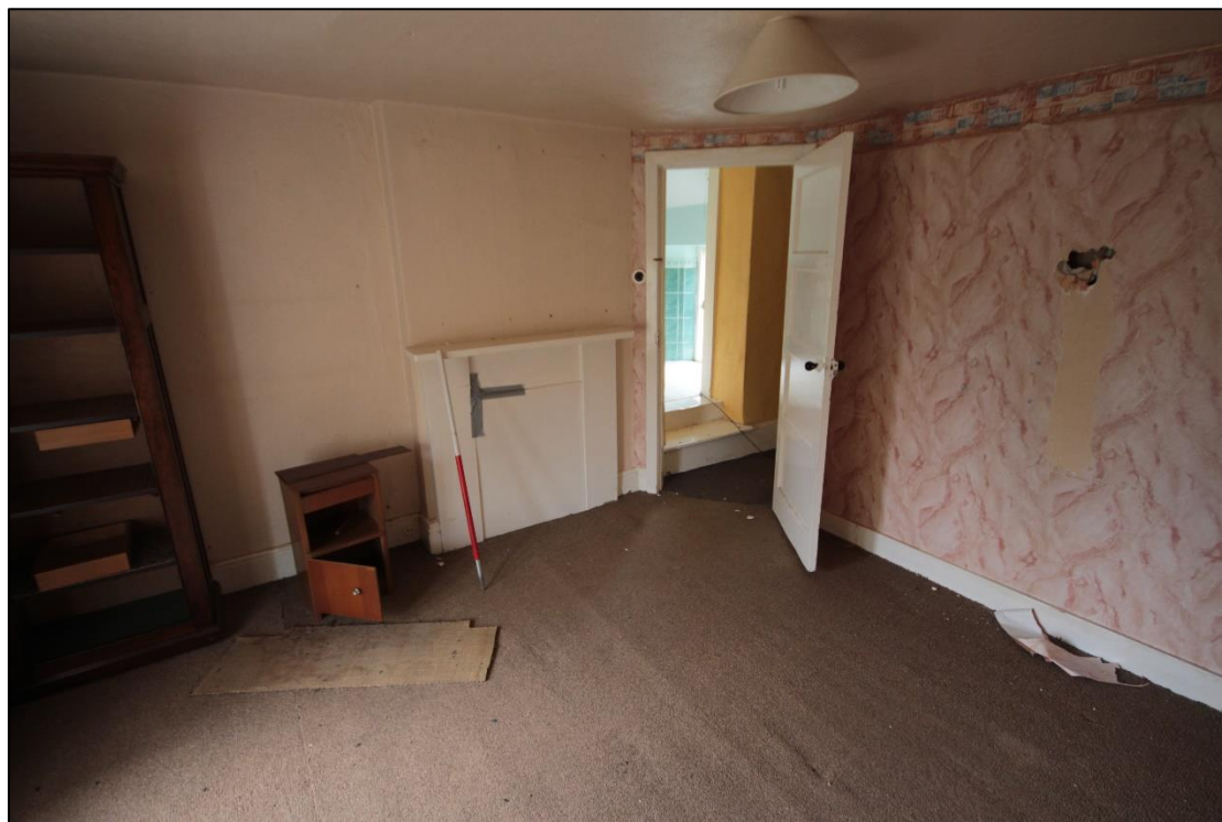
Plate 47: South view of the southern-most bedroom, featuring blocked fireplace, with 1m scale.
