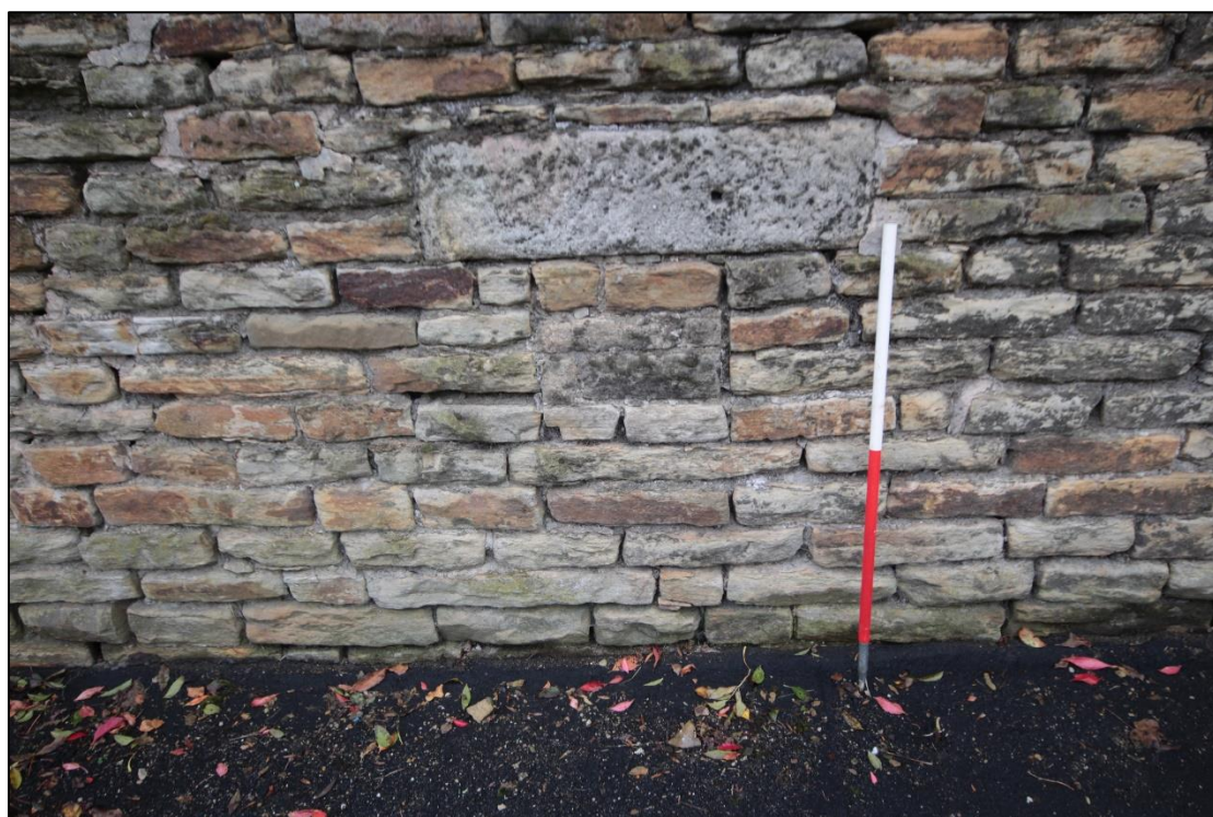
Plate 83: Blocked opening with lintel on the east elevation of the farmyard complex of buildings, with 1m scale.
