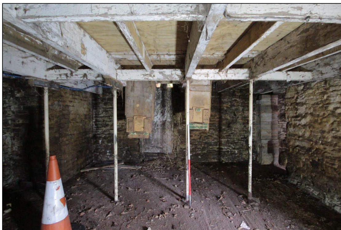
Plate 103: View of the northern wall within the western room of the north wing, with 1m scale.
