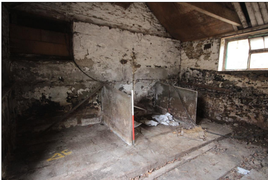
Plate 117: Oblique view of the concrete partitions within the extension on the western wing, with 1m scale.
