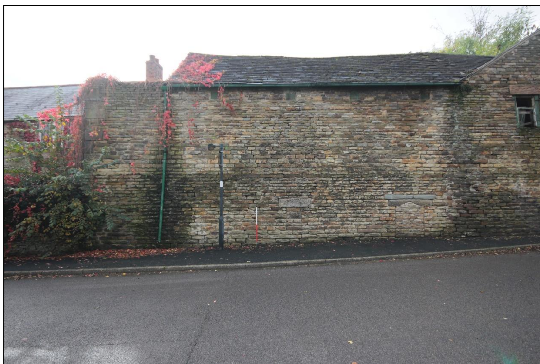
Plate 80: Totley Hall Lane view of the east elevation from the farmyard complex of buildings, with 1m scale.
