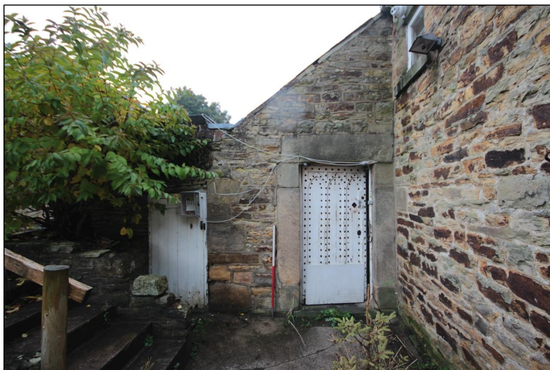
Plate 9: View of the rear entrance to the farmhouse, featuring the decorated timber doorway. Taken facing north-west, with 1m scale.
