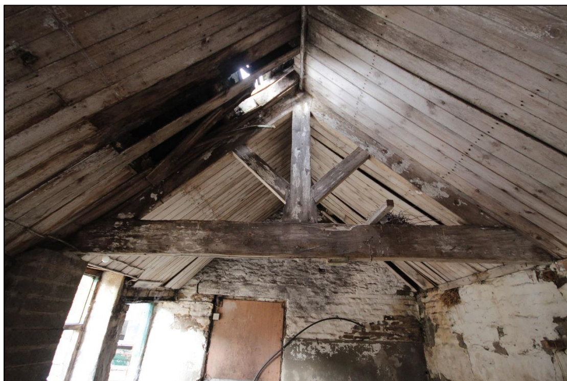
Plate 88: View of the timber framed roof with king post. The roof also features timber panelling.
