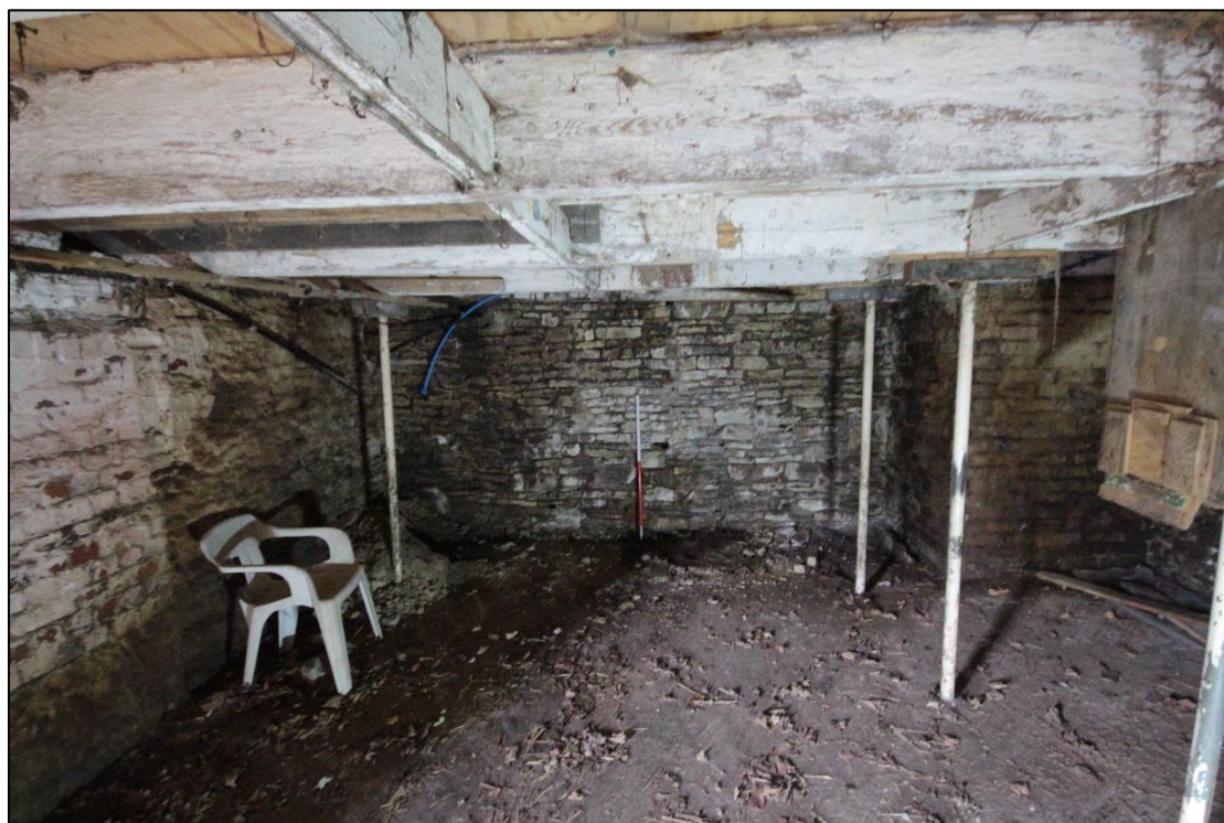
Plate 104: View of the western wall within the western room of the north wing, with 1m scale.
