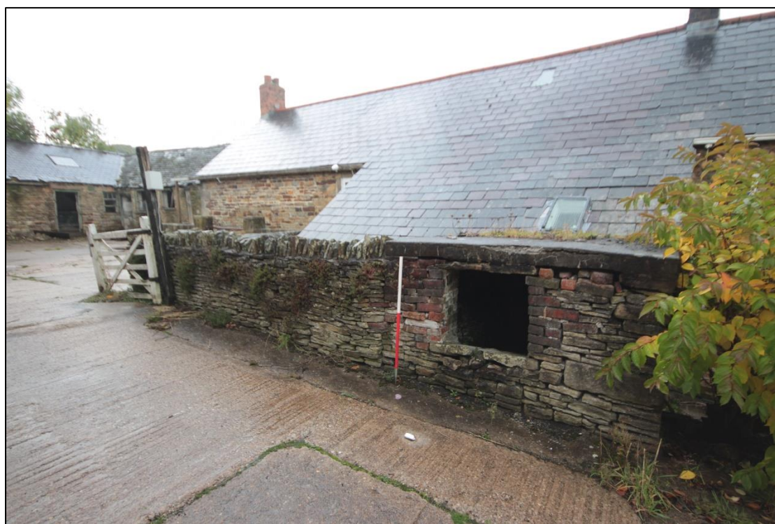
Plate 10: View of the external store on the western elevation, facing north, with 1m scale.
