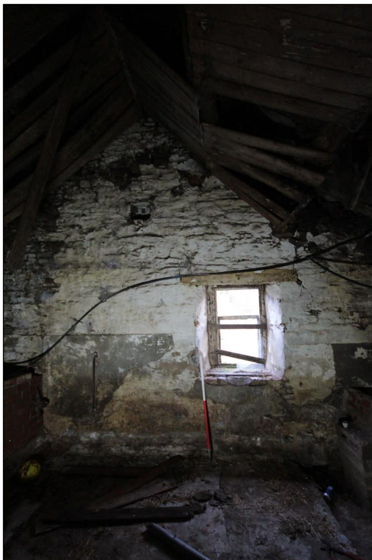
Plate 89: View of the north-east wall within the eastern interior of the north wing, with 1m scale.
