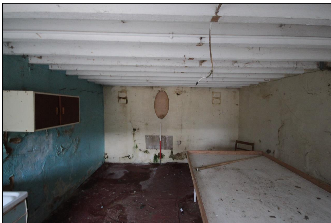
Plate 107: View of the western wall of the plain northern room within the western wing, with 1m scale.
