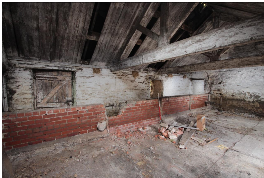
Plate 99: View of the rear wall within the northern wing's interior, with low brick wall. With 1m scale.
