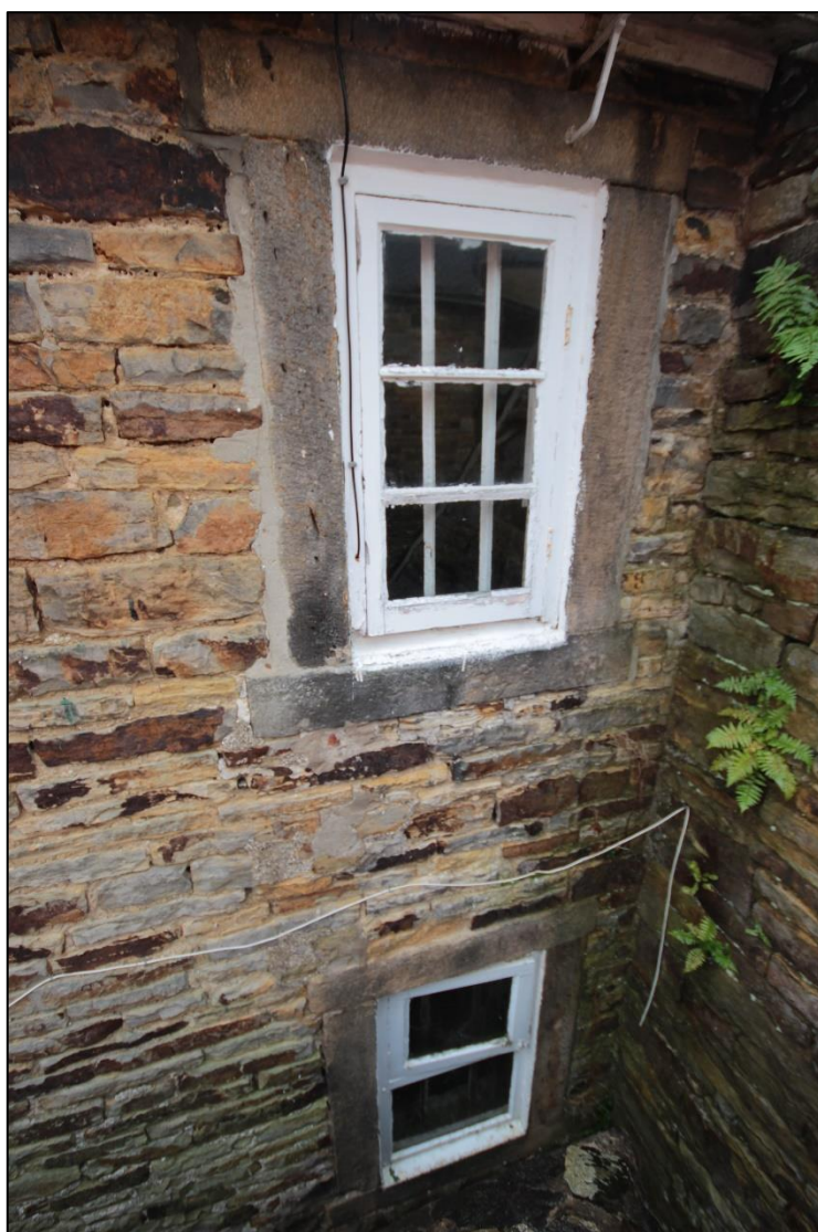
Plate 12: View of the ground floor subterranean window, and first floor window, facing east.
