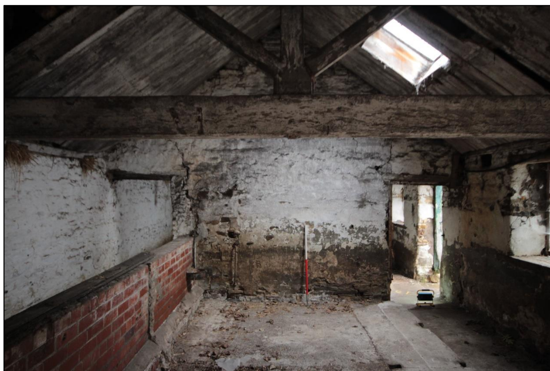
Plate 96: View of the north-east wall within the large central area of the northern wing, with 1m scale.
