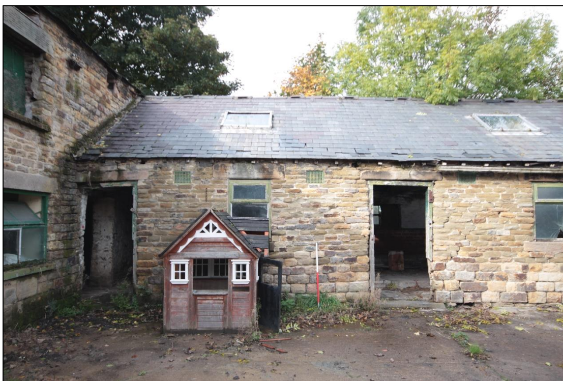
Plate 75: View of the western end of the single storey building within the farm yard, with 1m scale.
