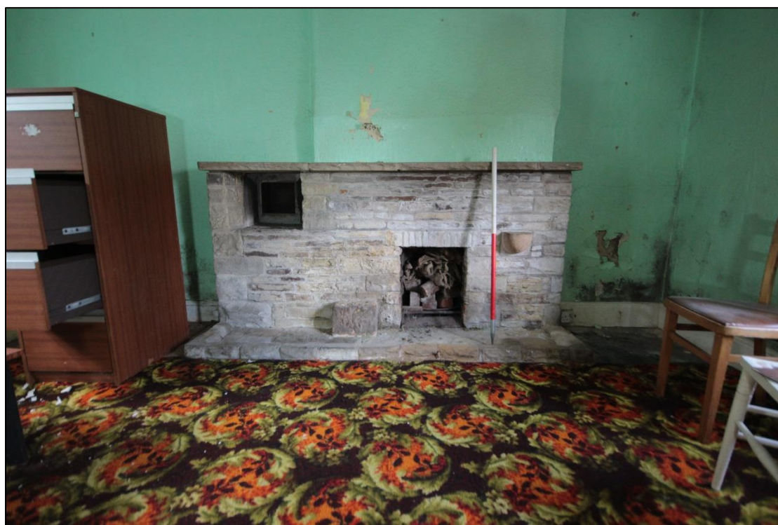
Plate 37: The large fireplace within the living room, facing north with 1m scale.
