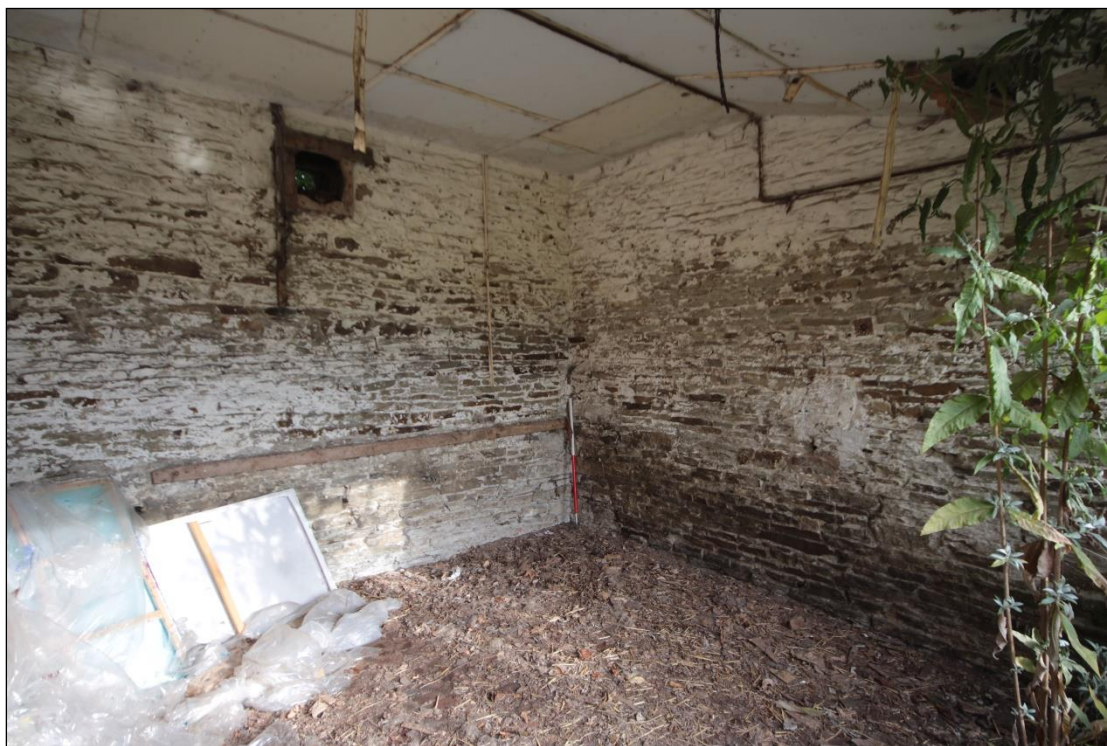
Plate 139: View of the north and east interior wall of the shelter shed extension.
