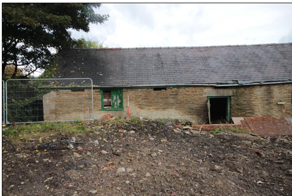
Plate 59: Northern extent of the western farmyard wing, taken facing east with 1m scale.
