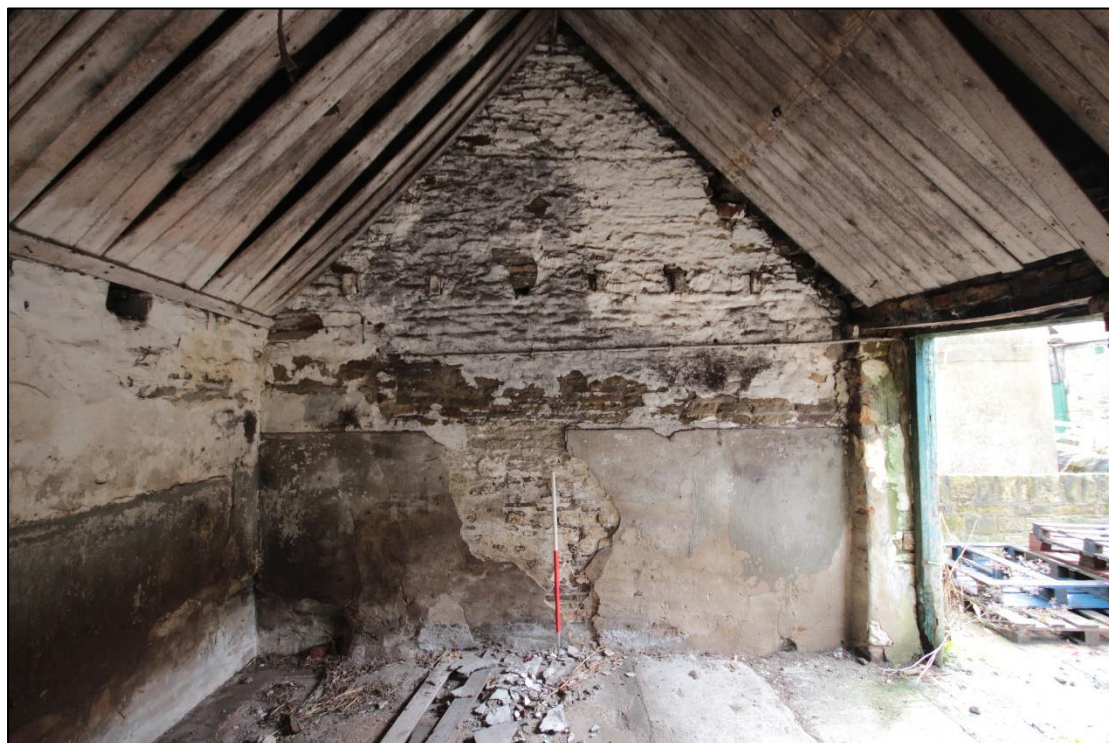
Plate 84: View of the internal wall within the north-east building of the farmyard complex, featuring holes from the previous roof, with 1m scale.
