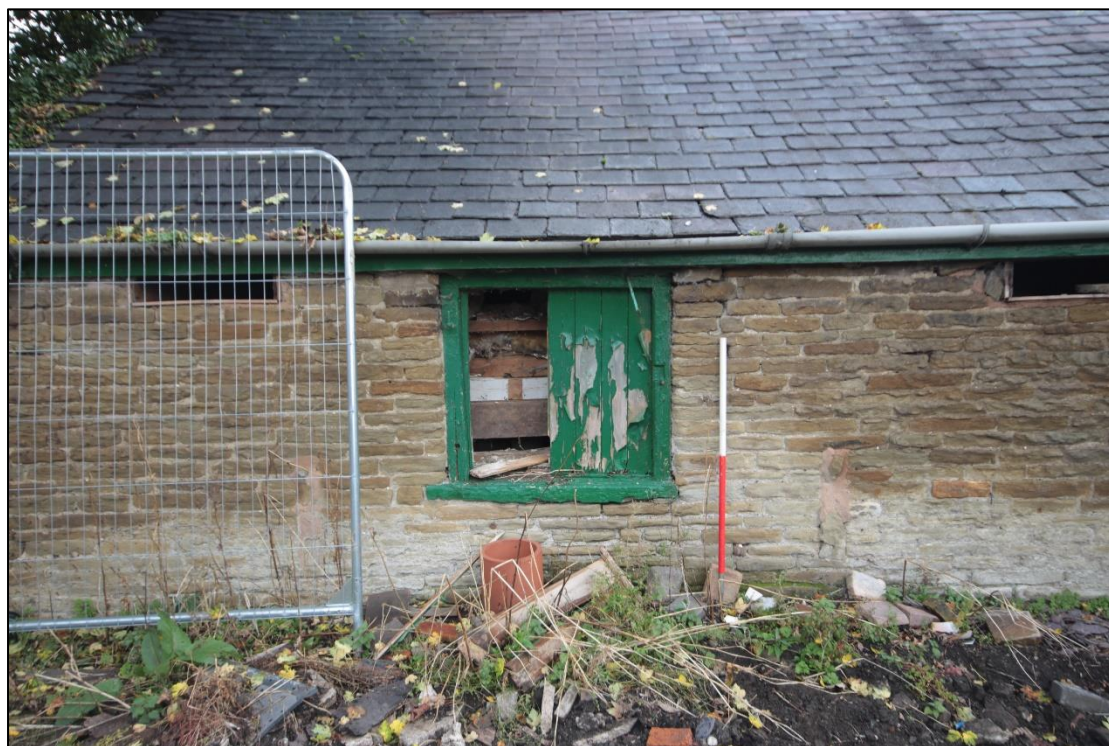
Plate 62: Boarded-up timber opening on the northern extent of western elevation. Taken facing east with 1m scale.
