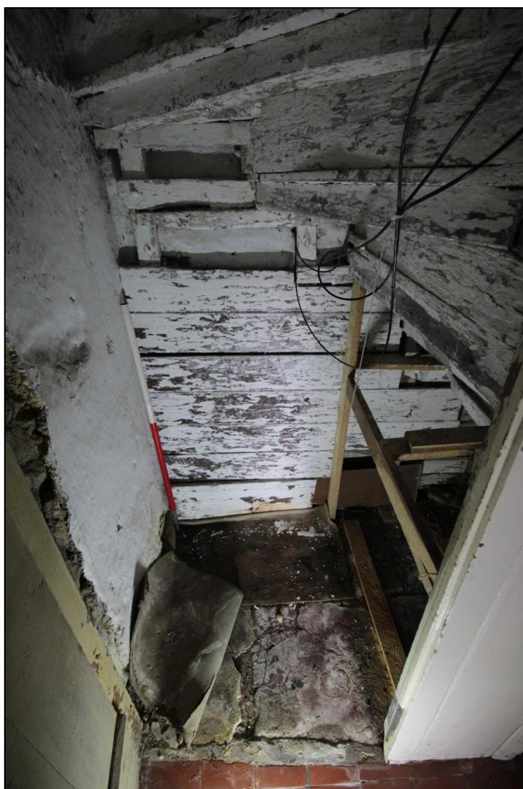
Plate 41: View of under the stairs next to the ground floor landing, with 1m scale.
