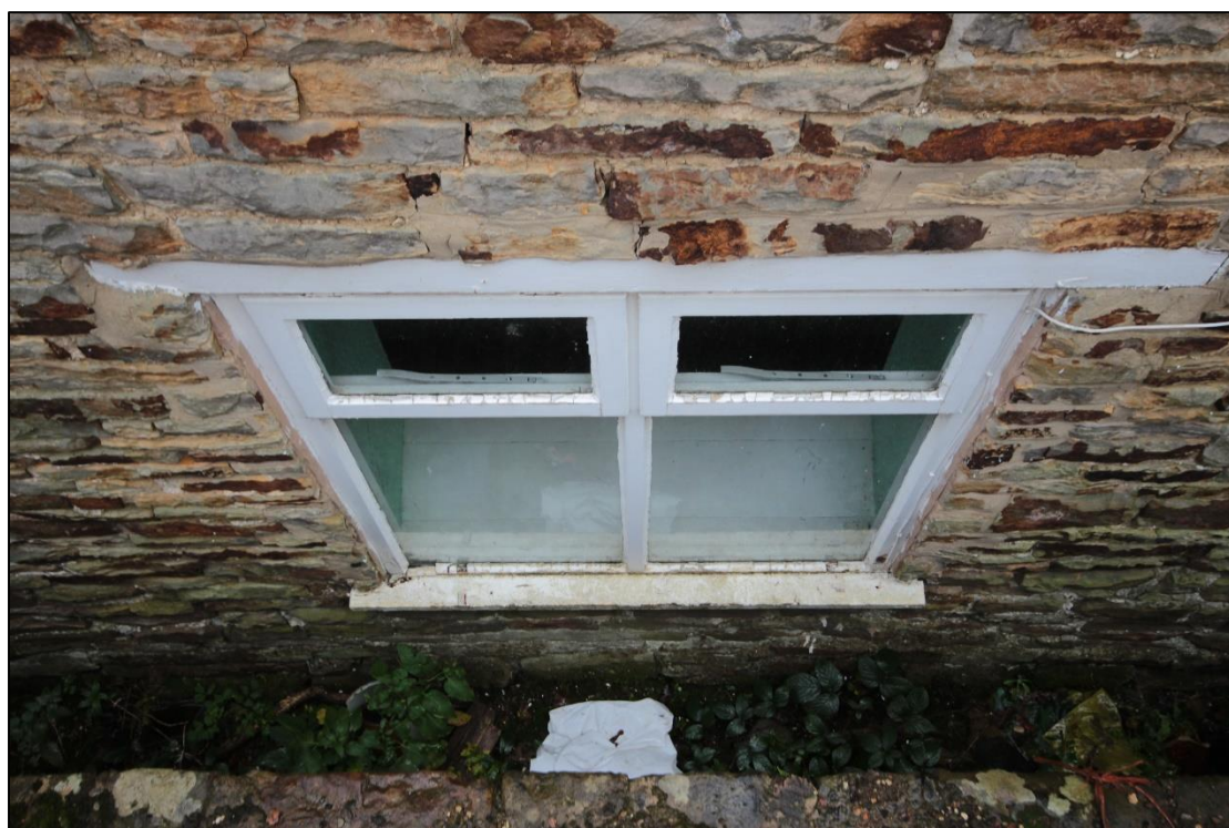
Plate 13: Ground floor modernized window on the western elevation of the farmhouse. Taken facing north-east.
