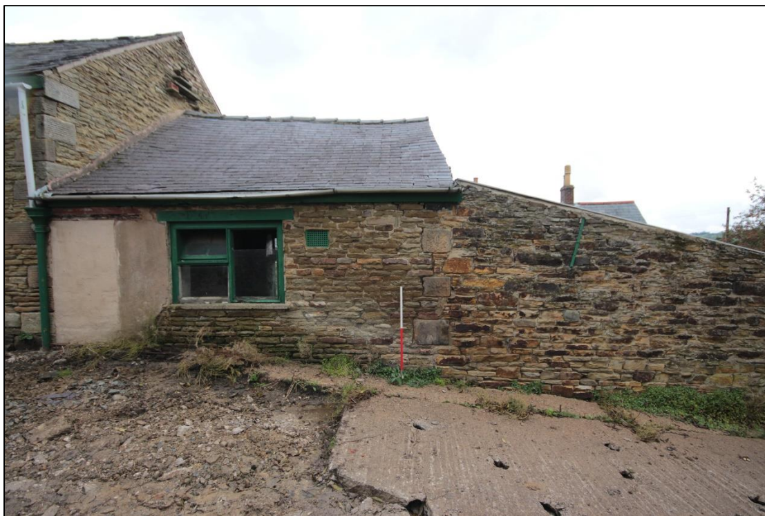
Plate 64: View of the two extensions on the western elevation, taken facing east with 1m scale.
