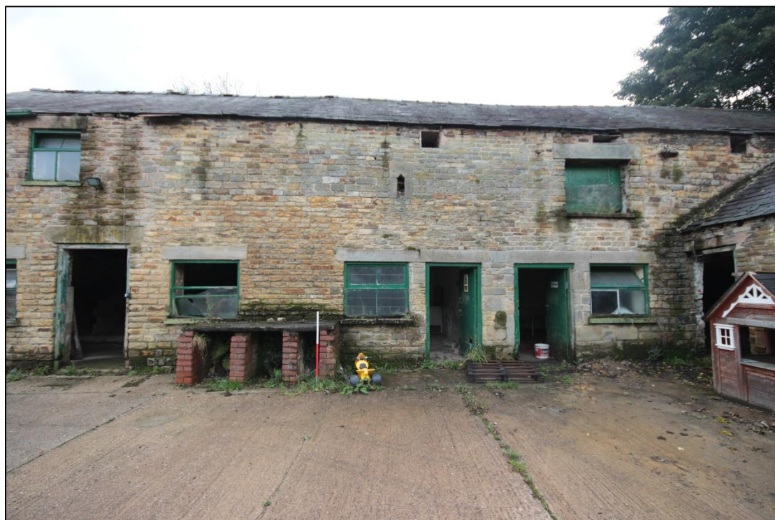
Plate 71: Northern end of the internal eastern elevation of the farmyard complex, featuring pitching hole on the right, and central ventilation slit, with 1m scale.
