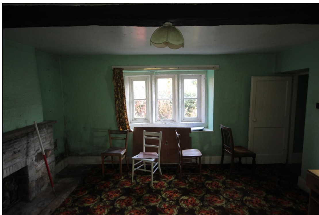
Plate 38: View of the eastern wall of the living room, with 1m scale.
