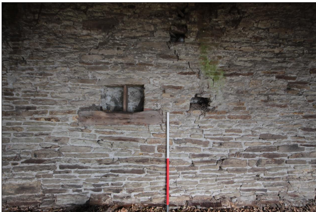
Plate 134: Two previous openings on the north wall of the shelter shed, with 1m scale.
