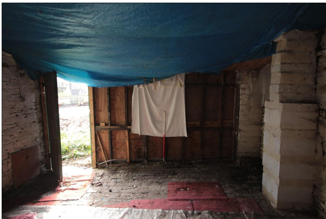
Plate 138: Timber panelled front wall of the shelter shed extension, with 1m scale.
